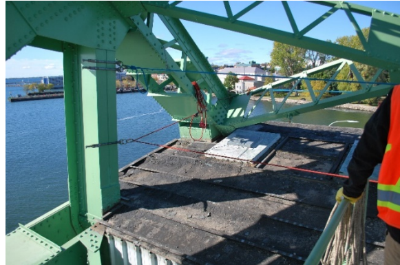
Figure 4-4: Top face covered with roofing material. South half of top face shown.
