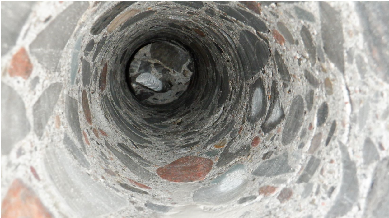
Figure A28 – Core holes C3. Cracking observed along core hole to depths of approximately 385 mm.
