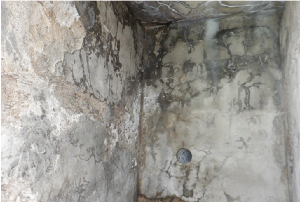
Figure A25 – Condition of concrete inside South compartment on East face. Excessive map cracking on the ceiling of compartment resulting in efflorescence. Core hole is that of C2 taken from the West face which protruded the entire thickness of the counterweight.
