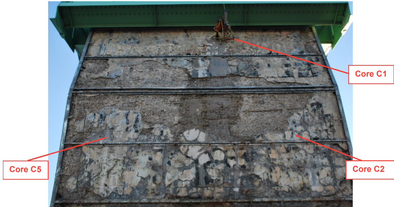
Figure 4-1: West face of Counterweight showing signs of spalling, delamination, and reinforcing corrosion (approximate core locations and areas of spalling and delamination are presented in Appendix C, detailed core locations found in Appendix A)
