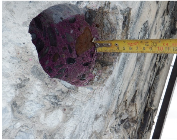
Figure 4-18: Carbonation depth at core location C2
