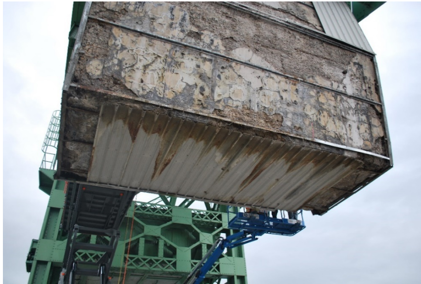
Figure 4-15: Bottom face showing panels removed from North and South ends
