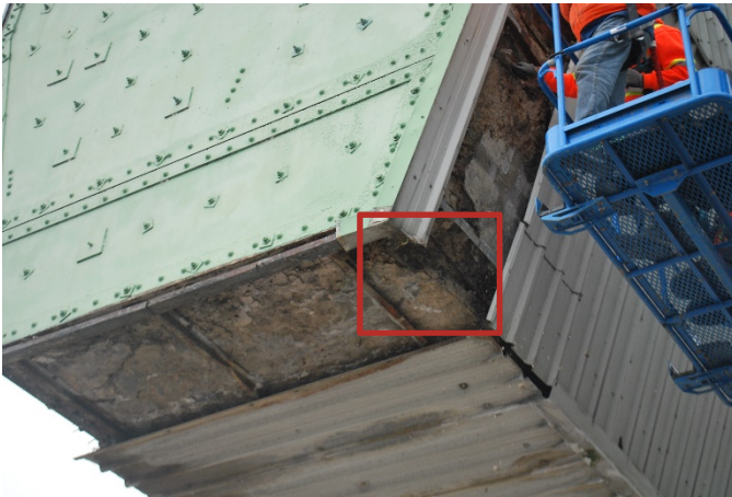
Figure 4-9: Concrete section loss and exposed reinforcing steel showing generalized corrosion of South end of bottom face.
