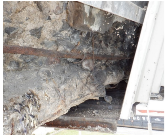
Figure 4-10: Zone indicated by red box in Figure 4-9 (South East corner of bottom South face).
