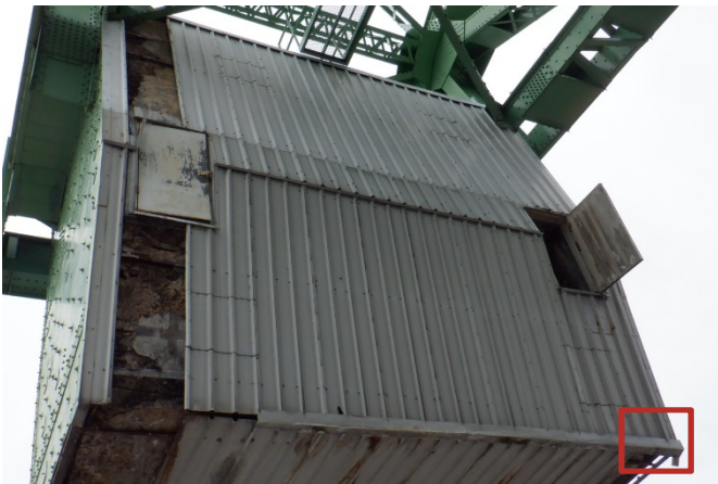
Figure 4-11: Concrete section loss at bottom North East bottom corner of East face.
