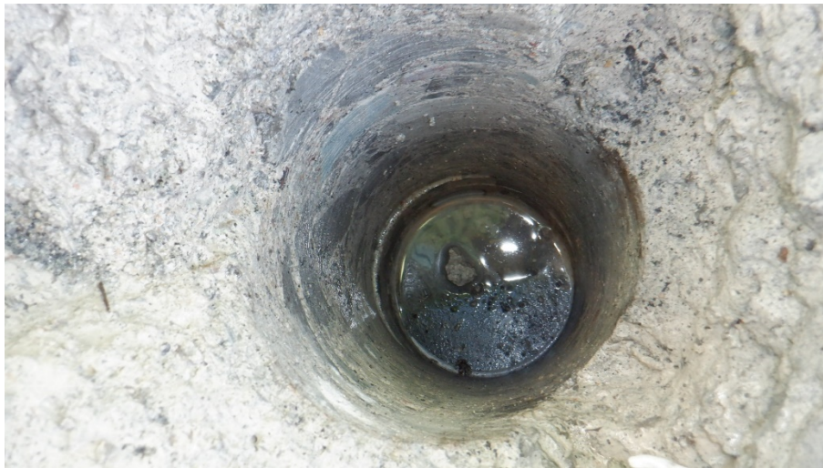
Figure 4-19: Counterweight truss steel plate exposed. Core hole C7 shown.
