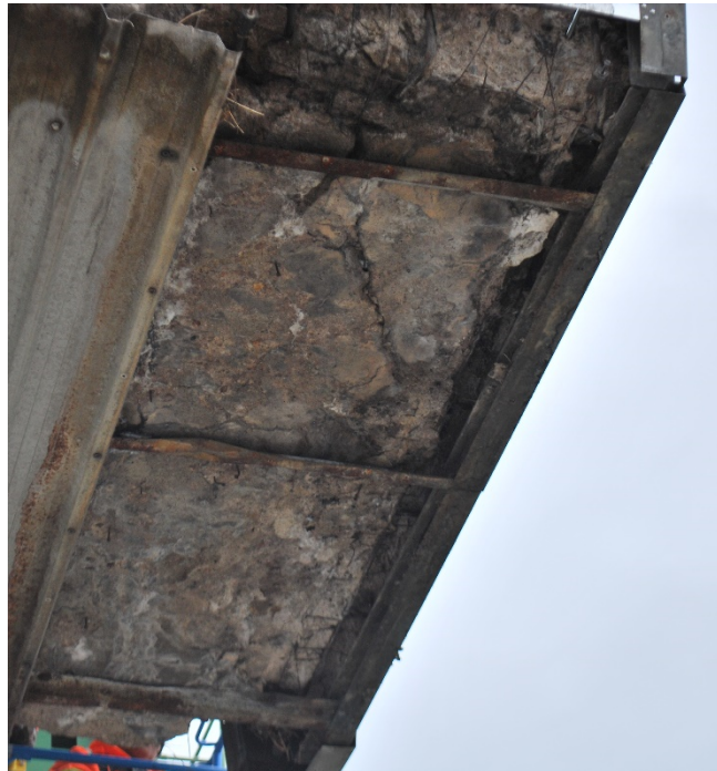
Figure 4-17: Condition of underside of counterweight. South end shown.
