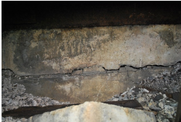
Figure 4-6: Fragments of deteriorated concrete and cracking along construction joint inside compartment on top face (second from South end) of Counterweight.
