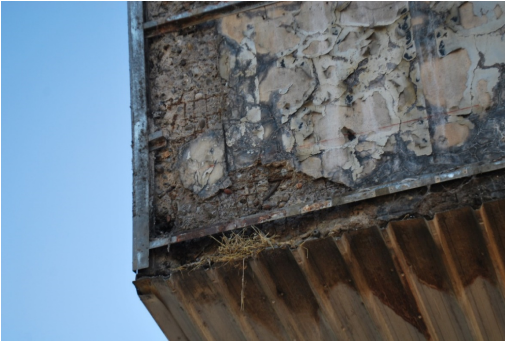
Figure A7 – North West bottom corner of West face showing concrete loss, spalling, exposed reinforcing steel and surface cracking. Corrosion observed along angle iron embedded in concrete.
