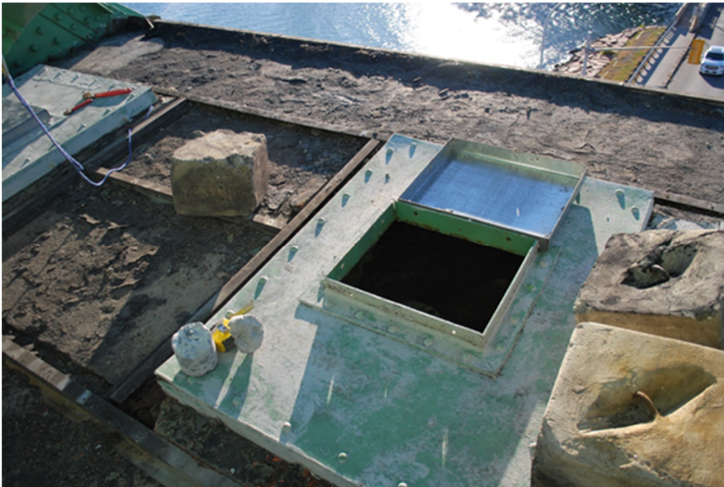
Figure A18 – Top face covered in roofing material. Door removed from one of four compartments located on the top face, which houses additional concrete weights.
