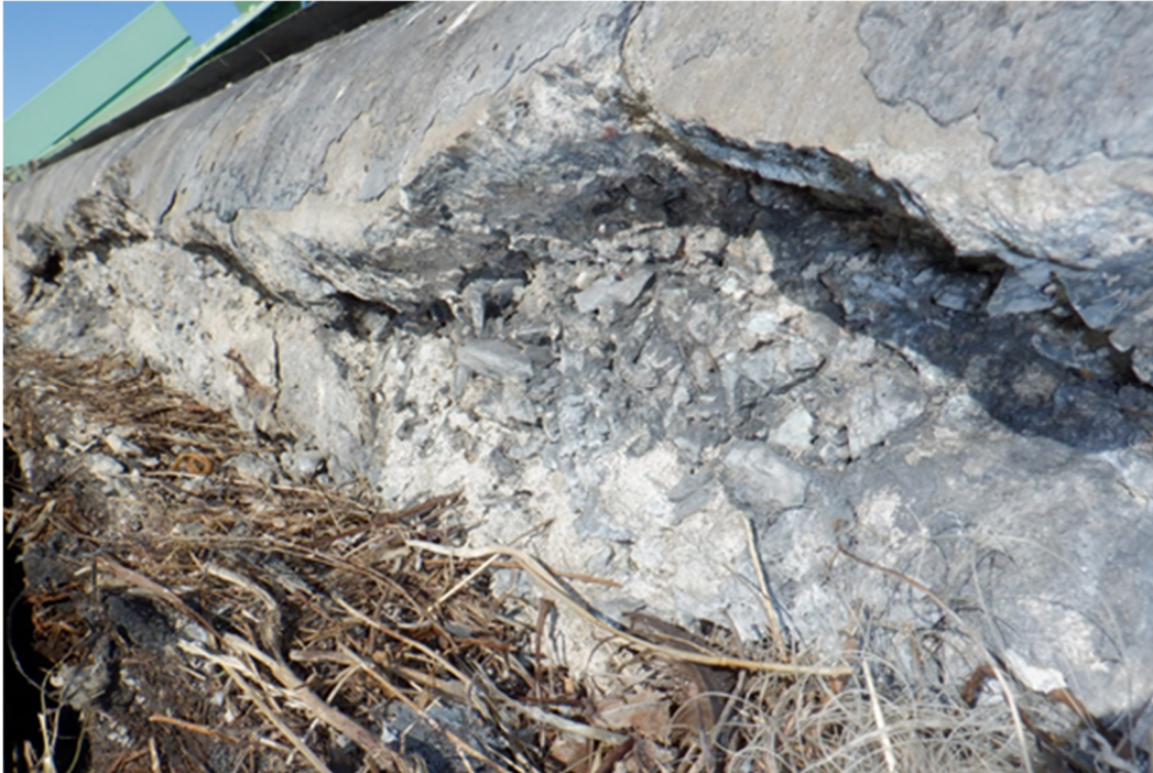
Figure A13 – Spalling at concrete found at the top of the West face (same location as in Figure A.12). Feather shown indicates debris is from birds nesting.
