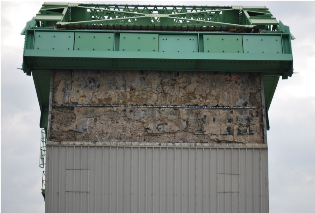
Figure A1 – Steel cladding removed from top half of West face. Underlying concrete showing areas of spalling, and map cracking.
