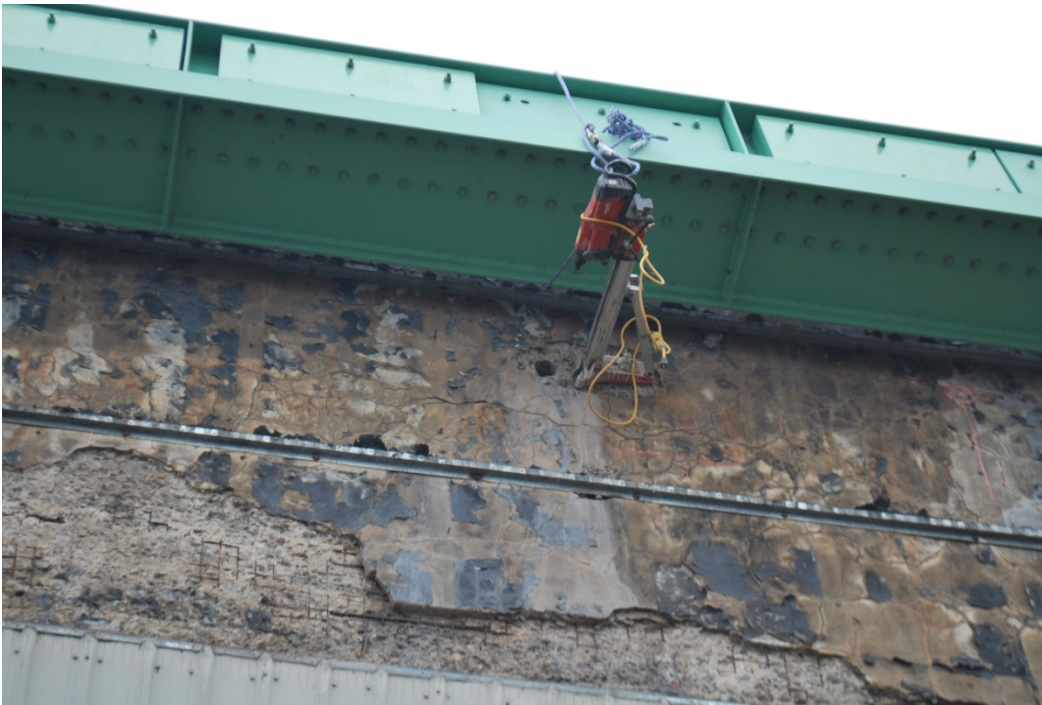
Figure A5 – Concrete coring at location C1. Area surrounding core location shows original yet delaminated concrete. Exposed reinforcing mesh and spalled concrete is present.
