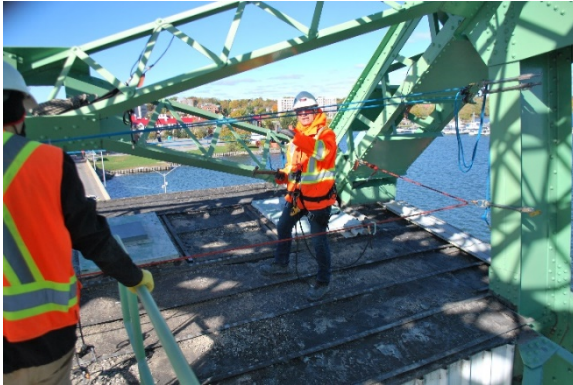
Figure 4-3: Top face covered with roofing material. North half of top face shown.
