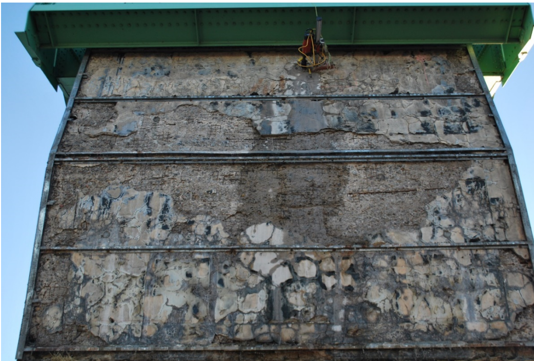
Figure A6 – Steel cladding removed from entirety of West face. Spalling and exposed reinforcing mesh in center portion of the face in addition to areas of delamination and cracking at top and bottom areas.
