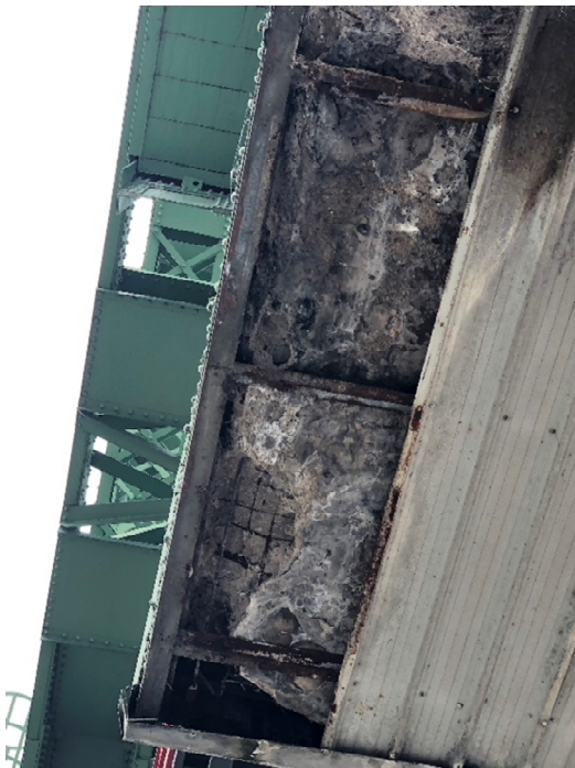
Figure 4-16: Condition of underside of counterweight. North end shown
