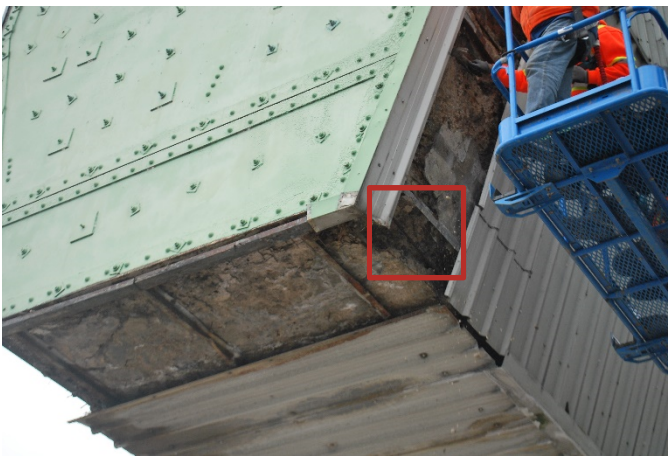
Figure 4-7: Bottom South East corner of East face showing cracking and areas of spalling. South end of bottom face also shown.
