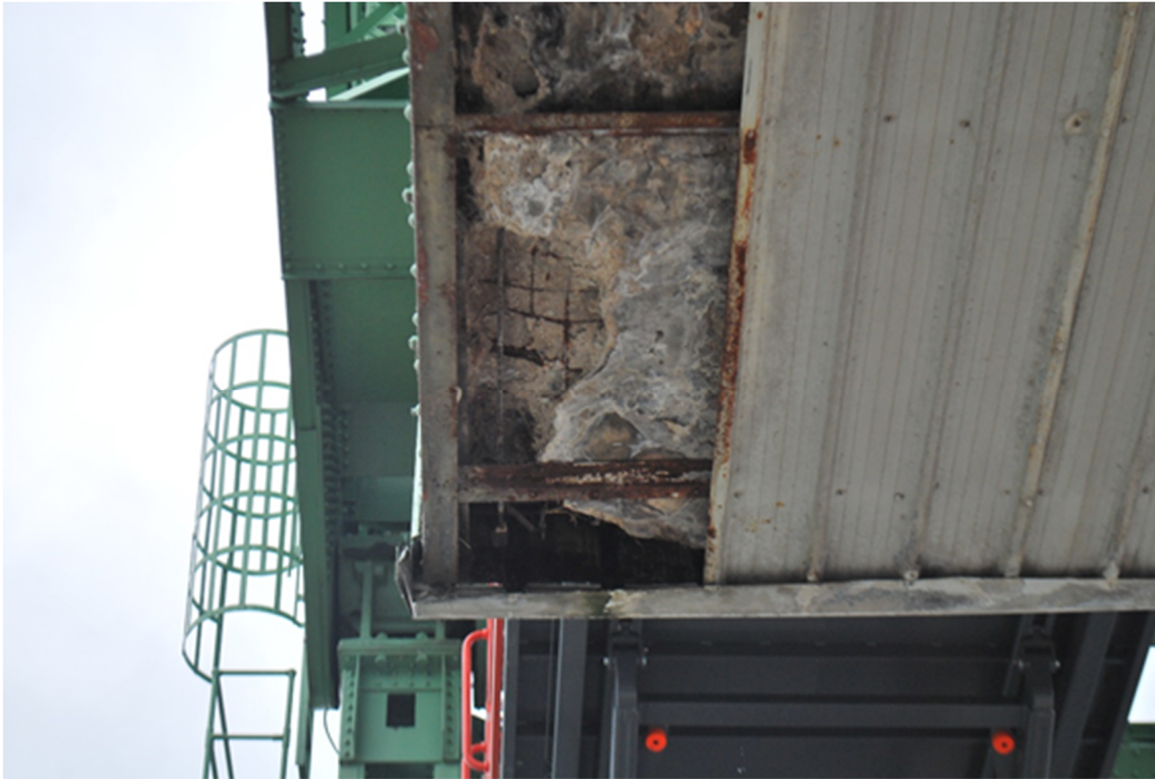
Figure A17 – Test pit taken from North East corner of bottom face. Underlying steel reinforcement showing severe signs of corrosion.
