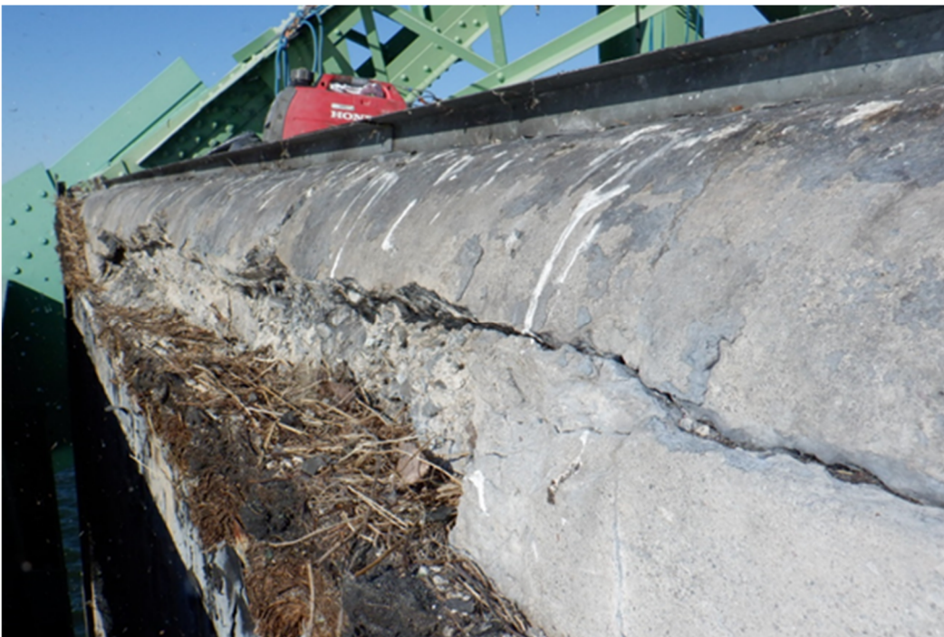
Figure A12 – Top edge of West face. Crack, 25 mm – 50 mm in width running entire top edge of West face. Debris shown is assumed to be from birds nesting.
