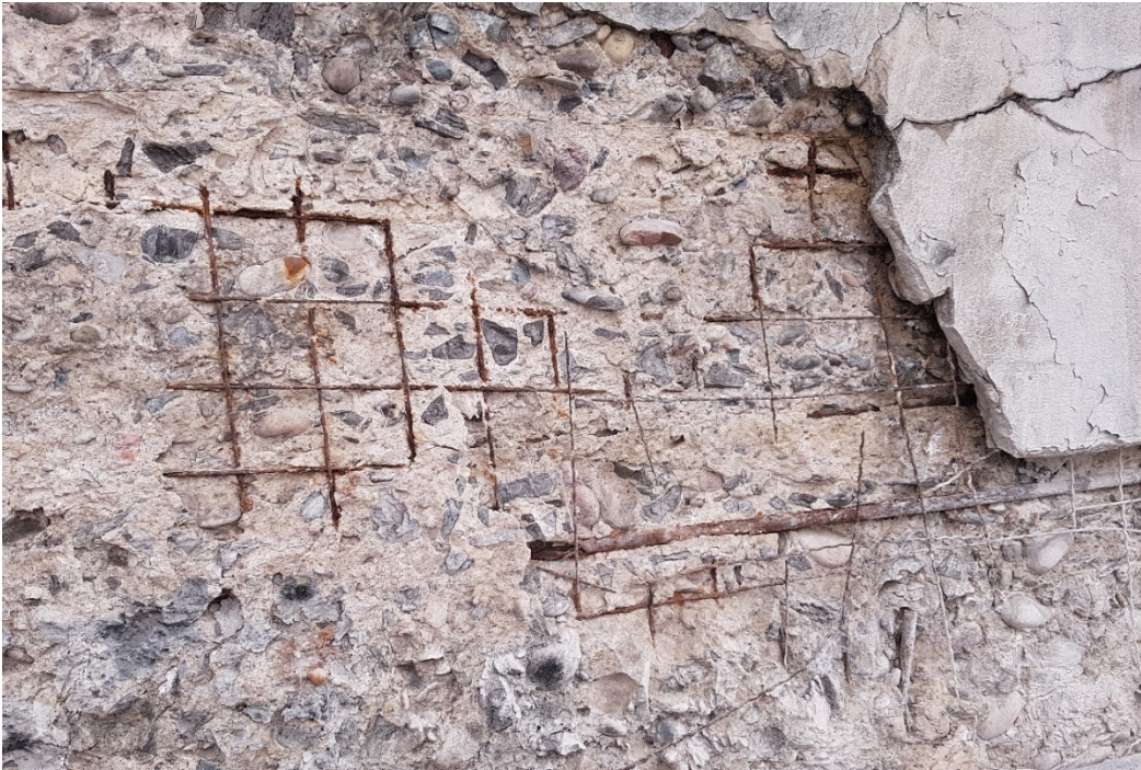
Figure A11 - Concrete condition in center portion of West face showing surface delamination, exposed reinforcing steel and steel mesh.
