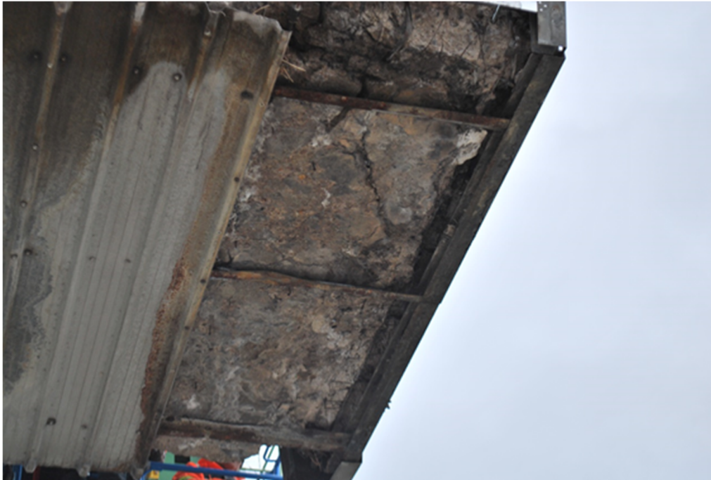
Figure A15 – Condition of concrete on South end of bottom face. Localized areas of cracking, delamination and spalling. Angle iron embedded in concrete is in poor condition showing generalized corrosion.
