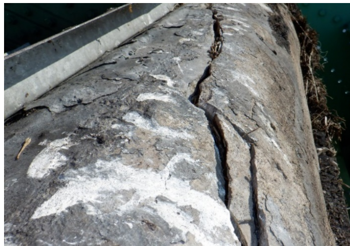
Figure 4-2: Crack (15 mm – 25 mm in width) running along top edge of West face.
