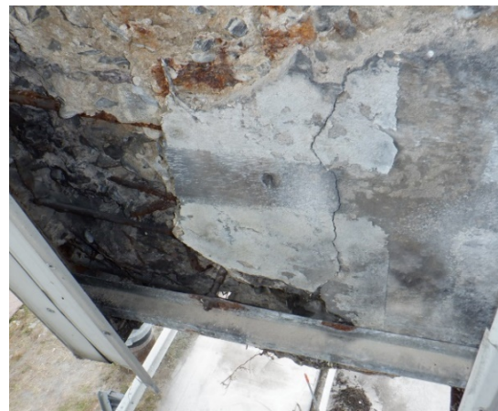
Figure 4-8: Zone indicated by red box in Figure 4-7 (Bottom South East corner of East face).
