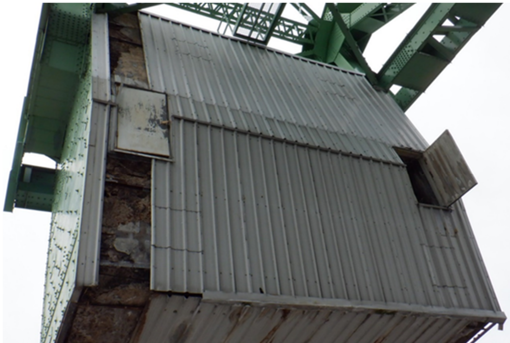
Figure A22 –Two compartments located on East face designated as South and North. Steel cladding removed from South side of East face. North compartment is where cores C3 and C4 were removed (see Figure A27).
