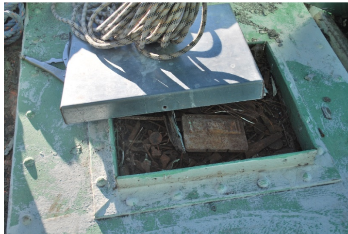
Figure 4-5: Metal debris inside compartment on top face of Counterweight.
