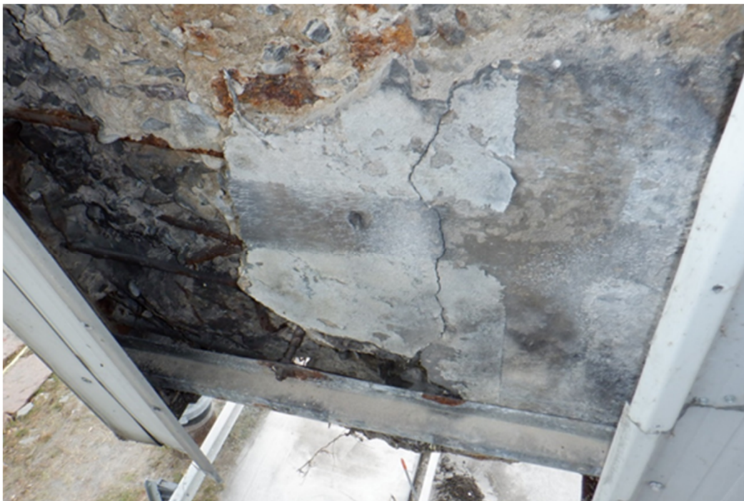
Figure A24 – Bottom left hand corner of East face showing signs of spalling, cracking, exposed reinforcement and areas of corrosion.
