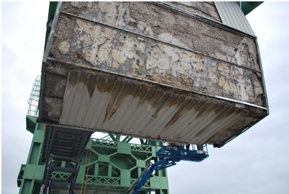
Figure A14 – Steel cladding removed from North and South ends of bottom face. Partial view of West face also shown.
