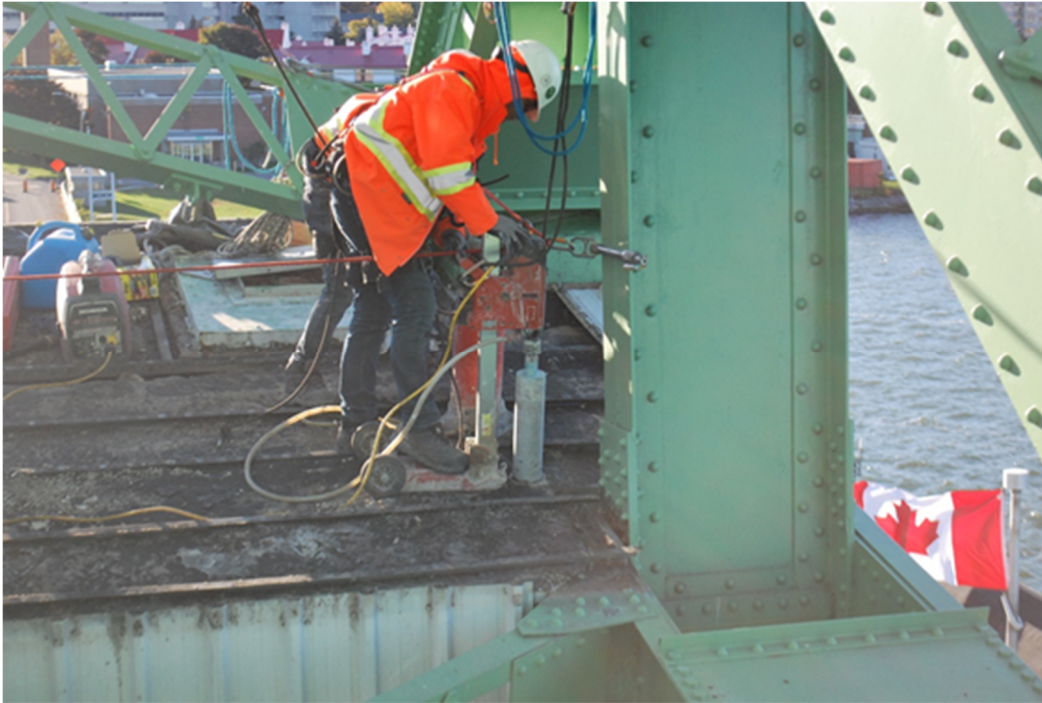
Figure A21 – Coring at location C7 (North East corner of top face).
