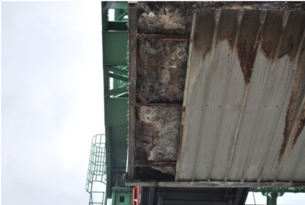
Figure A16 – Condition of concrete on North end of bottom face. Localized area of cracking, delamination and spalling. Surface staining is observed on remaining steel cladding.
