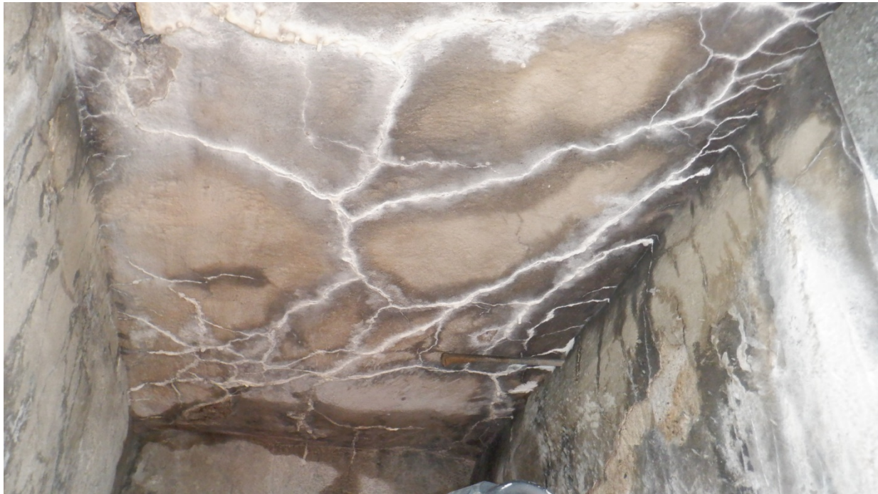
Figure A26 – Condition of concrete inside North compartment on East face. Excessive map cracking on the ceiling of compartment resulting in efflorescence.
