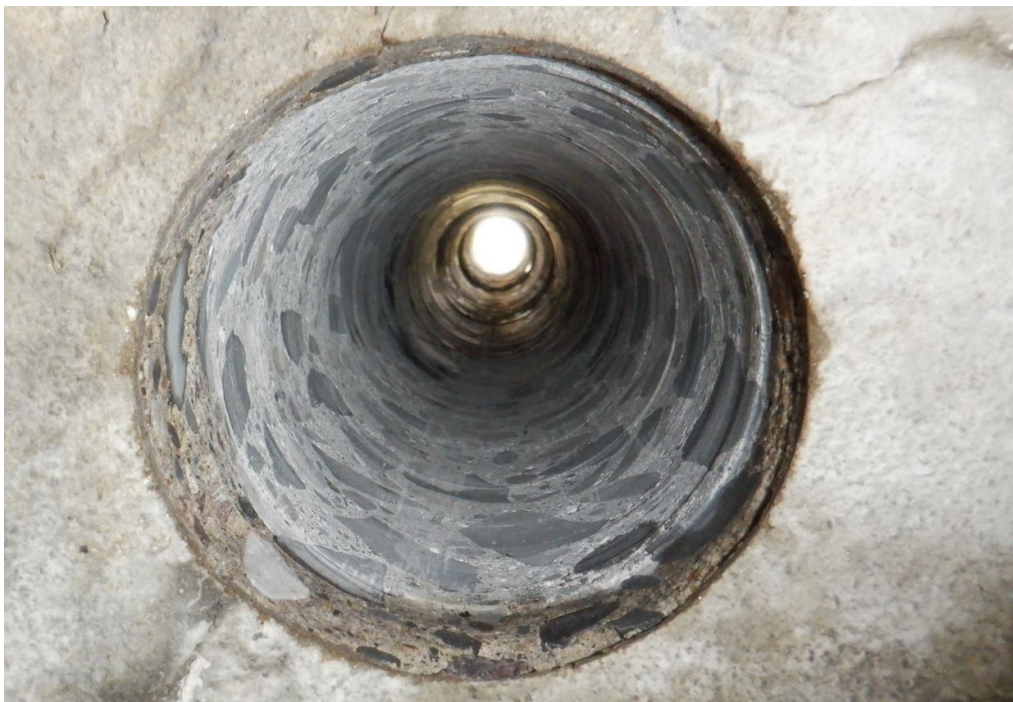
Figure A30 – Core hole C2 (full depth). Photograph taken from inside South compartment on East face. Photograph is looking in the West direction.
