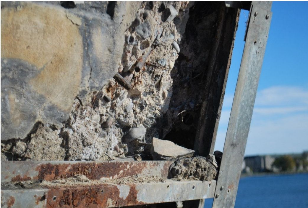
Figure A8 – South West bottom corner of West face showing concrete loss, spalling, exposed reinforcing steel and surface cracking. Corrosion observed along angle iron embedded in concrete.
