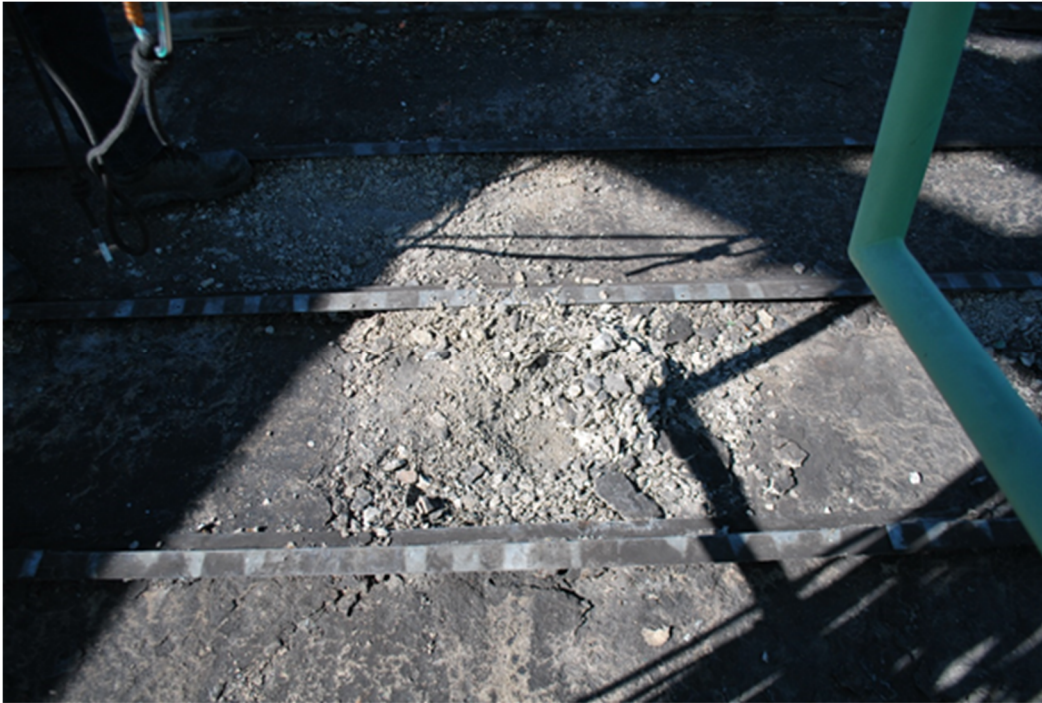
Figure A19 – Surface scaling on the top face (concrete fragments 10-50mm in diameter).
