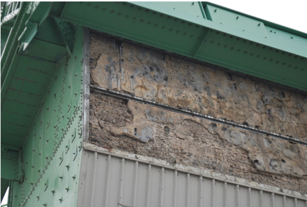
Figure A2 – Delamination, surface cracking and exposed reinforcing mesh. Concrete was originally designed with a concrete cover depth of 50mm over the reinforcing mesh.
