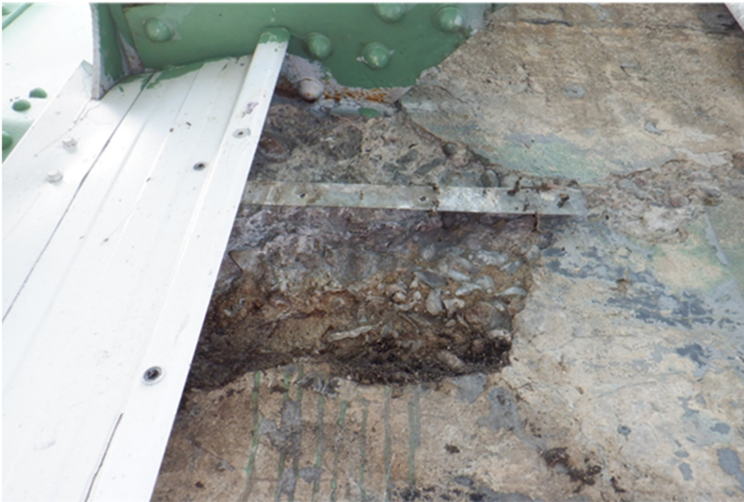
Figure A23 – Surface spalling on South end of East face
