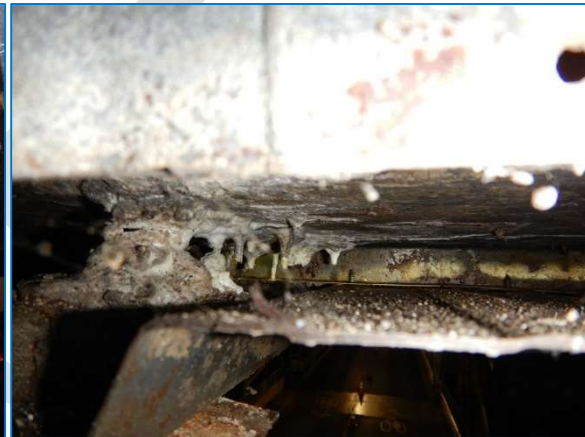
Photo 2 Soffit - Efflorescence, Stalactites, Stalagmites, Typ.
