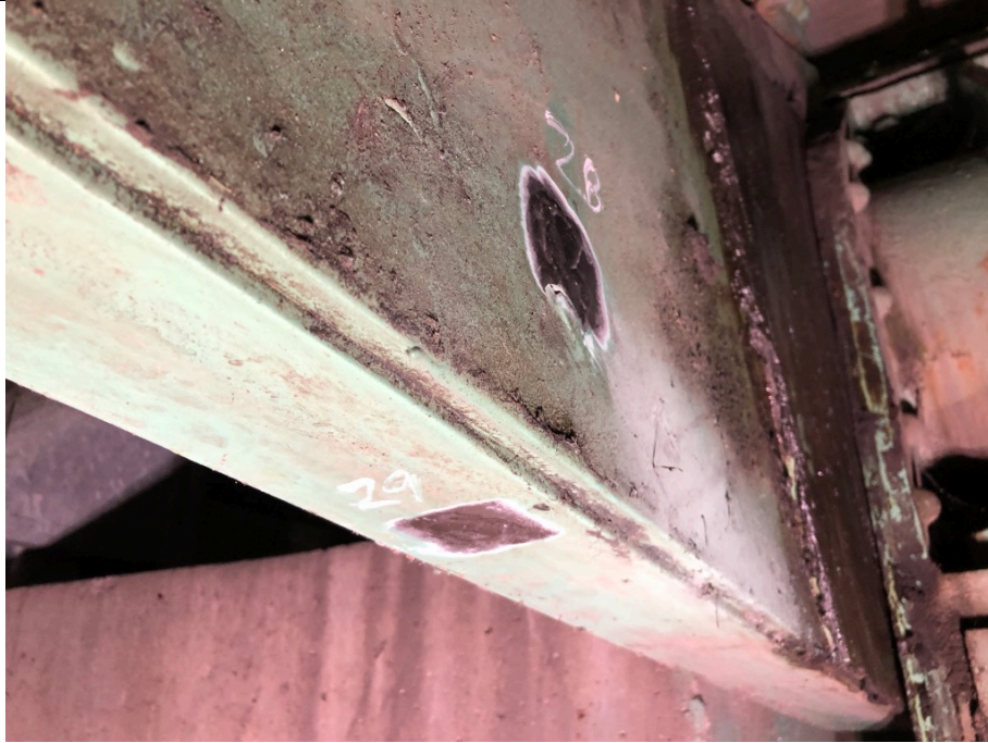
Figure9: Test Locations 28 and 29 at South Trunnion Plate Exterior Location (Readings Taken from Inside Surface and Bottom Surface of Angle)
