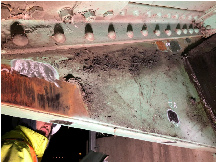
Figure8: Test Locations 25, 26 and 28 at South Trunnion Plate Exterior Location (Readings Taken from Inside Surface)
