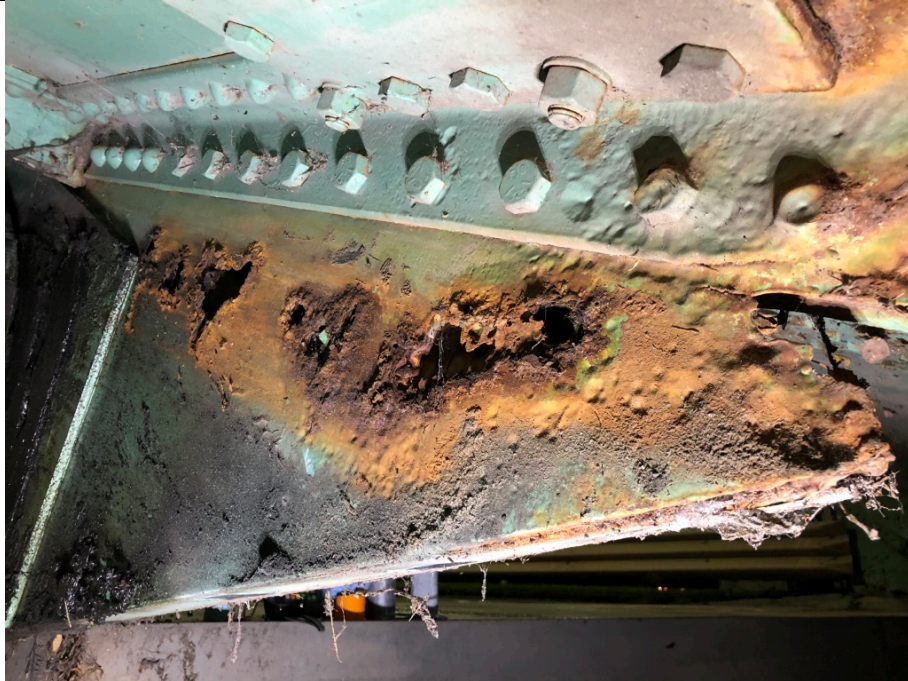
Figure7: Opposite Side of South Trunnion Plate Interior Location (Inside Plate Surface, see Figure 6 for Exterior Plate Surface)
