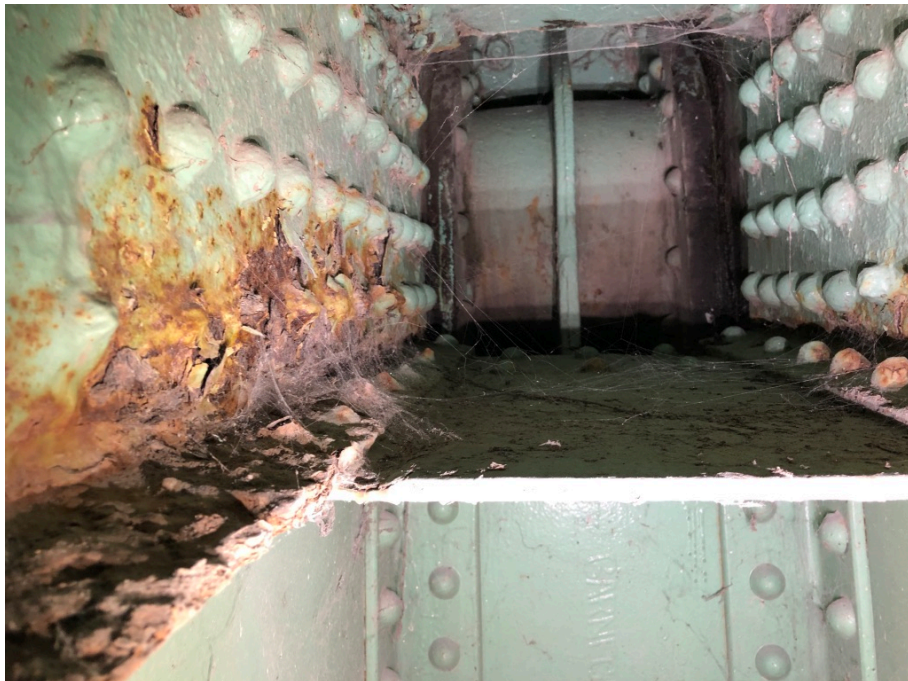
Figure12: Test Locations 43 and 44 at South Trunnion Exterior Plate at Interior Batten Plate and Angle
