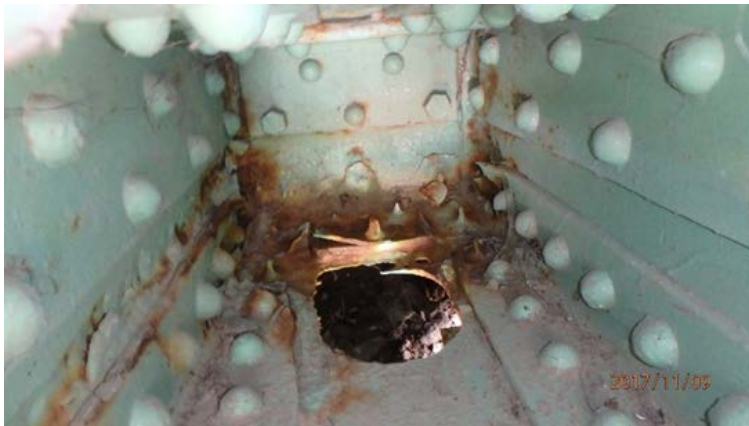
Figure 6 - Local deterioration at member 15-17
