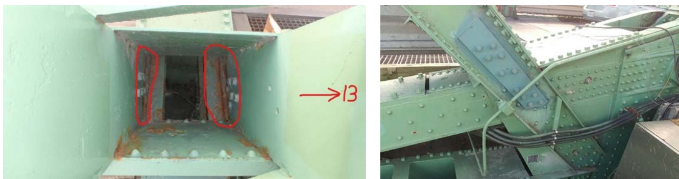
Figure 5 - Diagonal 13N-16N a) Left: Section loss of \pm 25\% on the webs of both channels (b) Right: Existing strengthening on the outside
