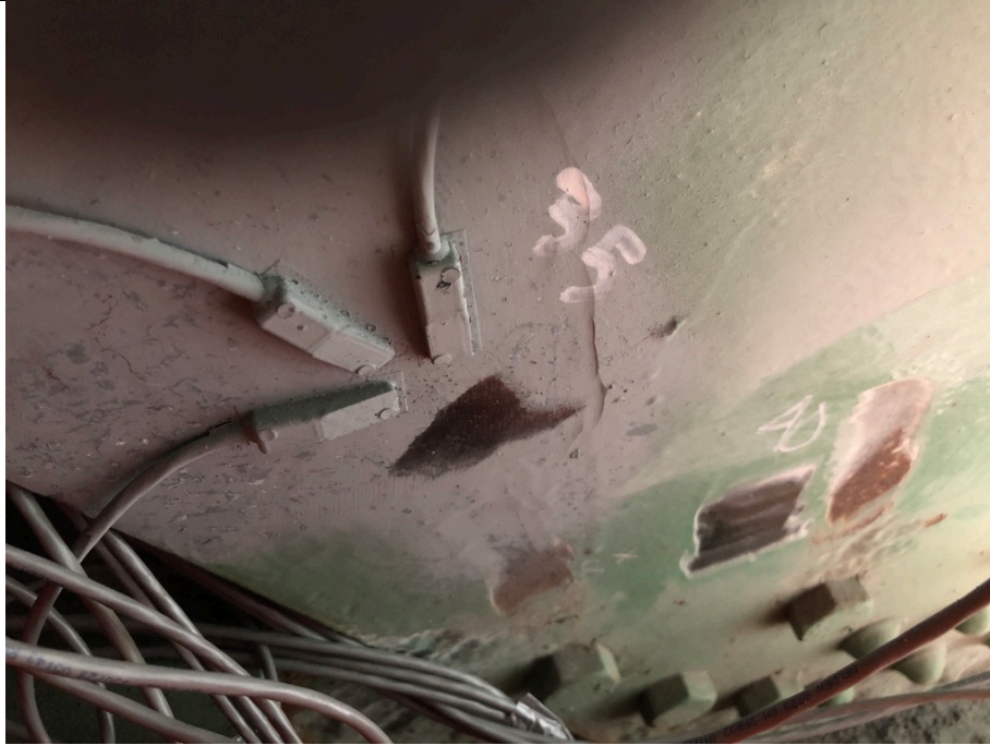
Figure15: Test Locations 35, and 40 at South Trunnion Exterior Plate Location (Readings Taken on Interior Surface of Plate)
