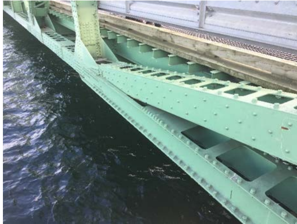
Figure 19 - Intersection between members 14-15 and 14-16
