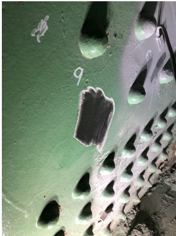
Figure3: Test Locations 9a and 9b at North Trunnion Plate Interior Plate (Readings Taken from Inside surface of Plate)
