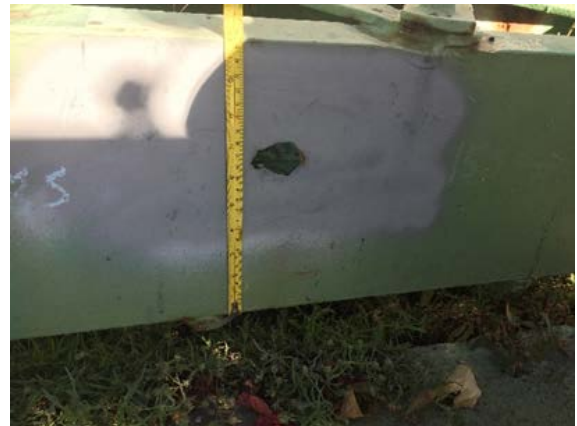
Figure 7 - Localized section loss near the middle of member 15S-18S
