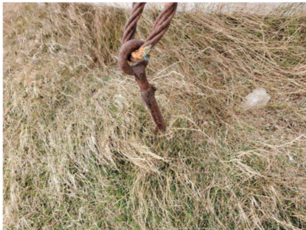
Guy wire not anchored to the ground
