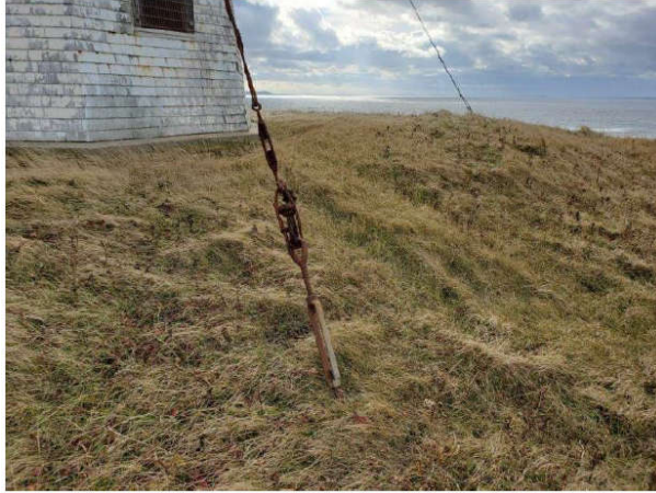
Corroded guy rope
