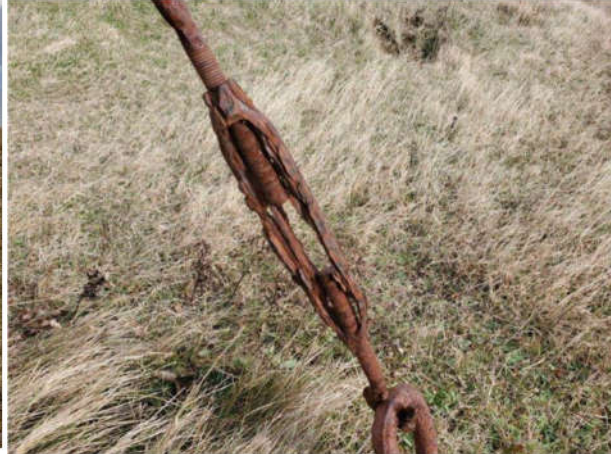
Severely corroded guy rope
