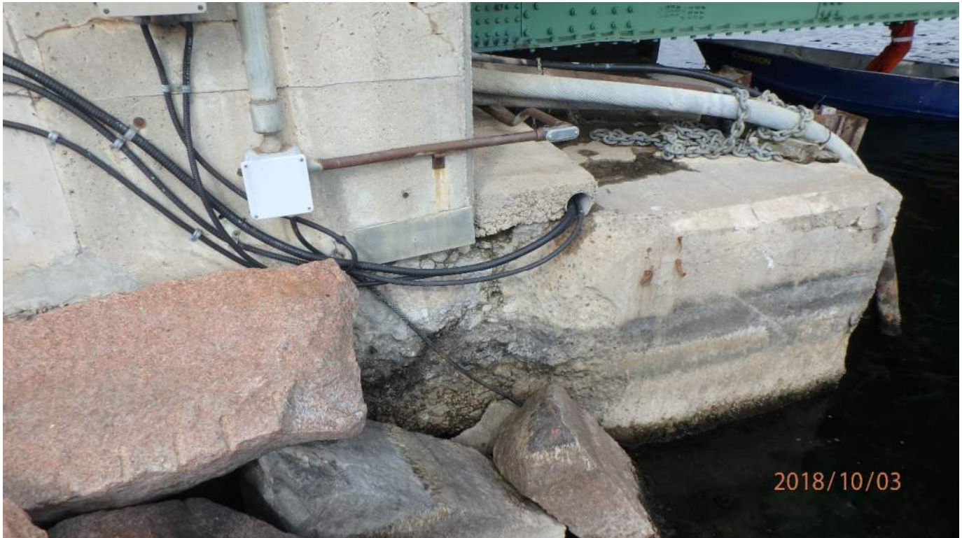
Photo S108: Very severe spall at the base of the southwest wingwall at the interface with the abutment.
