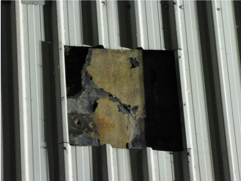
Photo S78: The counterweight concrete in the lower northwest corner exhibits a severe spall and wide cracks.
