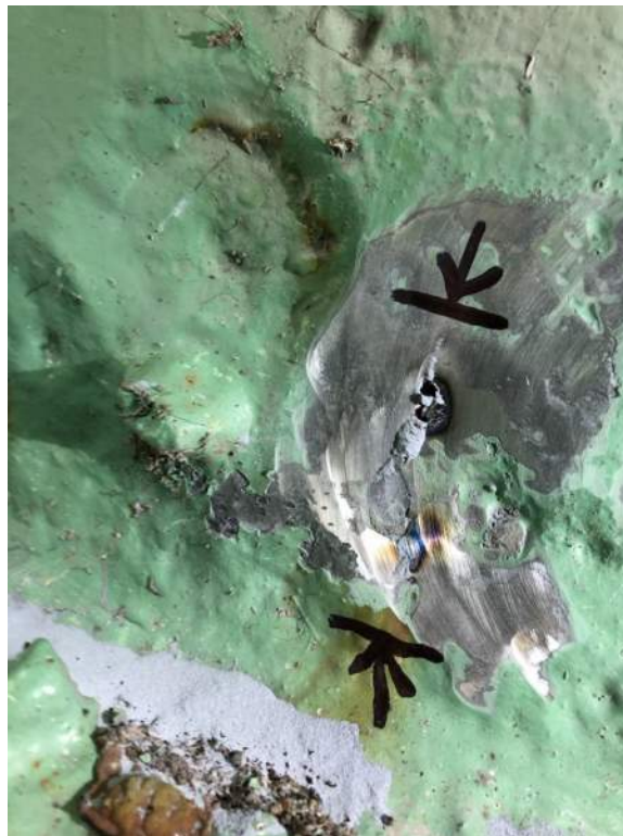
Photo S37: Perforation and 60mm long crack in south channel of tower truss bottom chord member 18S-19S (photo by Brouco NDT).
