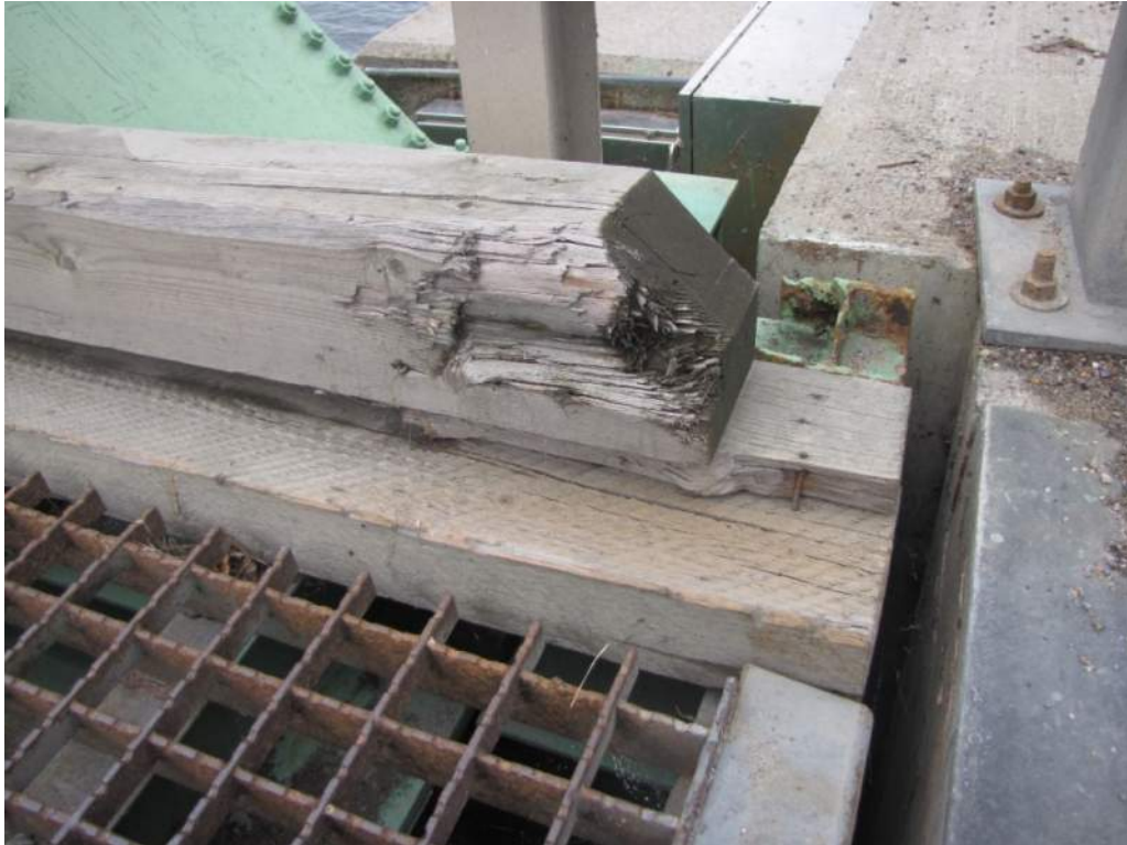
Photo S106: The east end of the north timber curb has some impact damage and is not anchored to the deck.
