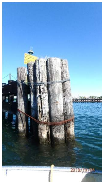
Photo S117: The lower cables securing the dolphin to the south end of the west training wall are loose and corroded. One pile has broken off.
