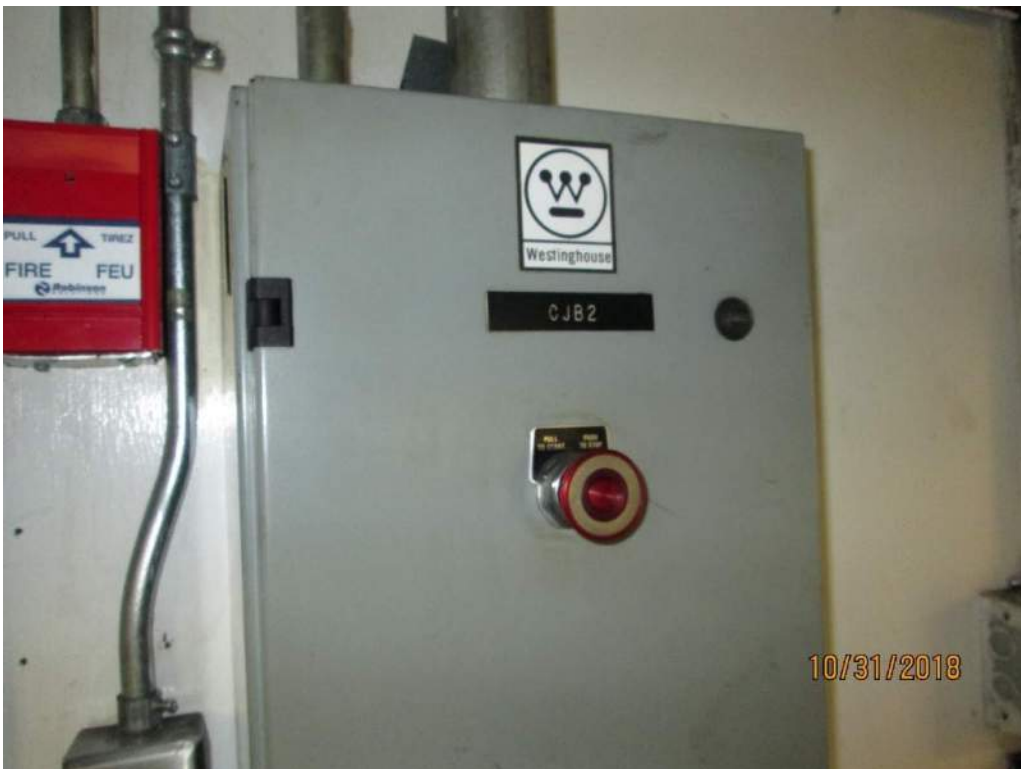
Photo E20: Machinery Space Local E-Stop. This E-Stop switch is located near the machinery space entrance. It allows maintenance personnel to prevent or stop bridge operation when work is being performed in the machinery space.
