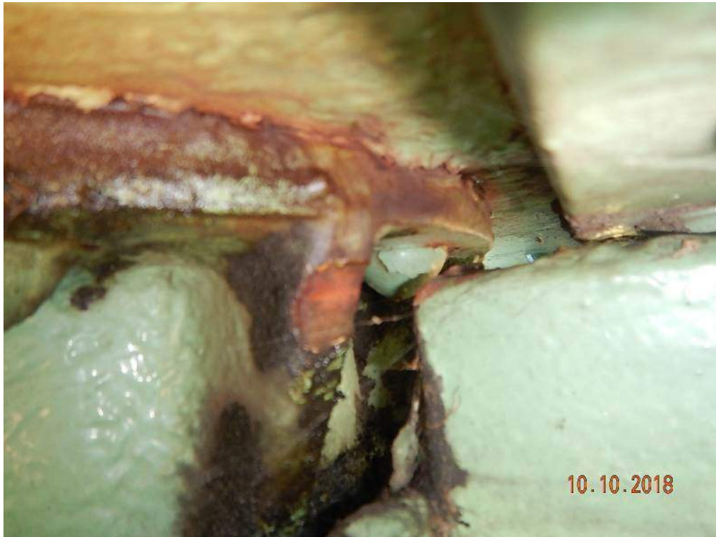
Photo M9: South Operating Strut, Outboard Bearing. The bearing housing stiffener is rubbing on the structure.
