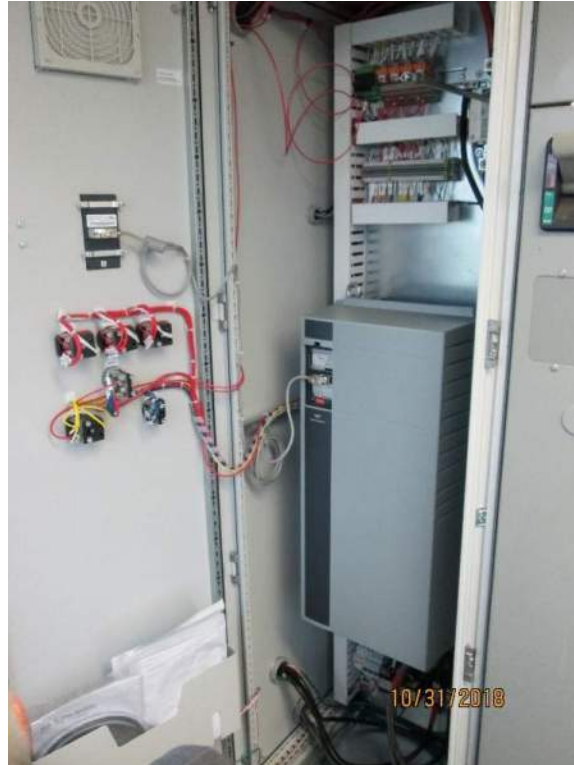
Photo E7: Span VFD Drive Cabinet. The span variable frequency drives are newly installed and replace the original drive motor controllers for the span drive. The new VFD drives are located in their respective drive enclosures and provide excellent and variable speed and torque control for the operating bridge.
