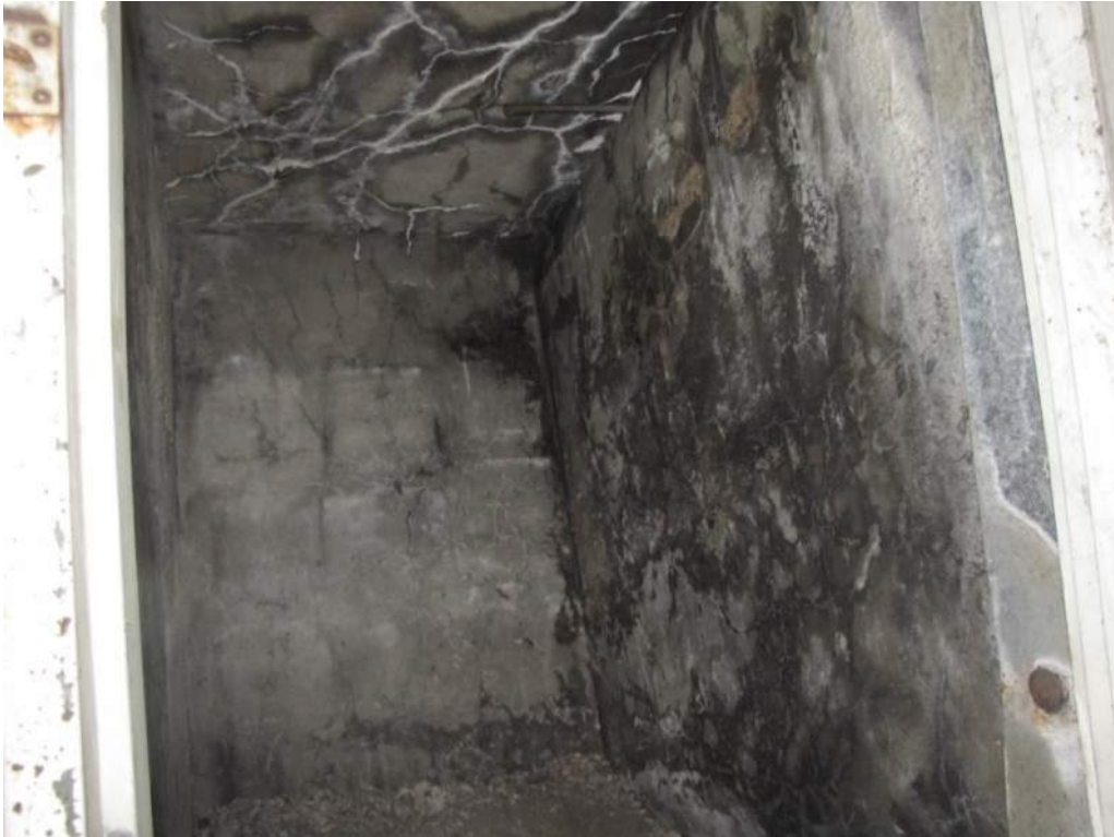
Photo S64: Spalls, disintegration, map cracking, efflorescence deposits, and wet stains were typically noted in the counterweight concrete inside the two voids in the east face (photo from 2017 inspection).
