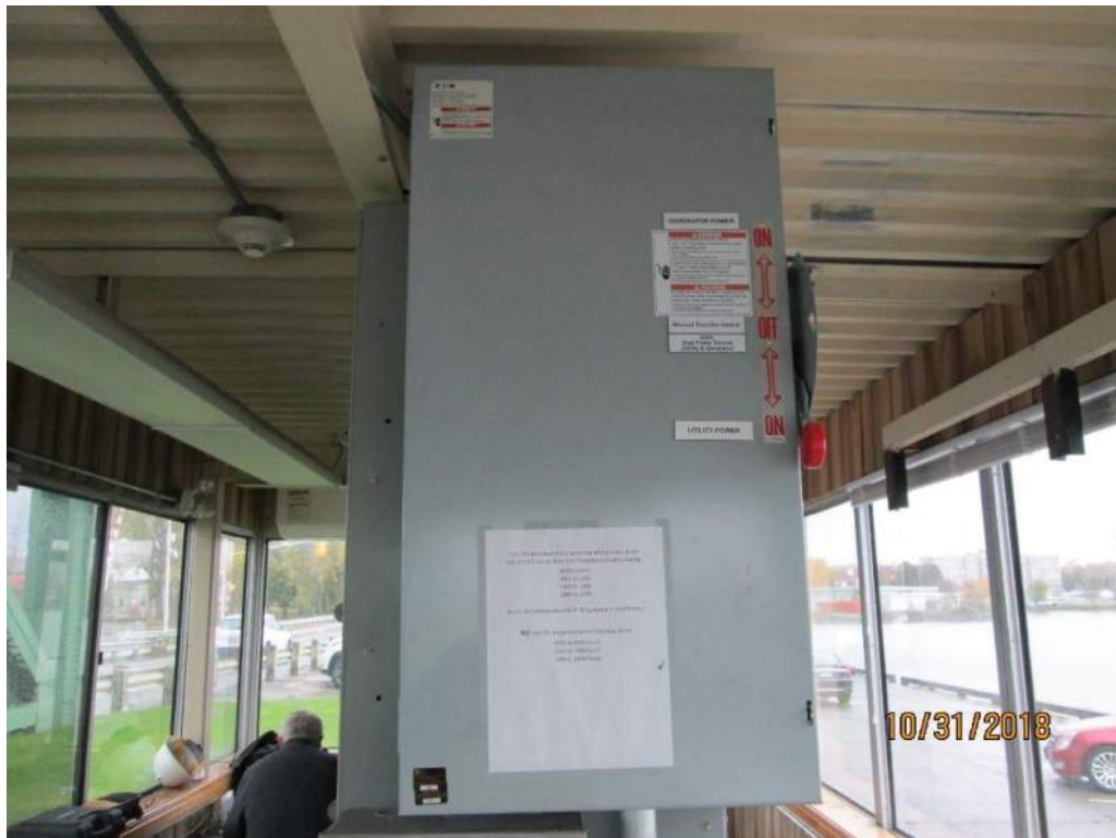
Photo E4: Manual Transfer Switch (MTS). A manual transfer switch has been mounted on the side of MCC in the operators control house to allow the transfer of power between utility power and the generator power. This MTS is in excellent physical and operational condition.
