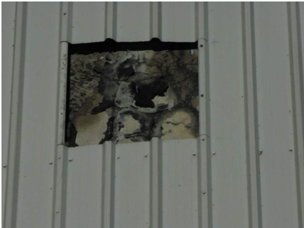
Photo S81: The counterweight concrete in the lower southwest corner exhibits an area of disintegration, and map cracking with wet stains.
