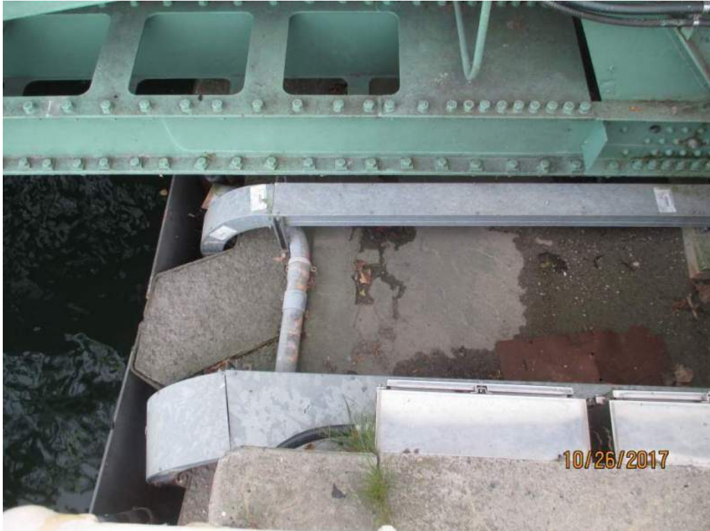
Photo E33: Typical Submarine Power Cables. The submarine cable is used to carry control and power across the channel. Both recently installed and originally installed submarine cables were found at the bridge. It was unclear if the old submarine cable was abandoned or still in service. Note the new submarine cable is of the Teck cable type and is protected with wireways above water level on the pier.
