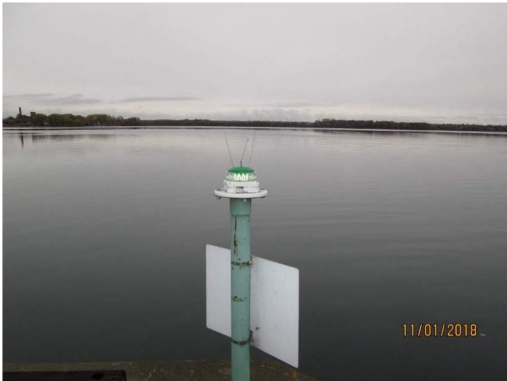
Photo E30: Typical Fender Light. The bridge is provided with 4 fender light fixtures, one at each corner of the fender. The north fender lights are flash red and the south fender lights are flash green. The fender lights are of LED type and are in good operational condition.
