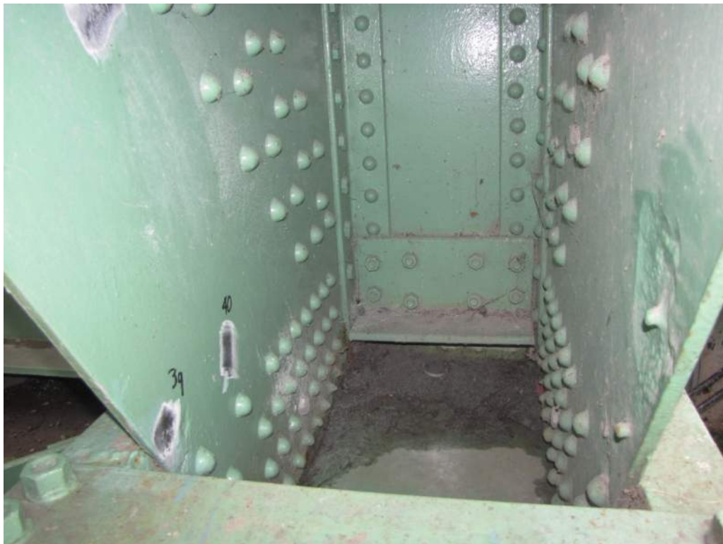
Photo S43: The interior faces of the plates and rivet heads at the base of the north trunnion have localized severe section loss.
