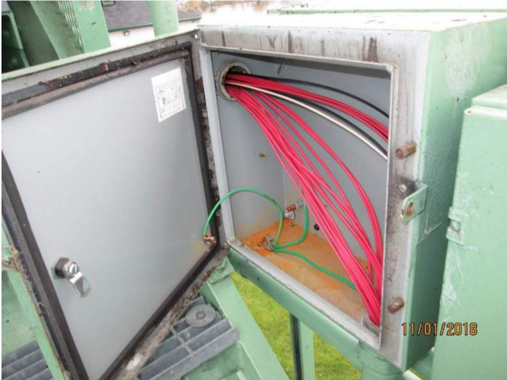
Photo E31: Typical Outdoor Junction Box. Many of the outdoor junction/pull boxes are NEMA 4X boxes. Note the junction/pull boxes are in good physical condition, but some of the boxes do exhibit signs of corrosion inside the boxes.
