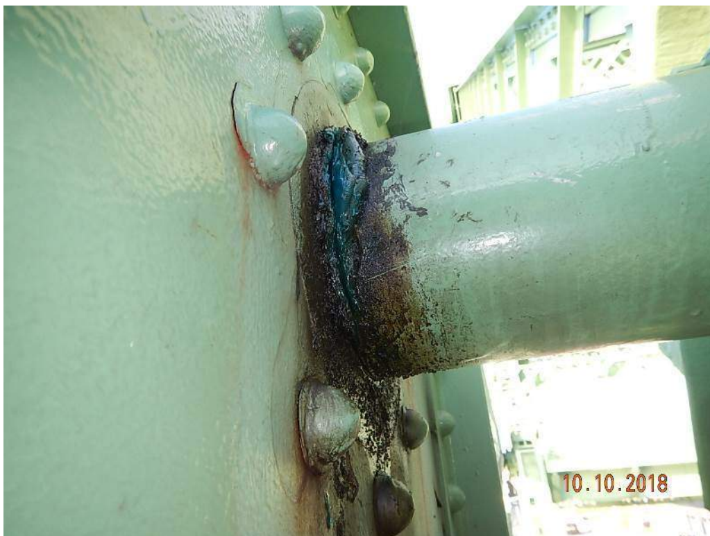
Photo M8: South Operating Strut, Inboard Bearing. The cracked paint and fretting corrosion at the rivets indicate that the connection is loose.
