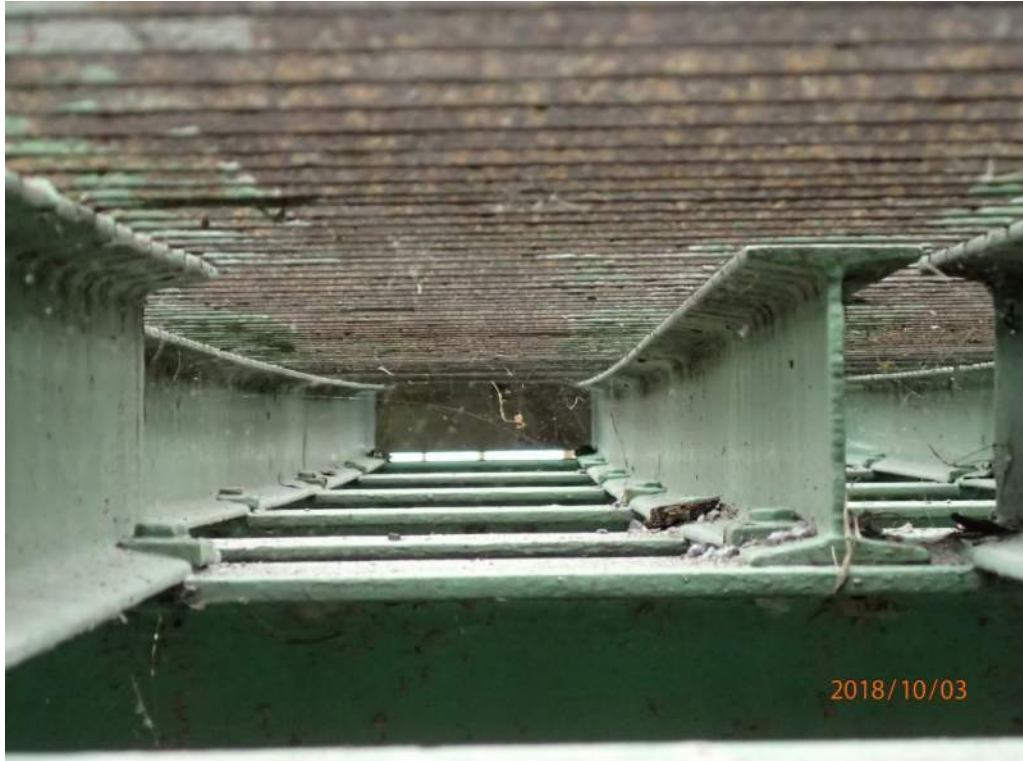
Photo S58: The sills supporting the deck grating are typically permanently deflected.
