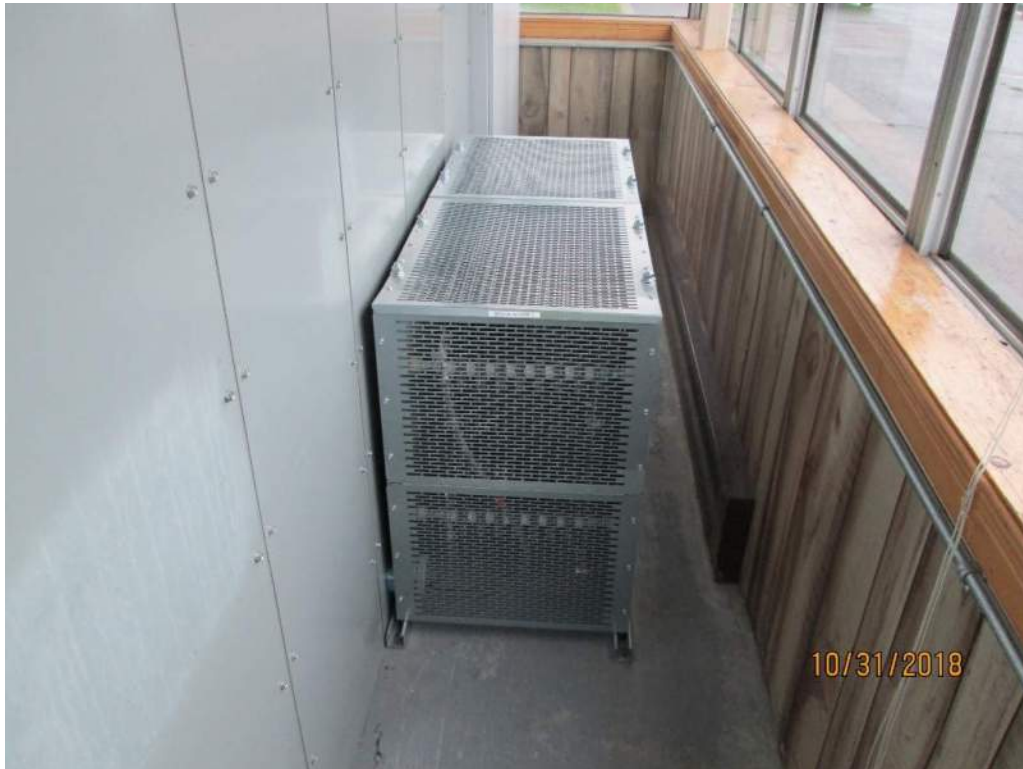
Photo E9: Typical Dynamic Braking Resistors. Dynamic braking resistors have been installed in conjunction with the VFD drives to provide speed and torque braking control for the span drive motors. These resistors were installed when the VFD drives were installed and are in freestanding enclosures located behind the MCC.
