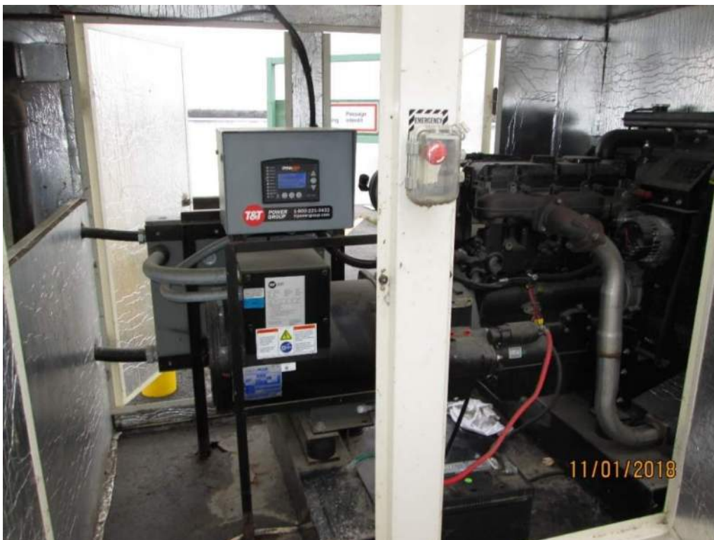
Photo E2: Standby Generator. The standby generator was installed in 2015 to provide a backup source of power for the bridge facilities in the event of utility power failure. Note that the generator, since the original drives and motors were replaced, is now capable of handling of span operation with one operating drive motor. Also note the generator and generator housing is in excellent physical condition.
