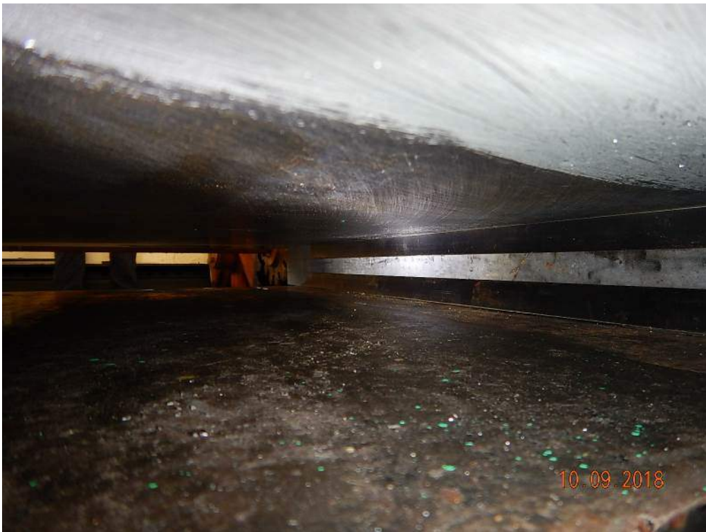
Photo M4: Span Drive Machinery South Motor. The underside of the motor mounting support is unpainted. The span drive north motor is similar.
