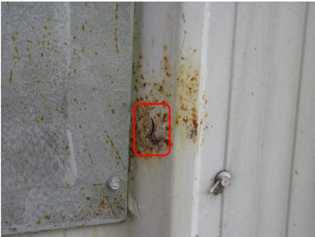
Photo S65: There is a small perforation beneath the north door in the east face of the counterweight panels adjacent to the previous repair.
