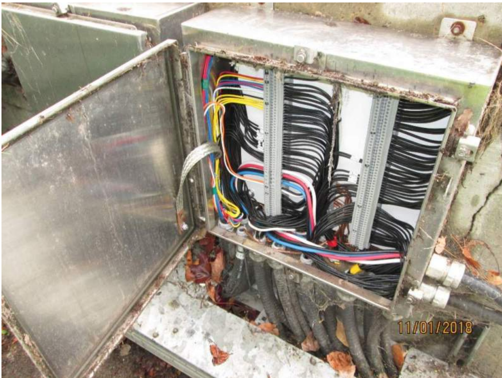
Photo E32: Typical Submarine Cable Junction Box. The submarine cable junction box is in good condition with proper grounding and bonding but covered with debris both internally and externally. Note the wires inside the submarine cable junction boxes are not properly labelled.
