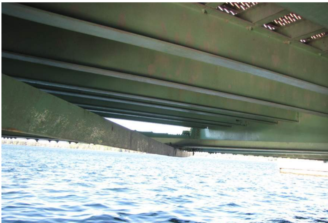
Photo S99: Lower cross bracing member 10N-12S is deformed.
