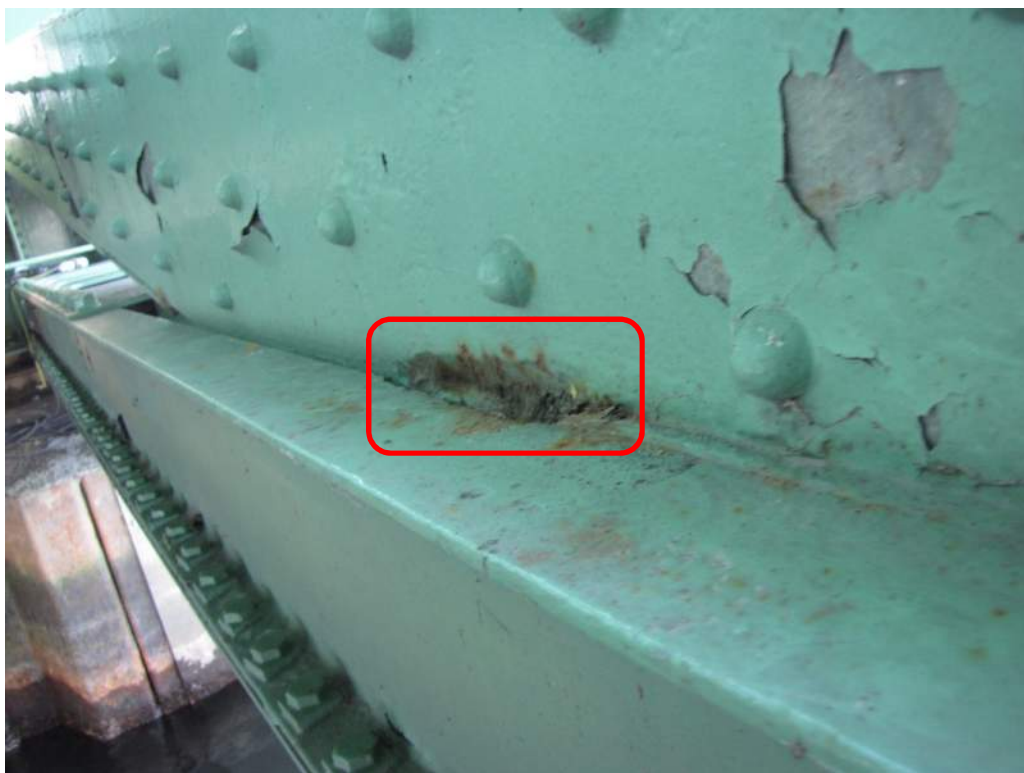
Photo S15: Severe pitting and rust jacking between member 14N-15N and 14N-16N.
