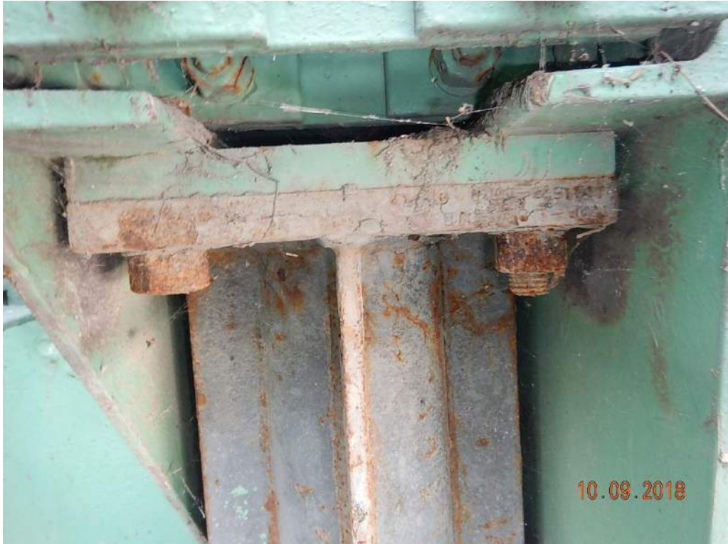
Photo M27: South Buffer. There is light corrosion between the top plate and the cylinder body. The mounting bolts exhibit moderate corrosion. The north buffer is similar.
