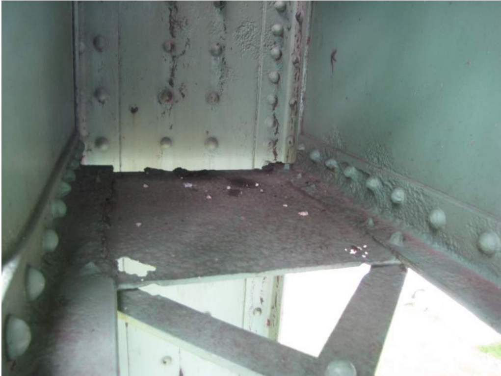
Photo S96: Tower truss sway bracing member 20N-20S has several perforations and deep pitting in the bottom gusset plate and severe section loss of the rivet heads at node 20N.
