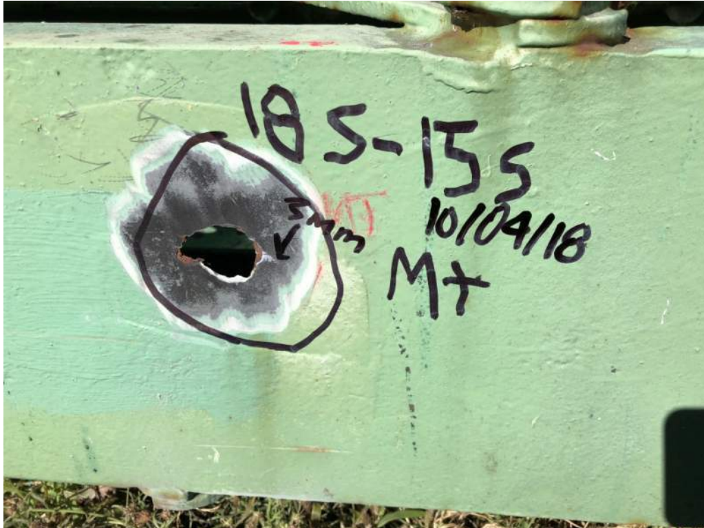
Photo S36: Perforation and 3mm long crack in south channel of tower truss bottom chord member 15S-18S (photo by Brouco NDT).
