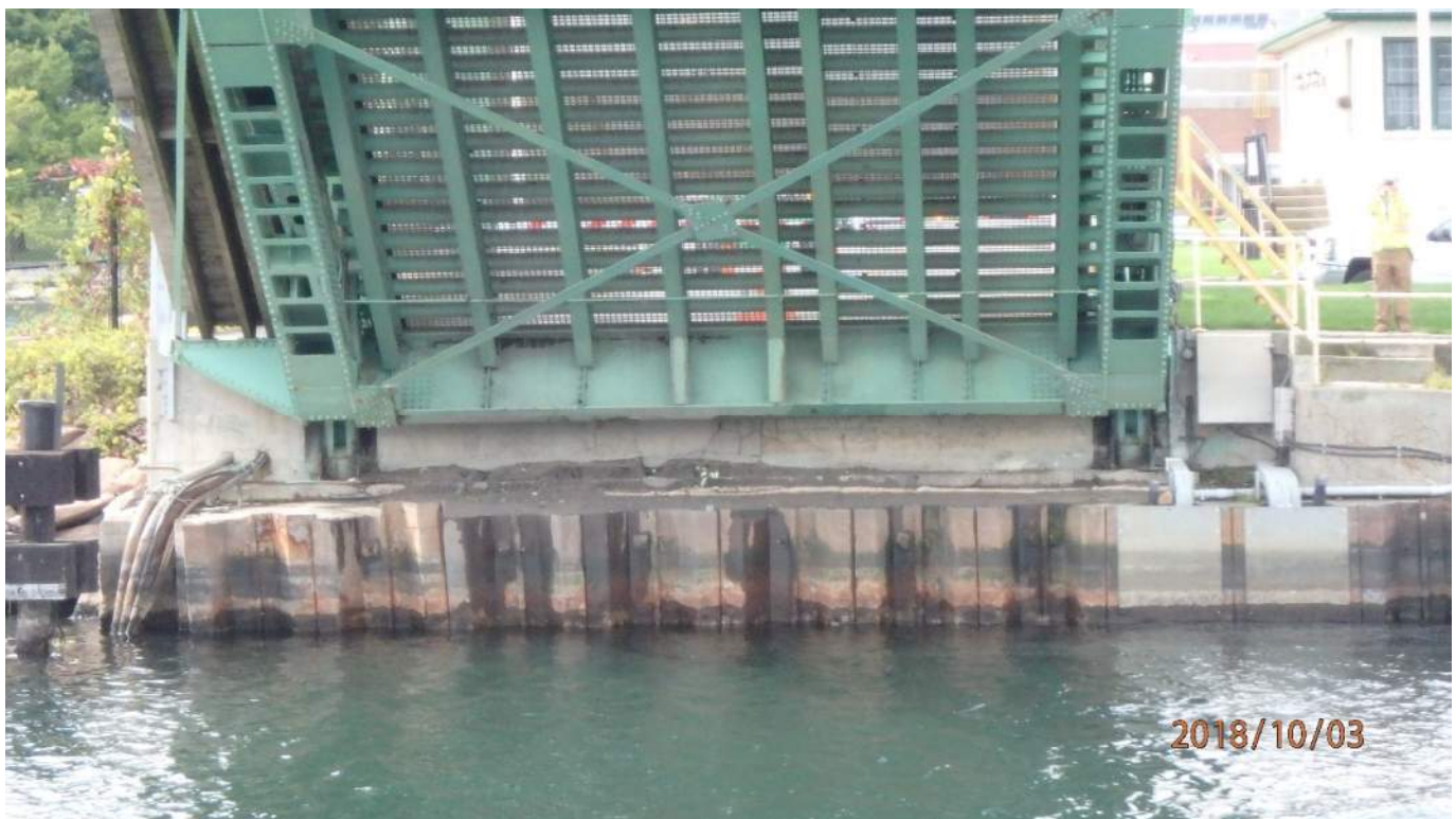
Photo S9: West abutment. Note the map cracking in the ballast wall.
