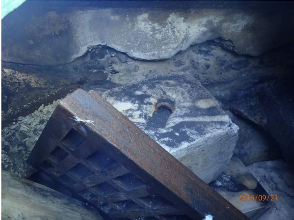
Photo S68: The concrete in the two upper chambers in the top face of the counterweight exhibits spalls, disintegration, and wet areas (2016 photo).
