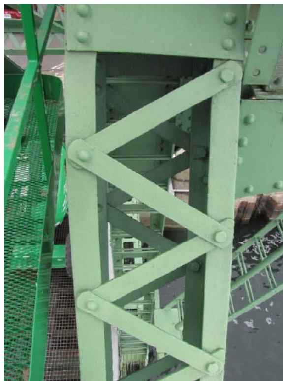
Photo S123: The top of 12N-13N near 13N is deformed.
