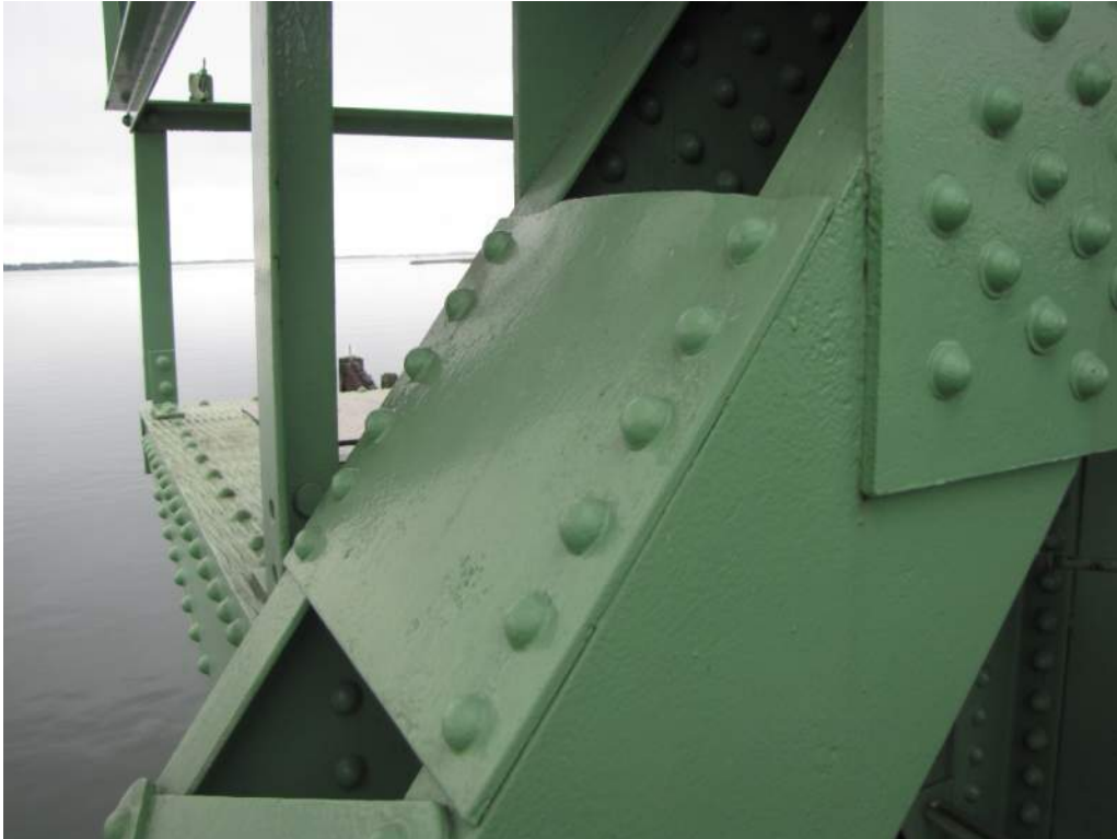
Photo S22: The upper batten plate of diagonal member 12S-13S near node 13S is deformed.
