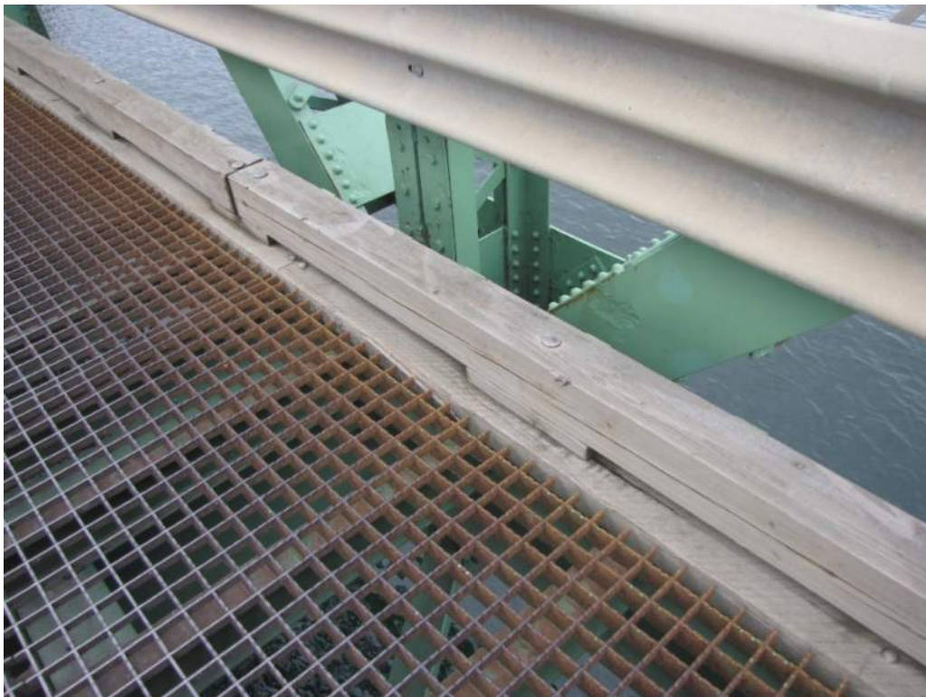
Photo S83: The roadway grating has widespread light to medium corrosion along the north and south edges (north side shown).
