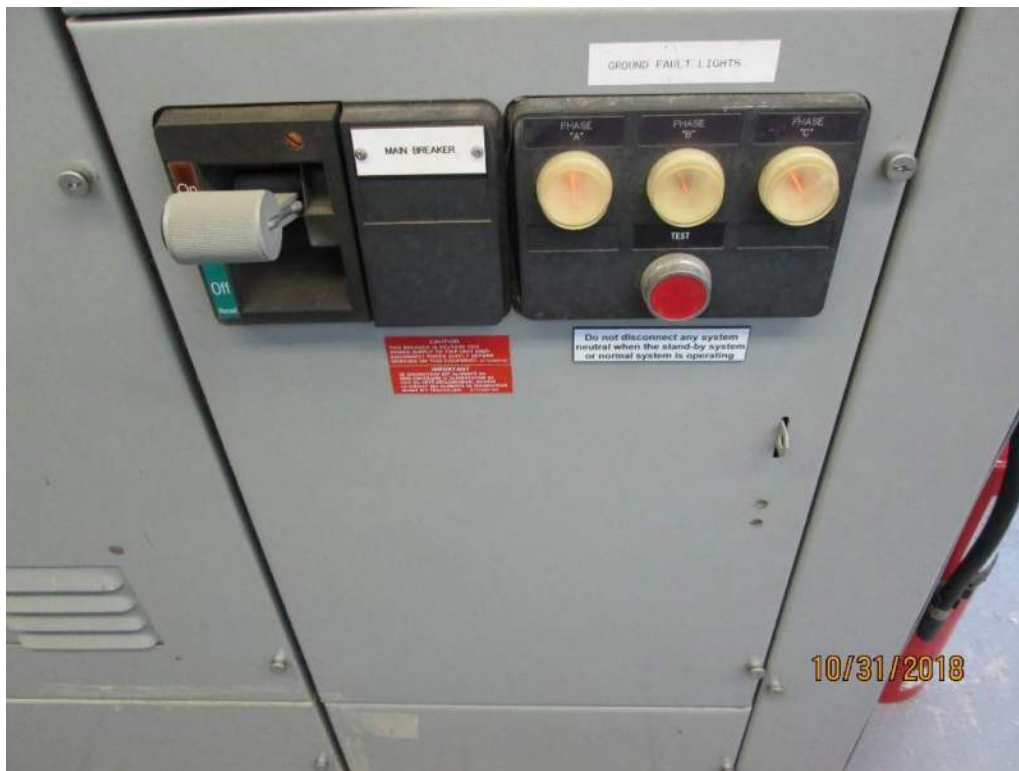
Photo E6: Ground Fault Indicators. A ground fault indicator light is provided for each phase of the 3-phase power. These indicator lights are provided on the MCC main breaker cubicle and were in an operational condition at the time of the inspection.
