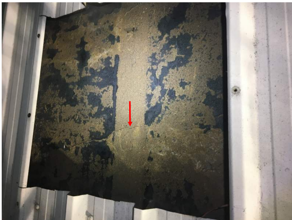
Photo S73: The counterweight concrete in the upper northeast corner has a wide crack but is otherwise in generally good condition (photo by Gemtec).
