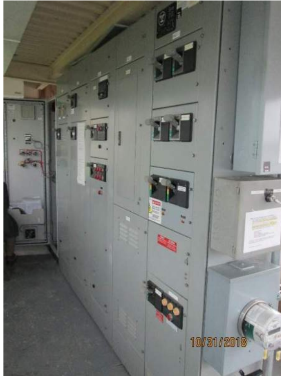
Photo E5: Motor Control Centre (MCC). The bridge is provided with a motor control center (MCC) for bridge power distribution. The MCC is located inside the operator’s control house. The MCC was installed in 1994 and is in good serviceable condition.
