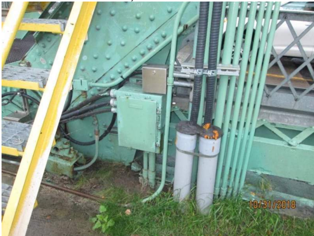
Photo E40: General Outdoor Installation. The bridge outdoor installation generally consists of Teck cable, painted RGS conduits, and stainless-steel junction boxes. The installation is generally in good serviceable condition but with some of the cable/conduit support brackets exhibiting moderate signs of corrosion.
