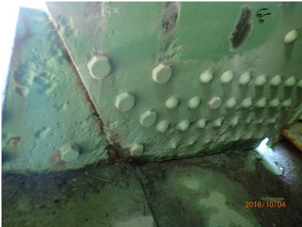
Photo S47: Severe pitting at the base of the interior face and rivet heads of the south plate of the south trunnion.
