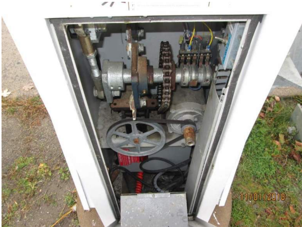
Photo E27: Typical Traffic Gate Housing. The motor starter is located inside the gate housing. Note that no door limit switches have been provided to prevent gate operation when the gate door(s) are open for maintenance or troubleshooting but a sign has been installed to indicate that the gate is powered and should be disconnected at the MCC prior to maintenance being performed. Also note no hand crank limit switch has been provided in accordance with code.
