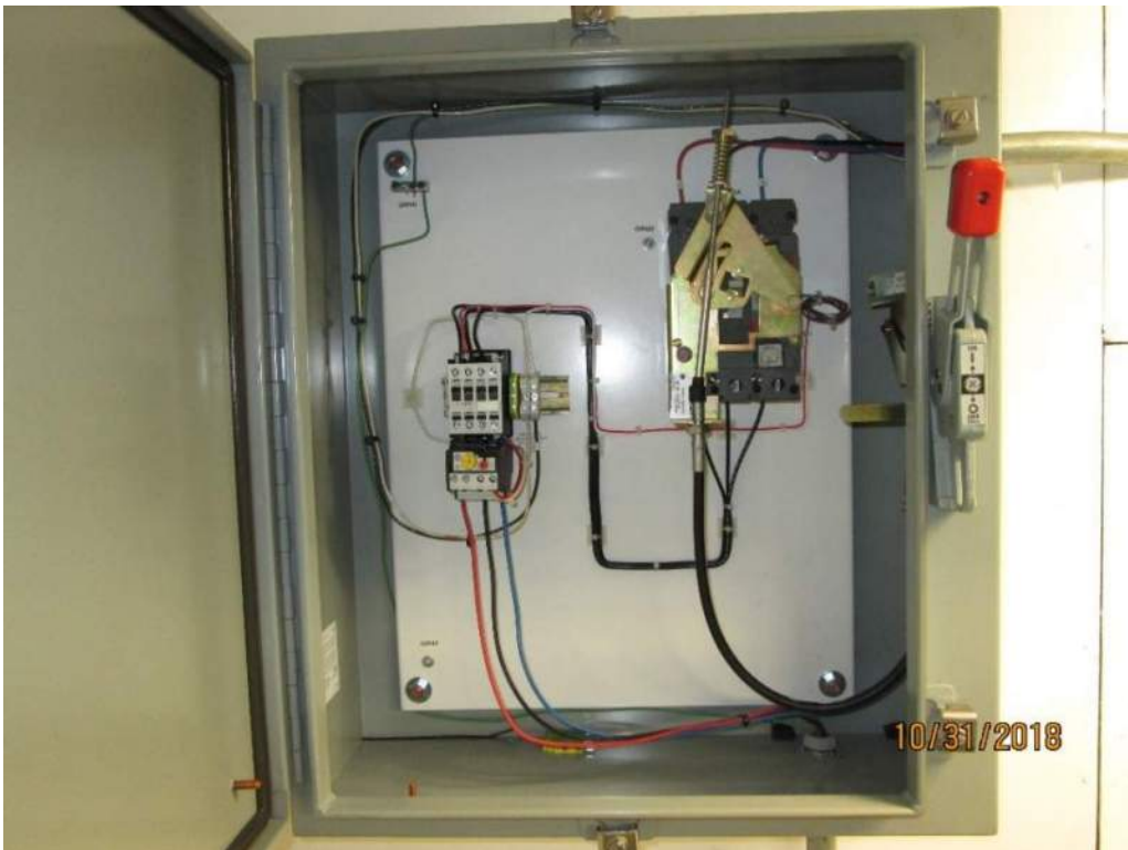
Photo E14: Motor Brake Disconnect and Starter enclosures. New motor brake starters were recently installed in the bridge machinery space and are in excellent condition. The MCP of the motor brake starter also serves as the local disconnect switch. The wires in the enclosure have not been labelled to aid troubleshooting.
