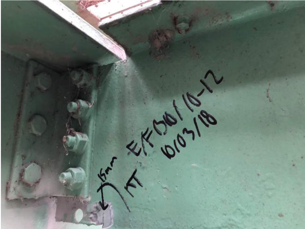
Photo S54: 15mm notch/crack in the bottom cope of Stringer E (FB10-FB12) at FB10 (photo by Brouco NDT).
