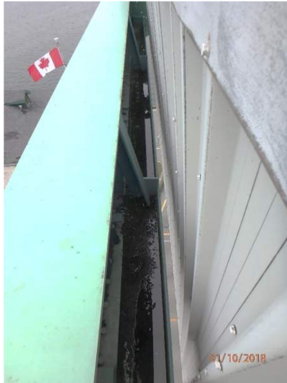
Photo S40: Debris and water are collecting on member 26N-26S.
