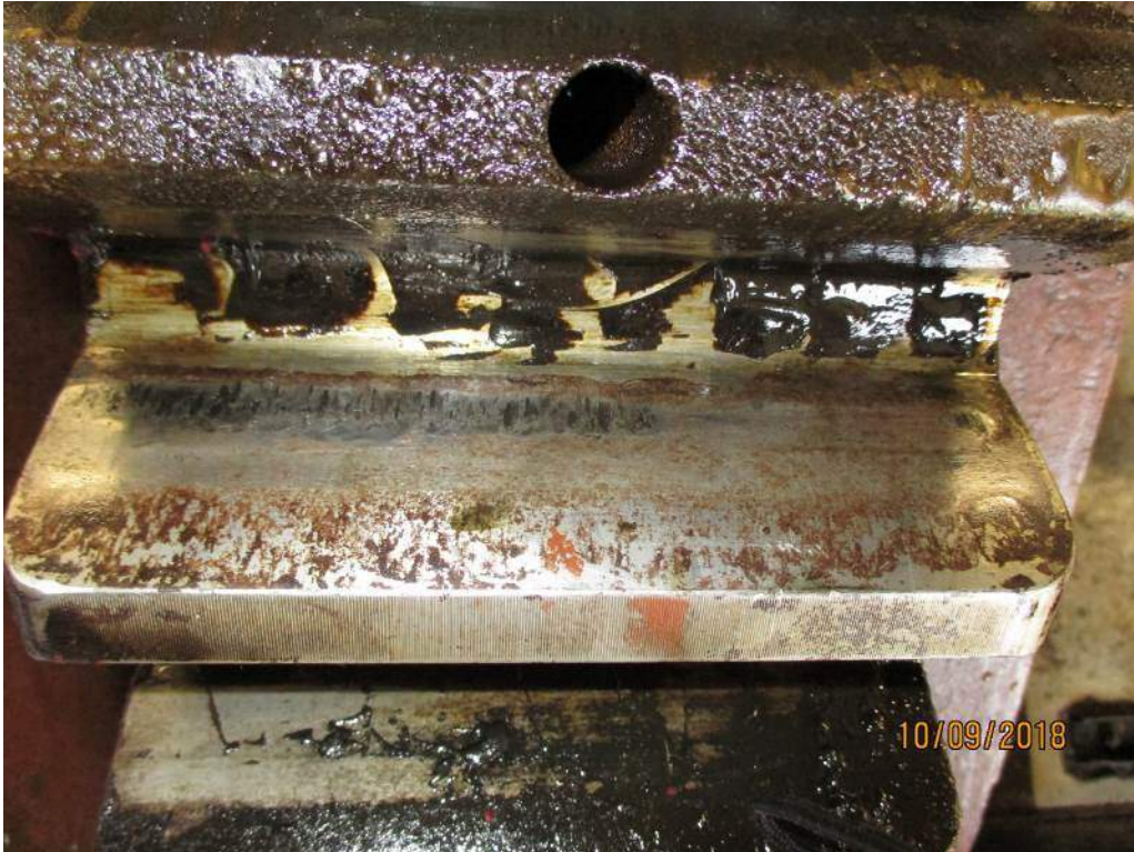
Photo M5: Span Drive Machinery Gear D. Note the light damage on the south side of the closing face of this gear.
