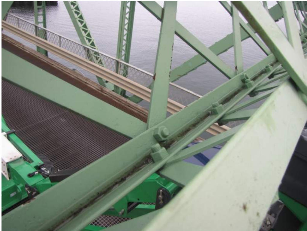
Photo S94: The lower angle of portal truss member 1S-1N is holding water.
