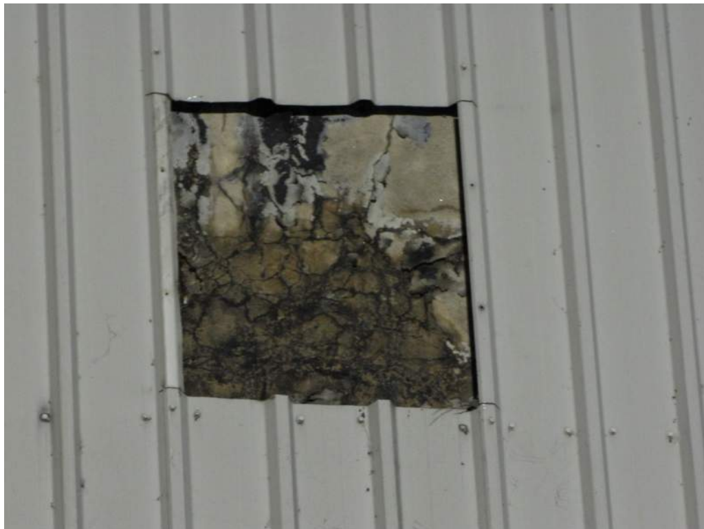
Photo S75: The counterweight concrete in the lower northwest corner exhibits widespread wide map cracking and a wet area.
