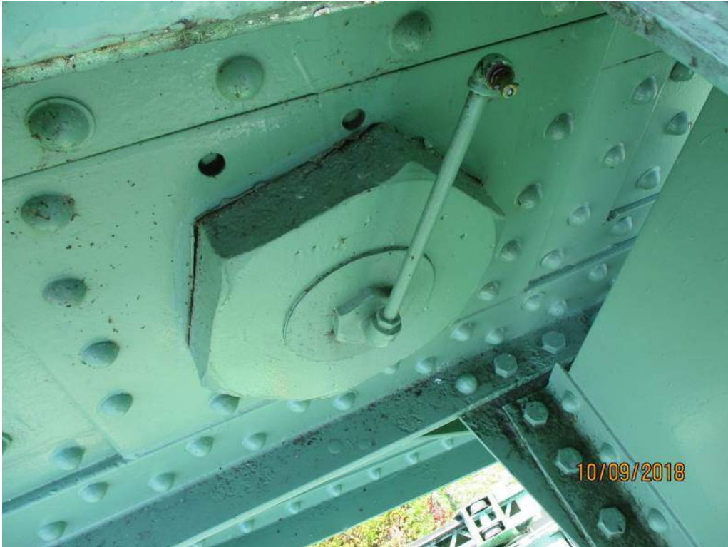
Photo M15: South First Link Pin. There is cracked paint and fretting between the nut and the structure indicating slight movement.
