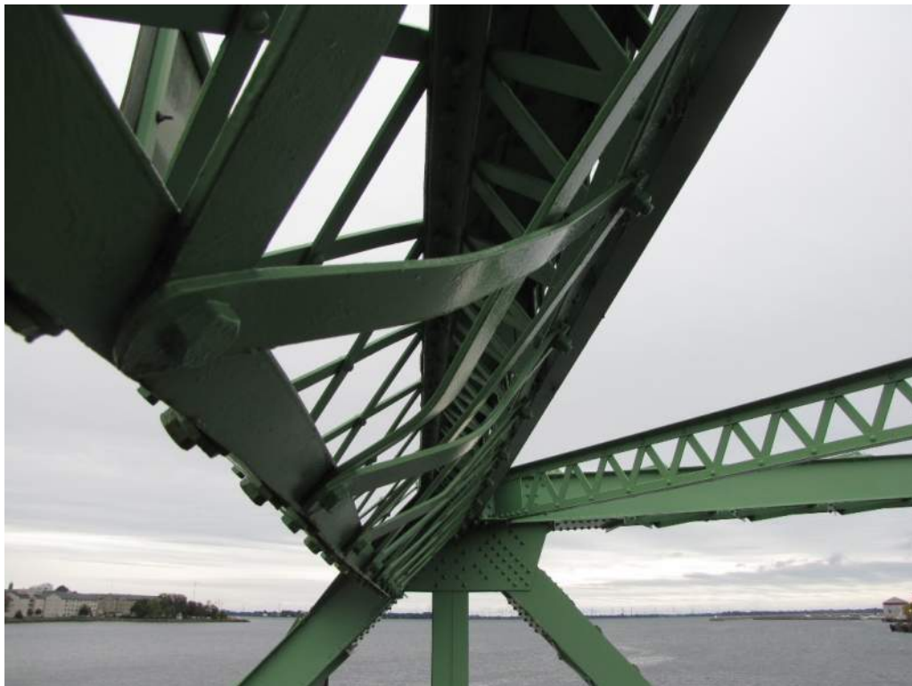
Photo S93: Six lattices in portal truss member 1S-1N are bent, likely due to vehicular impact of the bottom angle.
