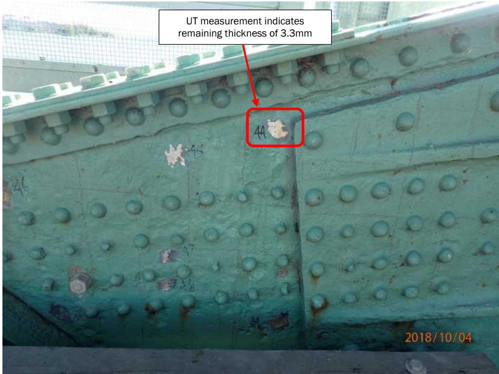
Photo S48: The north (roadway) side of the south trunnion has widespread pitting in the collar plate (right side), connection plate (left side) and some rivet heads.
