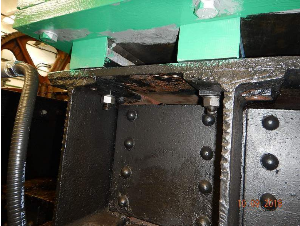
Photo M3: Span Drive Machinery South Motor. The underside of the motor mounting support is unpainted. The span drive north motor is similar. View Photo M4 for a detailed view under the mounting plate.
