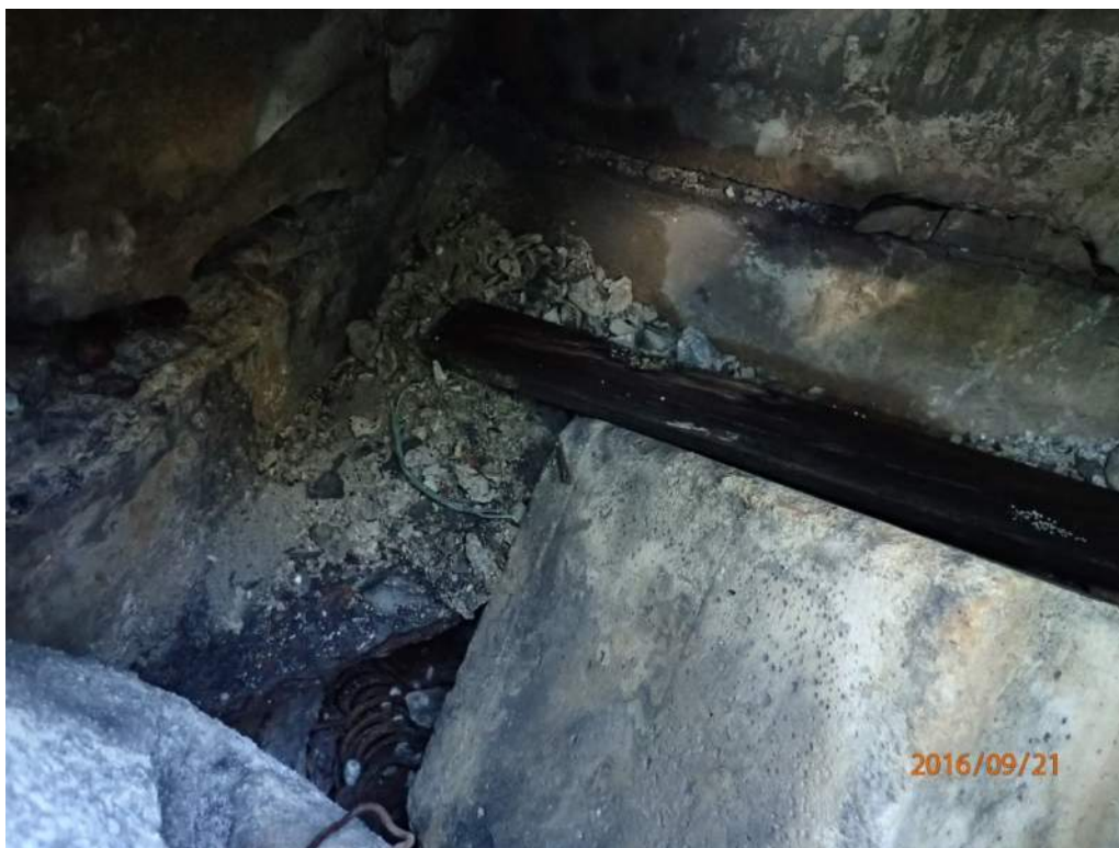
Photo S67: The concrete in the two upper chambers in the top face of the counterweight exhibits spalls, disintegration, and wet areas (2016 photo).
