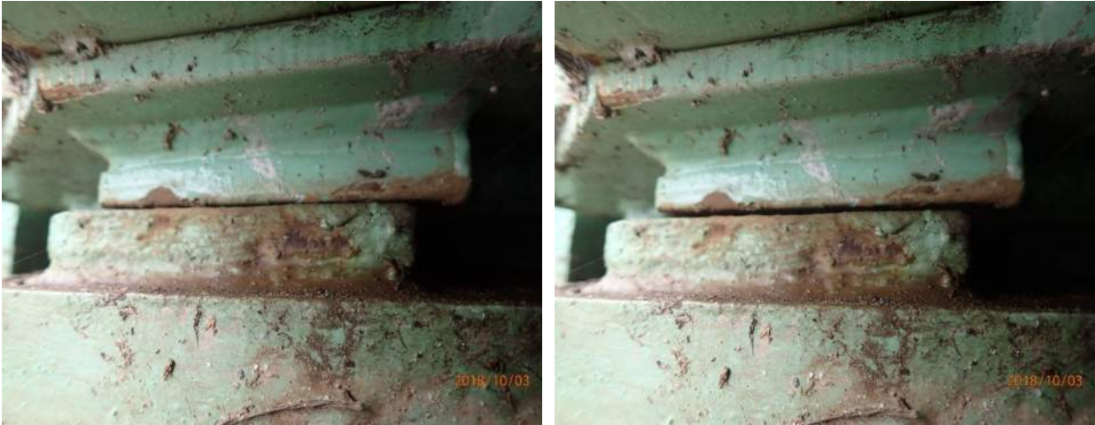
Photo S110: The leaf span is not fully seated on the northeast live load support (right) and only seats fully when vehicles are on the east end of the deck (left).
