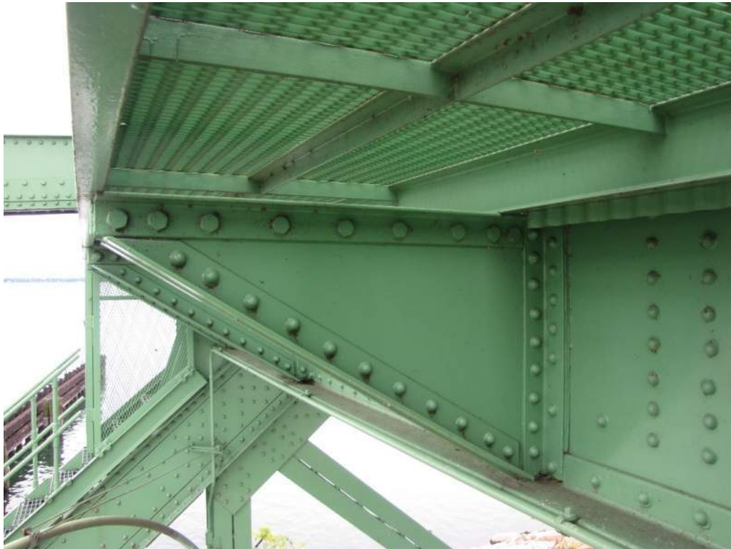
Photo S118: The east C-channel supporting the catwalk outside the mechanical room is supported by the tapered cantilevered members below but only 25mm of the bottom flange is actually supported.
