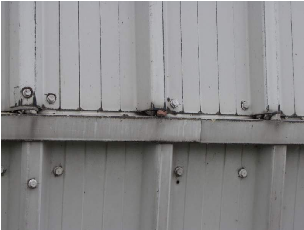
Photo S63: Gaps in the counterweight panels are permitting smaller pieces of aggregate from the disintegrated counterweight concrete to fall onto the roadway below.
