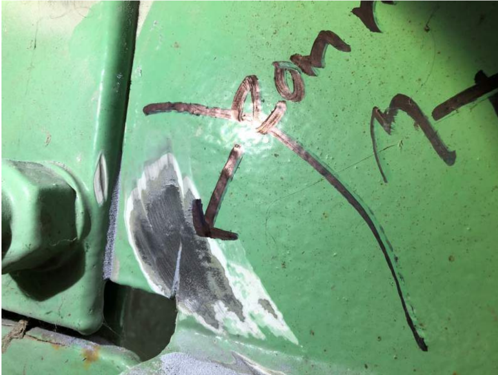
Photo S56: 20mm notch/crack in the bottom cope of Stringer E (FB14-FB16) at FB14 (photo by Brouco NDT).
