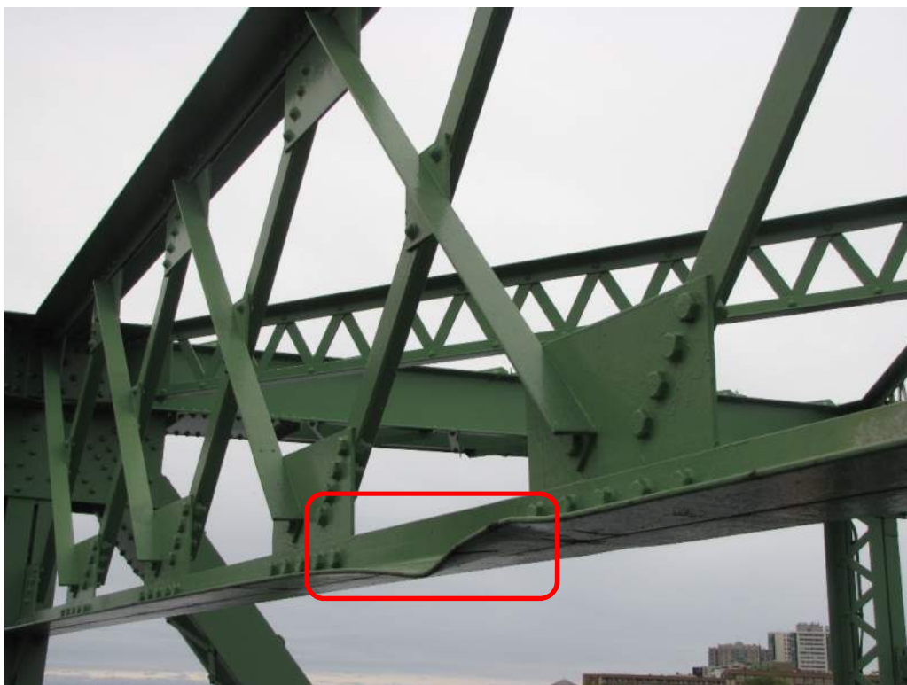
Photo S95: Severe impact damage to the bottom east angle of sway brace member 5S-5N.
