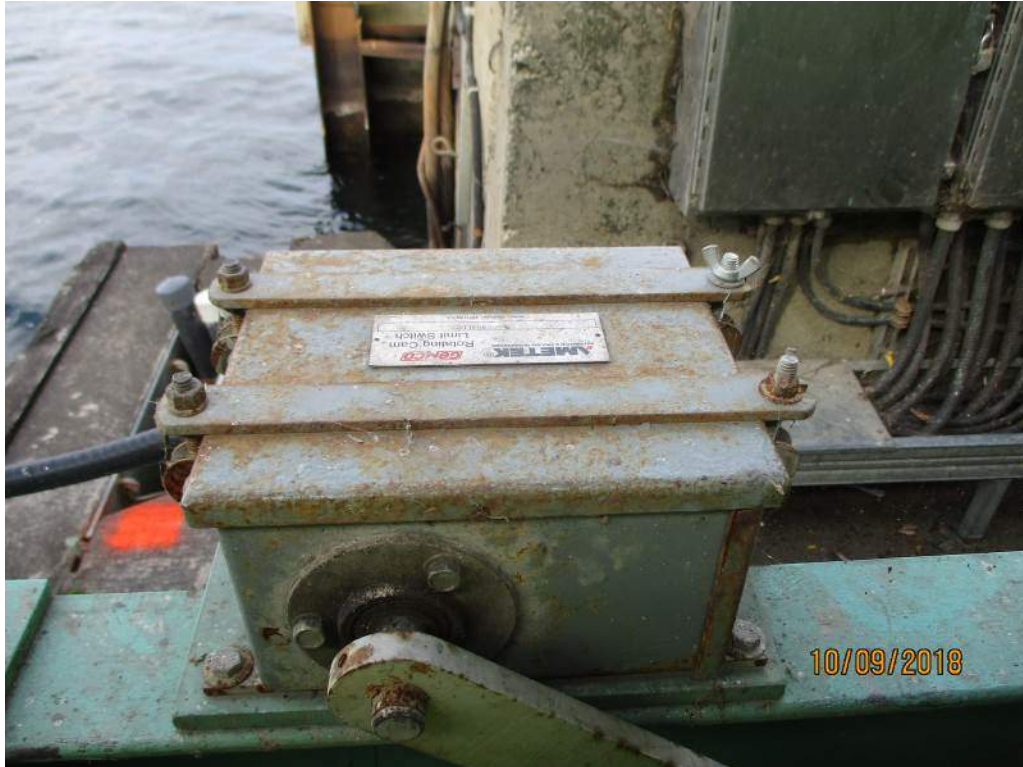
Photo M23: North Span Lock Rotary Cam. The rotary cam limit switch cover exhibits paint deterioration and light corrosion.
