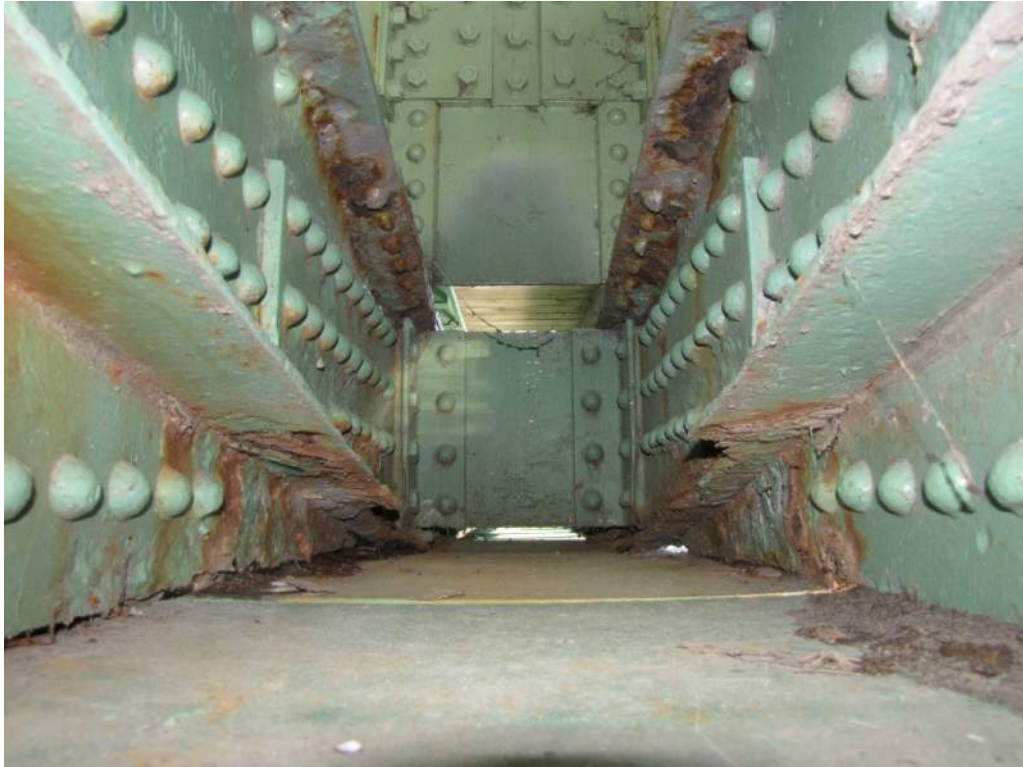
Photo S20: Severe localized pitting and section loss of flanges where 14S-16S and 14S-15S intersect. Several rivet heads have over 75% section loss.
