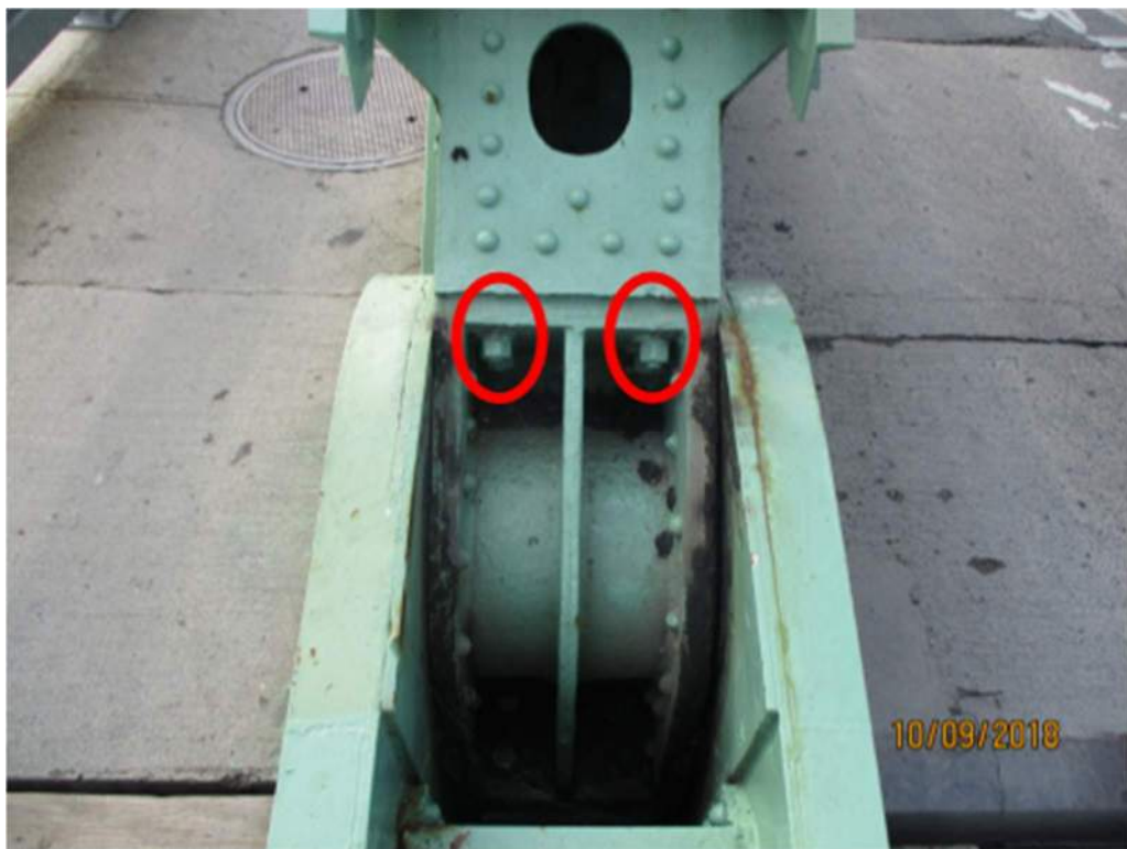
Photo M12: South Main Trunnion Bearing. The head end of the four bolts that secure the bearing housing to the structure has 100% section loss due to corrosion. The nut end of these bolts (circled) are pictured in this photo.
