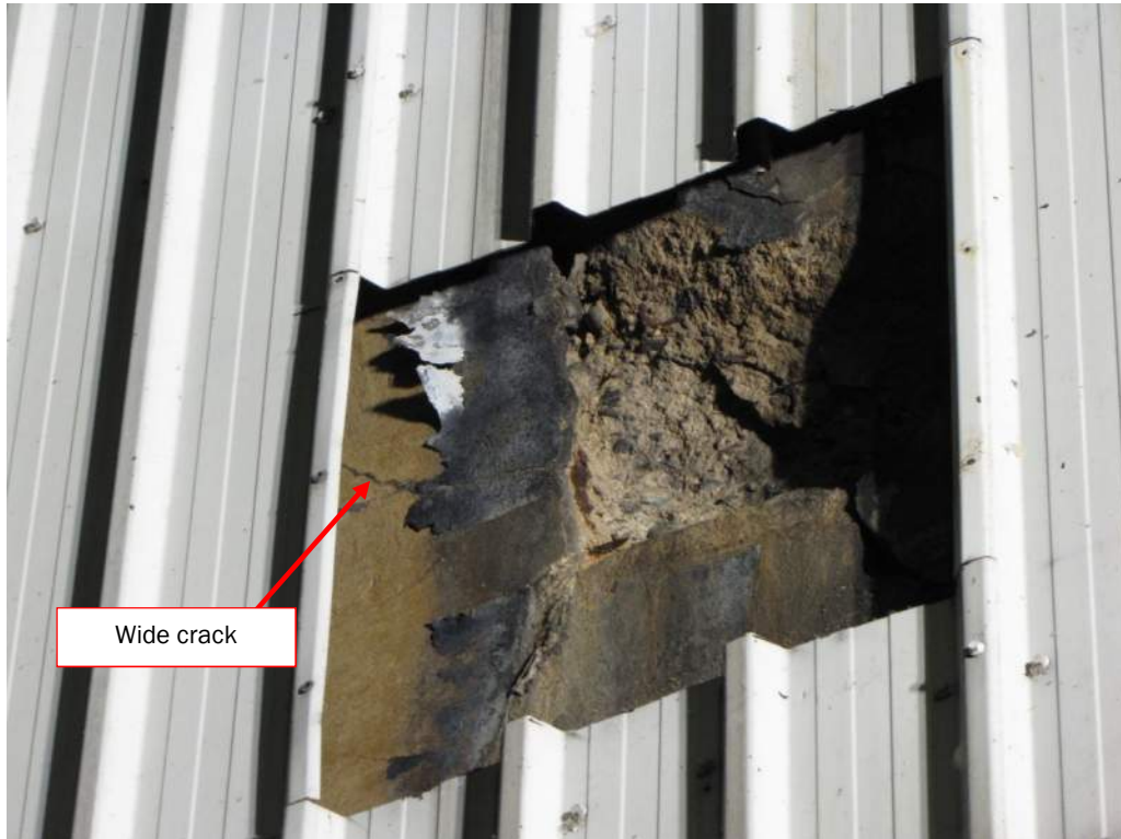
Photo S72: The counterweight concrete in the lower northeast corner has a severe spall/disintegration and a wide diagonal crack that extends at least 2 metres.
