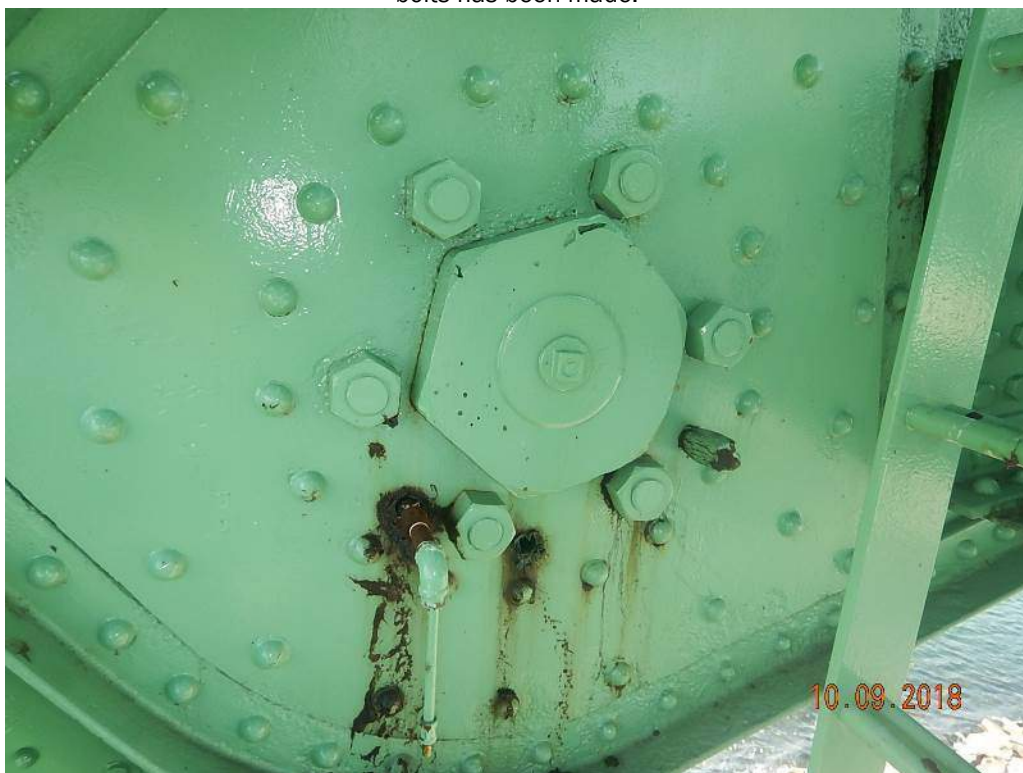
Photo M14: South Counterweight Trunnion Bearing, Inboard Side. All of the sleeve stud nuts are either not tight or show signs of movement. The east lubrication line has evidence of leakage, the center lubrication port has shear off, and the west lubrication port is plugged.
