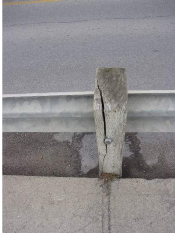
Photo S114: A timber post in the southwest guiderrail has been split by vehicular impact.
