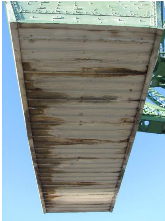
Photo S62: The panels on the underside of the counterweight have widespread corrosion and wet areas/stains.
