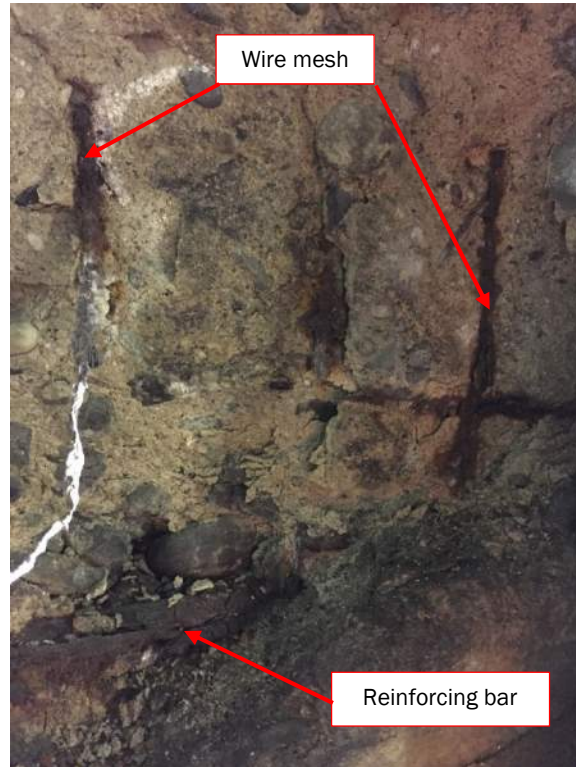
Photo S70: The counterweight concrete in the lower northeast corner exhibits a very severe spall/disintegration, delaminated areas, and exposed and corroded reinforcing bars and wire mesh.
