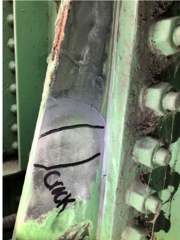
Photo S50: Crack in southwest vertical gusset plate at 2N (photo by Brouco NDT).
