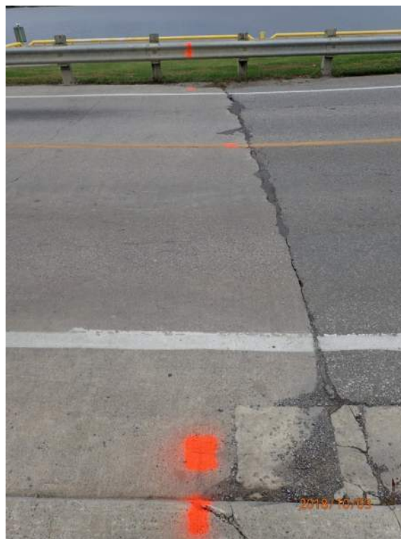
Photo S113: There is a wide crack and patched potholes at the interface between the east approach slab and adjacent roadway wearing surface.
