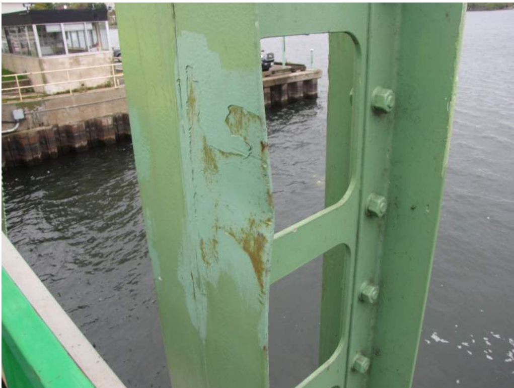
Photo S27: Impact damage to vertical member 9N-10N has bent a portion of the southeast flange.
