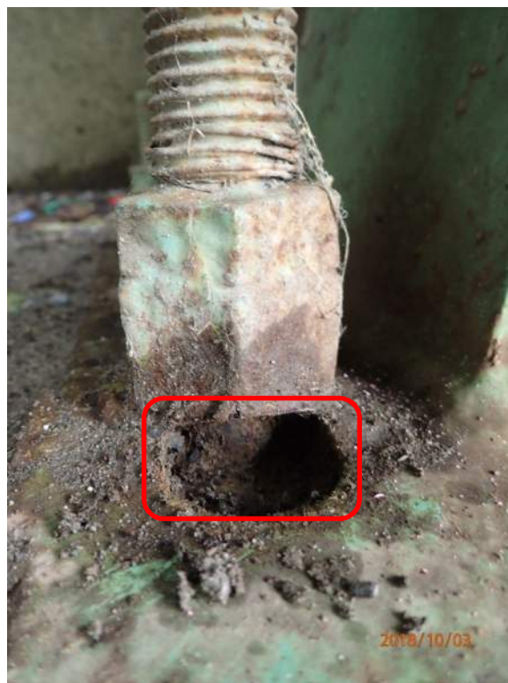
Photo S109: The northwest anchor bolt of the southeast live load support is bent and exhibits medium to severe corrosion.
