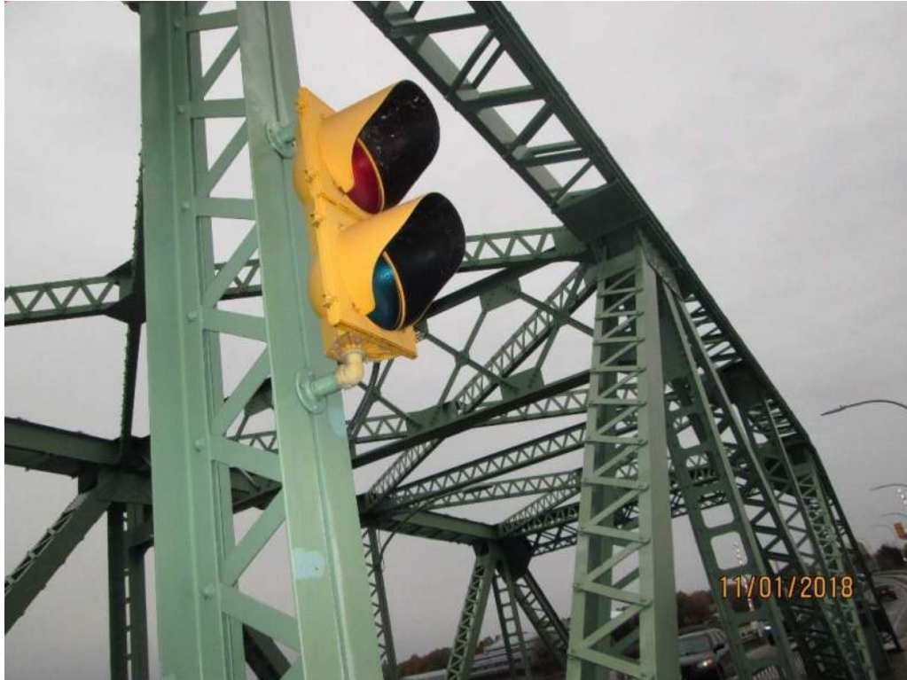
Photo E29: Typical Span Navigation Light. Note that roadway type lights are being used. The location of the navigation lights does not provide marine traffic with a clear visual indication as to when the span has been raised and it is safe to proceed.
