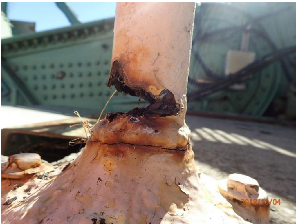
Photo S105: Two of the railing posts between the north trunnion and the control room are perforated at the base (north post shown, south post similar). These posts were subsequently repaired in October 2018.
