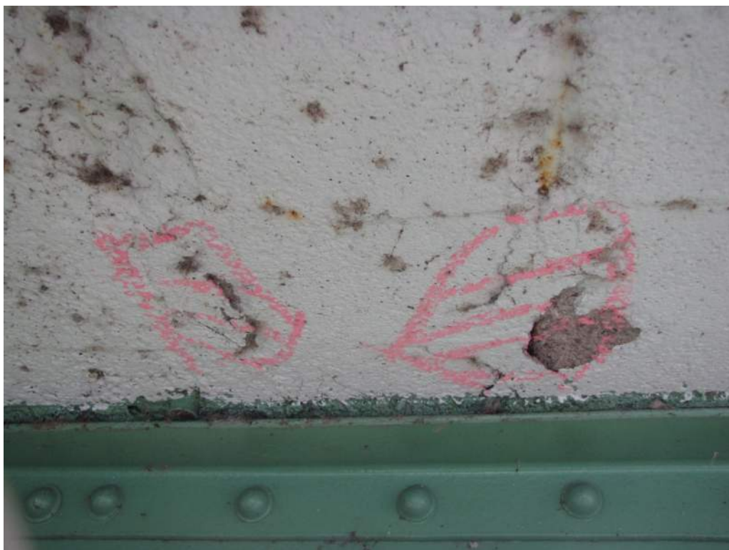
Photo S101: The mechanical room soffit exhibits several spalls and delaminated areas. Scaling of the delaminated areas is recommended as they are located over the roadway.
