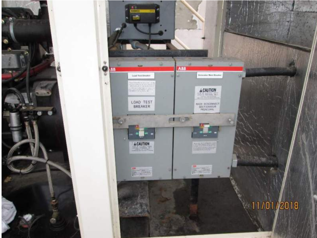
Photo E3: Standby Generator Breakers. The standby generator is provided with a 60A main disconnect breaker and a 60A load test breaker. Note the generator is not provided with a load bank and the load test breaker is not connected.
