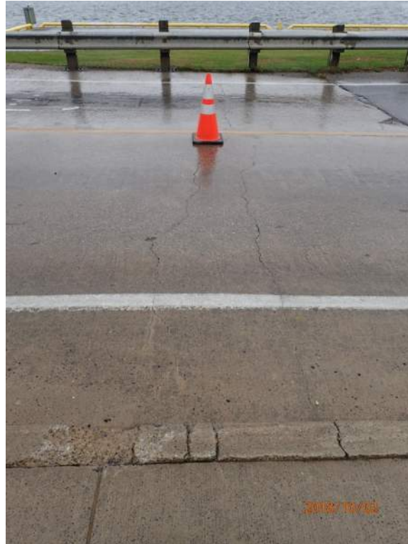
Photo S112: There are two wide cracks that extend across the full width of the east approach slab.
