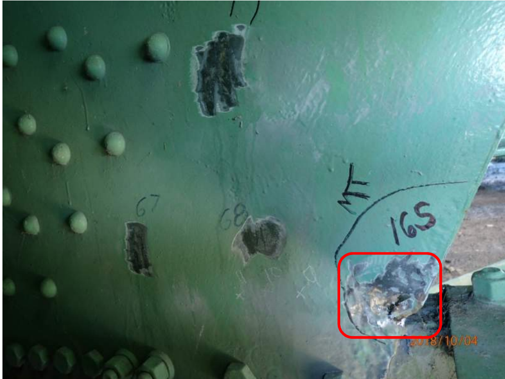
Photo S46: View of the interior of the north plate of the south trunnion below deck level. A crack was found at the perforation circled.
