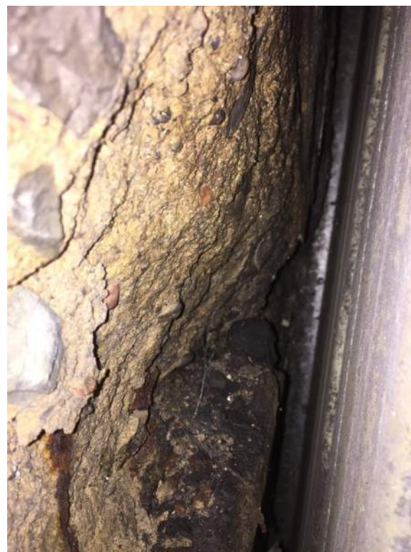
Photo S71: Very severe spall/disintegration of the counterweight concrete in the lower northeast corner (looking north).
