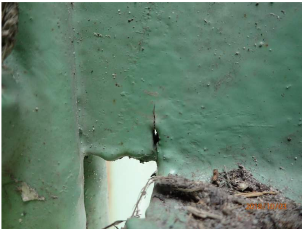
Photo S53: 15mm notch/crack in the bottom cope of Stringer E (FB0-FB2) at FB0.
