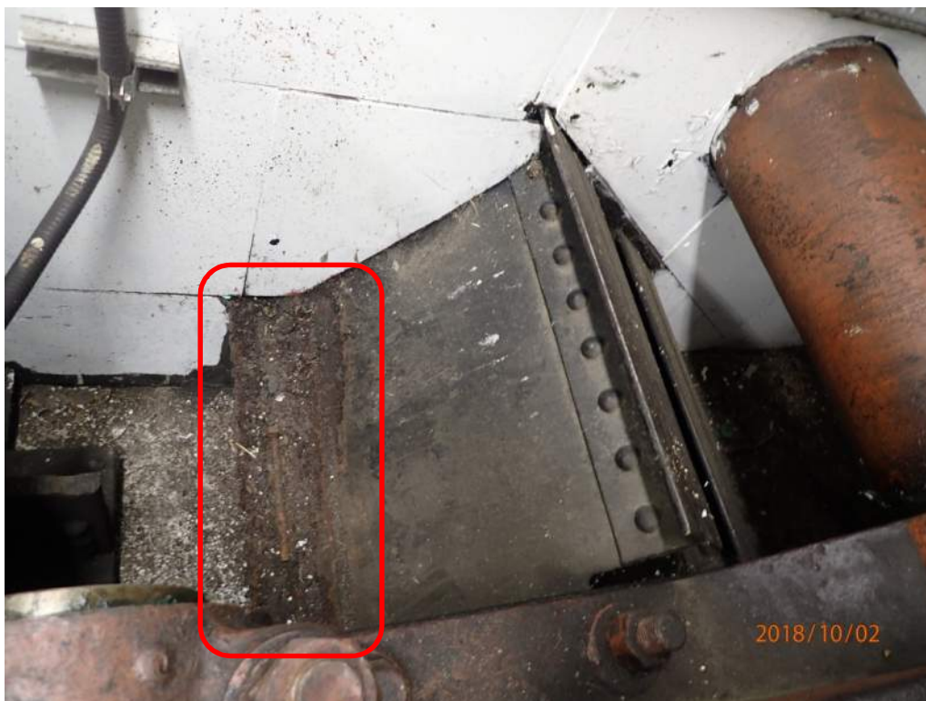
Photo S41: Severe corrosion on the bottom flange of the northeast transverse strut in the mechanical room.
