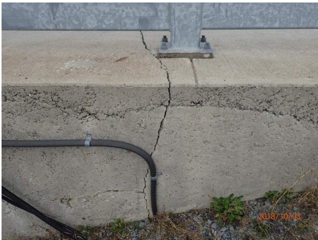
Photo S107: A wide crack in the southeast wingwall extends across the sidewalk.
