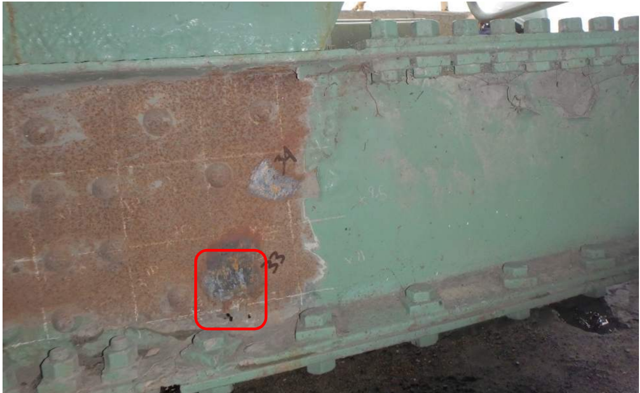
Photo S14: Perforation in the web of bottom chord member 14N-16N near node 16N and generalized light corrosion.
