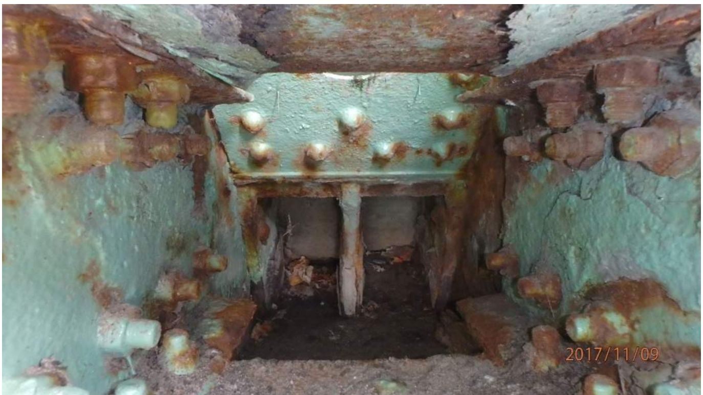
Photo S91: View of the west side of the south trunnion. Note the severe corrosion of member 15S-18S (photo from 2017 inspection).
