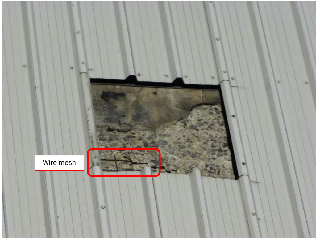
Photo S76: The counterweight concrete in the upper northwest corner exhibits a large area of disintegration, delaminated areas, and exposed and corroded wire mesh.
