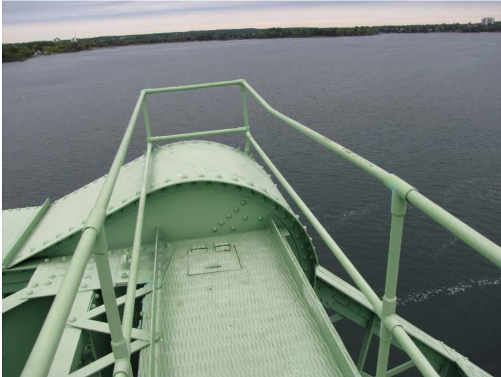
Photo S120: Bent catwalk safety railing above node 22N.
