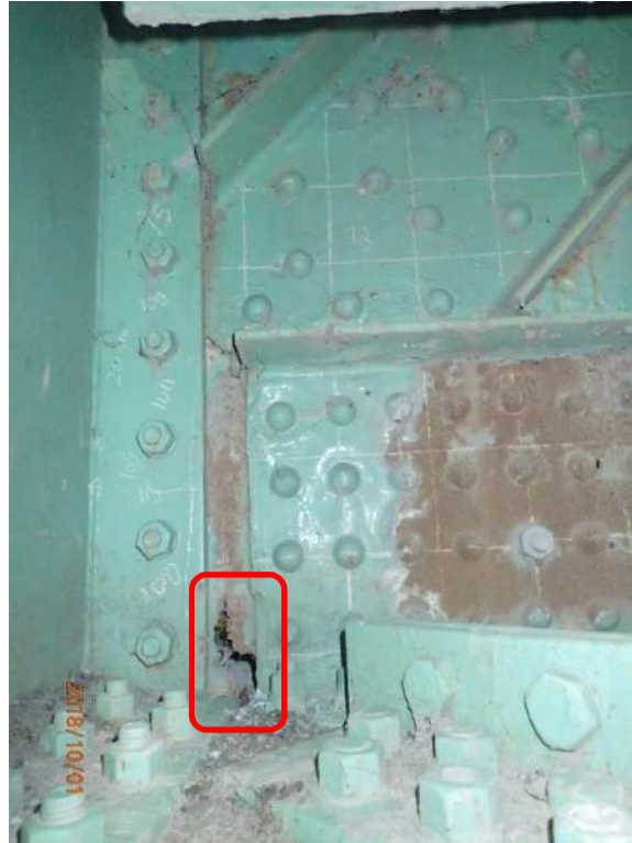
Photo S42: The interior vertical gusset plate at node 16N exhibits severe section loss and a perforation with a crack.
