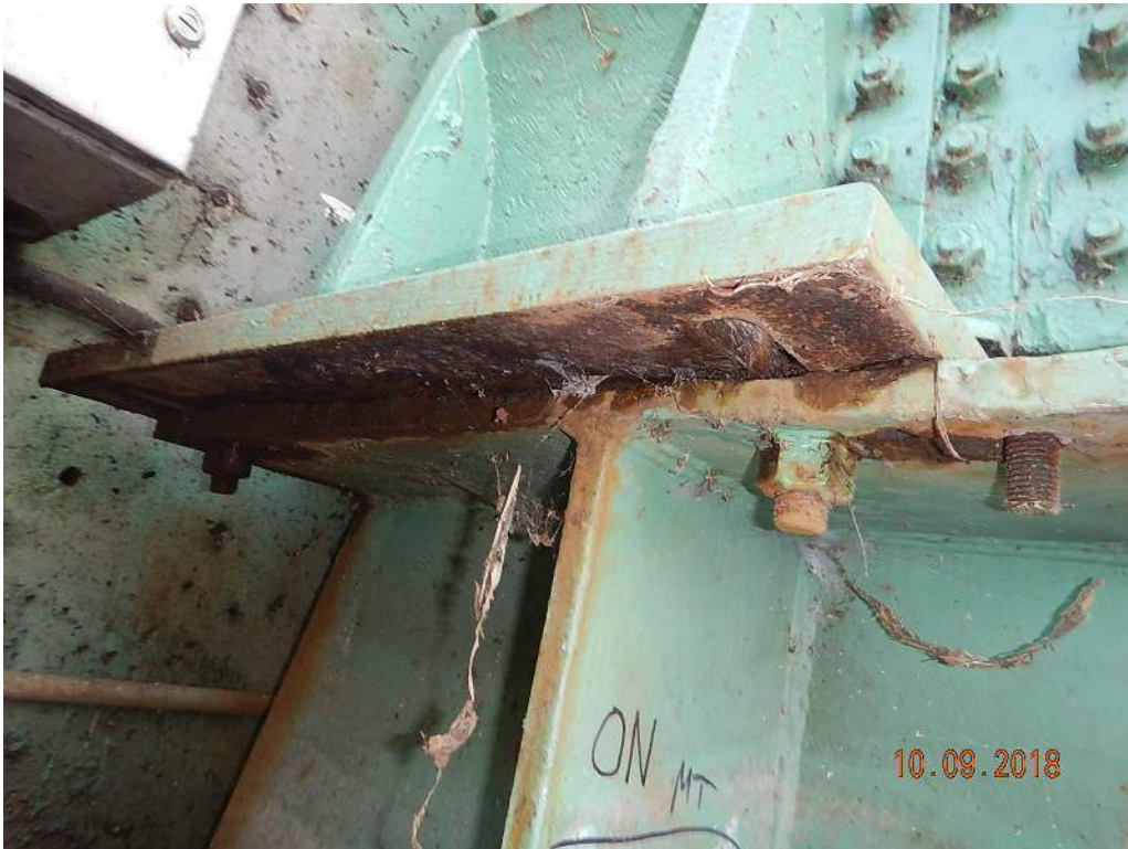
Photo M25: North Live Load Strike Plate. The underside of the strike plate support and mounting bolts are corroded. The south live load strike plate assembly is similar.
