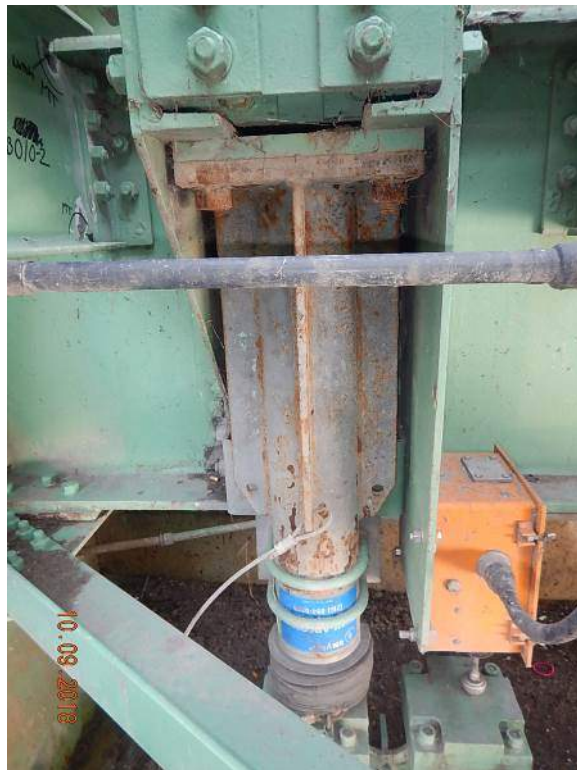
Photo M26: South Buffer. General View of the buffer, strike plate and seated limit switch. Note, the cylinder body has light to moderate spotty corrosion. The north buffer is similar.
