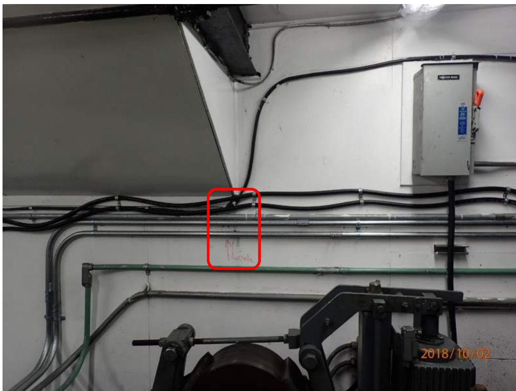
Photo S103: Water was leaking into the north side of the mechanical room during the inspection.
