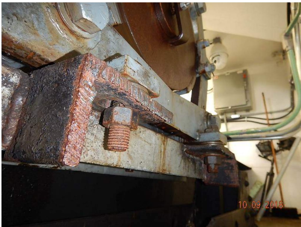
Photo M2: Span Drive Machinery Brake. The north east mounting bolt nut has poor bearing. The mounting bolt and surrounding areas are lightly corroded.
