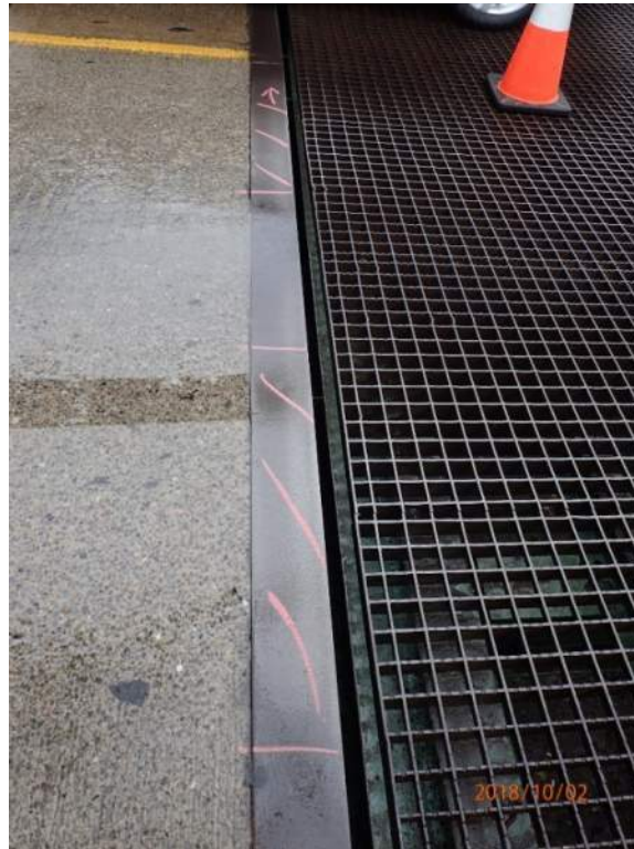
Photo S104: Areas of the west joint armoring sound hollow when tapped, indicating a void between the angle and underlying concrete.
