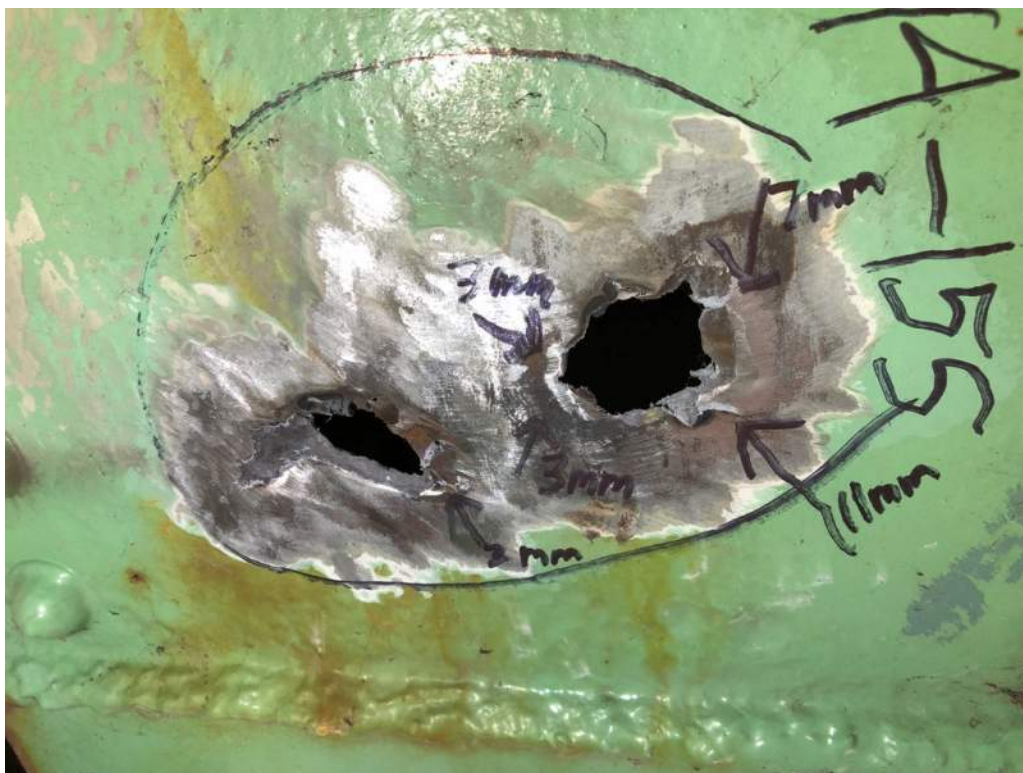
Photo S21: Perforations and cracks in bottom batten plate of bottom chord member 14S-15S near node 15S. The cracks range in length from 3mm to 11mm (photo by Brouco NDT).
