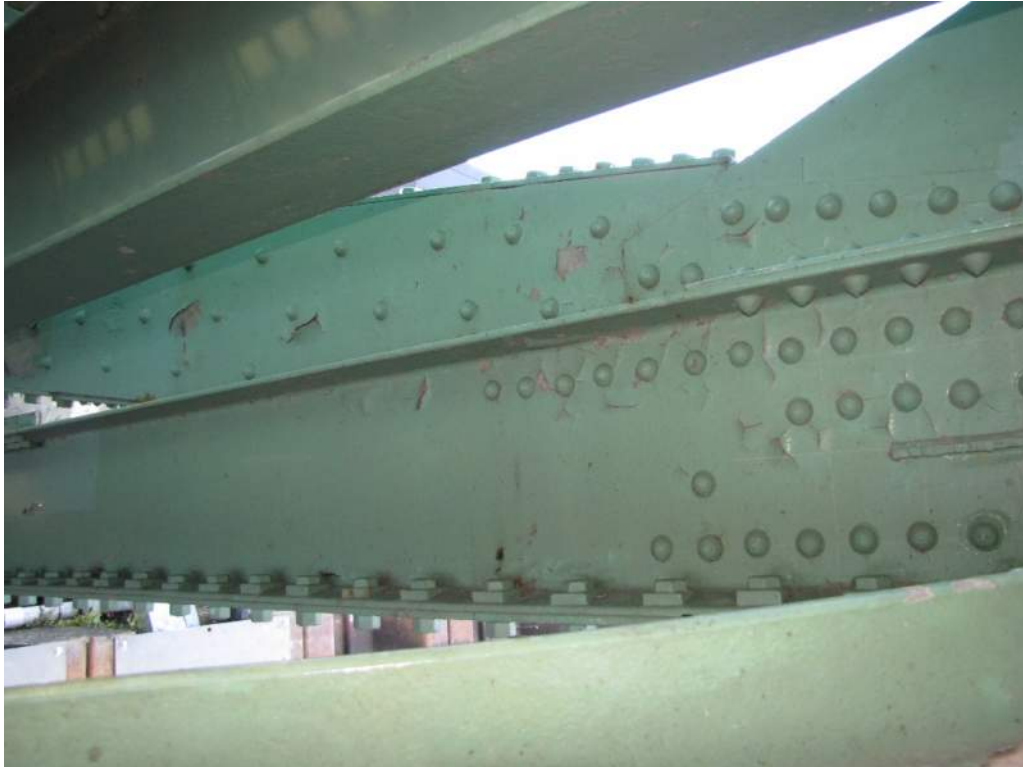
Photo S82: The painted coating is cracking and peeling off at several locations on the structure (members 14N-15N and 14N-16N shown).
