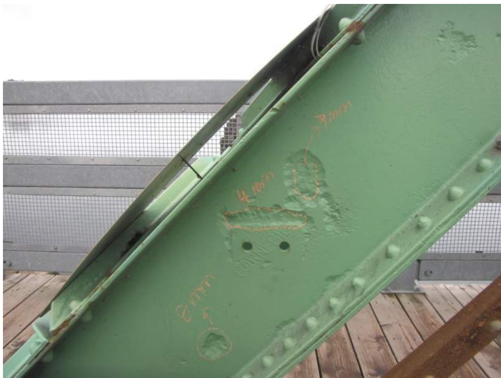
Photo S11: Localized severe pitting in north web of top chord member OS-1S.
