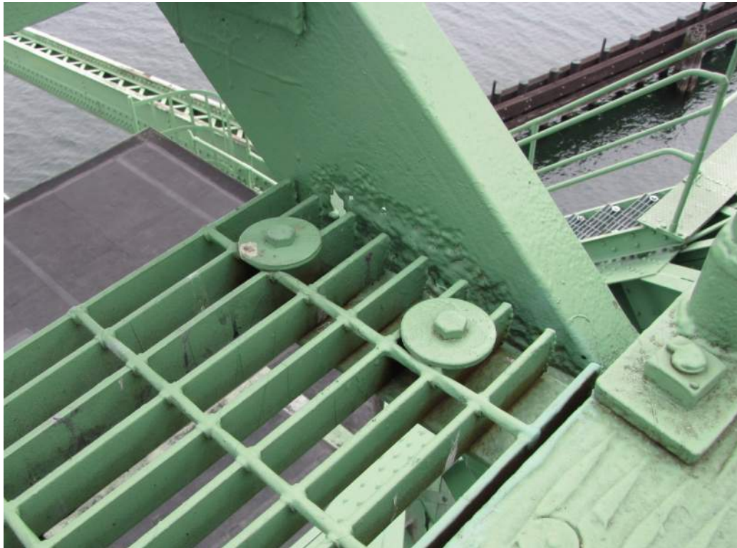
Photo S122: Severe pitting and perforation in south channel at bottom step of catwalk stairs from 21-22.
