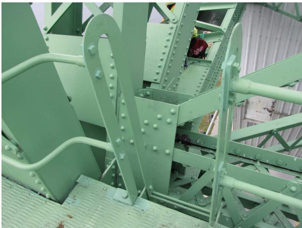
Photo S119: There are no safety chains across the two open sections of the west railing on catwalk 21N-21S which is a potential failing hazard (south side shown).
