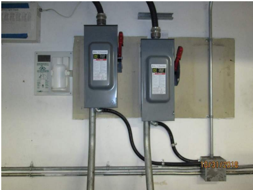
Photo E10: Span Drive Motor Disconnects. The span drive motors are provided with local disconnect switches as per Canadian Electrical Code. These disconnect switches were installed as the same time as the new drive motors and are in as new condition.
