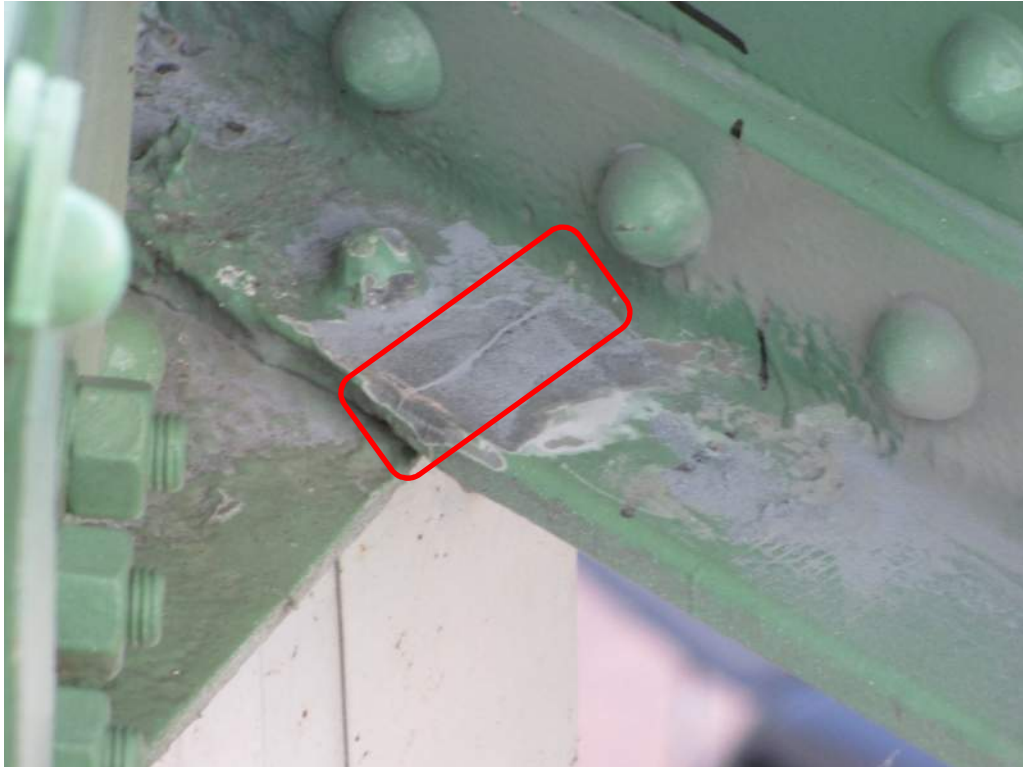
Photo S38: Crack across full width of bottom leg of interior angle of 21N-27N counter weight truss member at node 27N.
