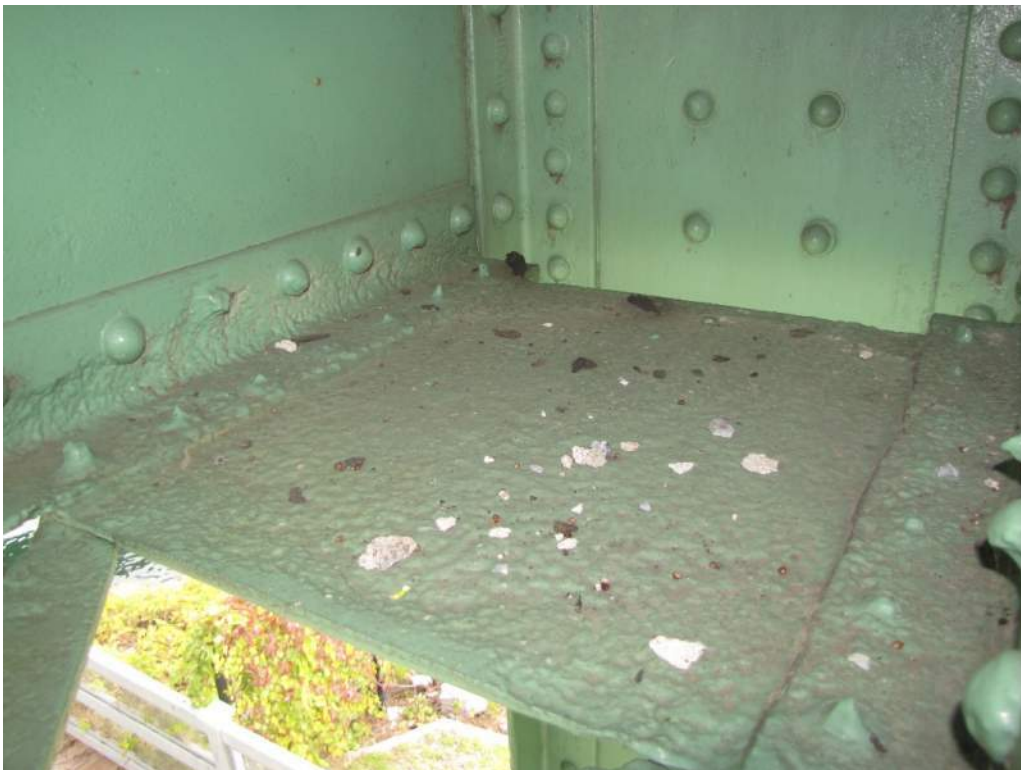
Photo S97: Tower truss sway bracing member 20N-20S has deep pitting in the bottom gusset plate and severe section loss of the rivet heads at node 20S.
