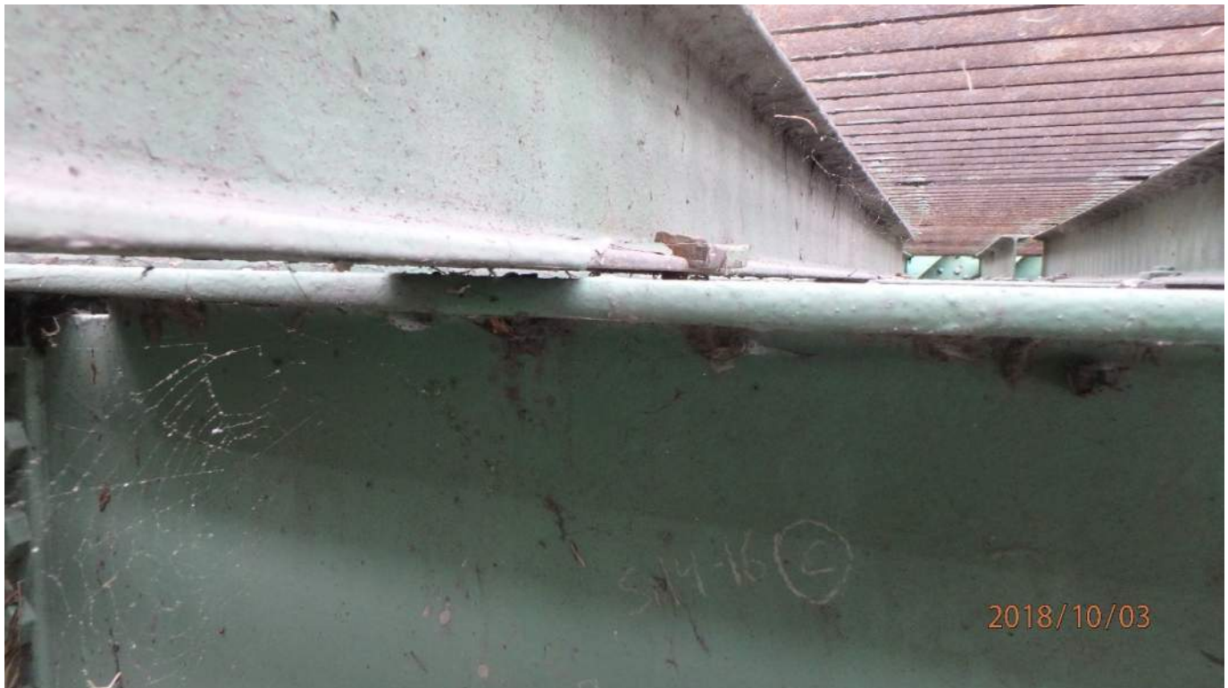
Photo S59: Multiple sills in bay 14-16 are not bearing on the stringers below.
