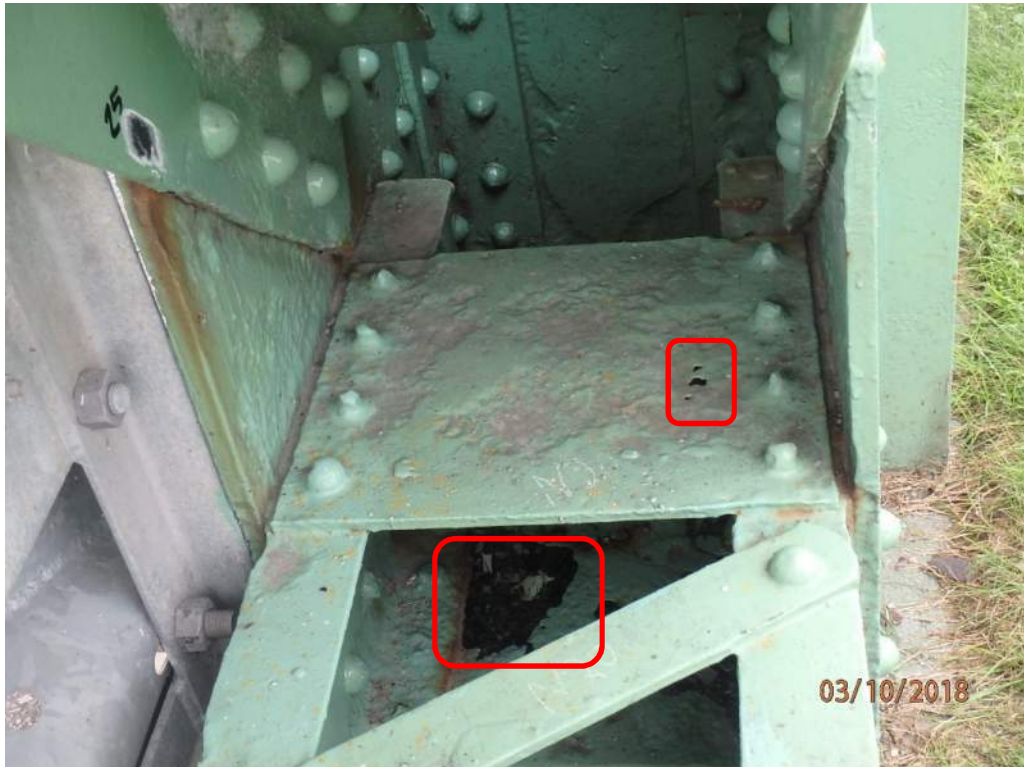
Photo S34: Perforations in upper and lower batten plates of bottom chord 18N-19N at node 19N.
