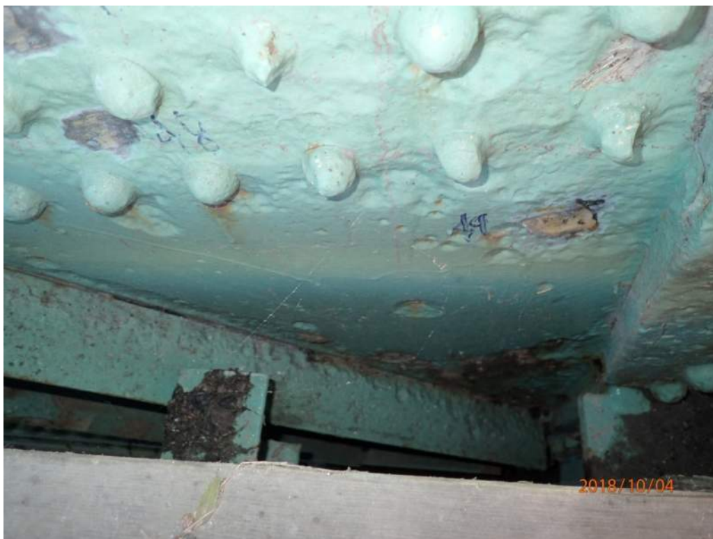
Photo S49: The north (roadway) side of the south trunnion has widespread pitting in the collar plate (not shown), connecting plate, and some rivet heads.
