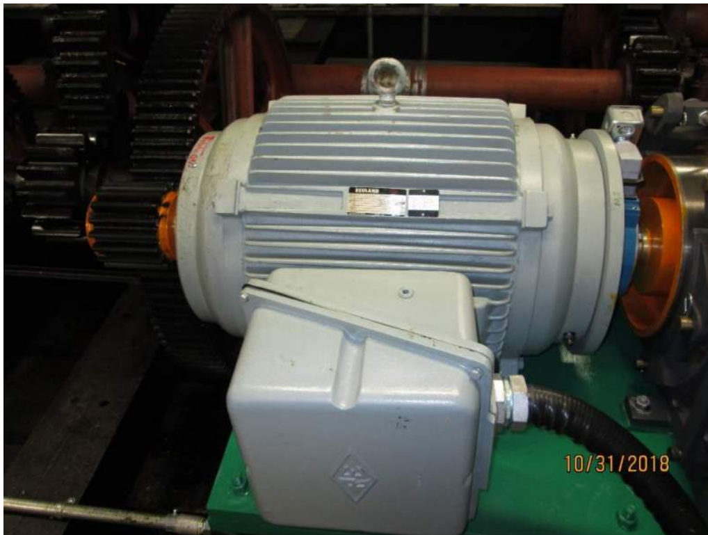
Photo E8: Typical Span Drive Motor. The bridge is provided with two span drive motors, the two motors can be configured to operate the span simultaneously or they can be configured to operate the span individually. These span drive motors are squirrel-cage induction type and replaced the original wound rotor motors when the new VFD drives were installed.
