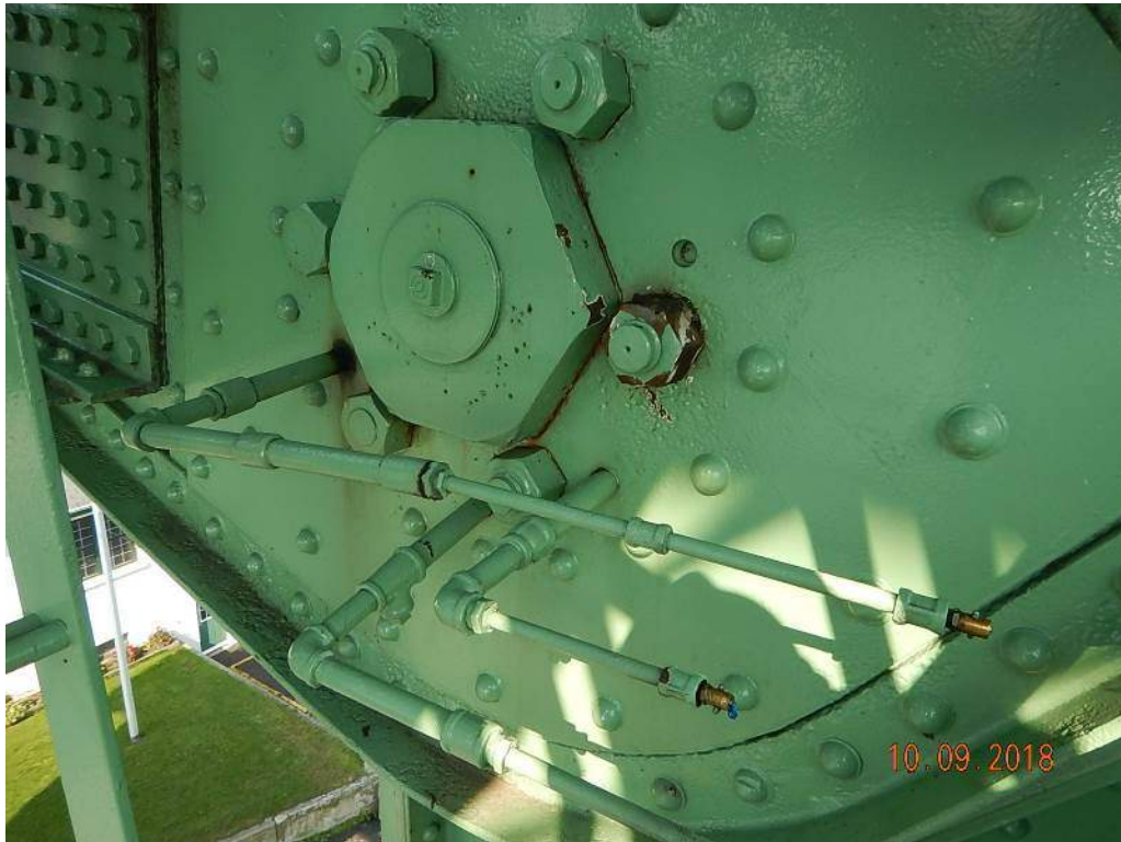
Photo M13: North Counterweight Trunnion Bearing, Inboard Side. All of the sleeve stud nuts are either not tight or show signs of movement. Paint removal from some of the nuts shows that an attempt at tightening these bolts has been made.
