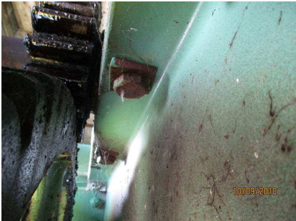
Photo M18: Span Lock Bearing B3. The span lock mounting bolt underside is not fully painted and corroded. The underside of bearing B4 mounting bolts are similar.
