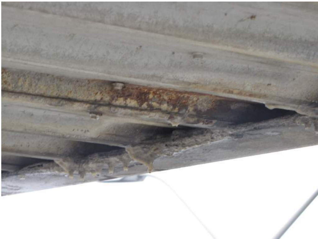
Photo S61: The underside of the east edge of the counterweight panelling is leaking and exhibits corrosion and efflorescence deposits.
