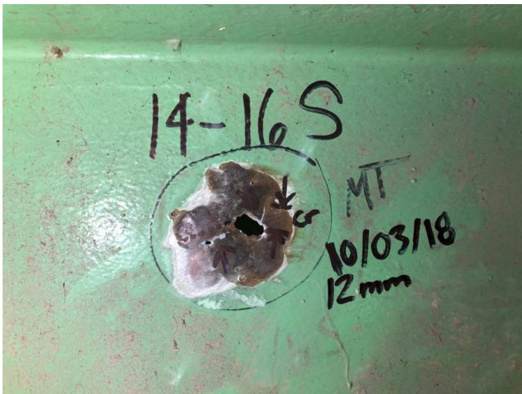
Photo S19: Perforation and 12mm long crack in interior channel of bottom chord member 14S-16S (photo by Brouco NDT).
