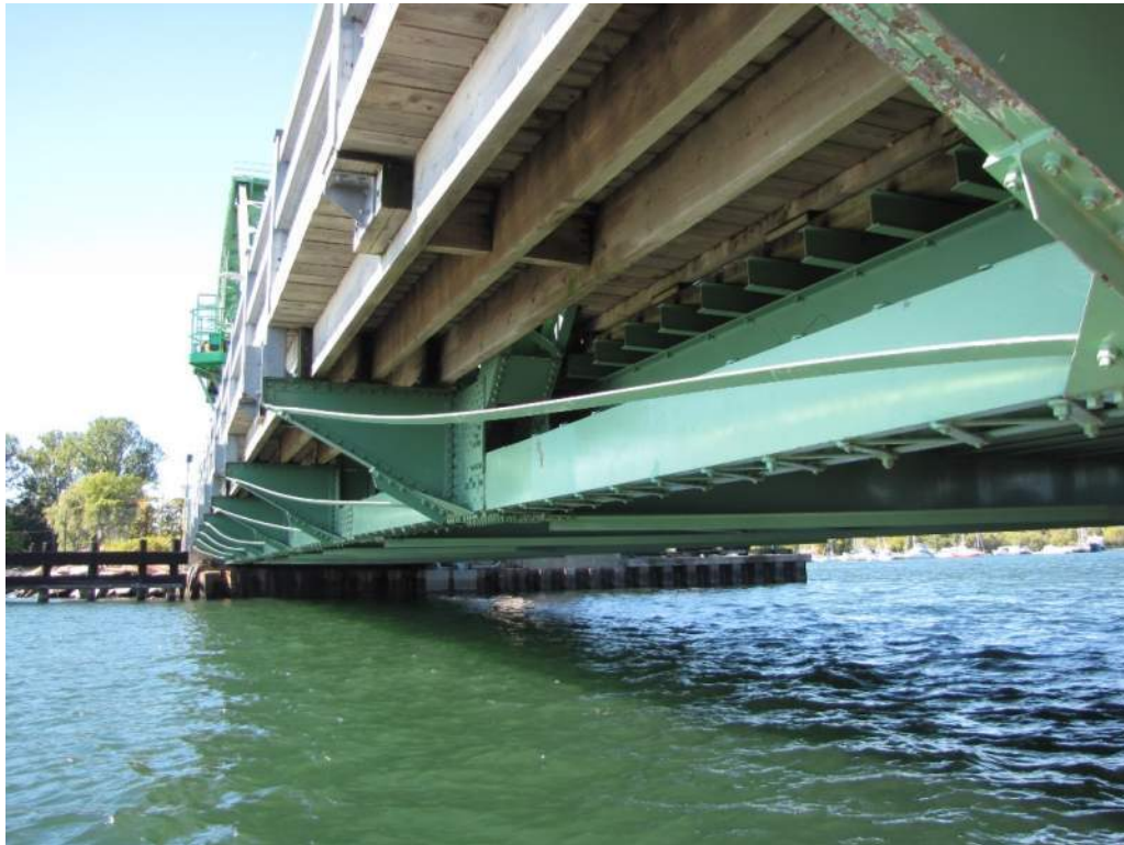
Photo S100: The bracing members that connect the cantilever sidewalk floor beams are typically sagging.
