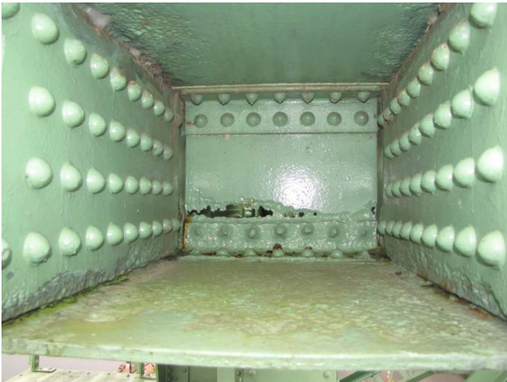
Photo S13: Perforation and severe pitting of diaphragm inside top chord member 11S-13S near node 13S.
