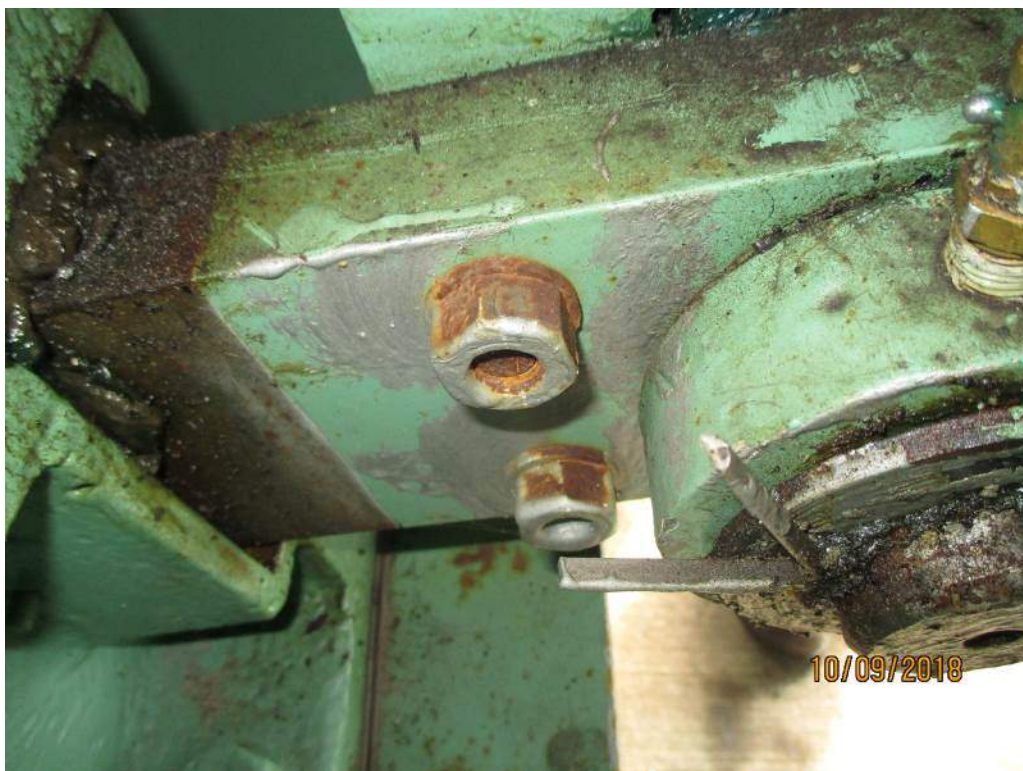
Photo M22: South Span Lock Crank Shaft CR2. The mounting bolts for the rotary cam position crank CR2 located on the lock bar are not fully painted and exhibit light corrosion. North Span Lock Crank Shaft CR2 is similar.
