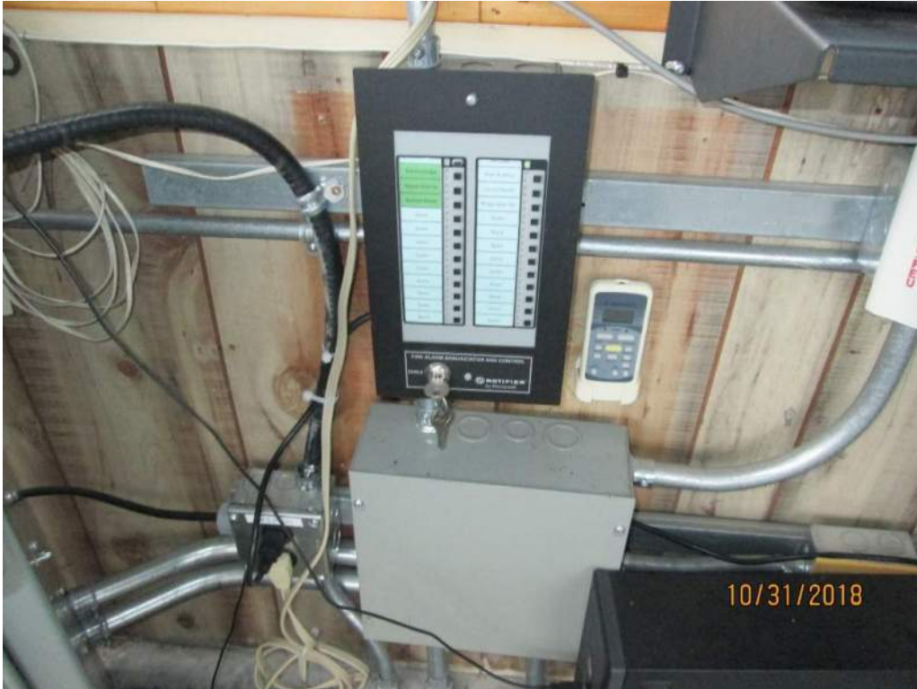
Photo E35: Fire Alarm System. The bridge is equipped with a fire alarm system. Fire detection devices are provided in the bridge maintenance building, the bridge control house and machinery space. The main fire alarm control panel is located in the bridge maintenance facility with a remote annunciator located in the bridge operators control house. All fire alarm equipment was in good serviceable condition at the time of the inspection.
