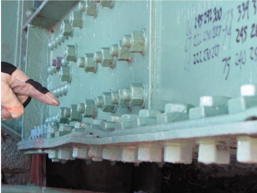
Photo S18: The top and bottom flanges of leaf truss bottom chord member 14S-16S have deformed near 16S.
