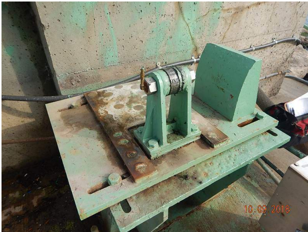
Photo M24: South Live Load Strike Plate. General view of strike plate and span lock receiver.
