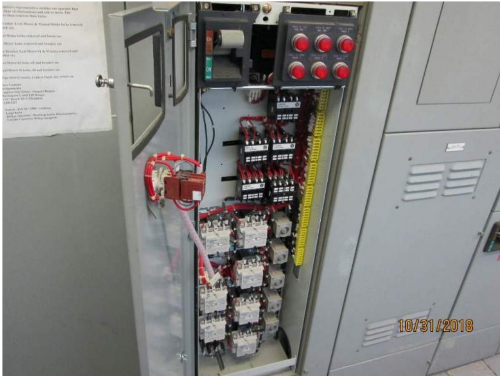
Photo E15: Span Lock Starter Compartment. Note the span lock was originally designed with 6-speed operating steps. However, at the time of the inspection the span lock was operating at single speed only and the speed stepping contactor and resistor circuit had been disabled.
