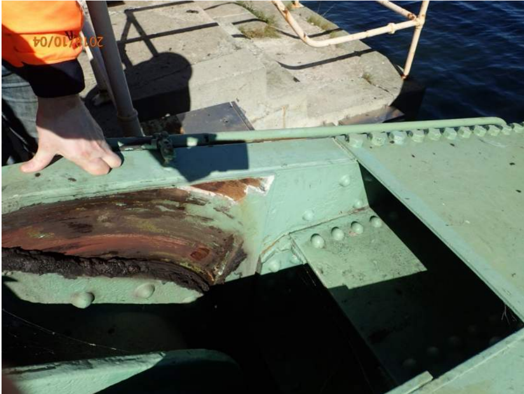
Photo S90: Areas of coating on the interior of the north plate of the north trunnion have been worn away.
