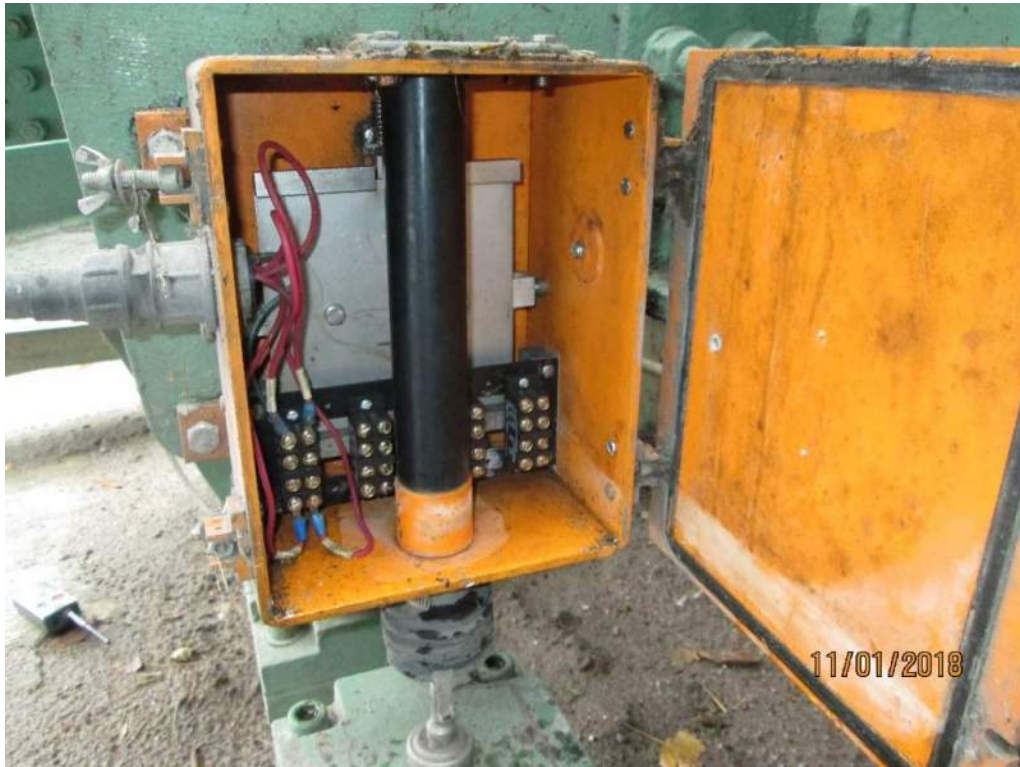
Photo E21: Span Fully Seated Limit Switch. Two span seated limit switches are provided at the toe end of the span, one at each corner. North seated limit switch exhibits standing water inside the enclosure.
