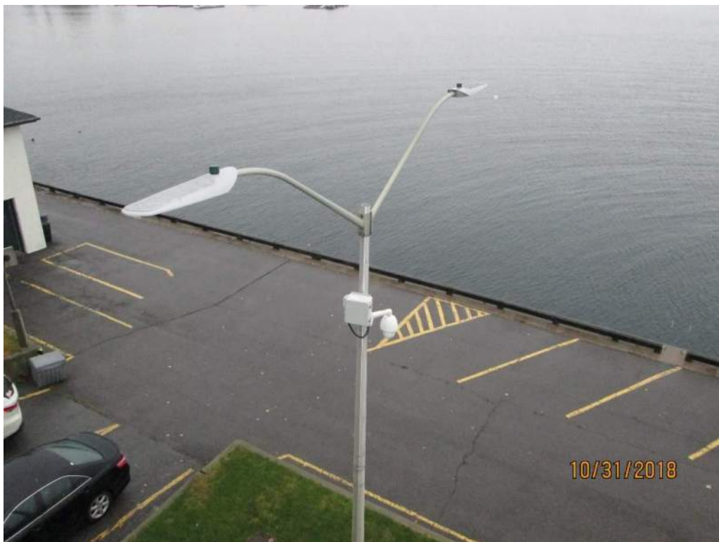
Photo E38: CCTV System and Roadway Lighting. A CCTV system was installed at the bridge for monitoring of the bridge roadway, waterway and machinery space from the maintenance facility and the operators control house. The CCTV installation is in excellent condition. LED type roadway lighting is provided on the bridge and is photocell controlled.
