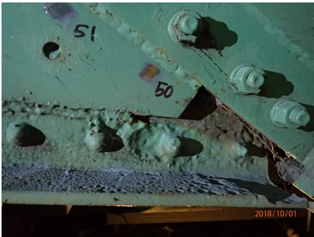
Photo S45: Very severe section loss in the rivet heads and angle at the base of the exterior face of the south plate of the north trunnion.
