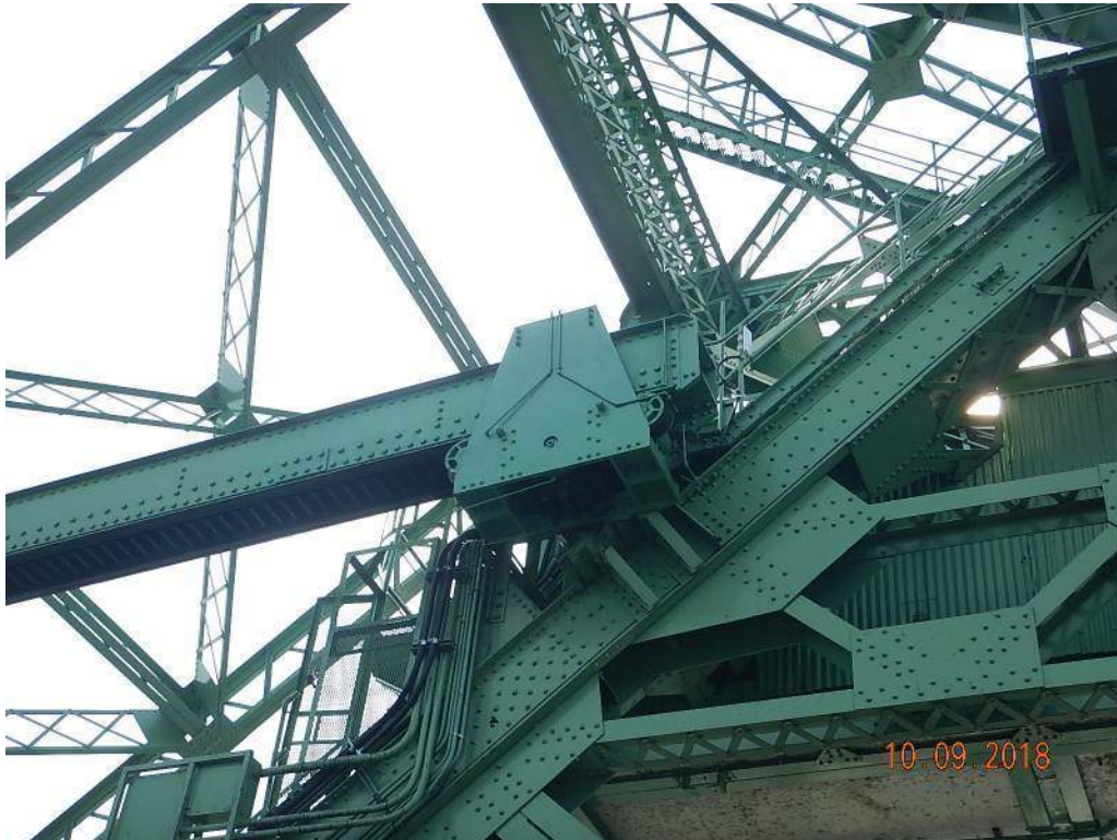
Photo M7: North Operating Strut Guide Assembly. There is no access to inspect many of the machinery interfaces internal to the guide assembly.
