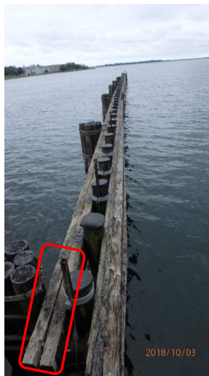
Photo S115: There is severe split in the top east fender at the north end of the east training wall.
