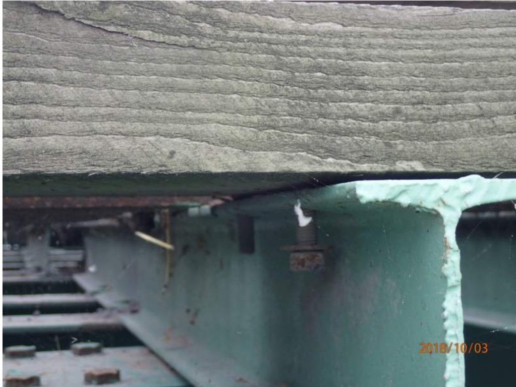
Photo S60: Several of the bolts connecting the north timber curb to the sills at the east end are loose.
