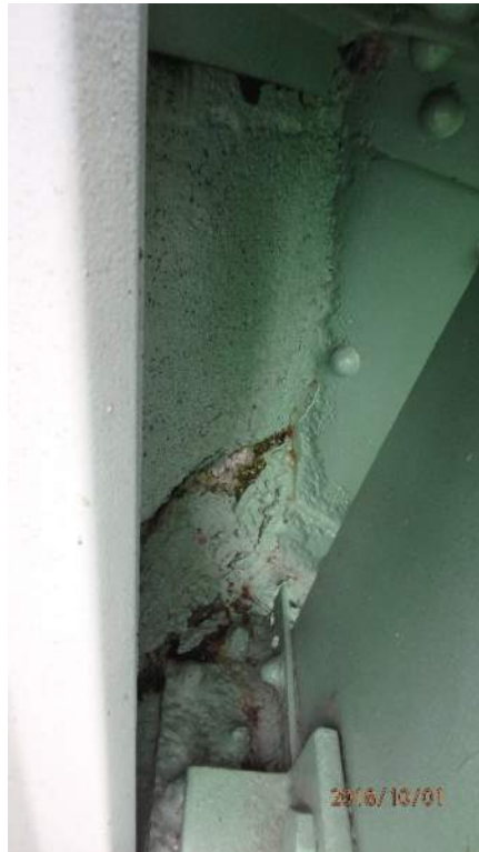
Photo S98: Counterweight truss member 21S-27N has severe localized section loss of the lower south angle at the west end at node 27N.
