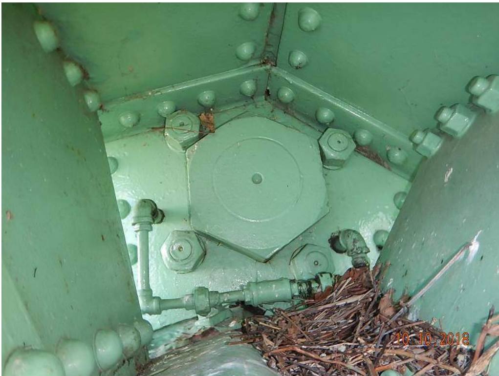
Photo M16: South Second Link Pin, Inboard Side. The lube ports at the inboard side of the second link pins are piped together to a common fitting. This is not good practice. Additionally, note the bird nest near the second link pin.
