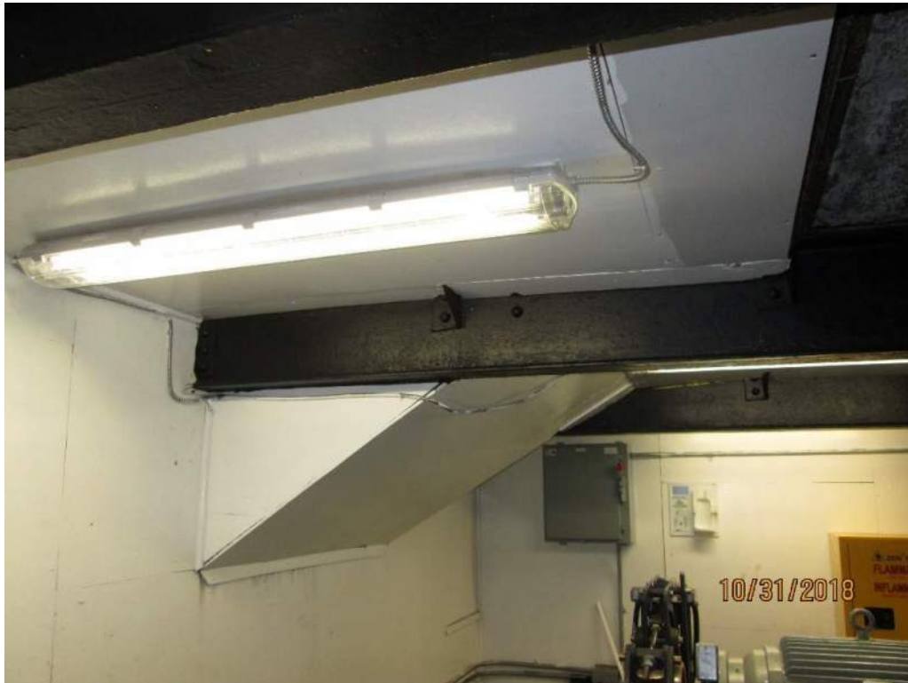
Photo E37: Machinery Space Lighting. The machinery space is provided with T5 light fixtures. These fixtures are in excellent operational condition and provide adequate lighting levels for maintenance and troubleshooting.
