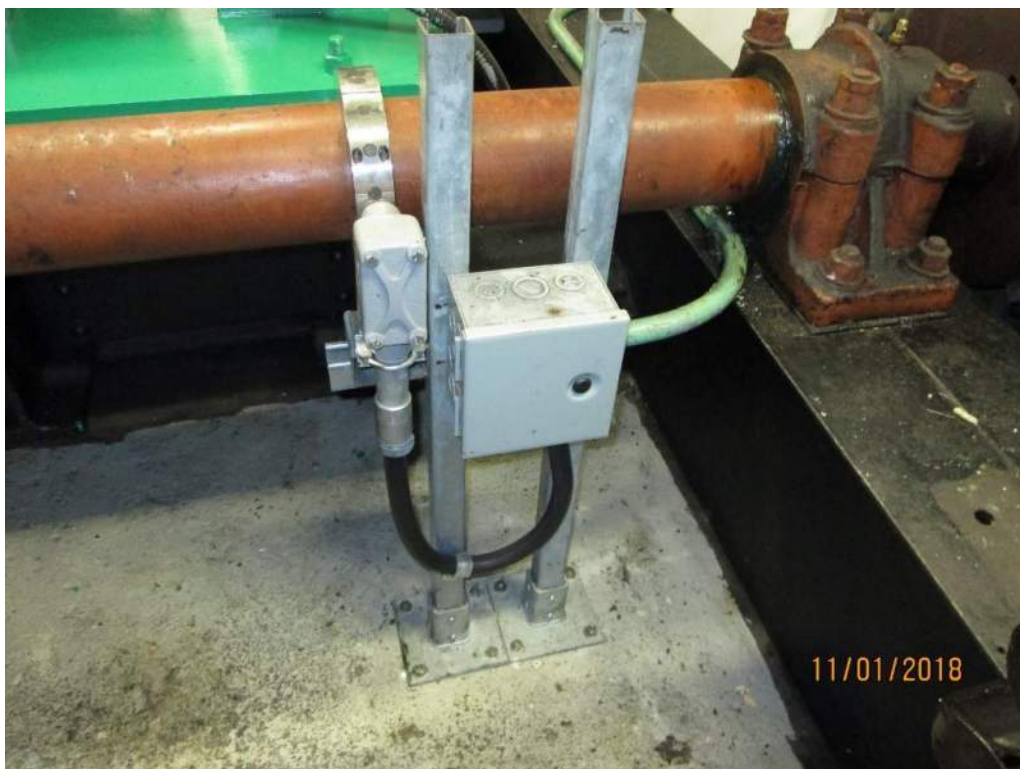
Photo E22: Speed Switch Sensor. A Hall Effect speed switch was installed as part of a 2012 rehabilitation project to provide span position and motor speed indication on the operator's control desk. The speed switch sensor is in excellent condition.
