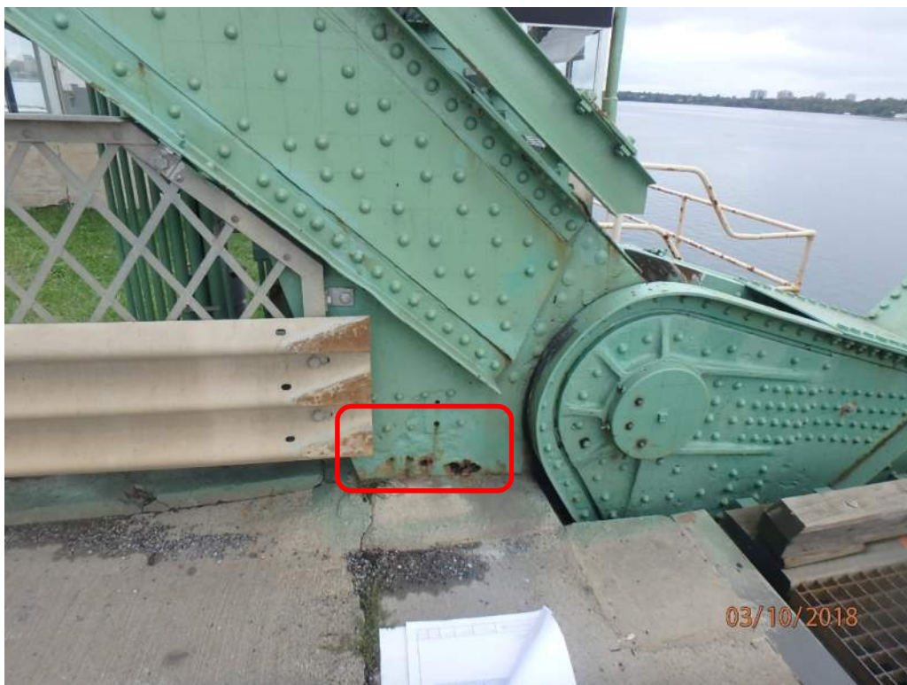
Photo S51: The vertical gusset plate at node 15N at roadway level exhibits very severe section loss and perforations.
