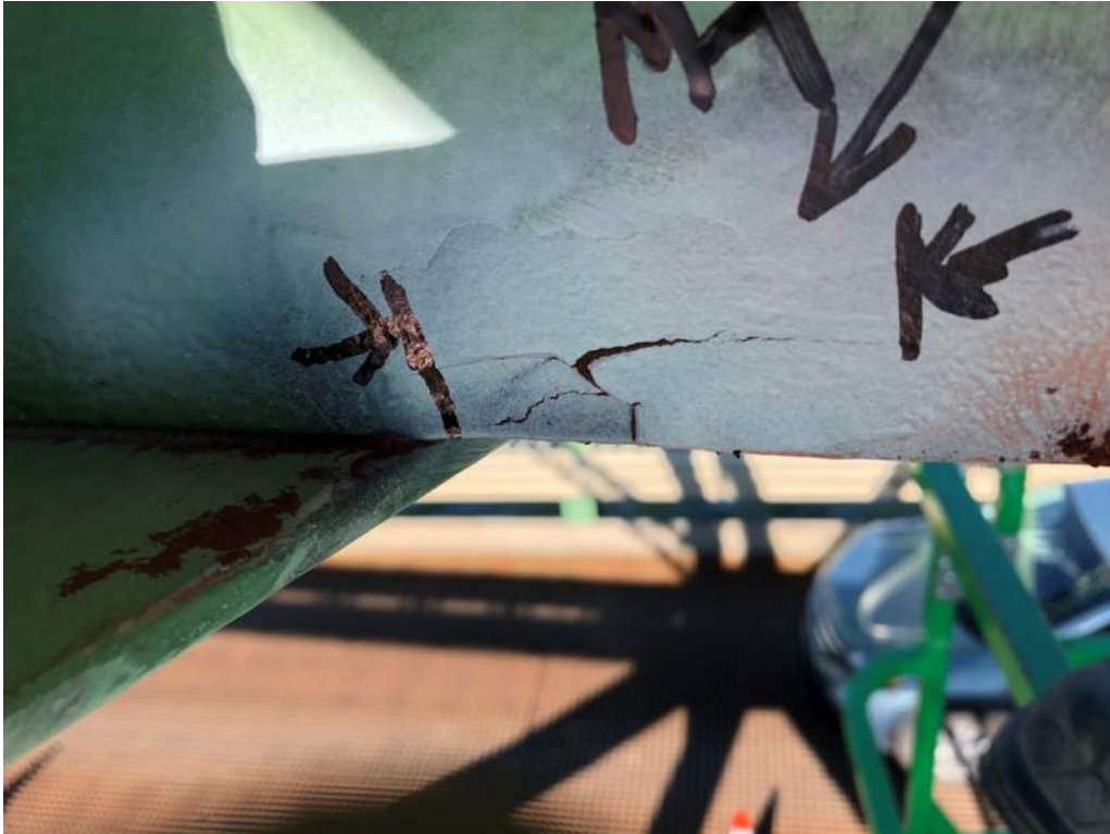
Photo S12: Leaf truss top chord member 3S-5S has a 60mm long lamination defect with a possible crack (photo by Brouco NDT).
