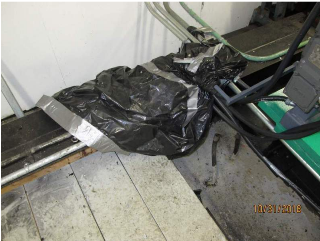
Photo E12: A black plastic bag is covering the junction box near motor brake #2. No water was observed at the time of the inspection, but traces of water stains indicate leaking of the roof is occurring.
