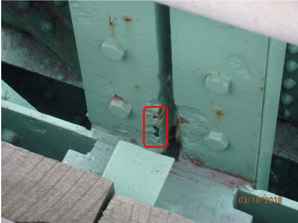
Photo S28: Perforation in the south angles of vertical member 11N-12N above node 12.
