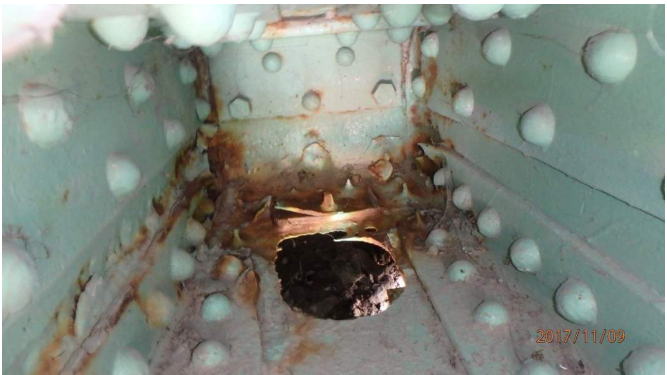
Photo S31: Severe corrosion and section loss of rivet heads at the base of 15N-17N and section loss of the gusset plate at the main trunnion (photo from 2017 inspection).
