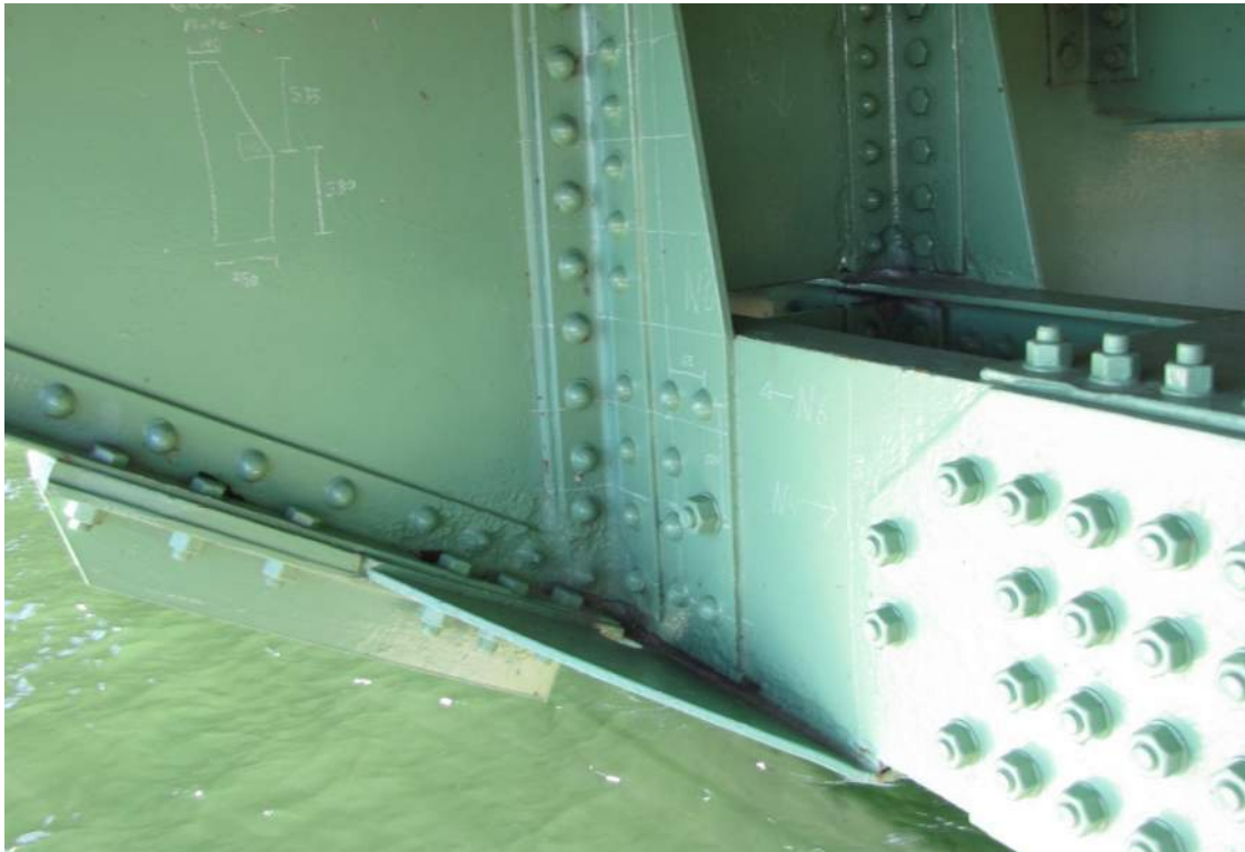
Photo S52: Severe localized section loss at the base of the gusset plate and sidewalk floor beam clip angle at 6S.
