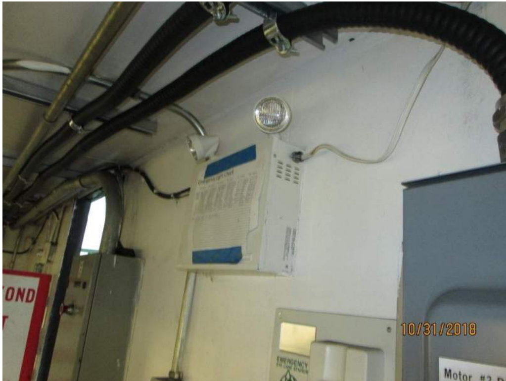
Photo E39: General Indoor Electrical Installation (Machinery Space Shown). Indoor electrical raceway installation in the machinery space and operators control house generally consists of rigid steel conduits. These conduits are in good condition. The bridge cable installation consists of wire in conduit and with Teck cables that were recently installed to feed the new drive motors.
