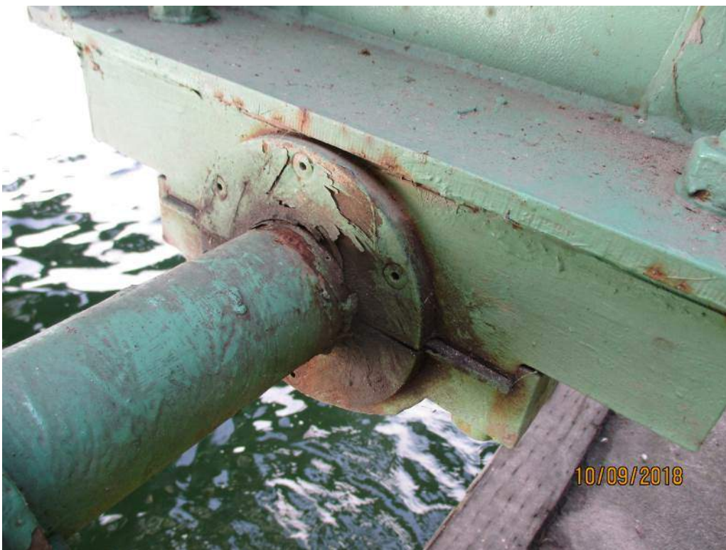
Photo M20: Span Lock Cross Shaft Bearing B1-S. The housing for the bearing exhibits paint deterioration and light corrosion. All of the span lock cross shaft bearings are similar.
