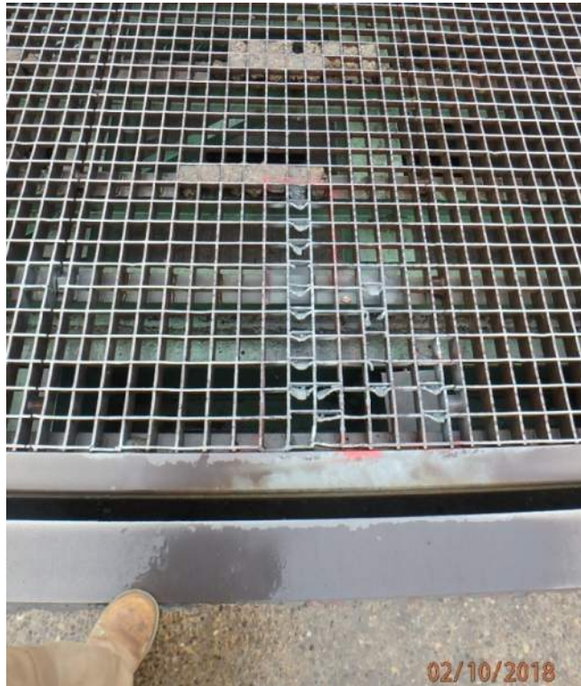
Photo S84: Repairs have recently been carried out to areas of the steel deck grating with broken and bent bars (east end shown).
