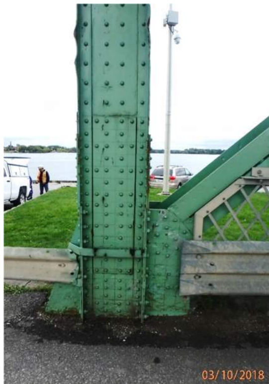
Photo S35: Tower truss vertical member 19N-20N has severe section loss in the rivet heads and web plate at roadway level and deformation (likely due to impact damage) in the southeast and southwest flanges.
