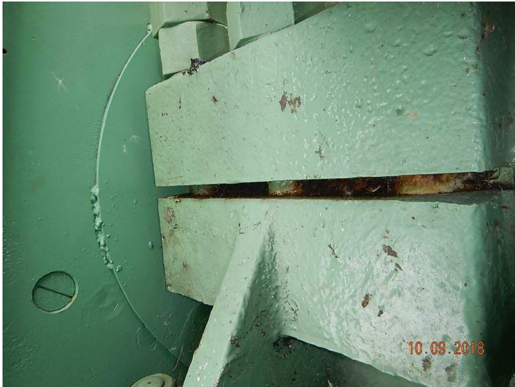
Photo M1: Span Drive Machinery B1-N Bearing. There is light paint deterioration and corrosion between the bearing cap and base at the upper split line. B1-S Bearing is similar.
