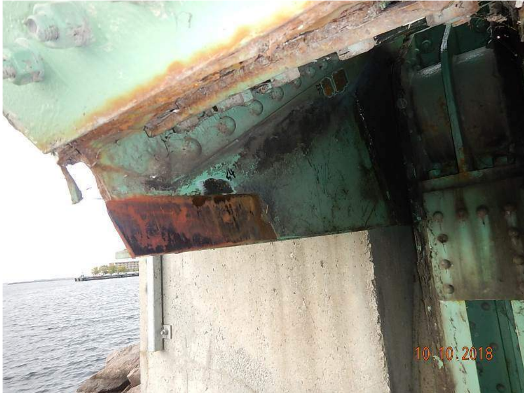
Photo M11: Truss Near South Main Trunnion Bearing. Note the evidence of contact between the span structure and the bearing support.
