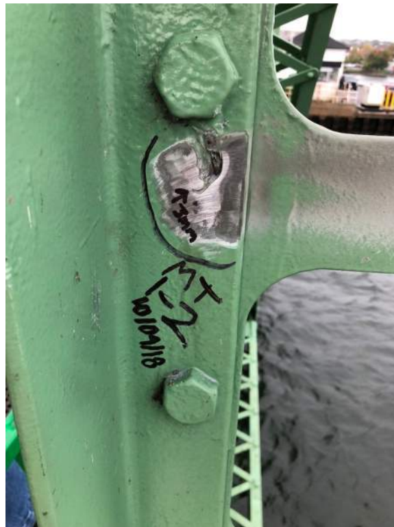
Photo S23: Suspected crack at flame-cut hole in southeast angle of vertical member 1N-2N (photo by Brouco NDT).
