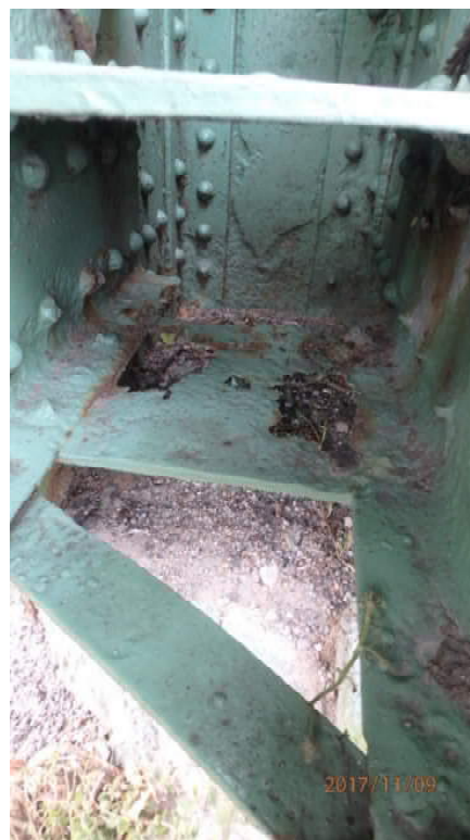
Photo S33: Truss tower horizontal member 18N-19N has severe section loss of interior angles and rivet heads plus a perforated lower batten plate (photo from 2017 inspection).
