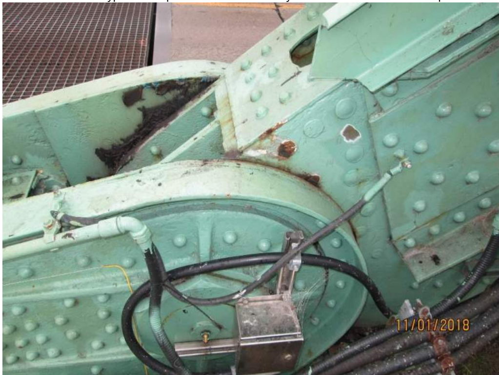
Photo E34: Bridge Grounding & Bonding System. The bridge steel structures are provided with proper grounding and bonding system in accordance with code.
