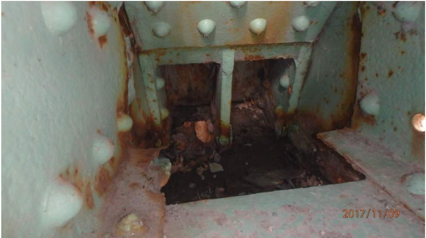
Photo S32: View of the west side of the north trunnion. Note the loss of the bottom flange of the north channel of tower truss member 15N-18N (photo from 2017 inspection).
