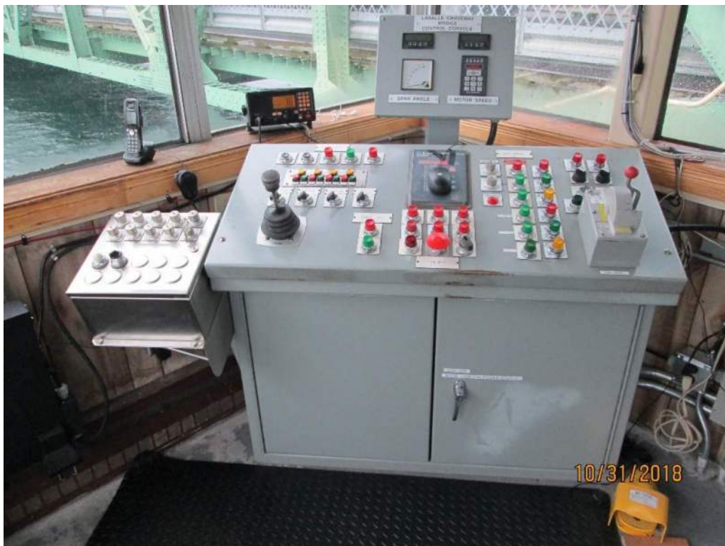
Photo E18: Control Desk. The location of the control desk provides the operator with a complete view of the channel and vehicular and pedestrian roadway traffic. The control desk is in acceptable condition. Note the foot switch next to the control desk on the floor is in good operational condition.
