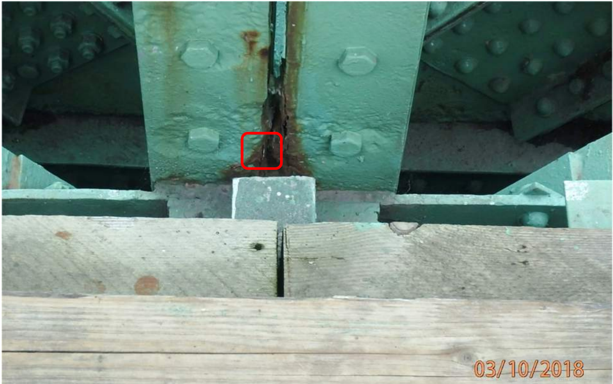
Photo S26: Very severe pitting with a small perforation in the south angles of vertical member 9N-10N above node 10.
