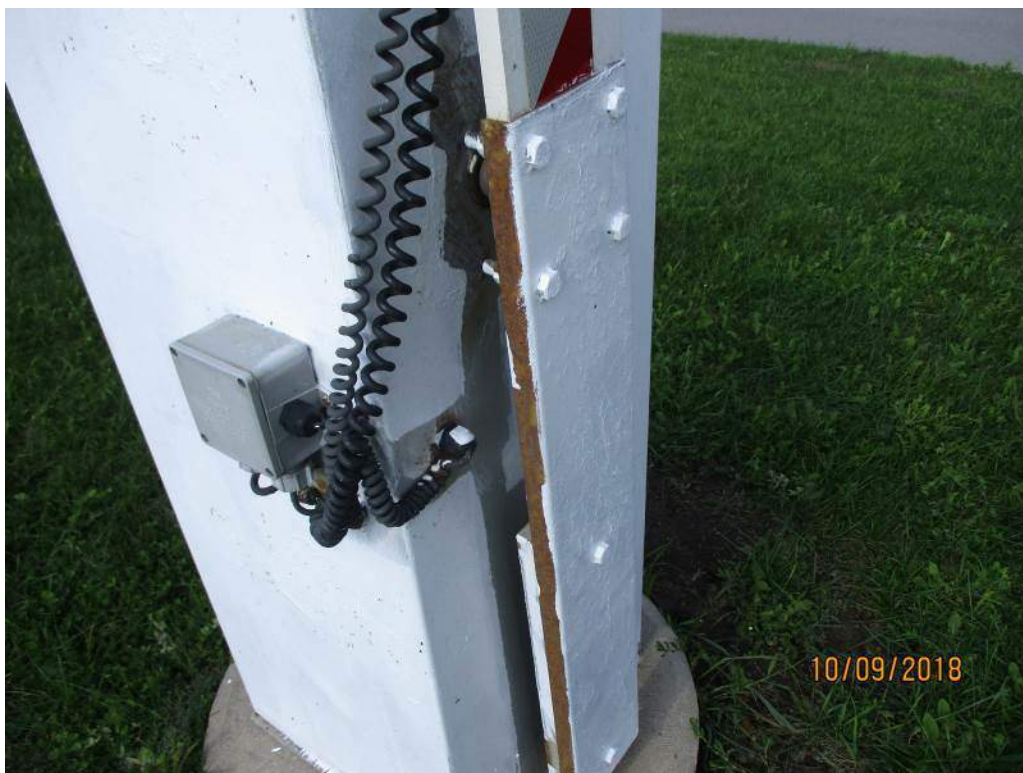
Photo M28: Northeast Warning Gate. The warning gate arms are not fully painted, and corrosion is still evident under the paint. The southeast warning gate is similar.
