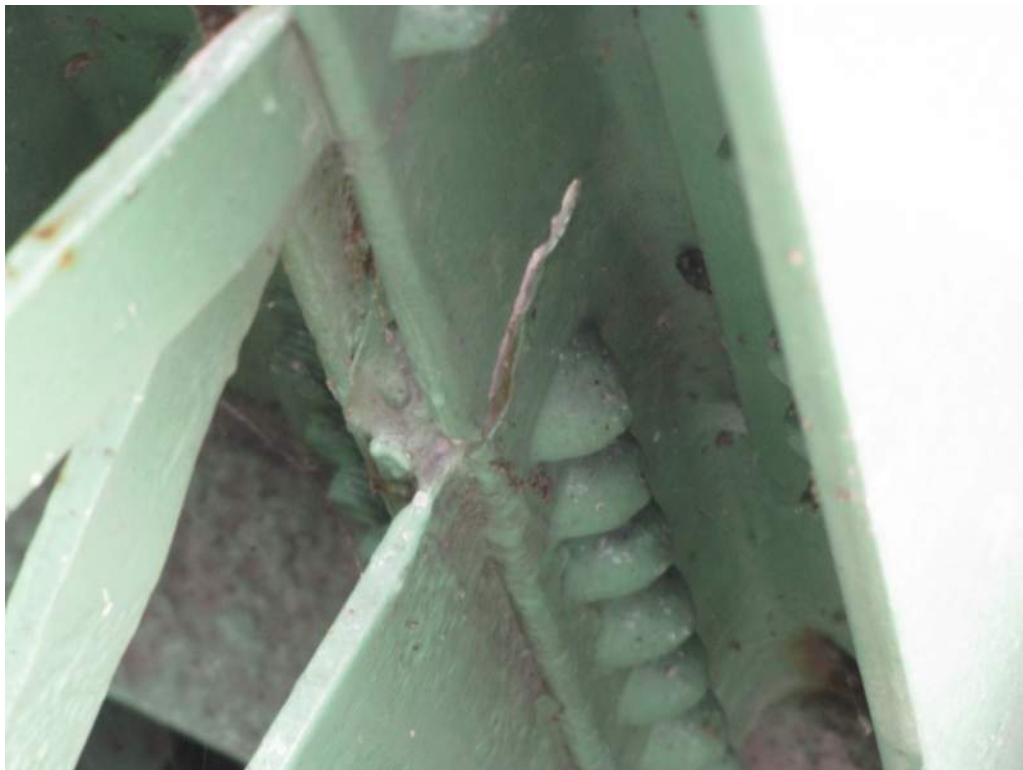
Photo S29: Both south flanges of vertical member 11N-12N near 12N are perforated but the member has been strengthened.
