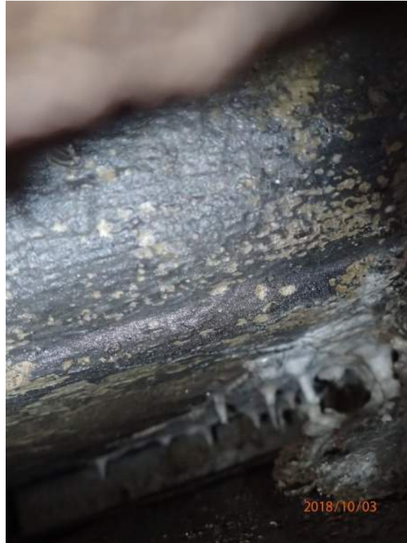
Photo S66: Efflorescence deposits and staining on the underside of the counterweight concrete.
