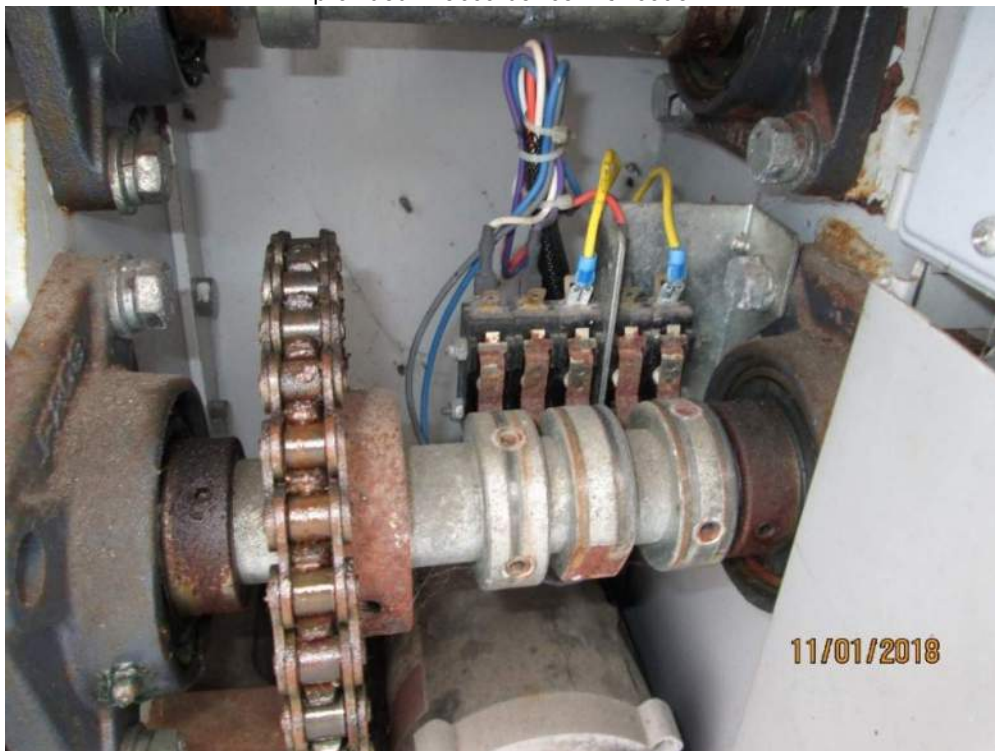
Photo E28: Typical Traffic Gate Limit Switches. The traffic gates are provided with a cam type limit switch. Although these limit switches were in operational condition at the time of the inspection, they are missing protective covers, switch contacts exhibit excessive corrosions due to the exposure which might cause premature failure.
