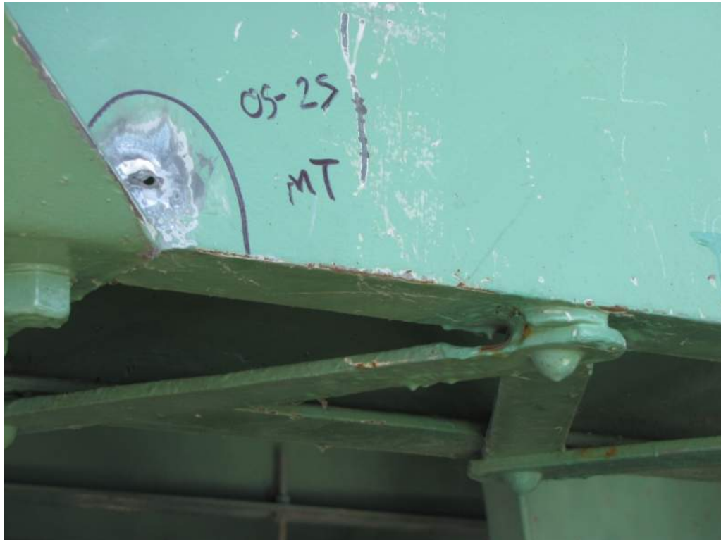
Photo S16: Severe localized section loss and perforation in web of south channel of leaf truss bottom chord member 05-2S at node 2S adjacent to the sidewalk floor beam connection.
