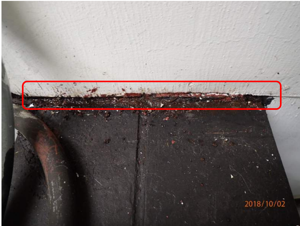
Photo S102: Water was leaking into the northwest corner of the mechanical room during the inspection. Over time this has caused corrosion of the top flange of one of the steel beams supporting the motors.
