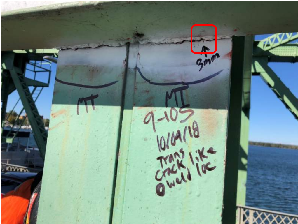
Photo S30: 3mm long crack in top of southeast leg of vertical member 9S-10S at weld location (photo by Brouco NDT).
