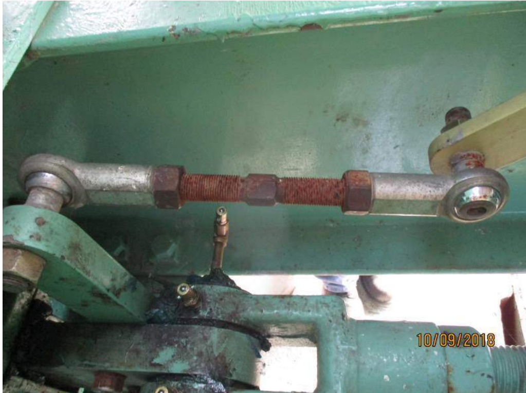
Photo M21: South Span Lock Crank Shaft CR1. The position indication shaft threads are not painted and corroded. The north location is similar.
