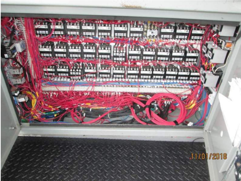
Photo E19: Relay Control Inside the Control Desk. This relay cabinet was modified during the drive/motor replacement project to accommodate the new control required for the new drive system.
