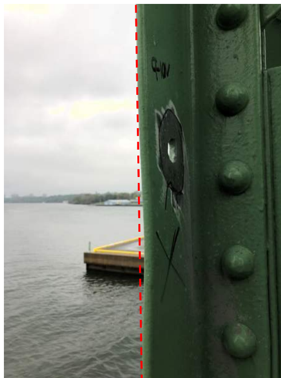
Photo S25: Deformation of the northwest leg of vertical member 9N-10N was noted below the flame-cut hole (photo by Brouco NDT).
