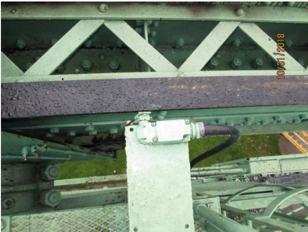
Photo E24: Span Over-Travel Limit Switch. The span control is provided with an over-travel limit switch to stop bridge operation in the event of span over travel.
