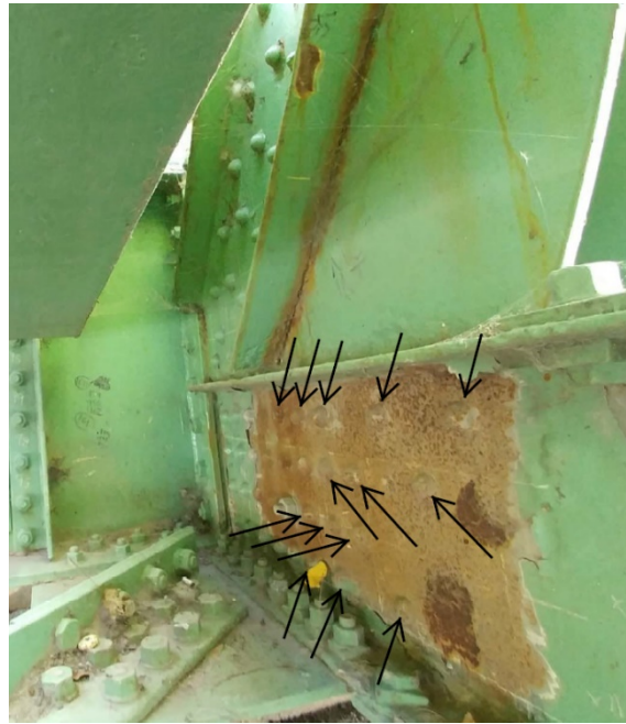
Figure 23 – Significant corrosion on the bottom chord connection of the south side of the north interior plate
