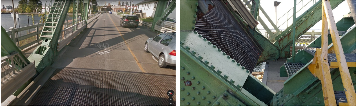
Figure 25 - Interior plate of the south trunnion located in the splash zone (a) Left: Bridge opened to traffic (b) Right: Bridge during operation
