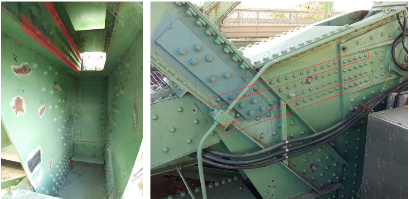
Figure 18 – Gusset Plate Strengthening Type A1 (a) Left: View from inside the trunnion (b) Right: View from outside.
