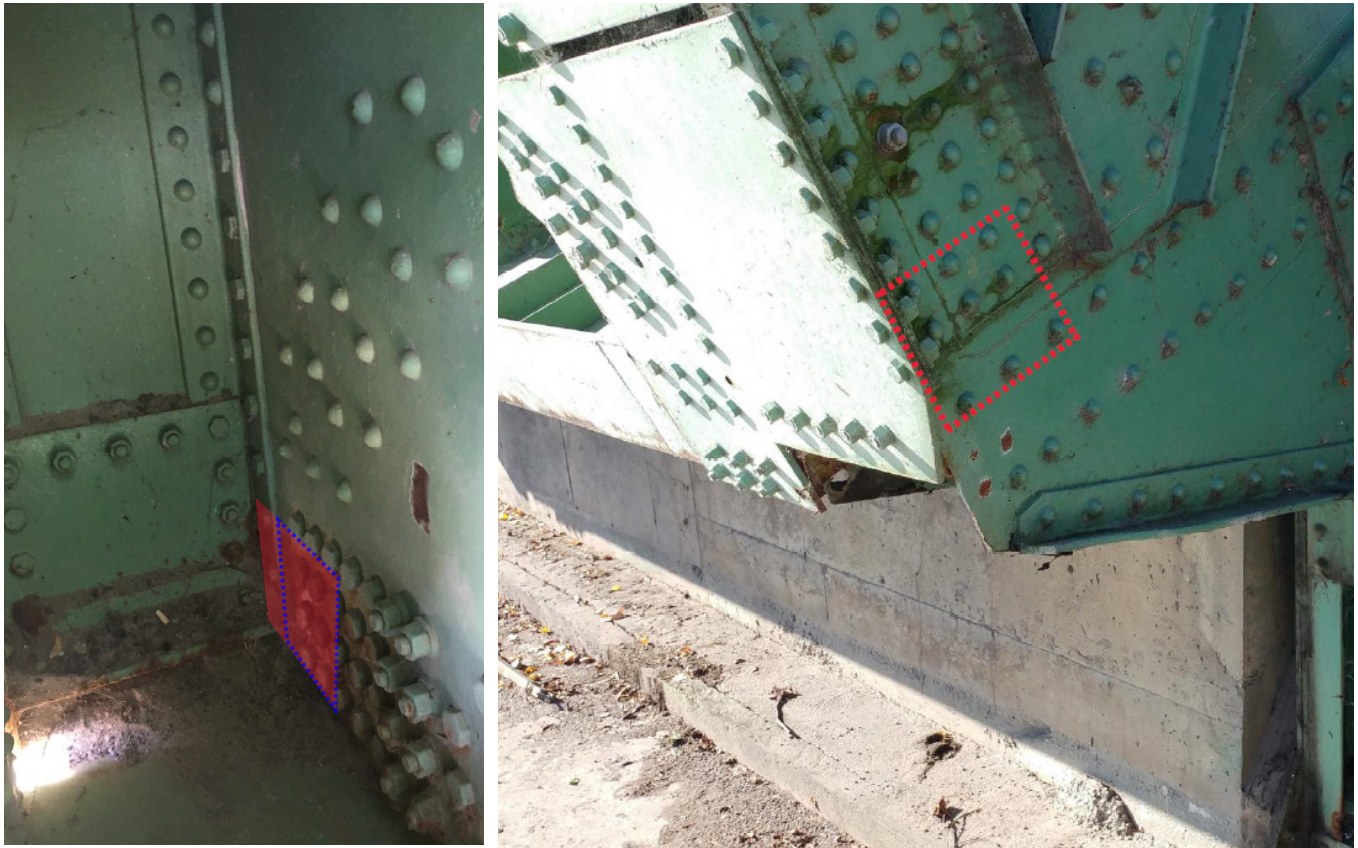
Figure 21 - Gusset Plate Strengthening Type C (a) Left: View from inside the trunnion (b) Right: View from outside
