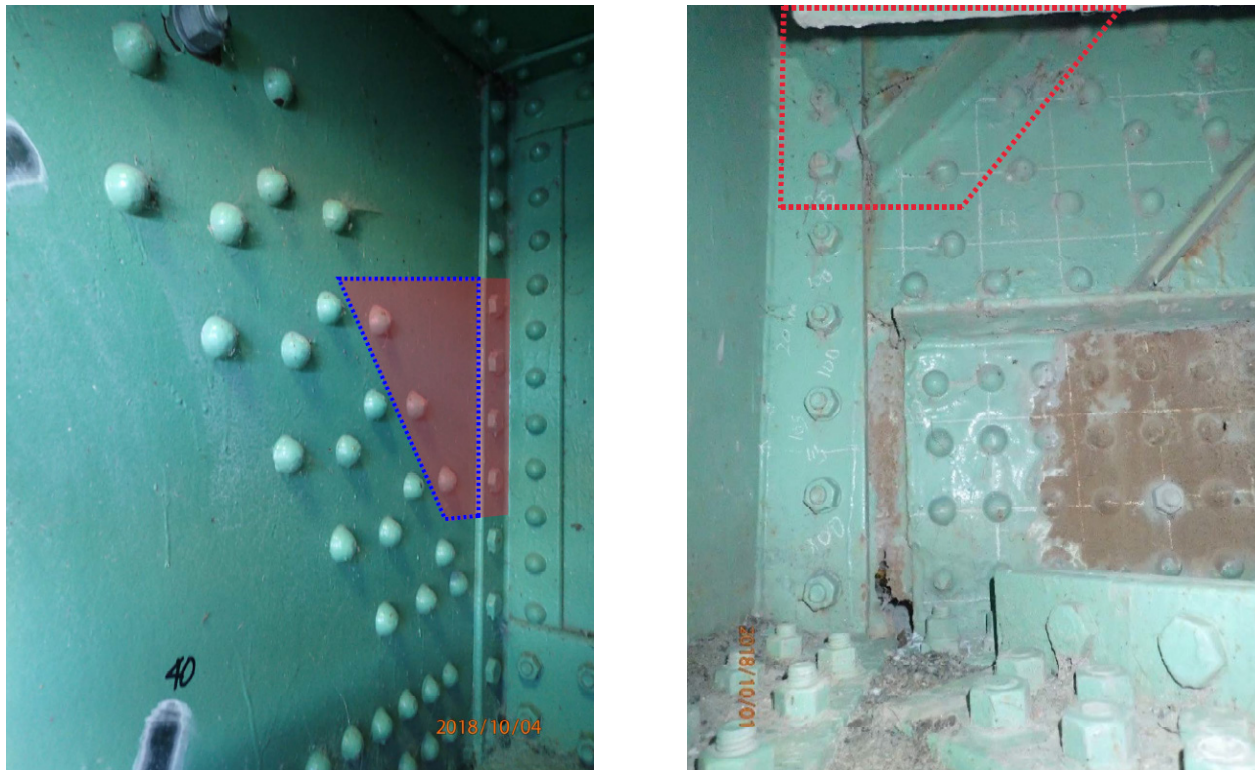
Figure 22 - Gusset Plate Strengthening Type D (a) Left: View from inside the trunnion (b) Right: View from outside
