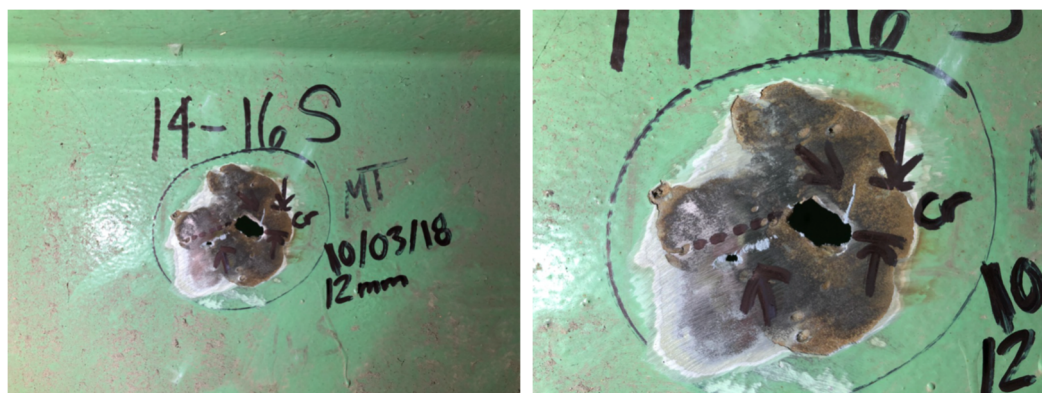
Figure 8: 12mm Crack in 14S-16S Interior Channel's Web, Perpendicular to Main Stress and Near Perforation/Crack Like Indication, Parallel to Main Stress
