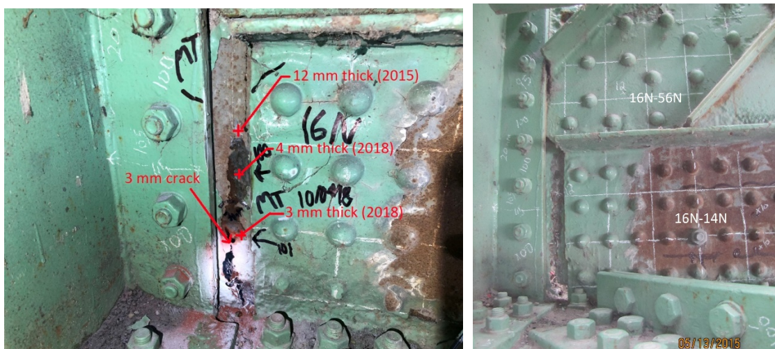
Figure 6: Linear Perforation in 16N Interior Plate, with Possible Crack
