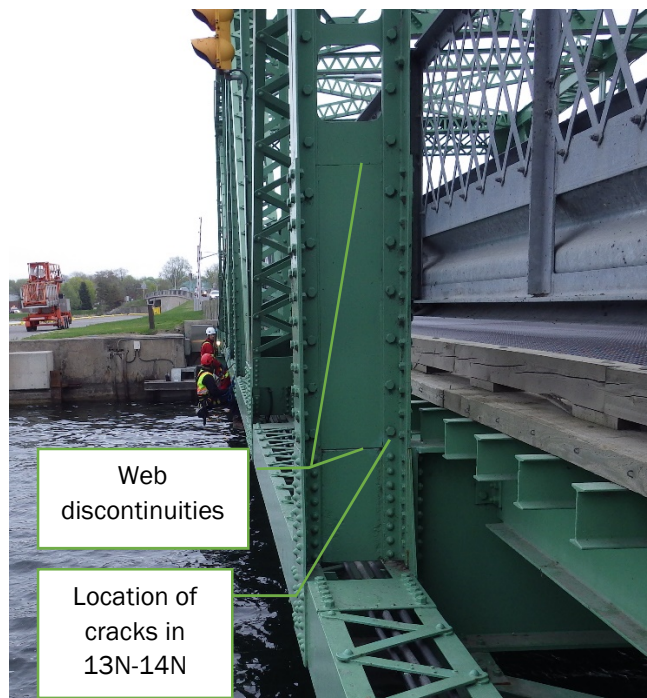
Figure 22: Discontinuity in Verticals Webs
