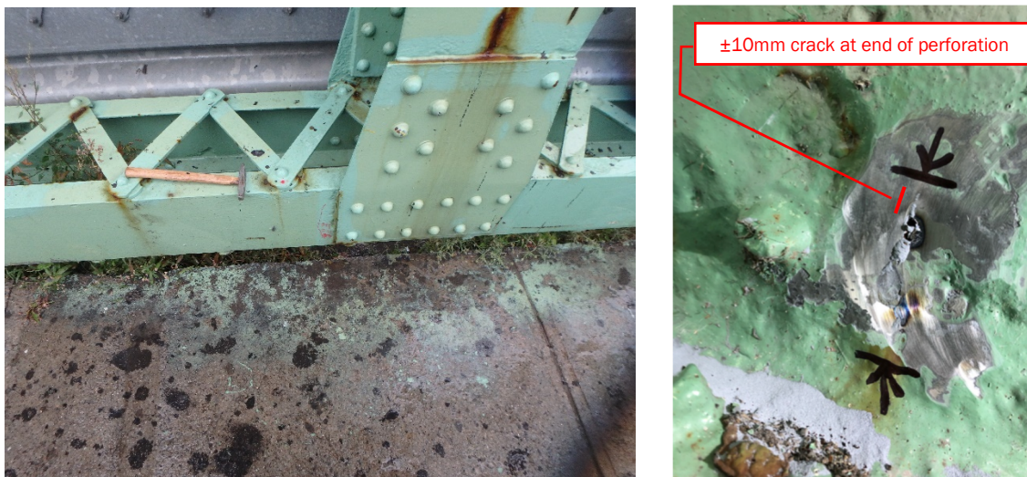
Figure 21: Linear Perforation in 18S-19S Exterior Channel, with Possible Crack
