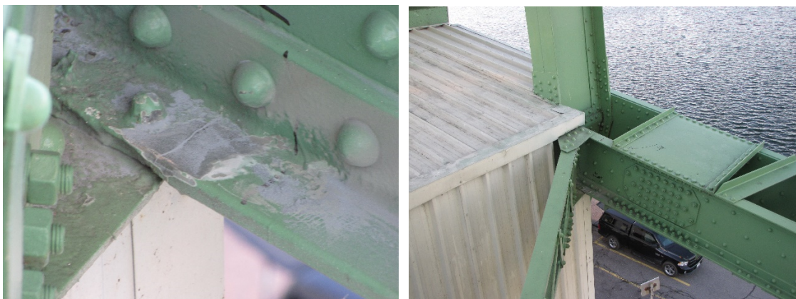
Figure 16 and Figure 17: Crack in 21N-27N Horizontal Flange of Bottom Interior Angle
