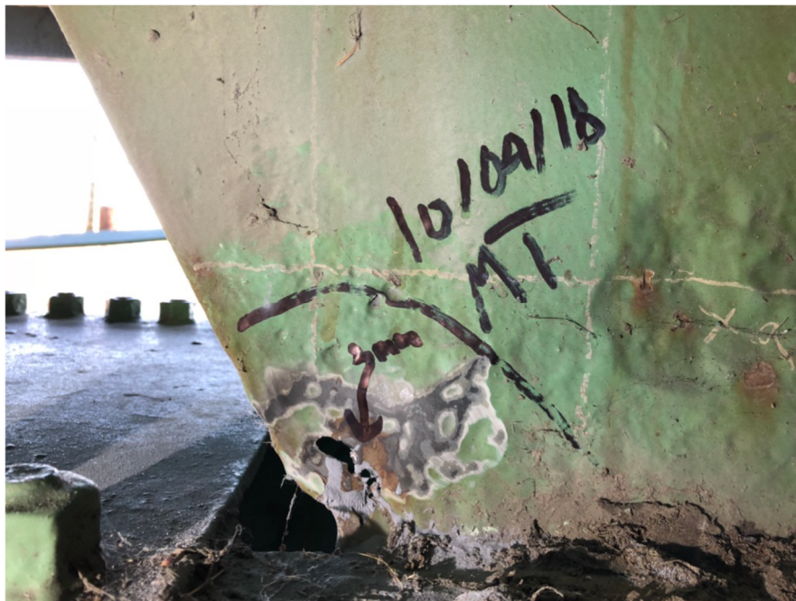
Figure 9: 3mm Crack in 16S Interior Plate, Perpendicular to Main Stress
