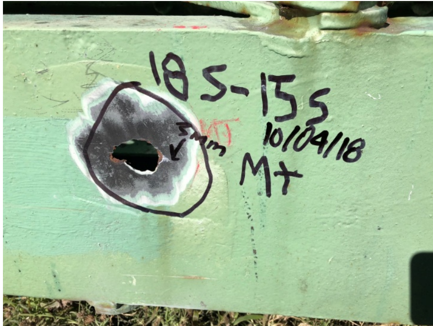
Figure 20: Perforation in 15S-18S Exterior Channel, with Possible 3mm Crack
