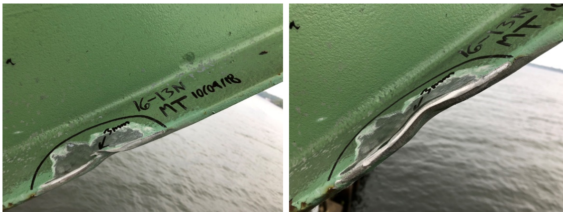
Figure 18 and Figure 19: 3mm Crack at Impact Damage (left), Removed by Light Grinding (right)
