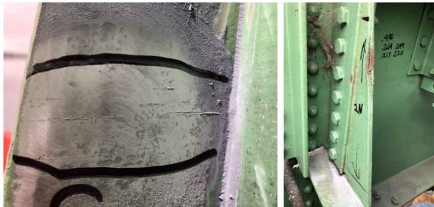
Figure 12 and Figure 13: Laminations and Hairline Crack, Perpendicular to Main Stress, in Interior Gusset Plate at 2N
