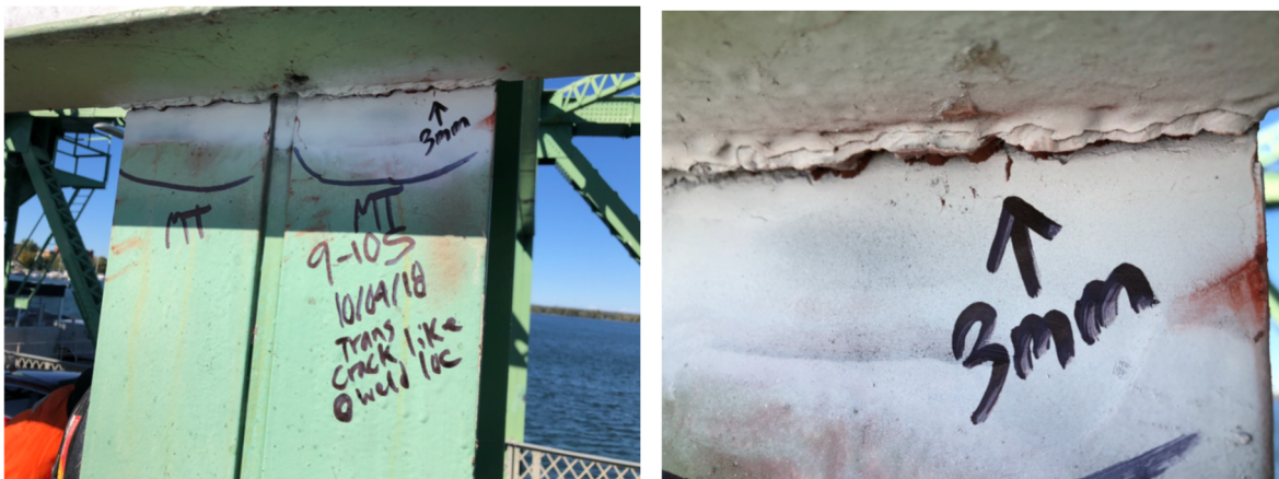
Figure 14 and Figure 15: 3mm Crack in HAZ Of Removed Weld on 9S-10S
