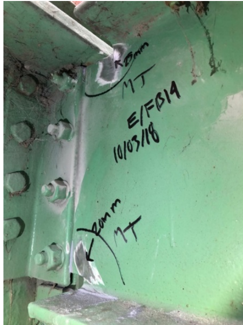
Figure 5: Typical Stringer Coped Ends Cracking – Stringer E, Floorbeam 14, Bay 14-16
