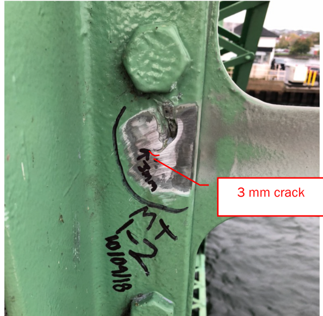
Figure 11: 3mm Crack Suspected, Perpendicular to Main Stress
