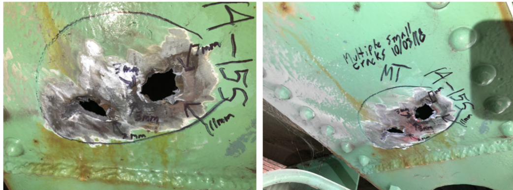
Figure 7: Cracks Originating from Perforation in Batten Plate of 14S-15S
