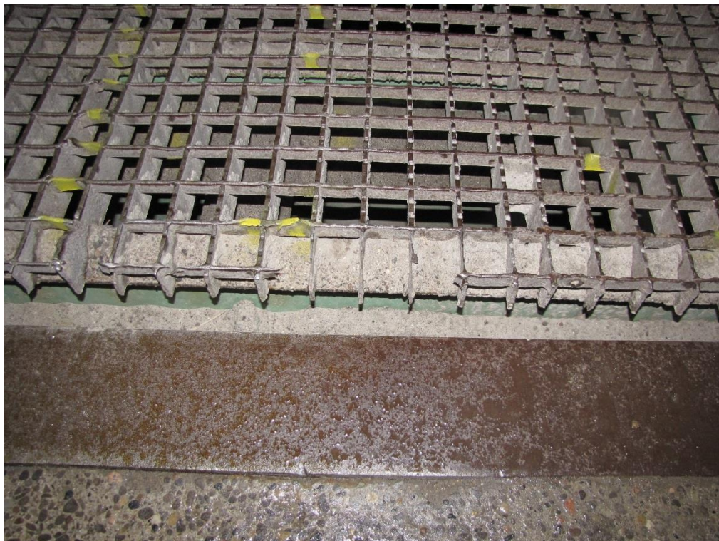
Photo 12: Condition of grating at east abutment prior to temporary repair.
