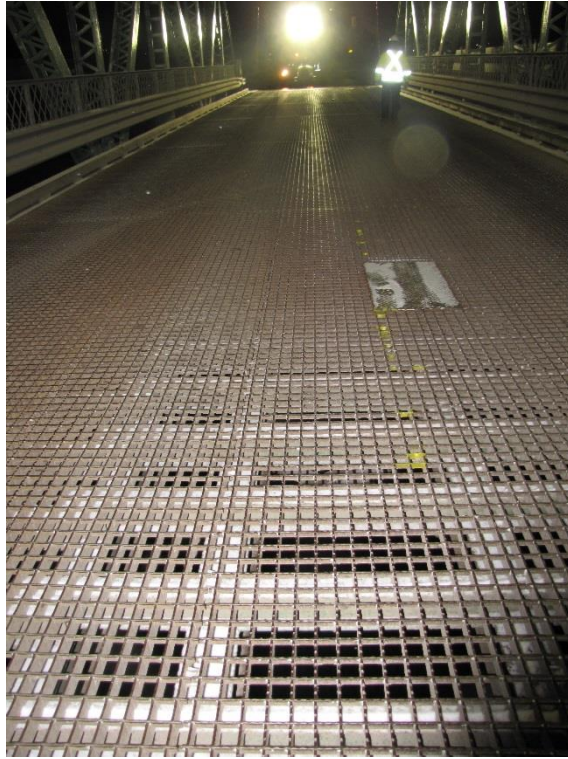
Photo 23: Bent Transverse Bars at location of grating hole
