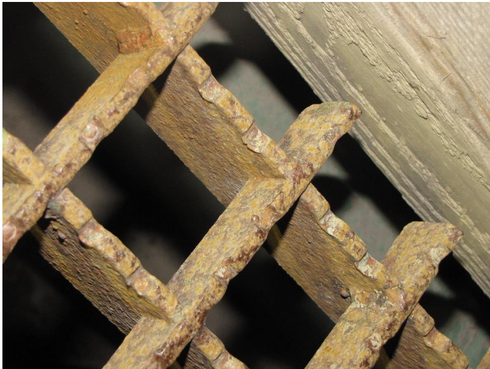
Photo 3: Light to medium corrosion of cross bars and bearing bars at the north curb by the west abutment.
