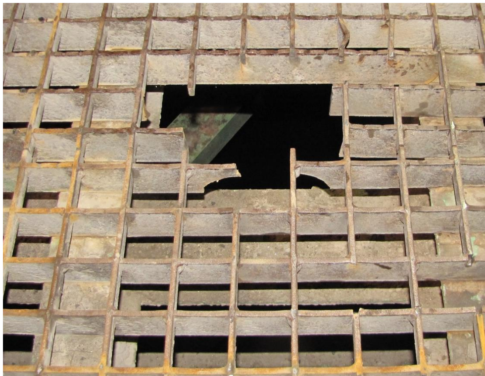
Photo 20: Crack in bearing bar propagating from cross bar notch.
