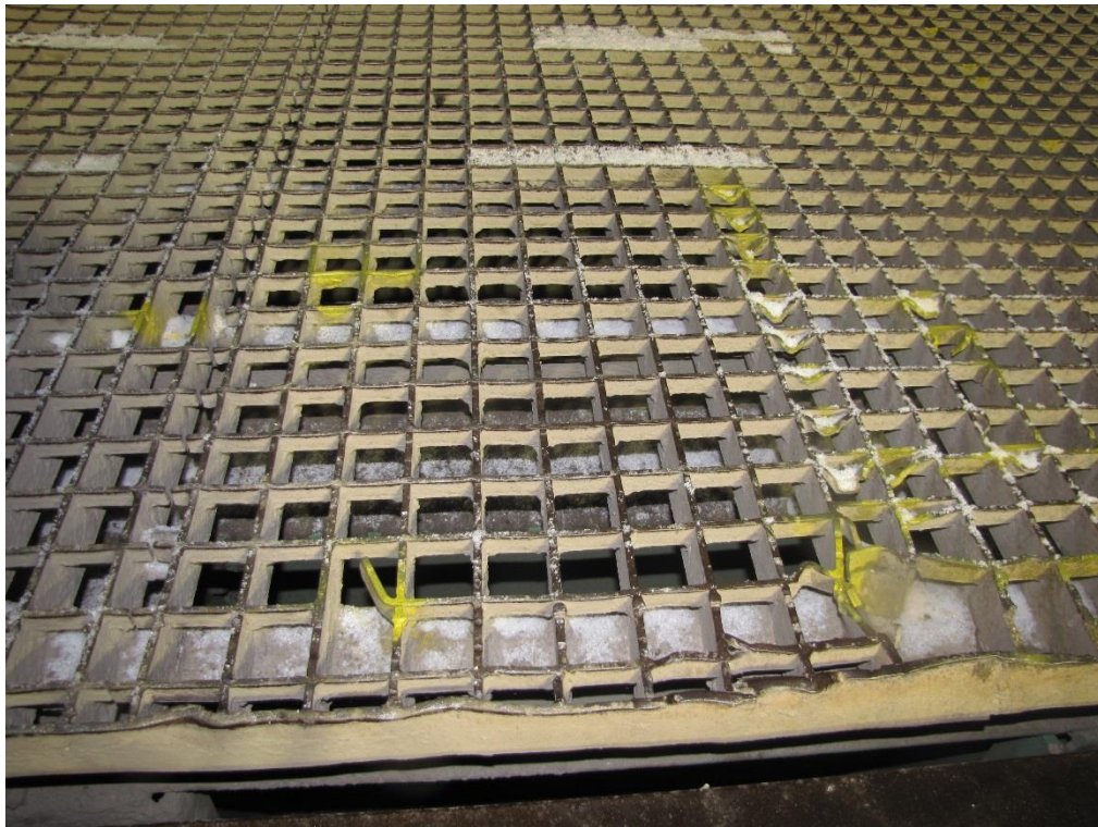
Photo 11: Broken and bent cross-bars and bearing bars at east abutment
