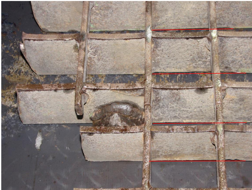
Photo 21: Wearing of base of bearing bars at sill location.
