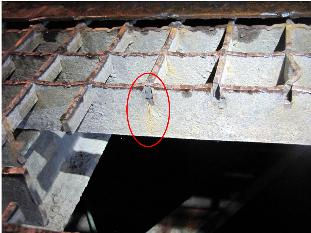
Photo 18: Crack in Bearing bar propagating from cross bar notch.
