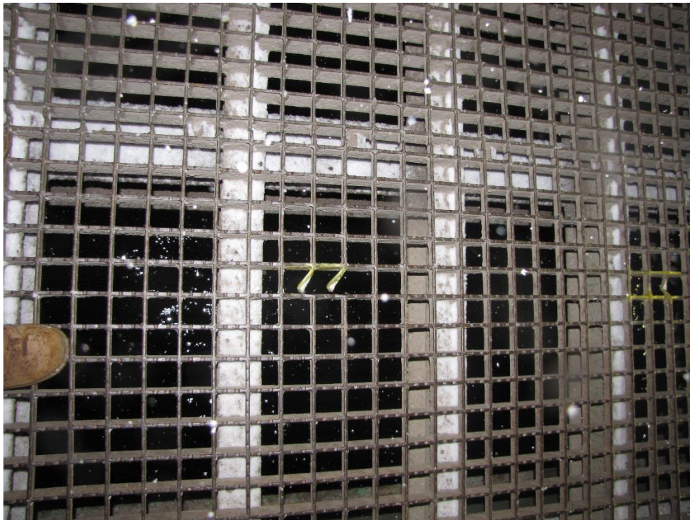
Photo 7: Broken Bars at (D14-15 at row 4)
