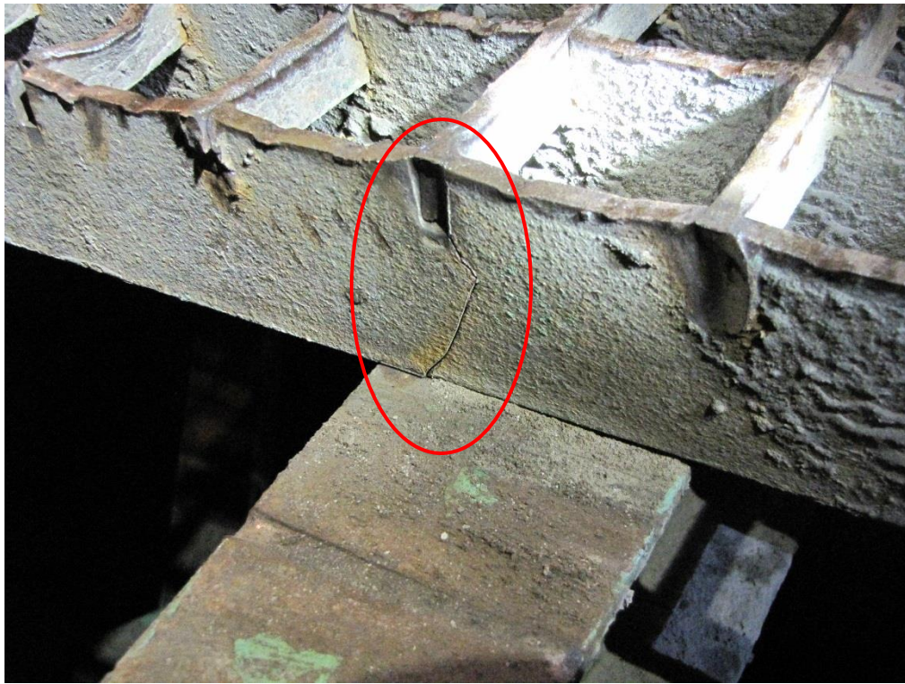
Photo 17: Crack in bearing bar propagating from notch for cross bar at sill. Adjacent to piece that was broken off.
