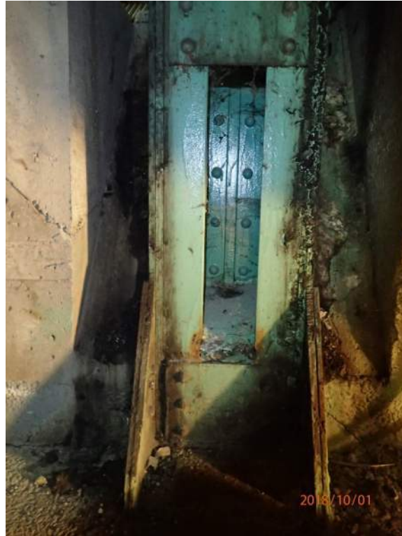
Photo 13: The visible / accessible sections of the post below 15N are in relatively good condition.
