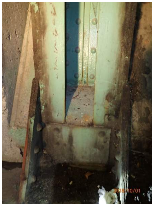
Photo 14: The visible / accessible sections of the post below 15S are in relatively good condition.
