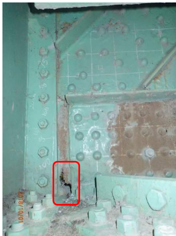
Photo 20: The interior (south) vertical gusset plate at node 16N exhibits severe section loss and a perforation with a crack (viewed from south).
