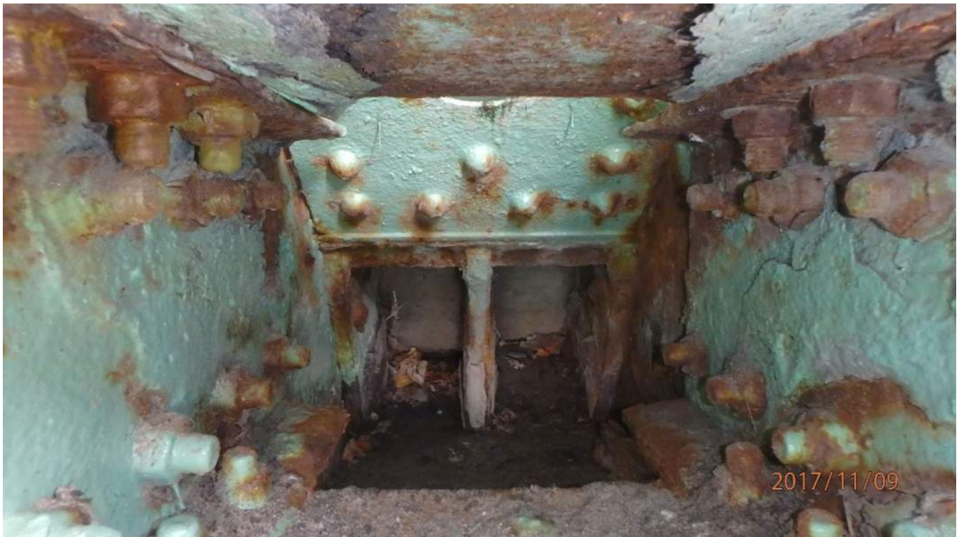
Photo 34: View of the west side of the south trunnion. Note the severe corrosion of member 15S-18S (photo from 2017 inspection).
