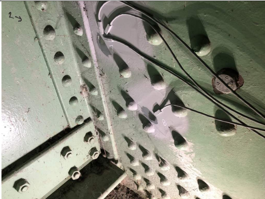
Figure2: Test Locations 7 and 8 at North Trunnion Plate Exterior Plate at Strain Gauge Locations (Readings Taken from Inside surface of Plate)
