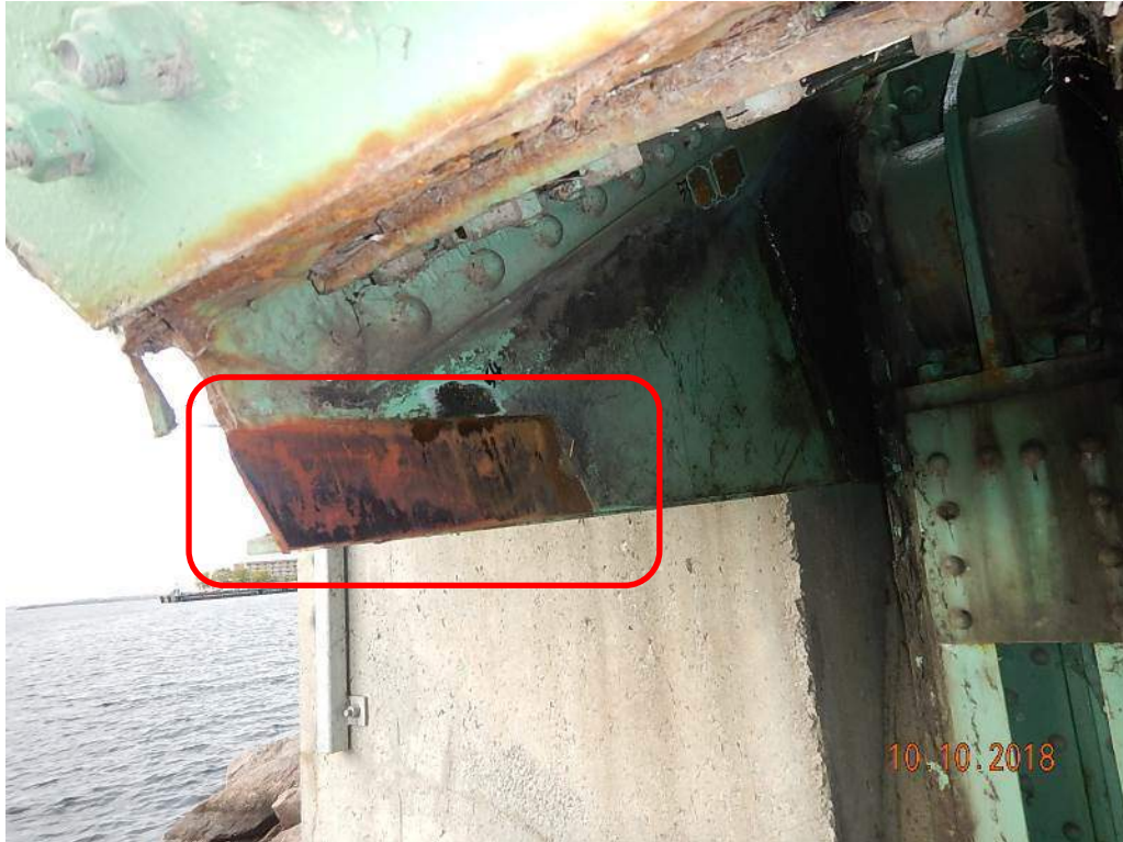
Photo 35: South trunnion. Note the evidence of contact between the span structure and the bearing support (photo by Stafford Bandlow).
