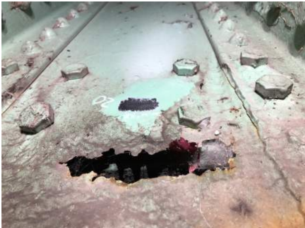
Photo 6: Perforation in batten plate of north trunnion (photo by Brouco NDT).
