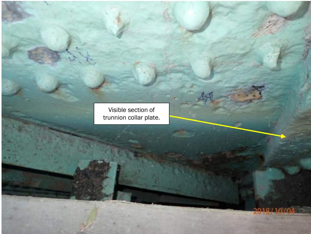
Photo 31: The north (roadway) side of the south trunnion has widespread pitting in the collar plate, connecting plate, and some rivet heads.
