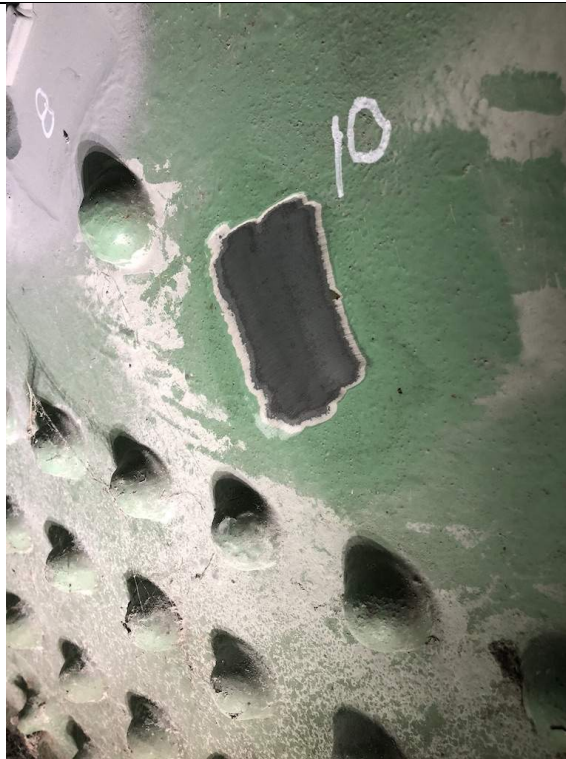
Figure4: Test Location 10 at North Trunnion Plate Exterior Plate (Readings Taken from Inside surface of Plate)
