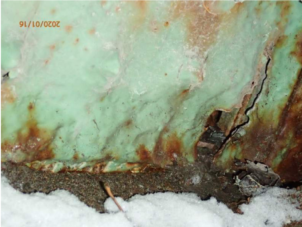
Photo 21: The interior (south) vertical gusset plate at node 16N exhibits severe section loss and a perforation with a crack (viewed from north, 2020 photo).
