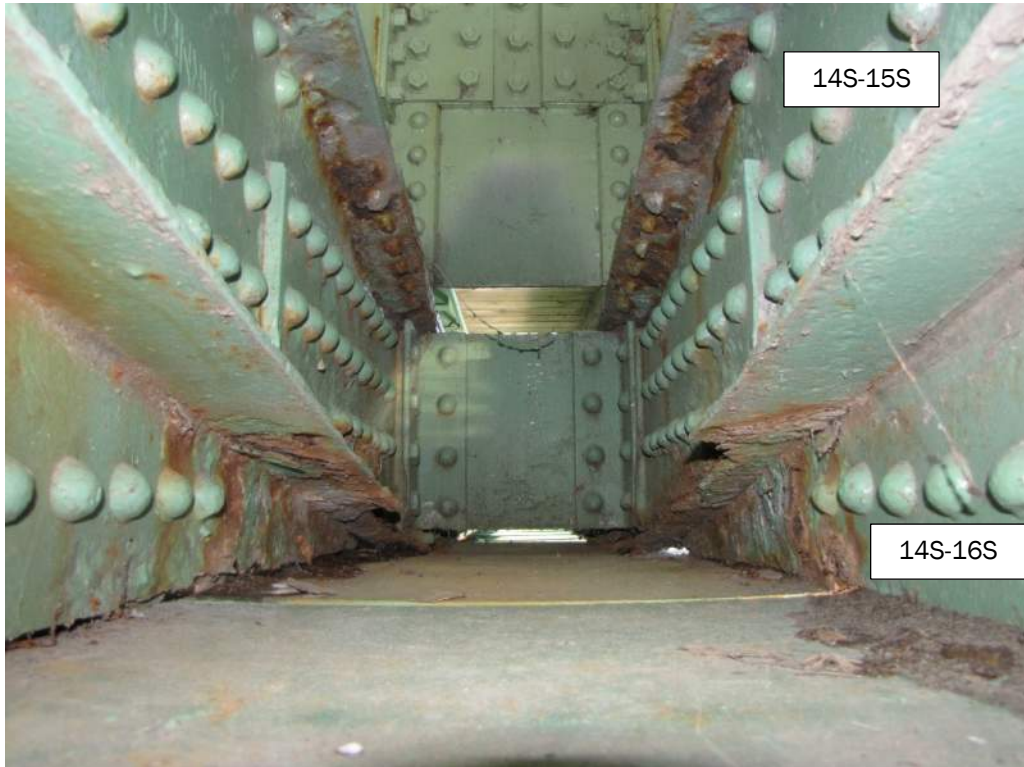
Photo 7: Severe localized pitting and section loss of flanges where 14S-16S and 14S-15S intersect. Several rivet heads have over 75% section loss.
