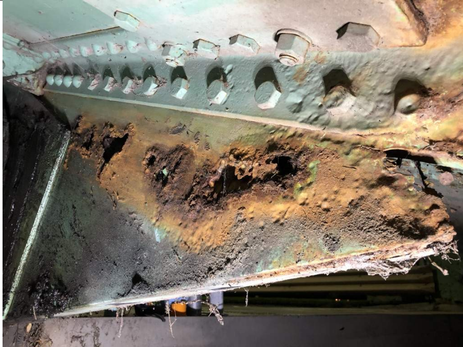
Figure7: Opposite Side of South Trunnion Plate Interior Location (Inside Plate Surface, see Figure 6 for Exterior Plate Surface)
