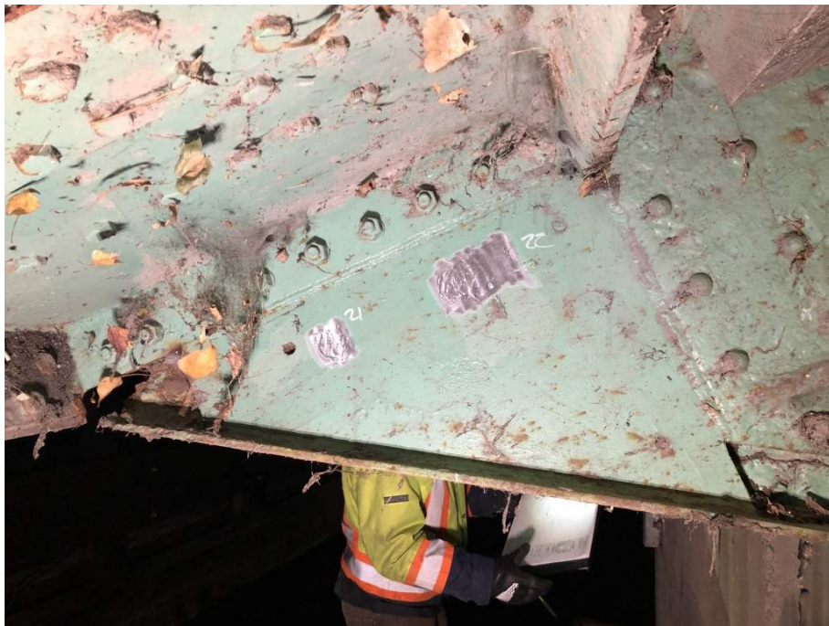
Figure6: Test Locations 21 and 22 at South Trunnion Plate Interior Location (Readings Taken on Exterior Plate Surface)
