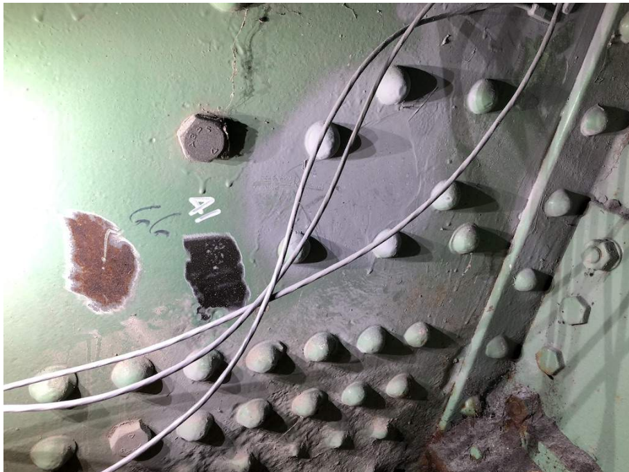
Figure16: Test Location 41 at South Trunnion Exterior Plate Location (Readings Taken on Interior Surface of Plate)
