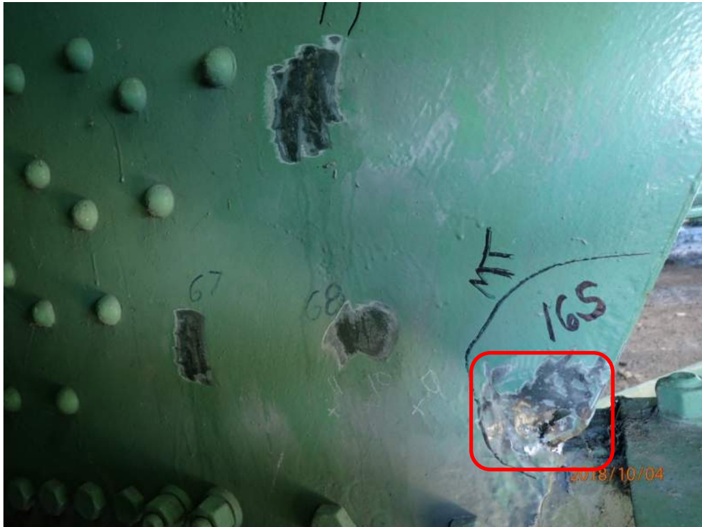
Photo 25: View of the interior of the north plate of the south trunnion below deck level. A crack was found at the perforation circled.
