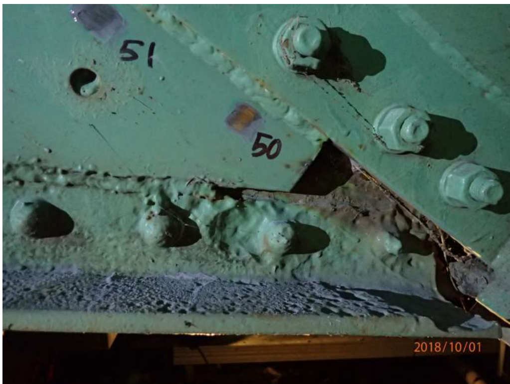
Photo 24: Very severe section loss in the rivet heads and angle at the base of the exterior face of the south plate of the north trunnion.
