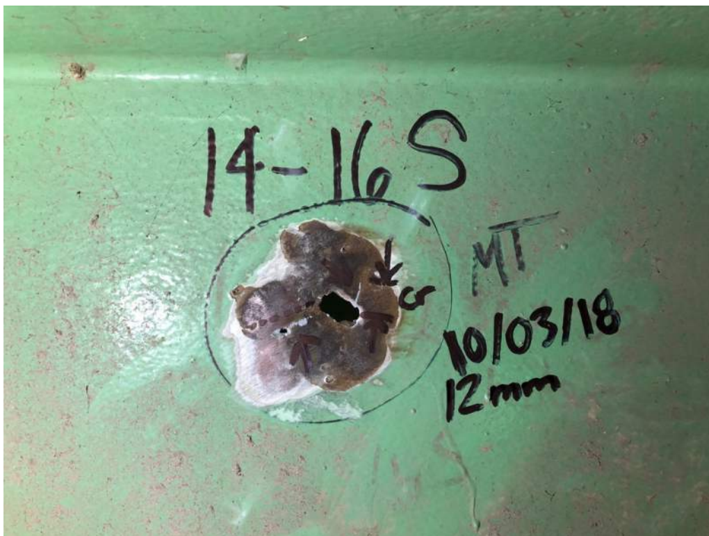
Photo 10: Perforation and 12mm long crack in interior channel of bottom chord member 14S-16S (photo by Brouco NDT).
