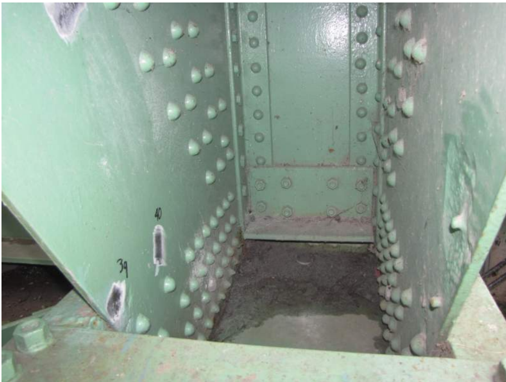
Photo 22: The interior faces of the plates and rivet heads at the base of the north trunnion have localized severe section loss.
