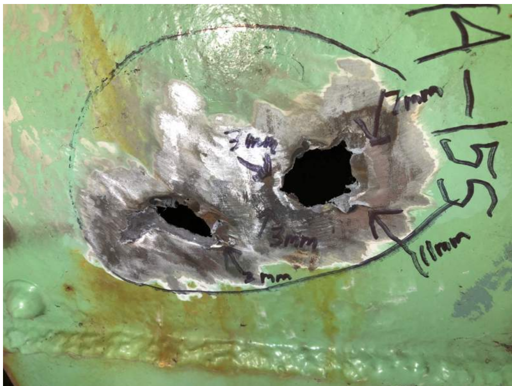
Photo 8: Perforations and cracks in bottom batten plate of bottom chord member 14S-15S near node 15S. The cracks range in length from 3mm to 11mm (photo by Brouco NDT).
