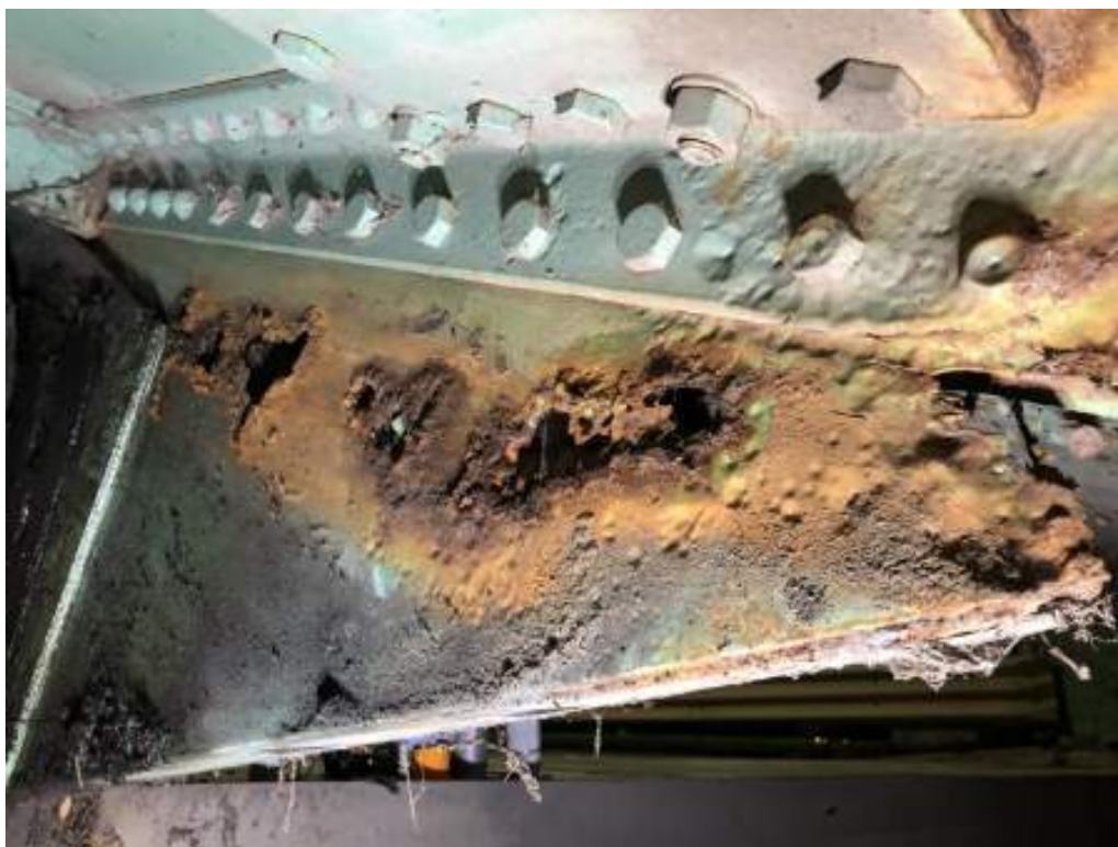
Photo 32: Inside face of north plate of south trunnion (photo by Brouco NDT, 2019).
