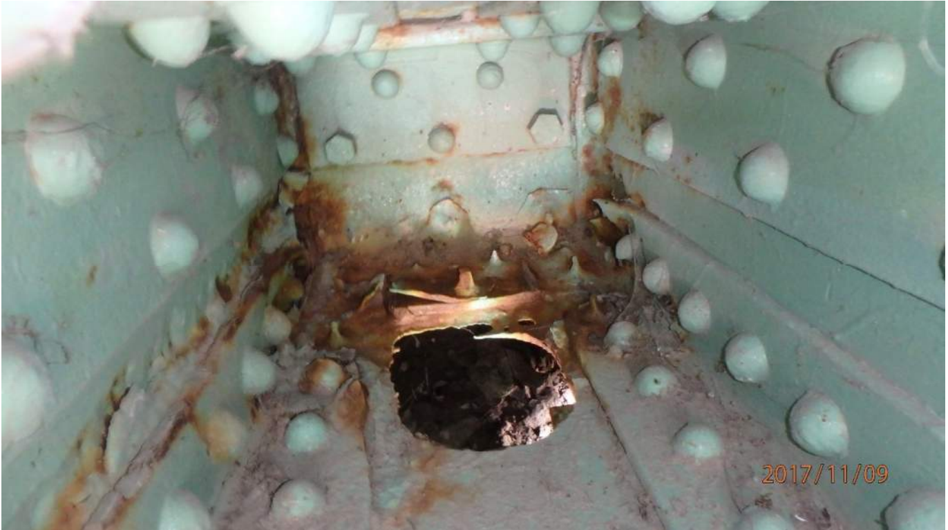
Photo 11: Severe corrosion and section loss of rivet heads at the base of 15N-17N and section loss of the gusset plate at the main trunnion (photo from 2017 inspection).
