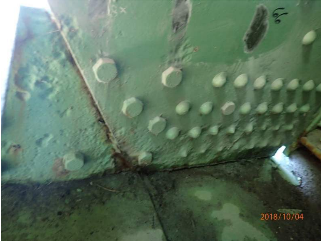
Photo 29: Severe pitting at the base of the interior face and rivet heads of the south plate of the south trunnion.
