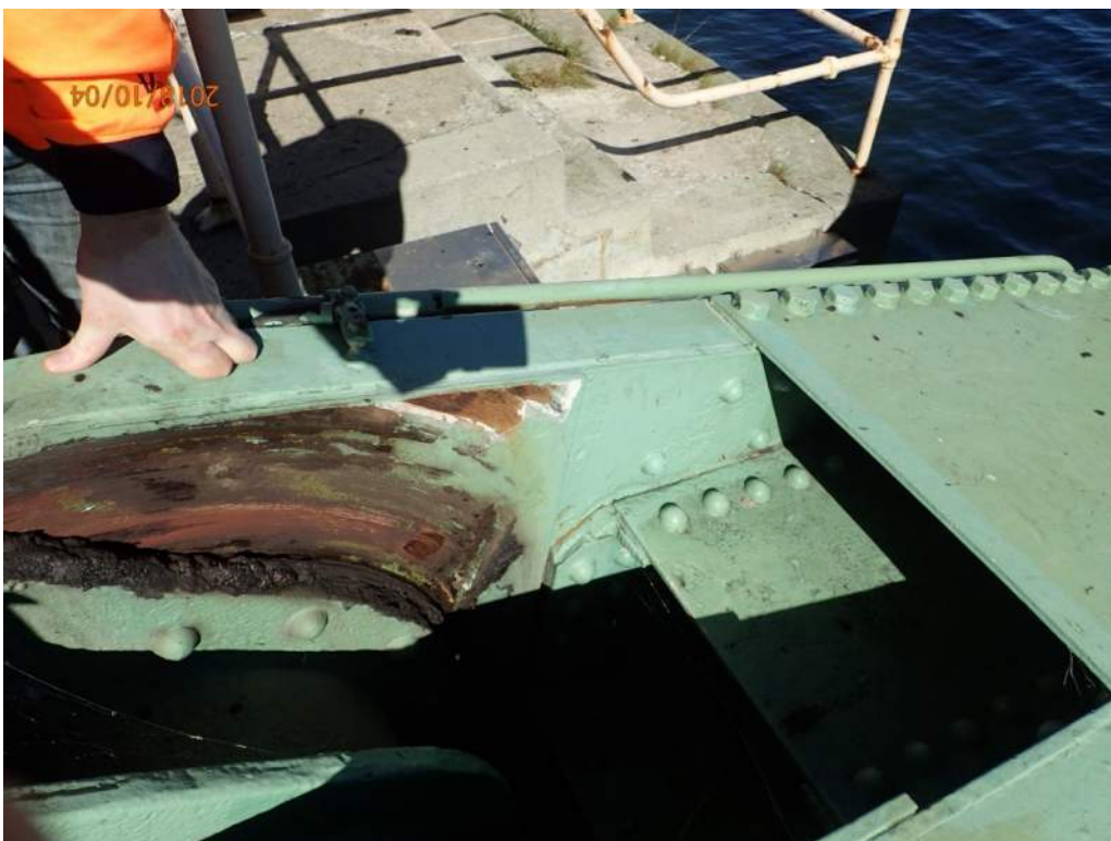
Photo 16: Areas of coating on the interior of the north plate of the north trunnion have been worn away due to contact between the moving structure and the fixed structure.
