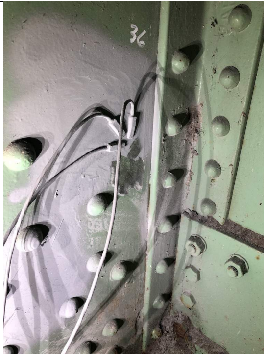
Figure13: Test Location 36 at South Trunnion Exterior Plate Location (Readings Taken on Interior Surface of Plate)
