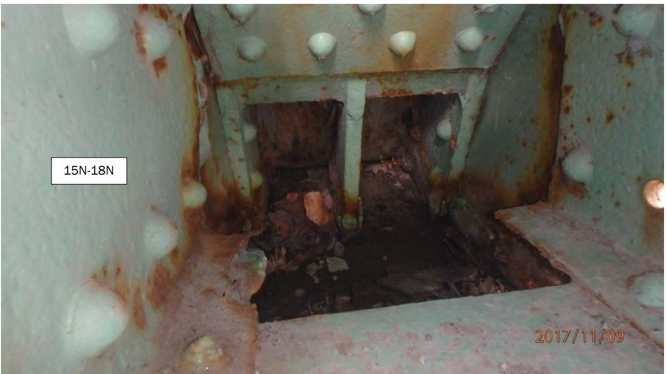
Photo 12: View of the west side of the north trunnion. Note the loss of the bottom flange of the north channel of tower truss member 15N-18N (photo from 2017 inspection).
