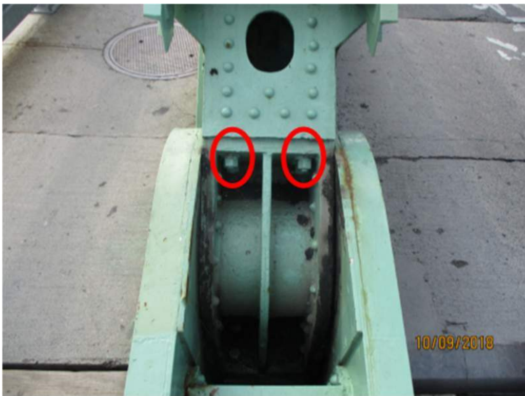
Photo 36: South trunnion. The head end of the four bolts that secure the bearing housing to the structure has 100% section loss due to corrosion. The nut end of these bolts (circled) are pictured (photo by Stafford Bandlow).
