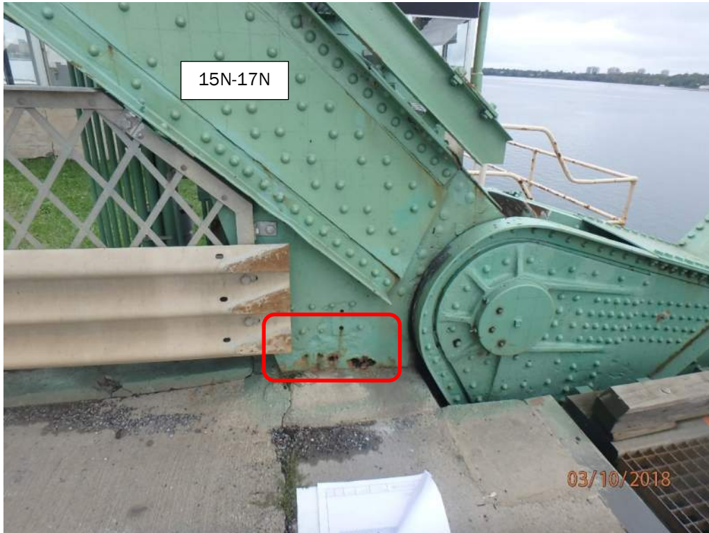
Photo 17: The vertical gusset plate at node 15N at roadway level exhibits very severe section loss and perforations.
