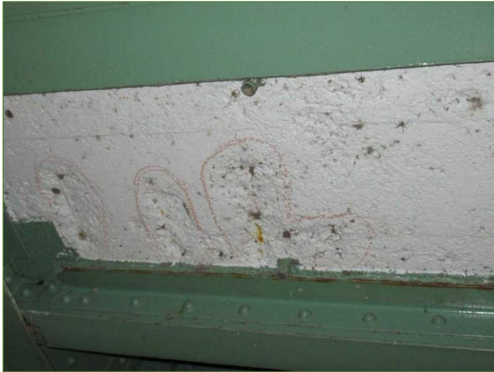
Photo P5 Machinery Room Slab Soffit Deterioration (spall and delamination)
