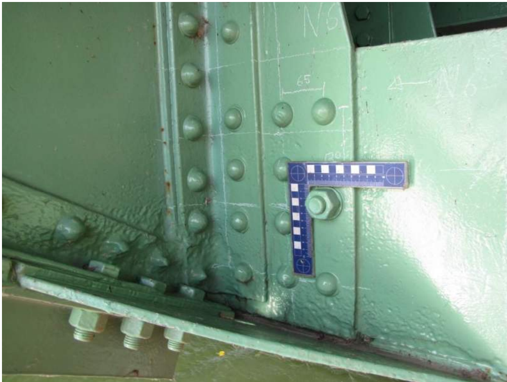
Photo S-56: Typical localized severe pitting and section loss of bottom flange, web, and rivet heads of sidewalk floor beams at the connection to the south truss. Node 6S shown.
