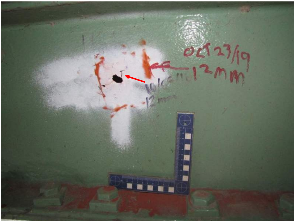
Photo S-21: Two perforations and 12mm long crack in interior channel of bottom chord member 14S-16S.
