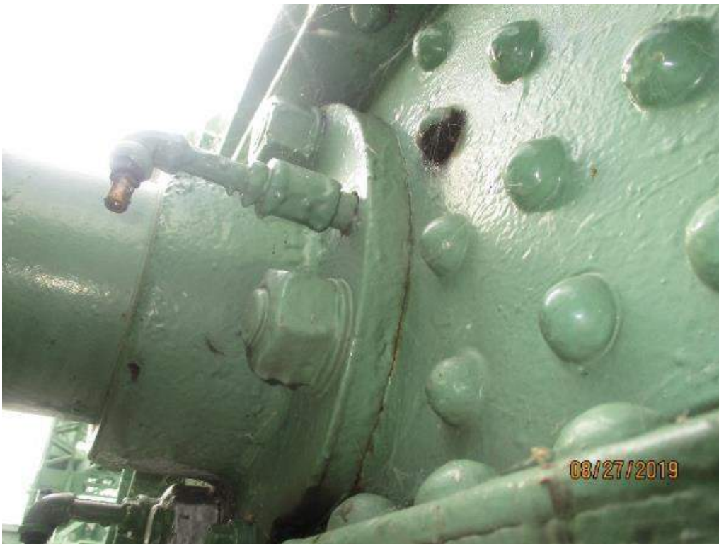
Photo M-15: South Second Link Pin, Inboard Side. There is cracked paint and fretting between the link pin housing and the structure, indicating slight movement.
