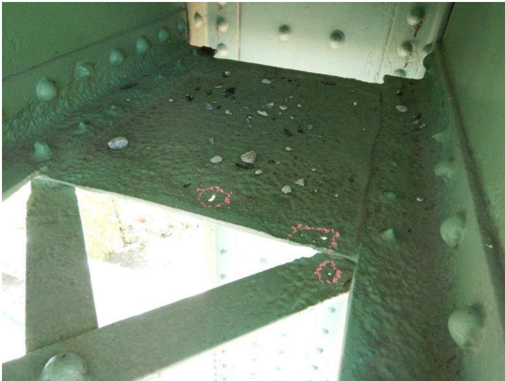
Photo S-91: Tower truss sway bracing member 20N-20S has deep pitting in the bottom gusset plate with 3 small perforations and severe section loss of the rivet heads at node 20S.
