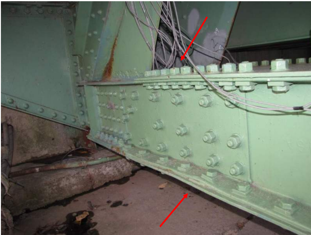
Photo S-20: The top and bottom flanges of bottom chord member 14S-16S have deformed near 16S.
