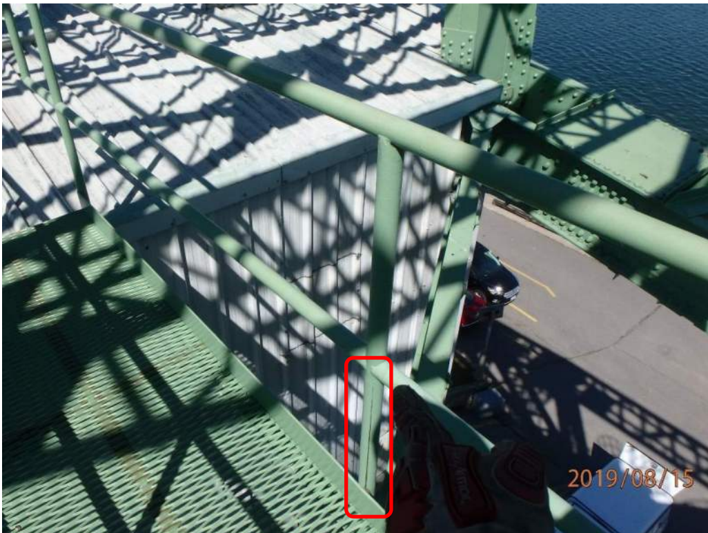
Photo S-121: Several catwalk railing posts have split (second post from west of counterweight catwalk 21-27 north railing shown).
