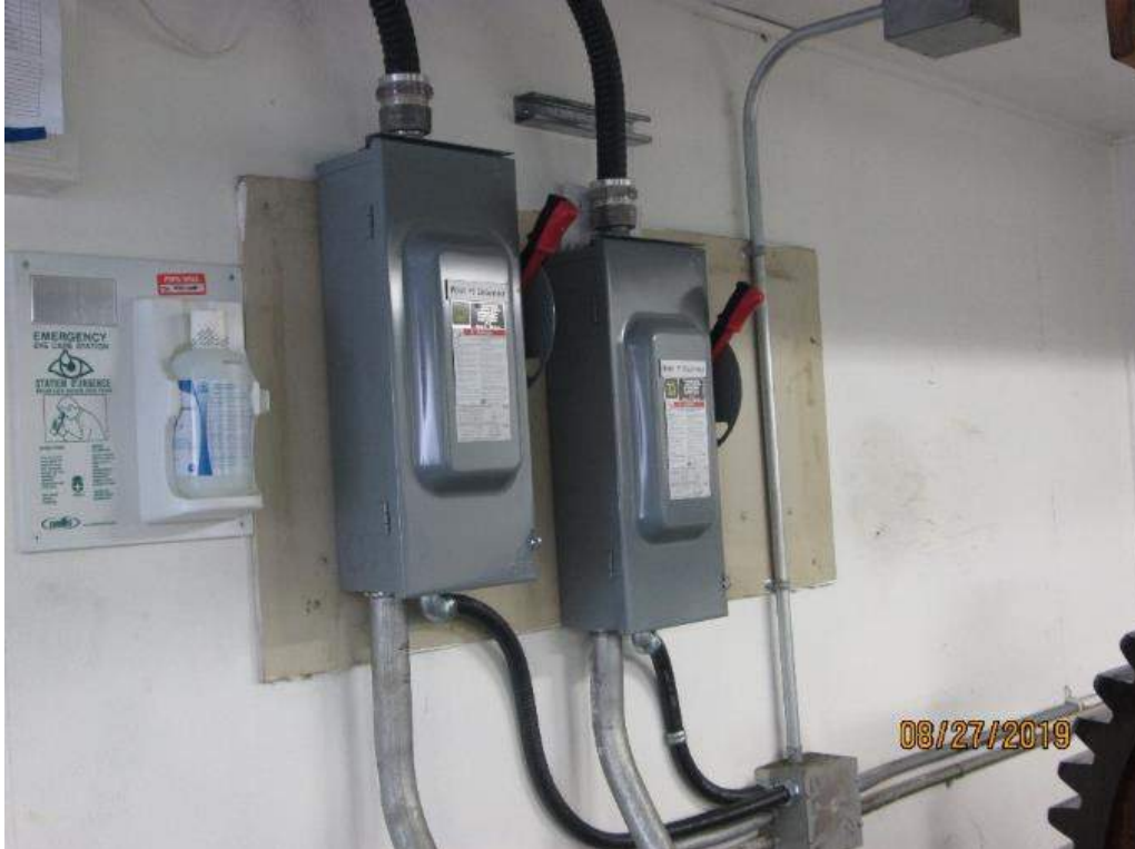
Photo E-10: Span Drive Motor Disconnects. The span drive motors are provided with local disconnect switches as per Canadian Electrical Code. These disconnect switches were installed as the same time as the new drive motors and are in as new condition.
