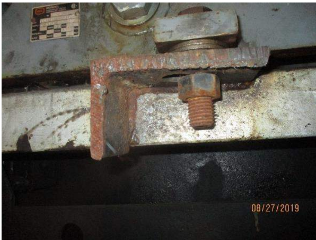
Photo M-2: Span Drive Machinery Brake. The northeast mounting bolt nut has poor bearing. The mounting bolt and surrounding areas are lightly corroded.
