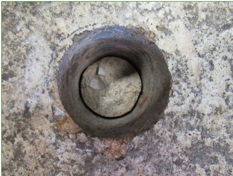
Photo P20 Typical Condition of Inside Core C6
