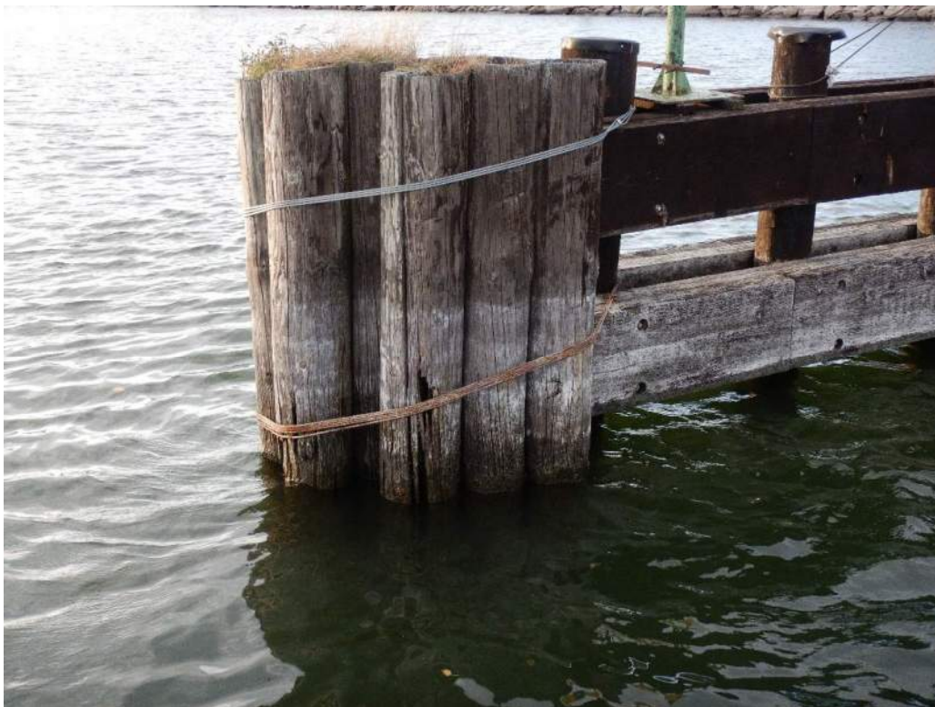
Photo S-113: The lower cables securing the dolphin to the south end of the west fender wall are loose and corroded. One pile has broken off.
