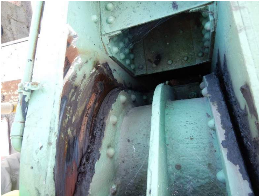
Photo S-82: Areas of coating on the interior of the north plate of the north trunnion have been worn away.
