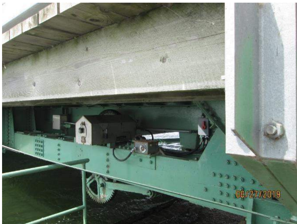
Photo E-16: Span Lock Motor, Rotary Cam Limit Switch (RCLS) and Disconnect Switch. The span lock motor is housed in a stainless steel enclosure and is provided with a local disconnect switch. The span lock is also provided with a two cam limit switch for control, interlock and indication during bridge operation. Note the minor corrosion on the RCLS enclosure.
