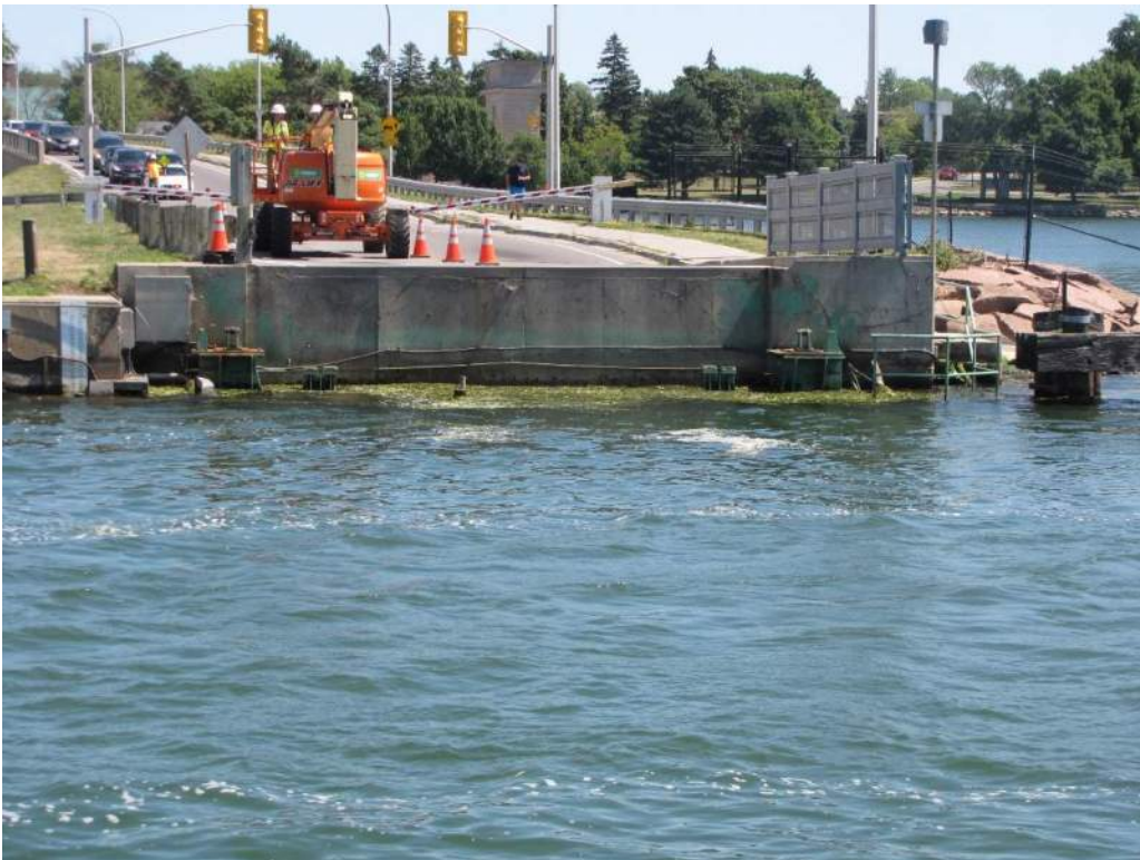
Photo S-9: East ballast wall. Note that the abutment is submerged at the time of the inspection (August 14, 2019).
