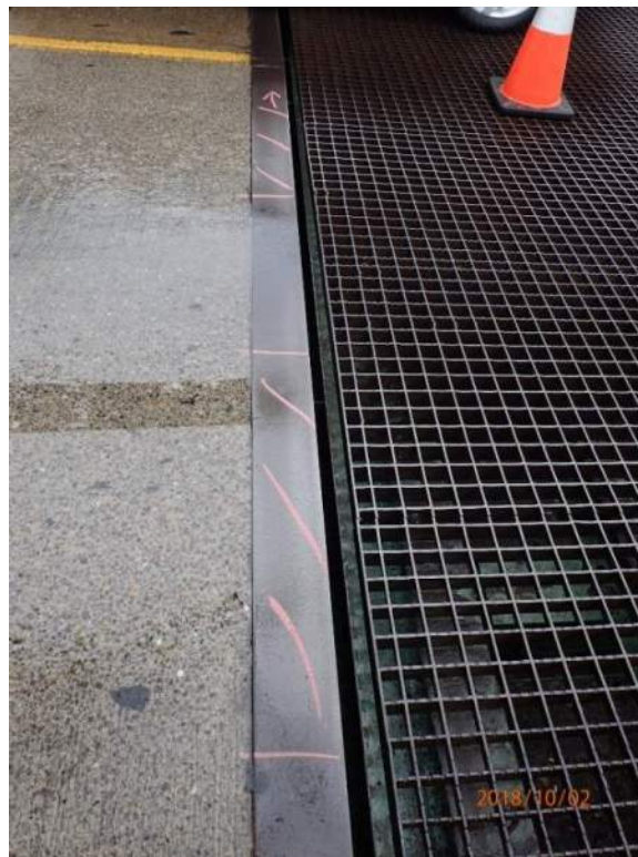
Photo S100: Areas of the west joint armouring sound hollow when sounded, indicating a void between the angle and underlying concrete (photo from 2018 inspection).
