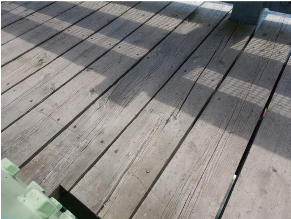
Photo S-103: Light to severe splitting and checks throughout sidewalk timber decking.
