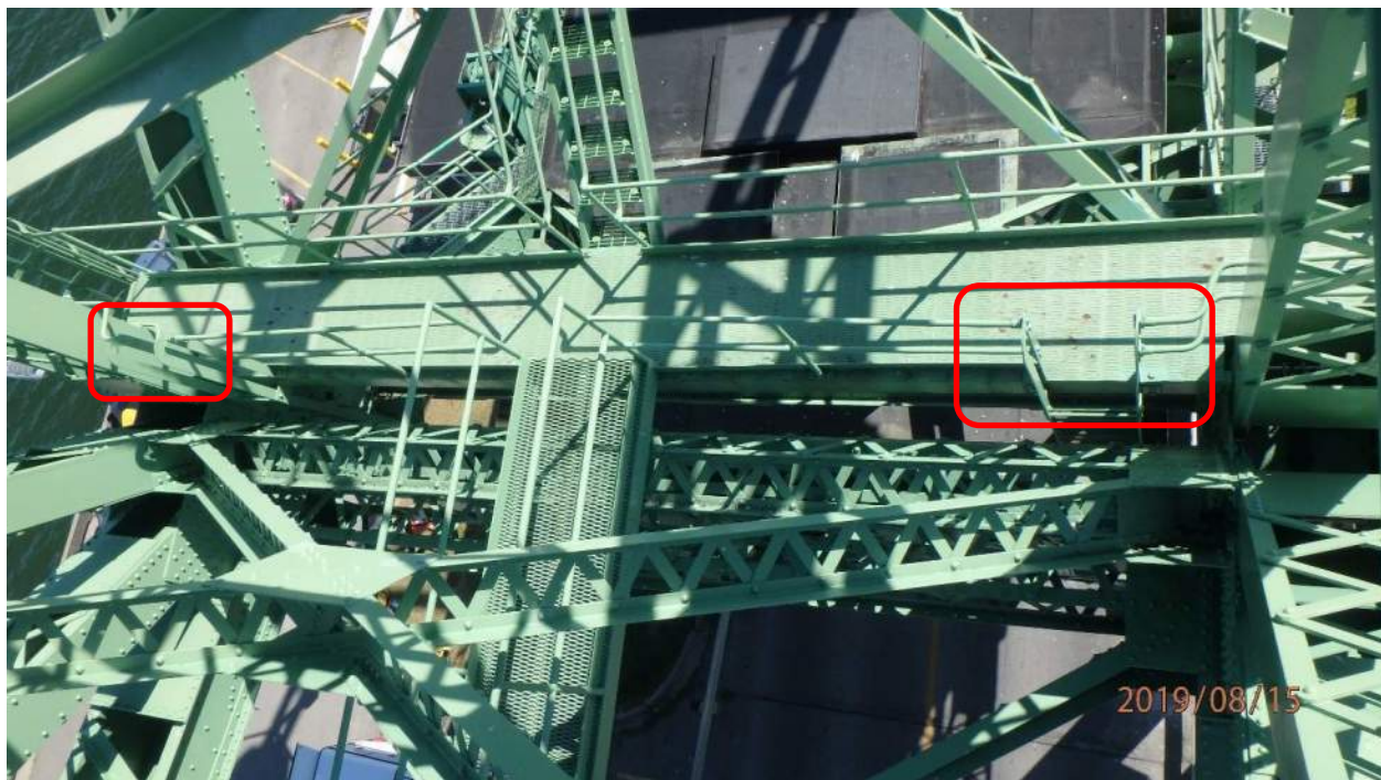
Photo S-119: There are no safety chains across the two open sections of the west railing on catwalk 21N-21S which is a potential falling hazard.
