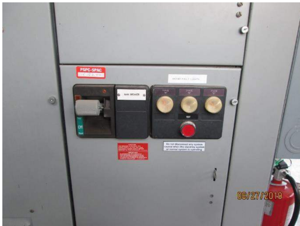
Photo E-6: Ground Fault Indicators. A ground fault indicator light is provided for each phase of the 3-phase power. These indicator lights are provided on the MCC main breaker cubicle and were in an operational condition at the time of the inspection.
