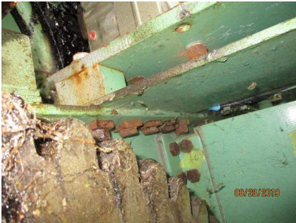
Photo M-17: Span Lock Gearmotor Support. The support mounting bolts are not painted. Note the corrosion.
