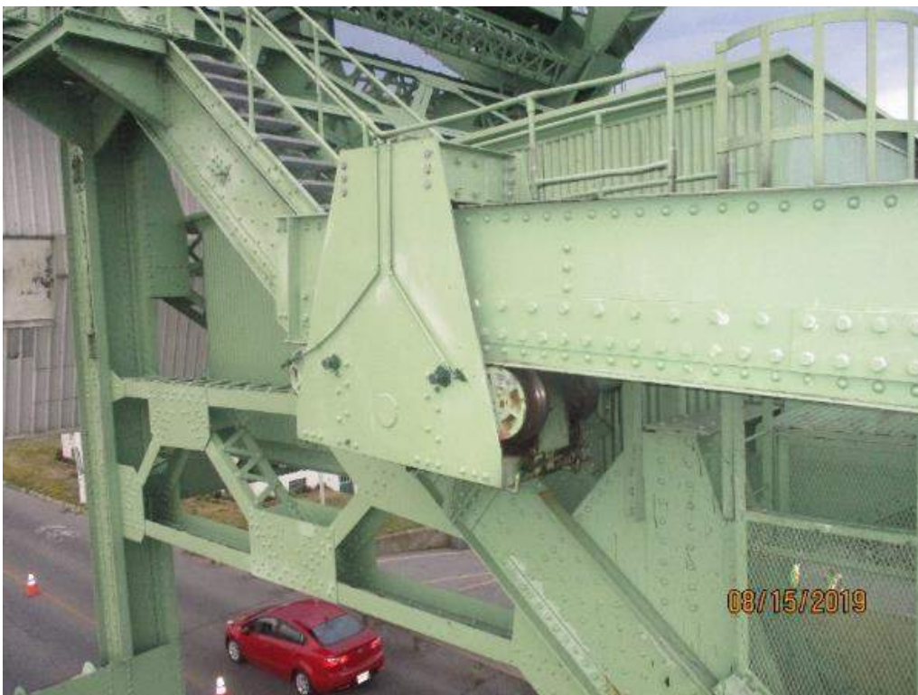
Photo M-8: South Operating Strut Guide Assembly. There is no access to inspect many of the machinery interfaces that are internal to the guide assembly and there is limited access to the assembly from the existing platform. Note that a man-lift was used for additional access at the time of the inspection.
