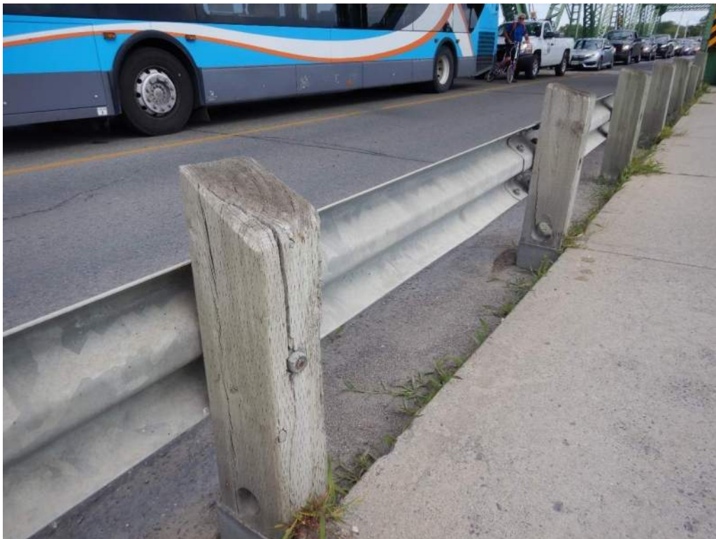
Photo S-111: A timber post in the southwest guiderail has been split by vehicular impact.
