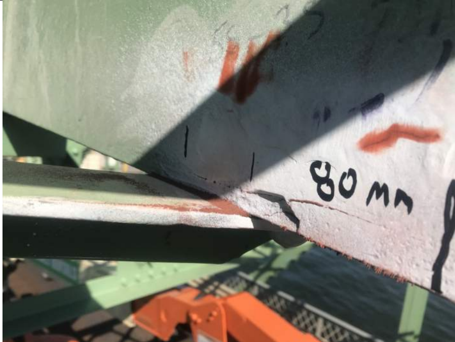
Figure 1: 80mm Crack Identified (Previously Reported as 60mm)
