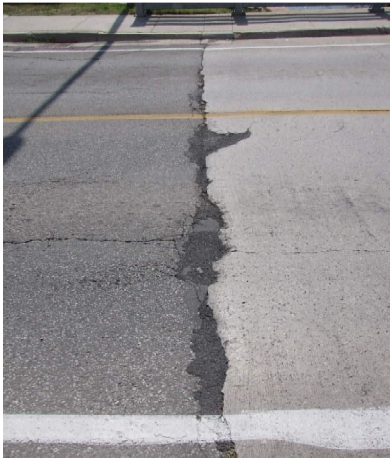
Photo S-110: There is a wide crack and patched potholes at the interface between the east approach slab and adjacent roadway wearing surface.
