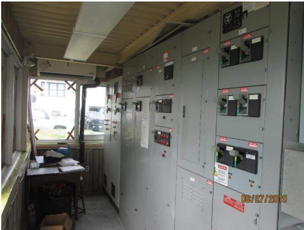
Photo E-5: Motor Control Centre (MCC). The bridge is provided with a motor control center (MCC) for bridge power distribution. The MCC is located inside the operator's control house. The MCC was installed in 1994 and is in fair serviceable condition.
