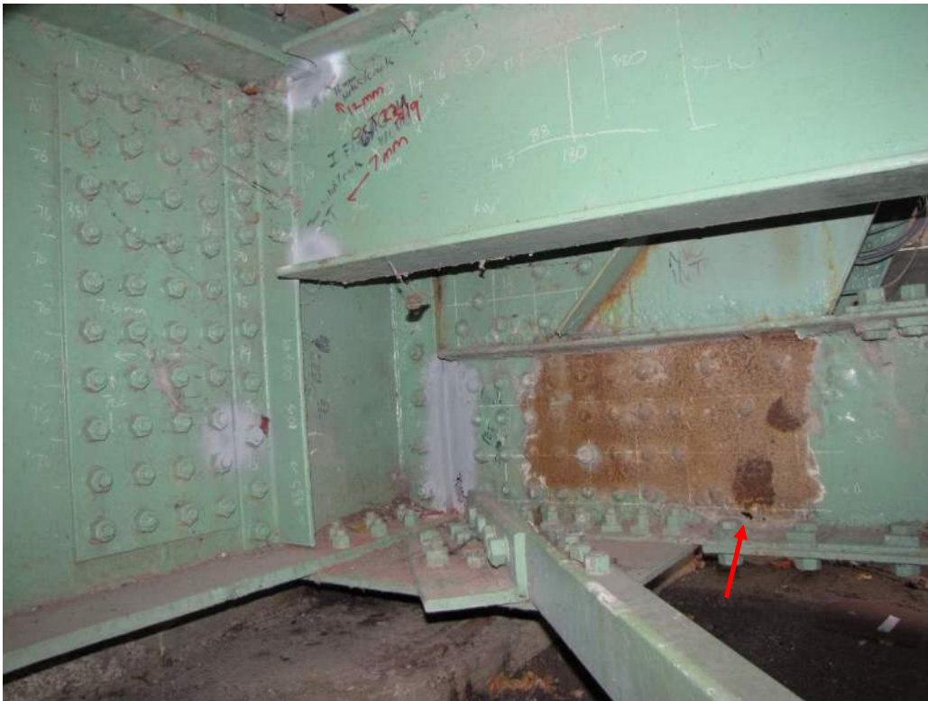
Photo S-16: Perforation in the inner web and generalized light corrosion where coating is missing on bottom chord member 14N-16N near node 16N.
