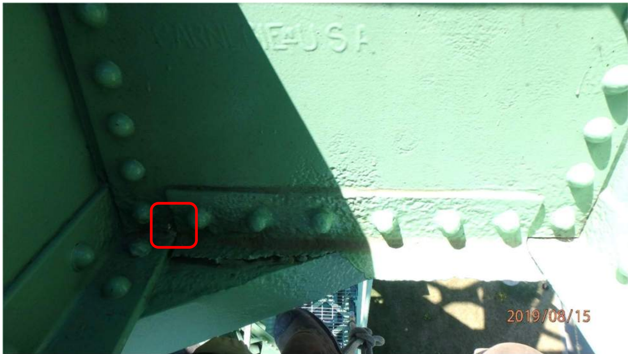
Photo S-42: Localized area of pitting 2-7mm deep with a perforation above the lowest rivet in the lower batten plate on the south side of counterweight truss member 21N-22N. Also note that the outstanding leg of the angle has an area of 100% section loss.
