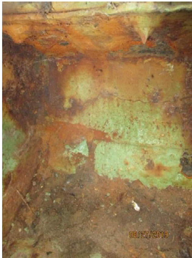
Photo M-13: North Main Trunnion Bearing. The head end of the four bolts that secure the bearing housing to the structure has 100% section loss due to corrosion.
