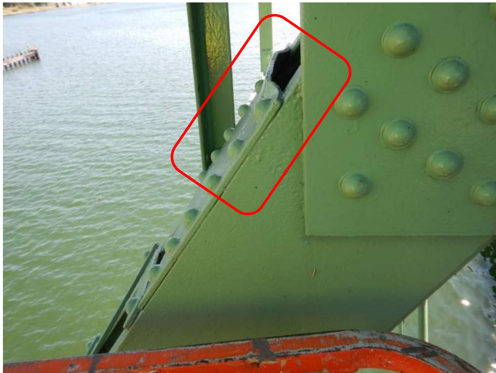
Photo S-25: The upper batten plate of diagonal member 12S-13S near node 13S is deformed.
