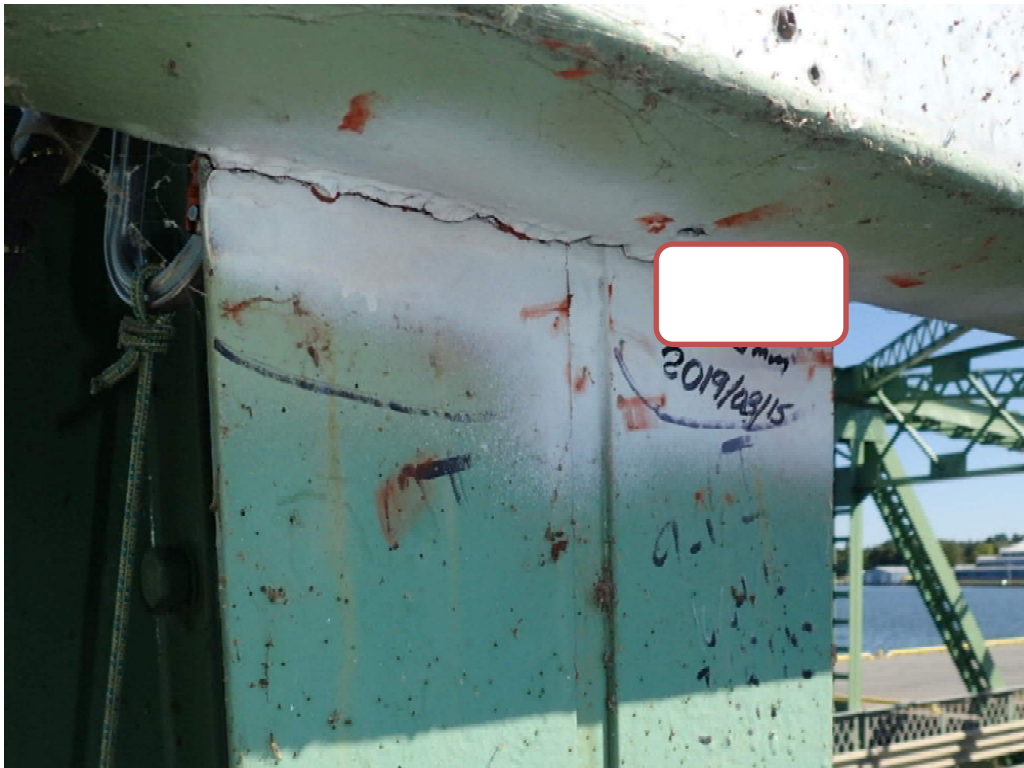
Photo S-31: 3mm long crack in top of southeast leg of vertical member 9S-10S at weld location.
