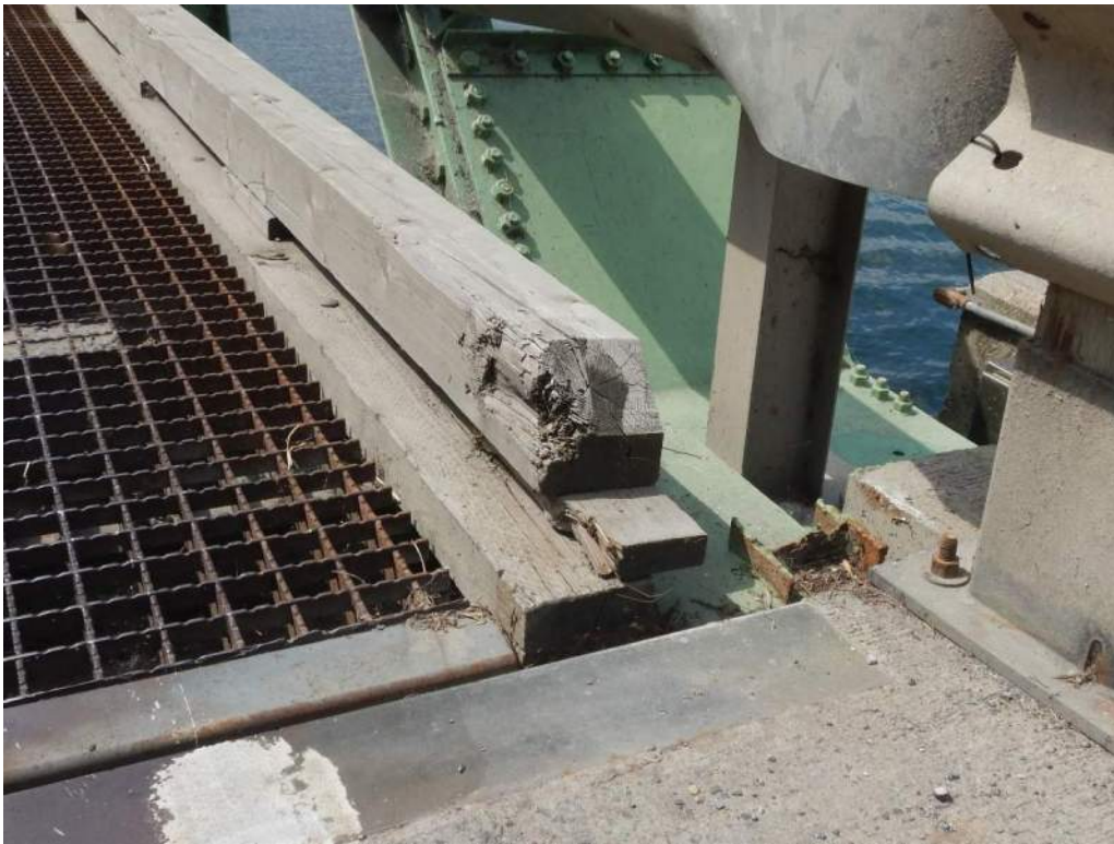
Photo S-102: The east end of the north timber cur has some minor impact damage and is not anchored to the deck.
