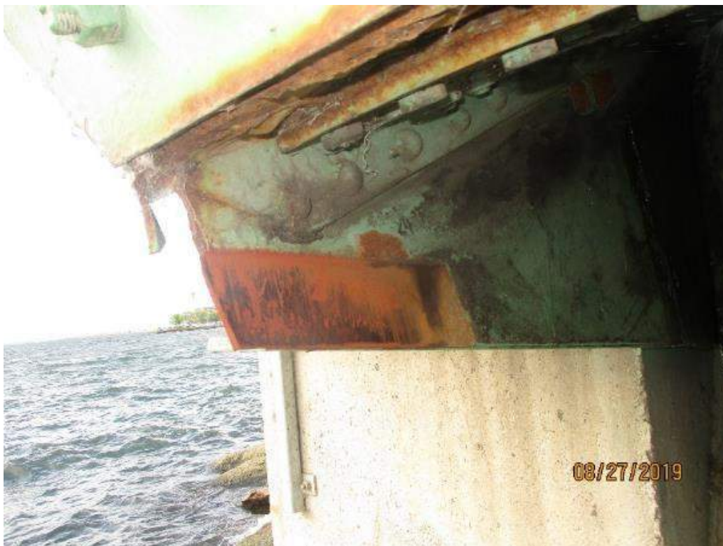
Photo M-12: Truss Near South Main Trunnion Bearing. Note the wear due to contact between the span structure and the bearing support.
