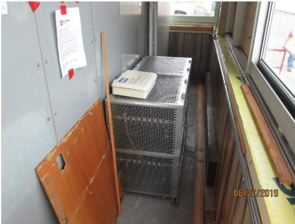
Photo E-9: Typical Dynamic Braking Resistors. Dynamic braking resistors have been installed in conjunction with the VFD drives to provide speed and torque braking control for the span drive motors. These resistors were installed when the VFD drives were installed and are in freestanding enclosures located behind the MCC.
