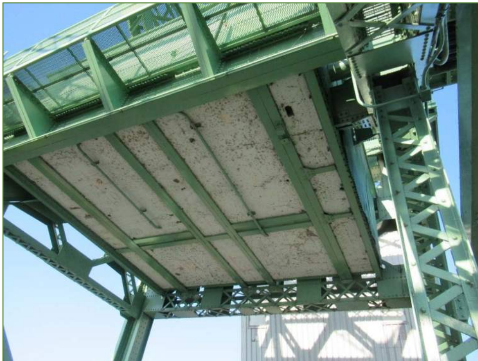
Photo P2 Machinery Room Slab Soffit (fair condition – cracks, spall, delamination, light scaling and honeycombing)
