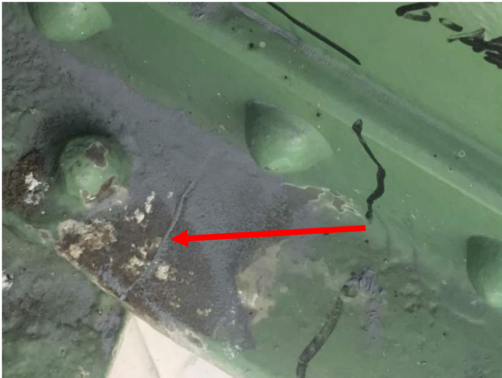
Photo S-40: Crack across full width of bottom leg of interior angle of counterweight truss member 21N-27N at node 27N (photo by Brouco NDT).
