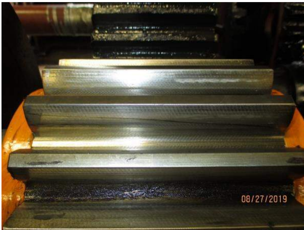
Photo M-6: Span Drive Machinery North Pinon G. The contact wear pattern indicates light cross bearing with heavier contact on the north side of the opening face and heavier contact on the south side of the closing face.
