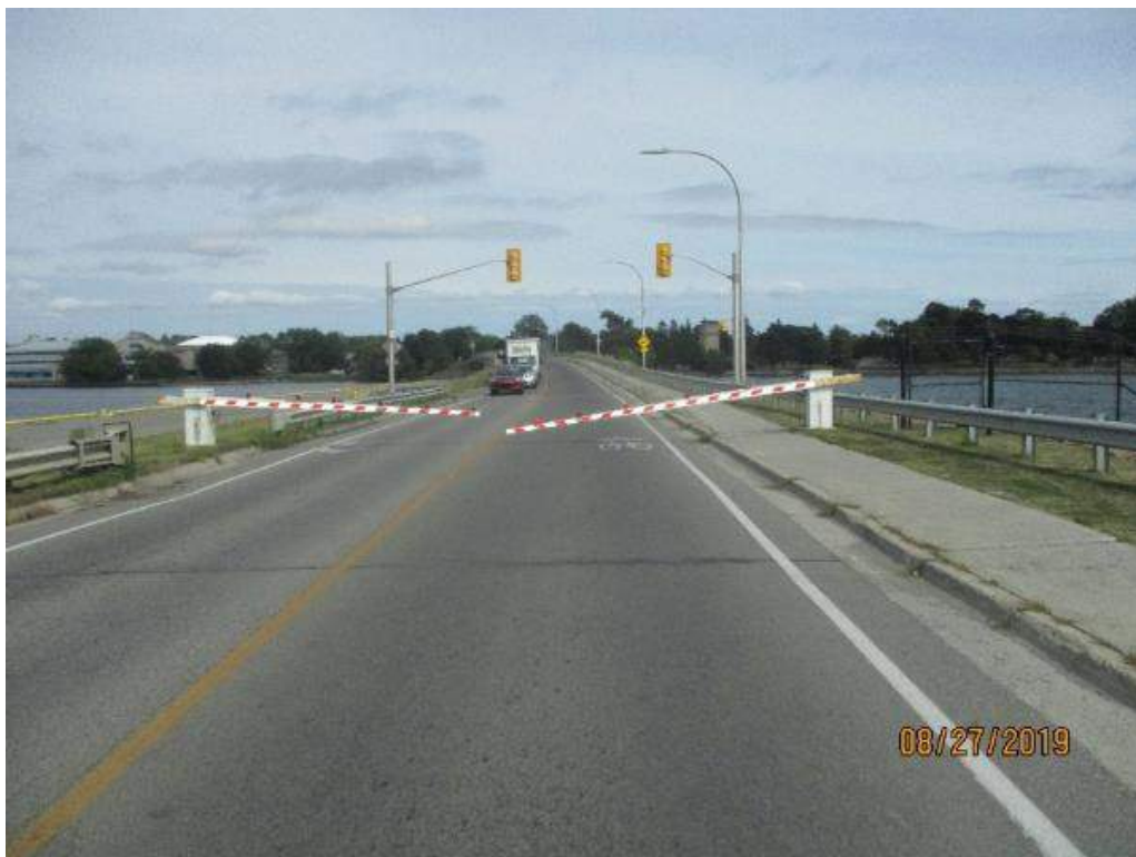
Photo M-30: East Warning Gates. The warning gate arms are not horizontal in the lowered position. The west warning gates are similar.
