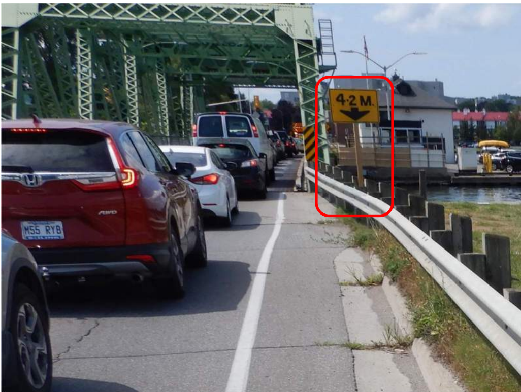
Photo S-117: The west clearance sign has been removed from member 1S-1N and placed on a timber post due to cracked welds in the sign bracket.
