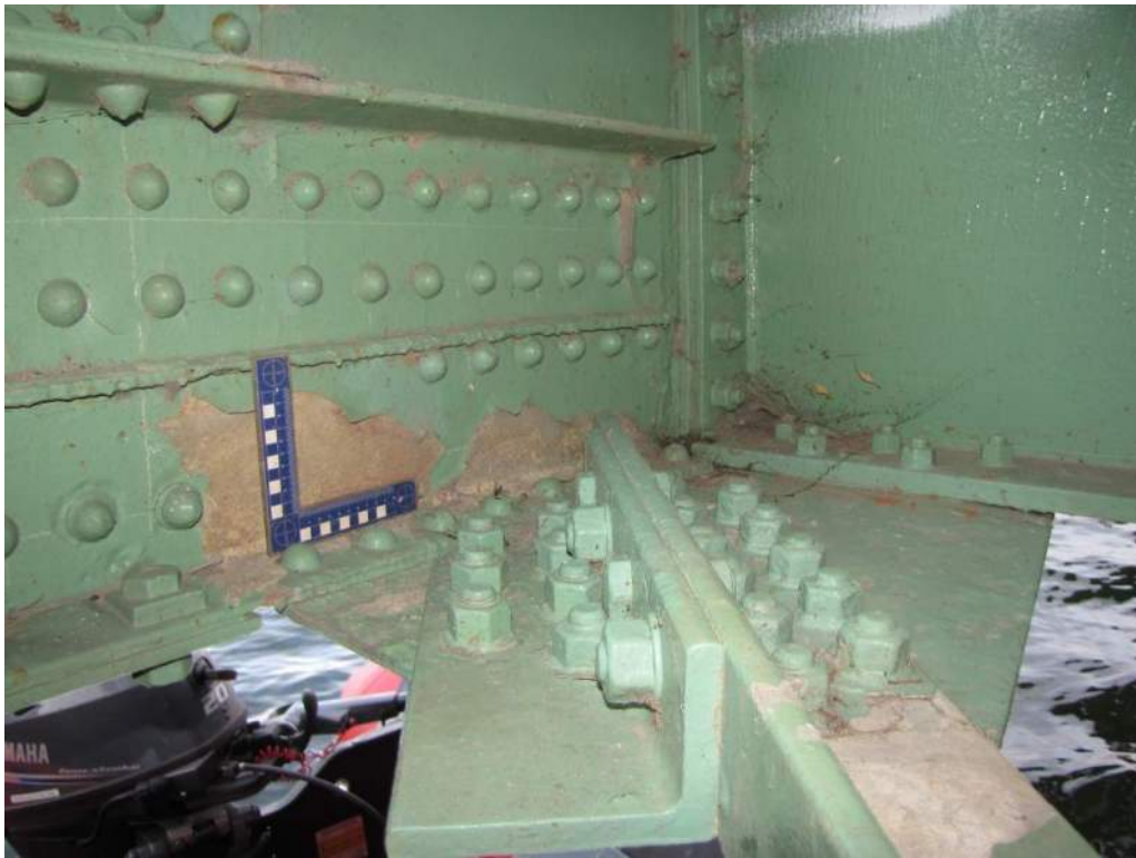
Photo S-74: The painted coating is cracking and peeling off at several locations on the structure (node 14N below deck shown).
