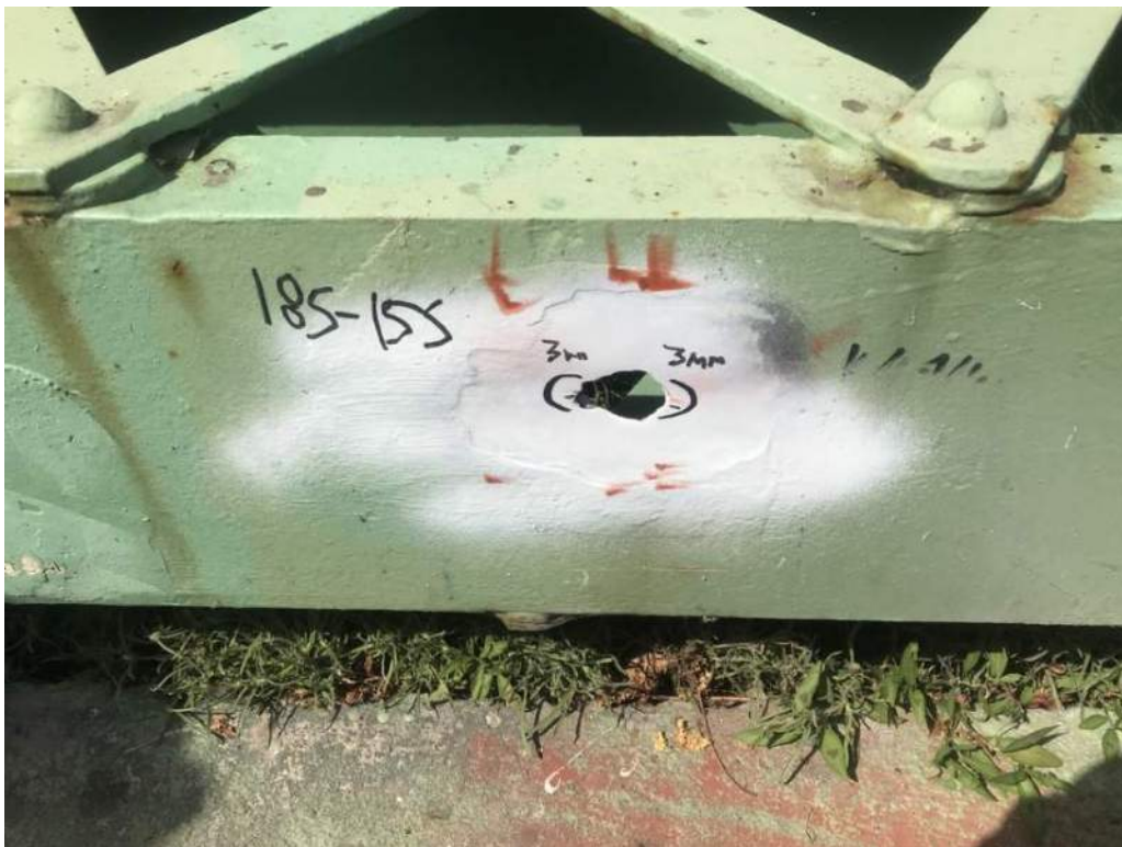
Photo S-37: Perforation and two 3mm long cracks in the south channel of tower truss horizontal member 15S-18S (photo by Brouco NDT).
