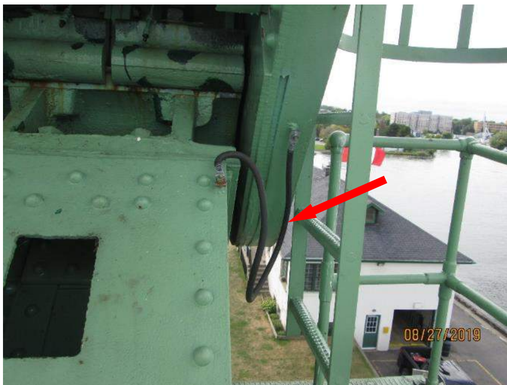
Photo E-34: Bridge Grounding & Bonding System. The bridge steel structures are provided with proper grounding and bonding system in accordance with code.
