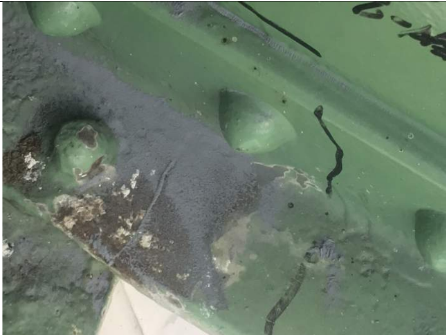
Figure 9: No Change in Crack Length from Previous Report
