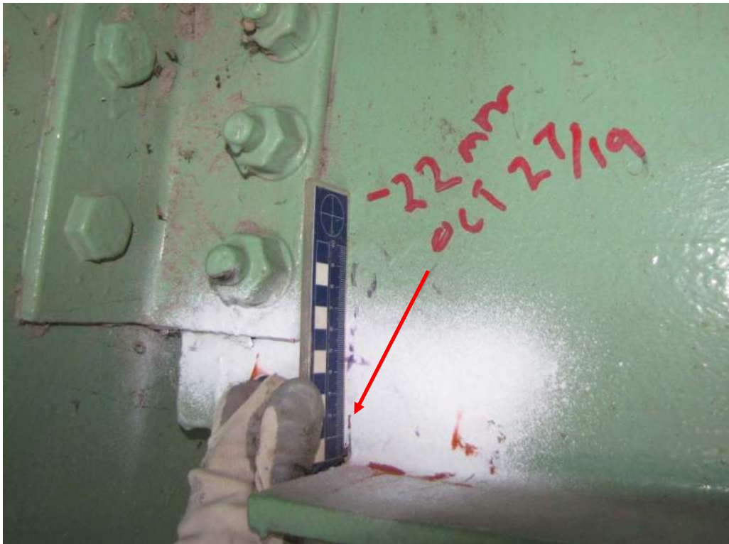
Photo S-58: 22mm notch/crack in the bottom cope of Stringer F (FB2-FB4) at FB2.
