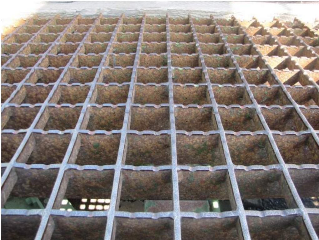
Photo S-75: The roadway grating has widespread light to medium corrosion along the north and south edges (north side shown). The serrated edges have been completely worn away within the wheel tracks.
