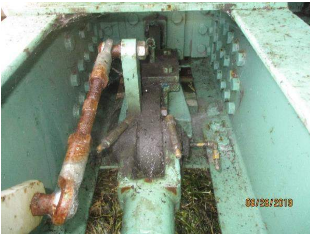
Photo M-22: North Span Lock Crank Shaft CR1. The position indication shaft threads are not painted, and they are lightly corroded. The north location is similar.
