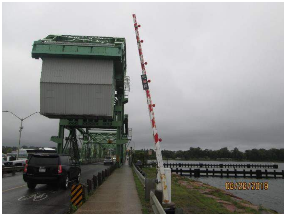
Photo E-26: Typical Traffic Gate (Fully Raised). The bridge is provided with four (4) traffic gates, one at each approach to the span. All gates and gate arm lights were in good operational condition at the time of the inspection. Note the SW gate fully raised position is not adjust to the vertical position.
