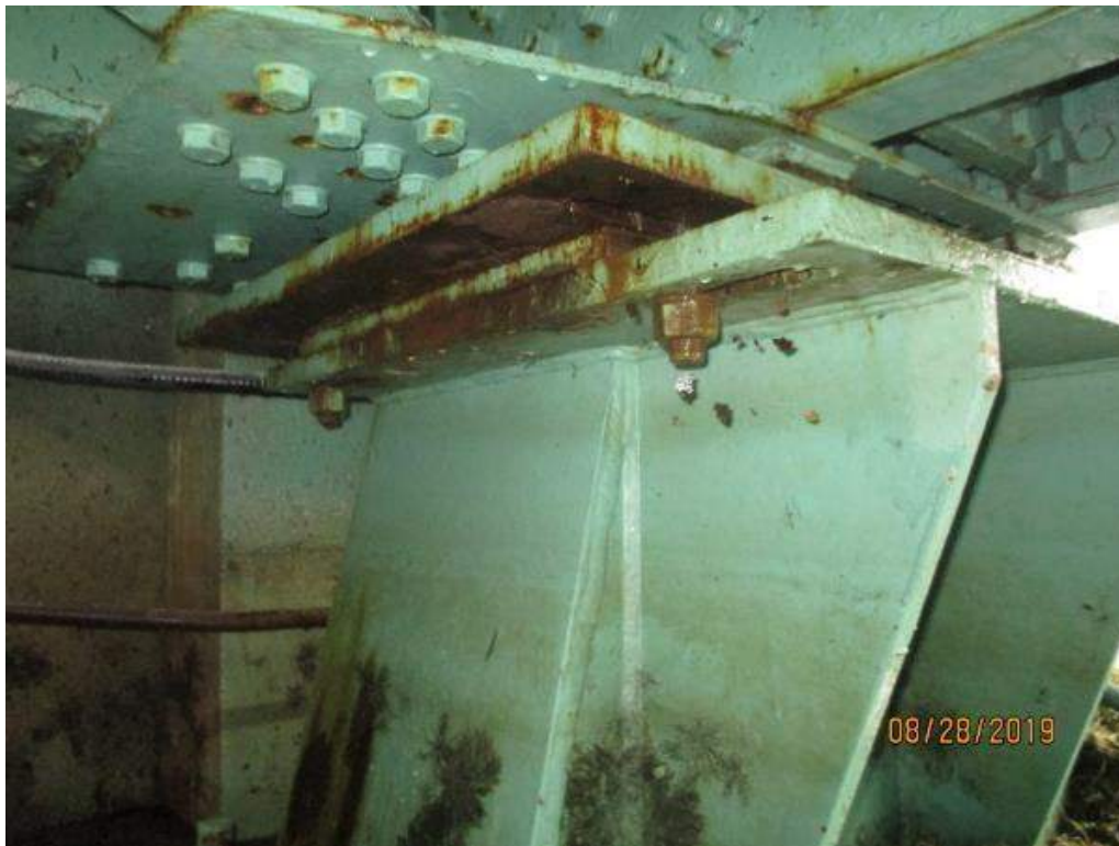
Photo M-27: South Live Load Strike Plate. The underside of the strike plate support and the mounting bolts are corroded. The north live load strike plate assembly is similar.
