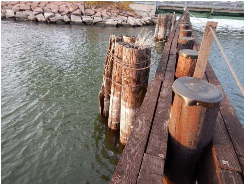
Photo S-114: All pile clusters at the west fender wall have little to no structural strength as they all exhibit rotting, splitting, and crushing (third pile cluster from the north end shown).
