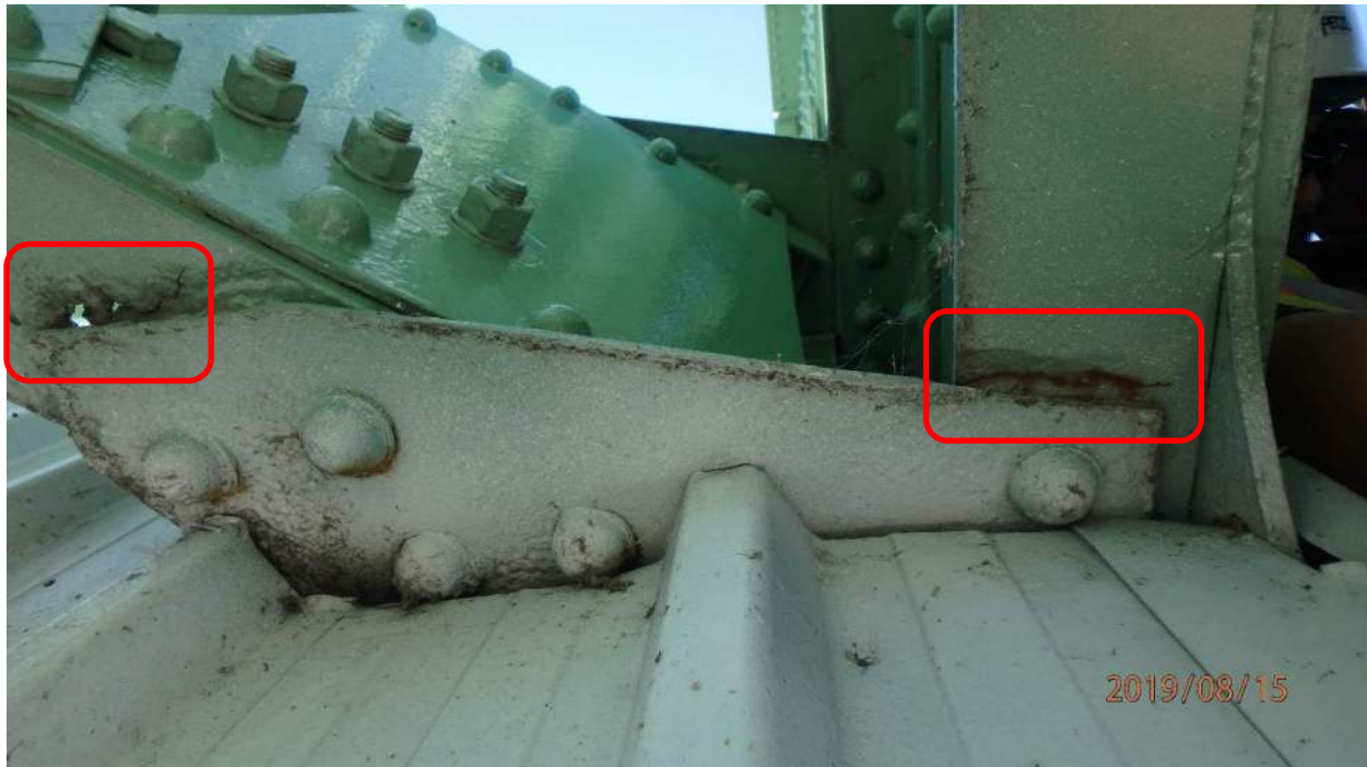
Photo S-41: The northwest end of counterweight truss cross bracing member 21S-27N has several perforations in the lower flange (left). Crack in the south lower flange of member 21N-27N (right).
