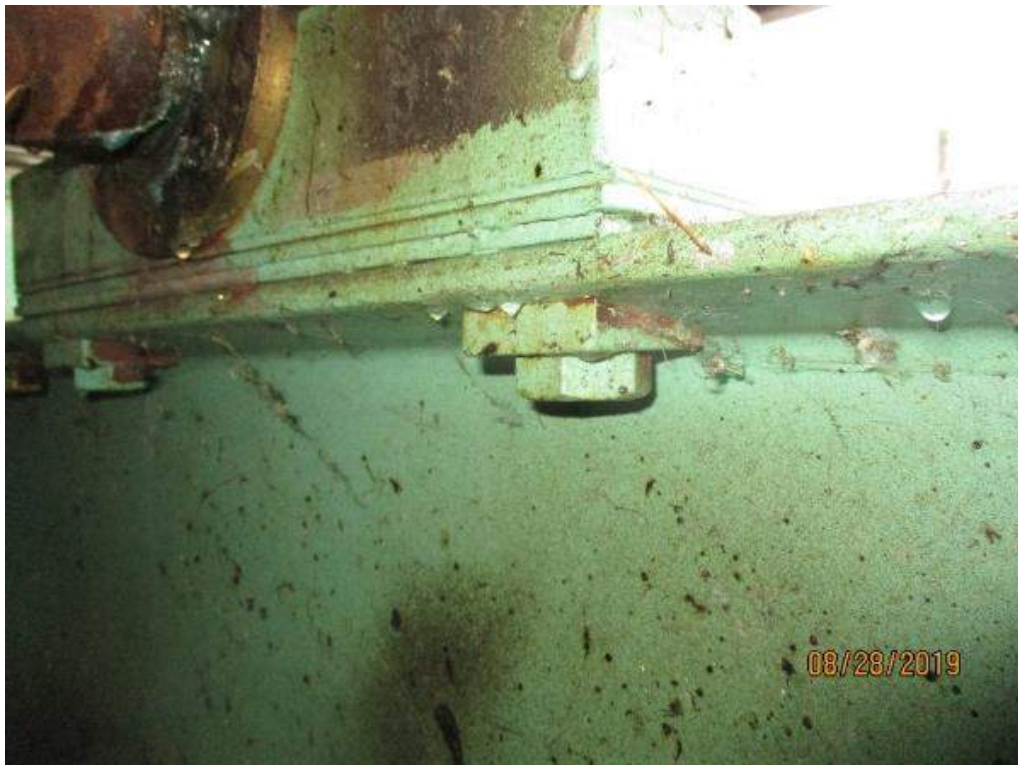
Photo M-18: Span Lock Bearing B4. The span lock mounting bolt underside is not fully painted. Note the light corrosion. The underside of bearing B4 mounting bolts are similar.
