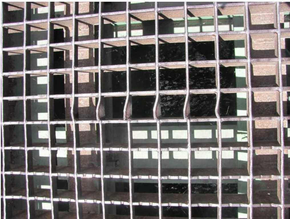
Photo S-77: Broken and bent cross bars in deck grating panel 0-2 F. The serrated edges have been completely worn away within the wheel tracks (at top of photo).
