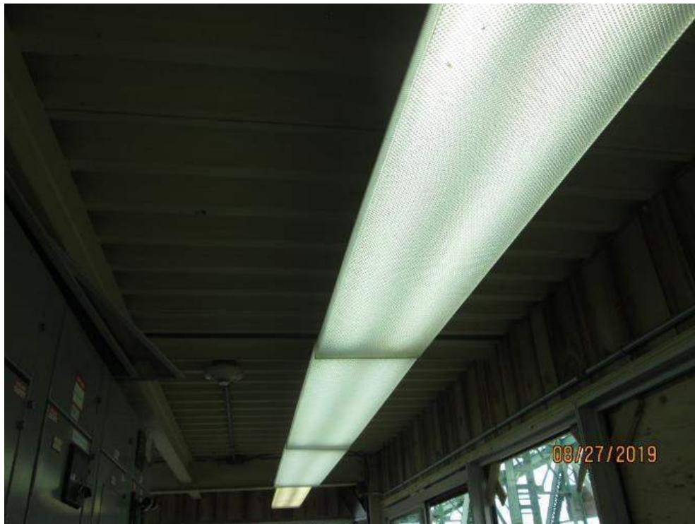
Photo E-36: General and Emergency Lighting. The lighting in the operator's control house provides sufficient illumination level for both operation and maintenance and is in good working condition. The emergency lights were tested at the time of inspection and are operational.
