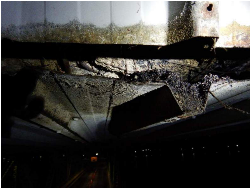
Photo S-72: Disintegrated counterweight concrete accumulating on the soffit cladding of the counterweight on the west side (photo taken after removal of bottom west angle, prior to removal of the debris).
