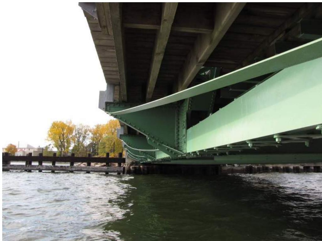
Photo S-95: The bracing members that connect the cantilever sidewalk floor beams are typically sagging.
