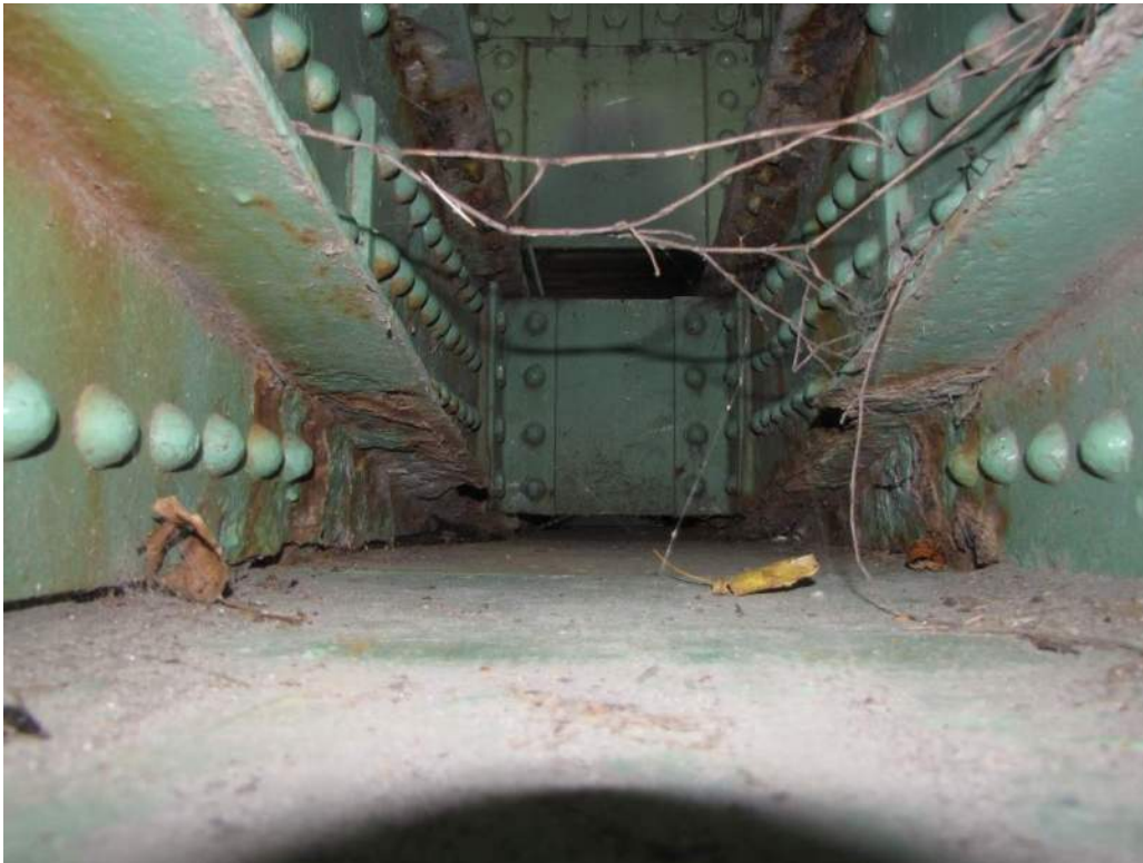
Photo S-22: Severe localized pitting and section loss of flanges where 14S-16S and 14S-15S intersect. Several rivet heads have over 75% section loss.
