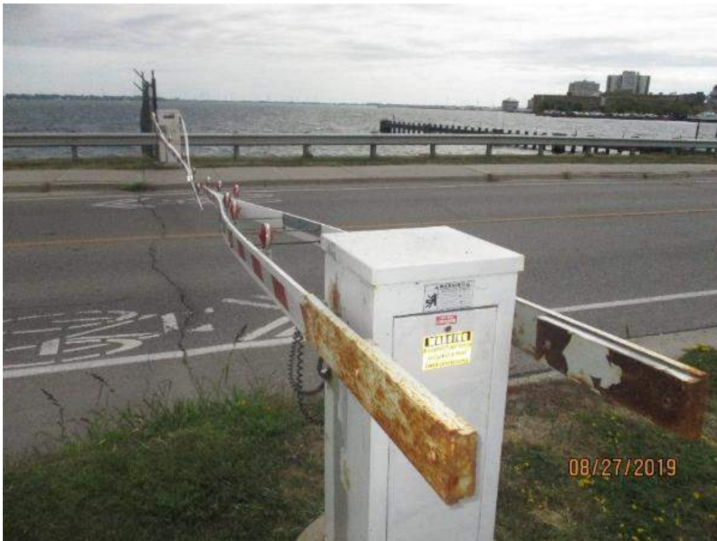
Photo M-29: Southeast Warning Gate. The gate arms and gate housings had spotty areas of corrosion. The other gates are similar.
