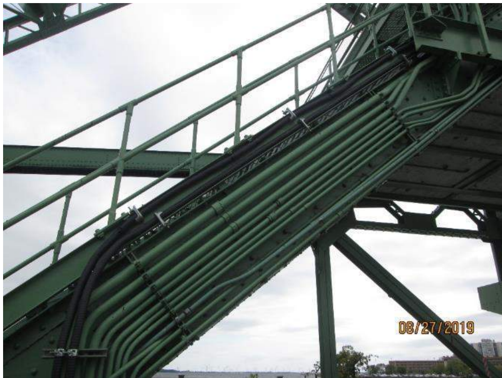
Photo E-40: General Outdoor Installation. The bridge outdoor installation generally consists of Teck cable, painted RGS conduits, and stainless steel junction boxes. The installation is generally in good serviceable condition but with some of the cable/conduit support brackets exhibiting moderate signs of corrosion. The junction box at the bottom of the staircase leading to the machinery space is in poor condition.
