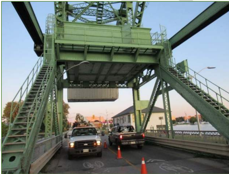
LaSalle Causeway Bascule Bridge – Machinery Room
