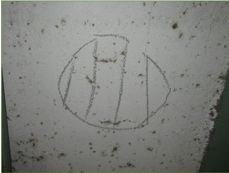
Photo P7 Soffit at Machinery Room (delamination and honeycombing)
