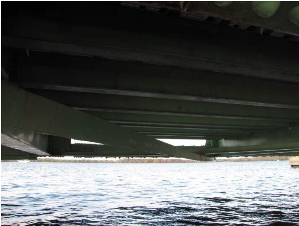
Photo S-94: Lower cross bracing member 10N-12S is deformed.
