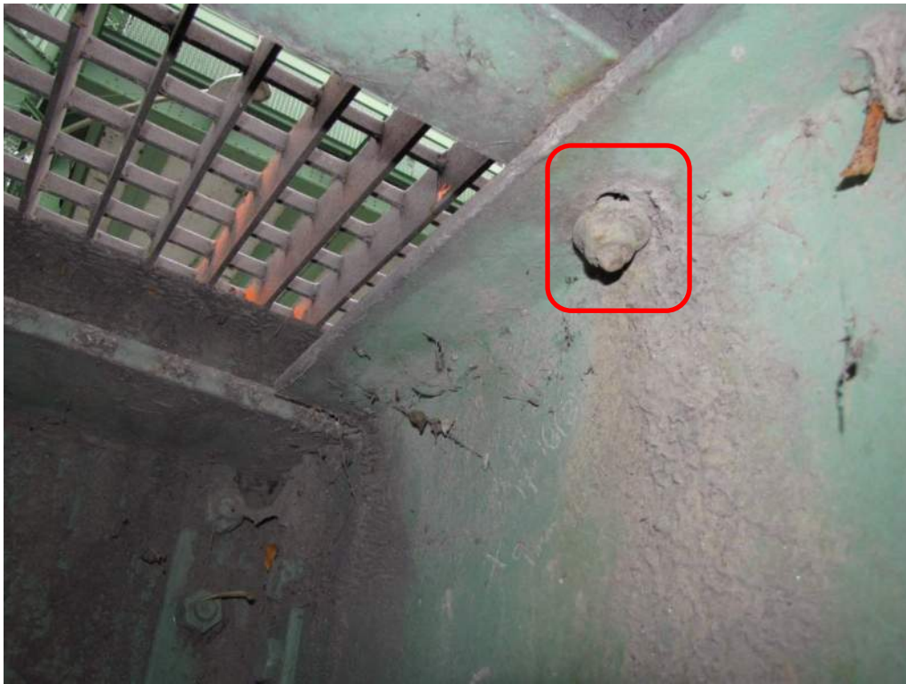
Photo S-64: One of several loose anchor bolts connecting the sills to the stringers. Several others were noted to be missing or severely corroded (not shown).
