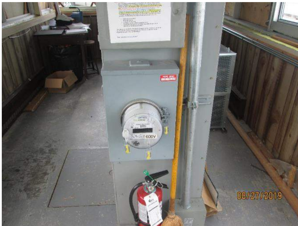
Photo E-1: Utility Meter. The bridge electric service is provided with a utility meter that is located inside the operator's control house and is mounted on the side of the MCC. Note both the meter and metering pan are in good condition.
