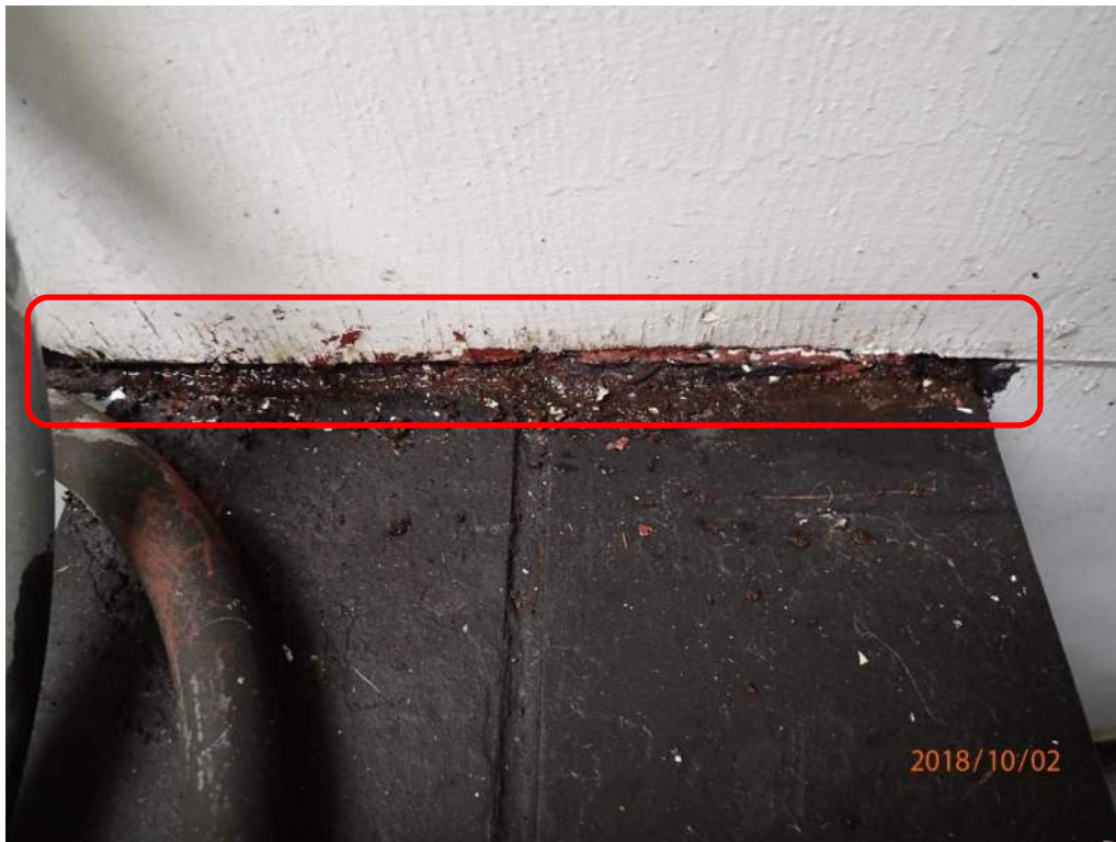
Photo S-97: Water was leaking into the northwest corner of the mechanical room during the inspection. Over time this has caused corrosion of the top flange of one of the steel beams supporting the motors. (photo from 2018 CDI).
