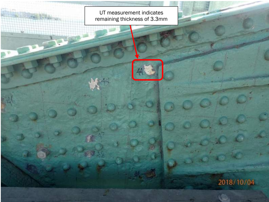
Photo S-51: The north (roadway) side of the south trunnion has widespread pitting in the collar plate (right side), connection plate (left side) and some rivet heads (photo from 2018 CDI).
