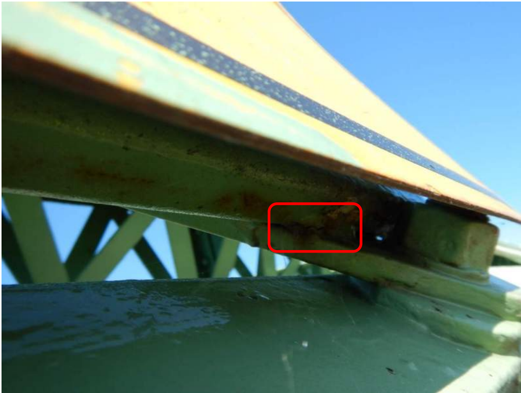
Photo S-116: Cracked weld of the east clearance sign bracket.
