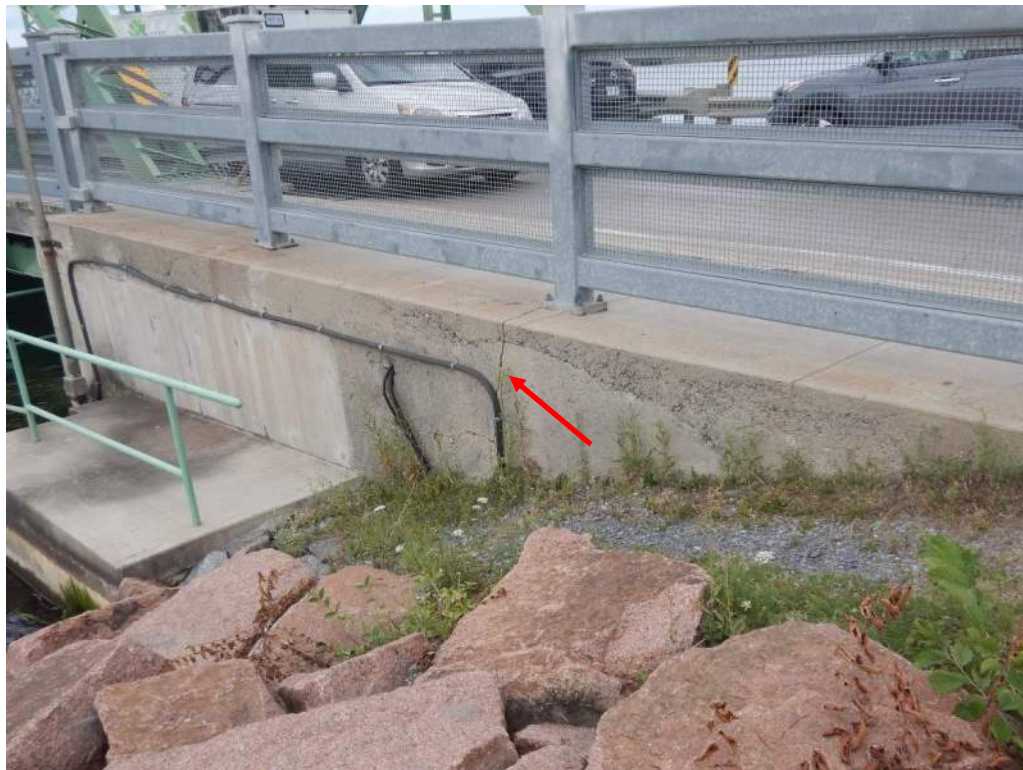
Photo S-105: The southeast wingwall exhibits extensive light honeycombing and a 10mm wide vertical crack extending into the concrete approach sidewalk.
