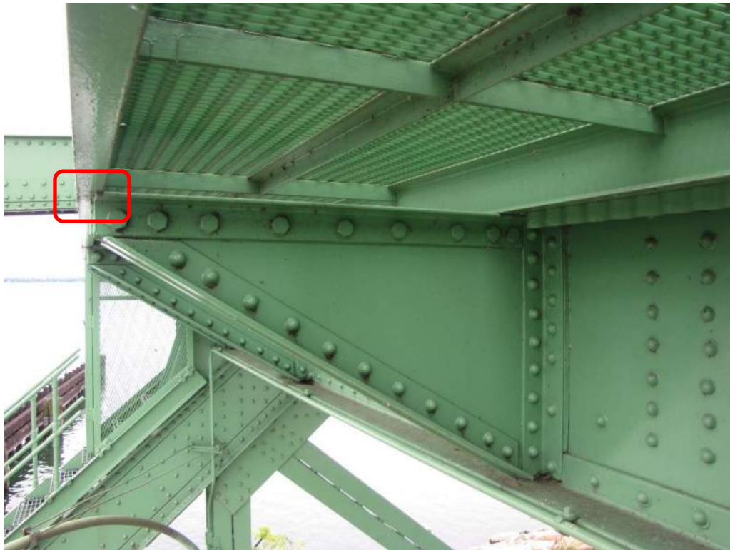
Photo S-118: The east C-channel supporting the catwalk outside the mechanical room is supported by the tapered cantilevered members below but only 25mm of the bottom flange is actually supported (photo from 2018 CDI).
