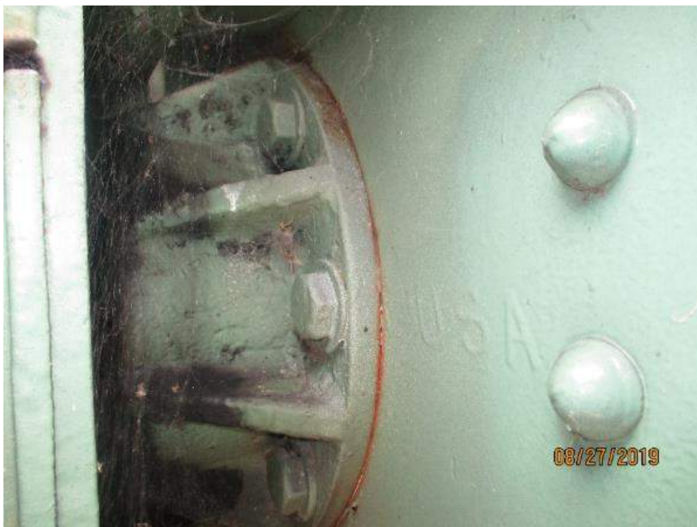
Photo M-10: North Operating Strut, Inboard Bearing. The cracked paint and fretting corrosion between the bearing housing and structure indicate relative movement.
