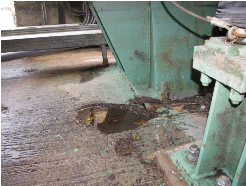
Photo S-84: Spall in the east bearing seat with an area of about 500mm 2 .
