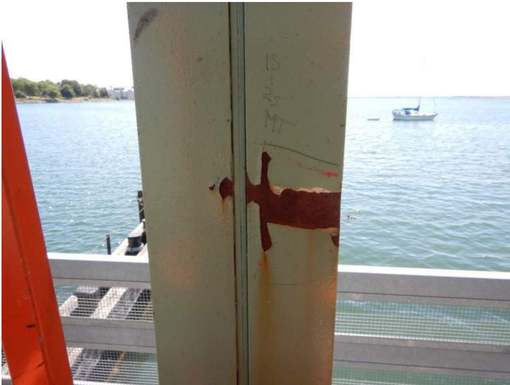
Photo S-30: Impact damage to vertical member 1S-2S has caused the northwest flange to be slightly bent, caused coating damage allowing light corrosion to occur.
