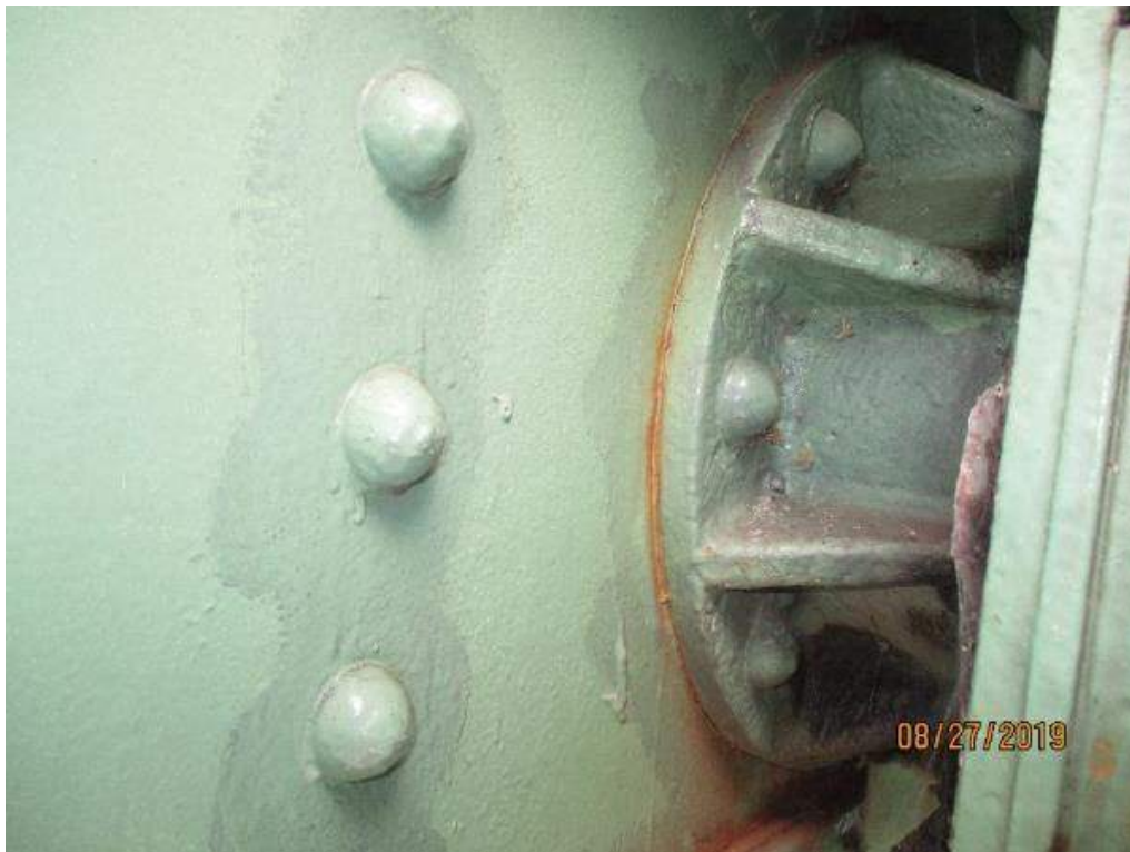
Photo M-9: South Operating Strut, Outboard Bearing. The cracked paint and fretting corrosion between the bearing housing and structure indicate relative movement.
