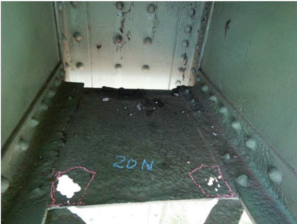
Photo S-90: Tower truss sway bracing member 20N-20S has several perforations and deep pitting in the bottom gusset plate and severe section loss of the rivet heads at node 20N.
