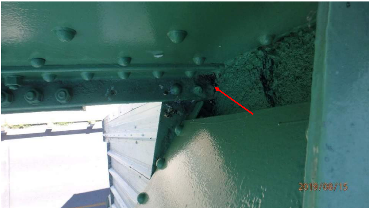
Photo S-93: Counterweight truss member 21S-27N has severe localized section loss of the lower south angle at the west end at node 27N.
