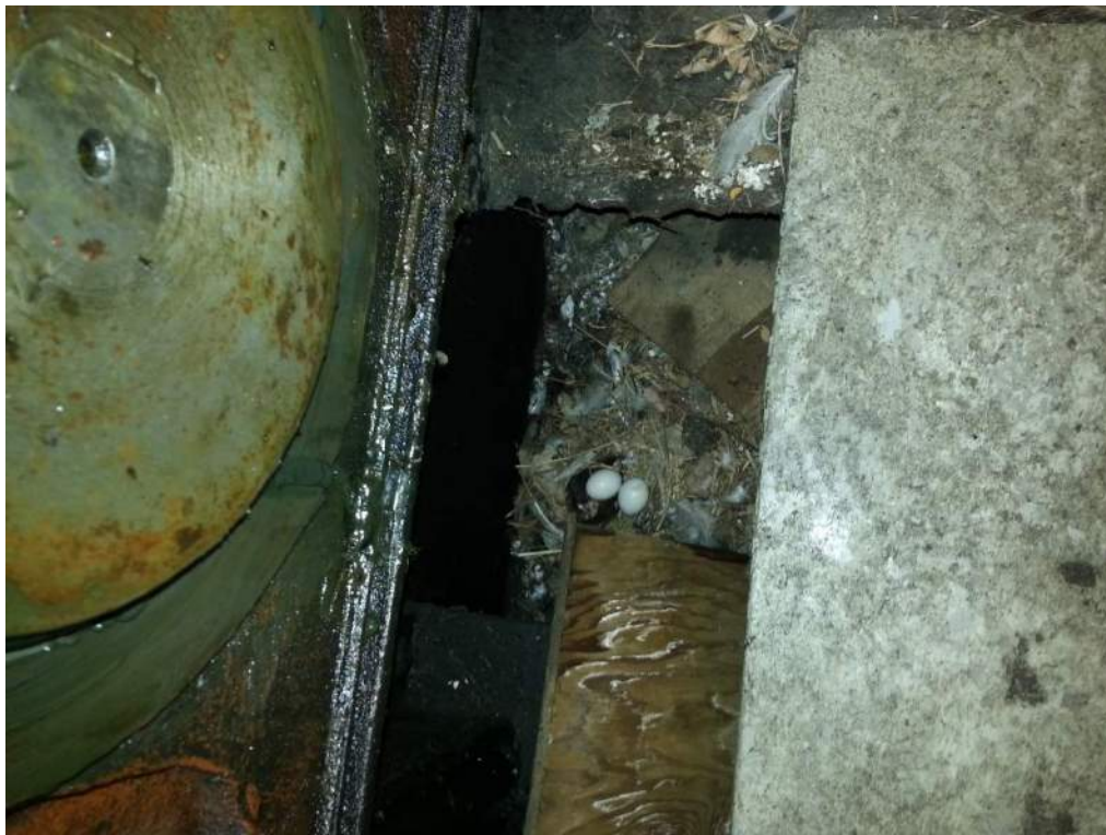
Photo S-99: Bird's nest with eggs in the mechanical room at the south side at time of August 2019 inspection.
