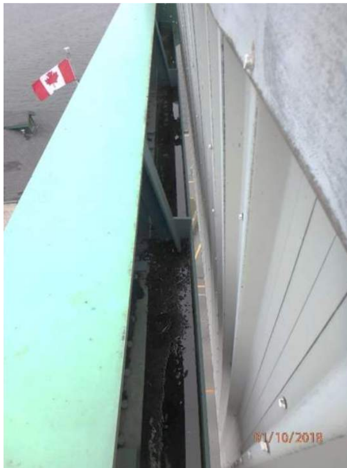
Photo S-43: Debris and water collecting on member 26N-26S (photo from 2018 CDI).
