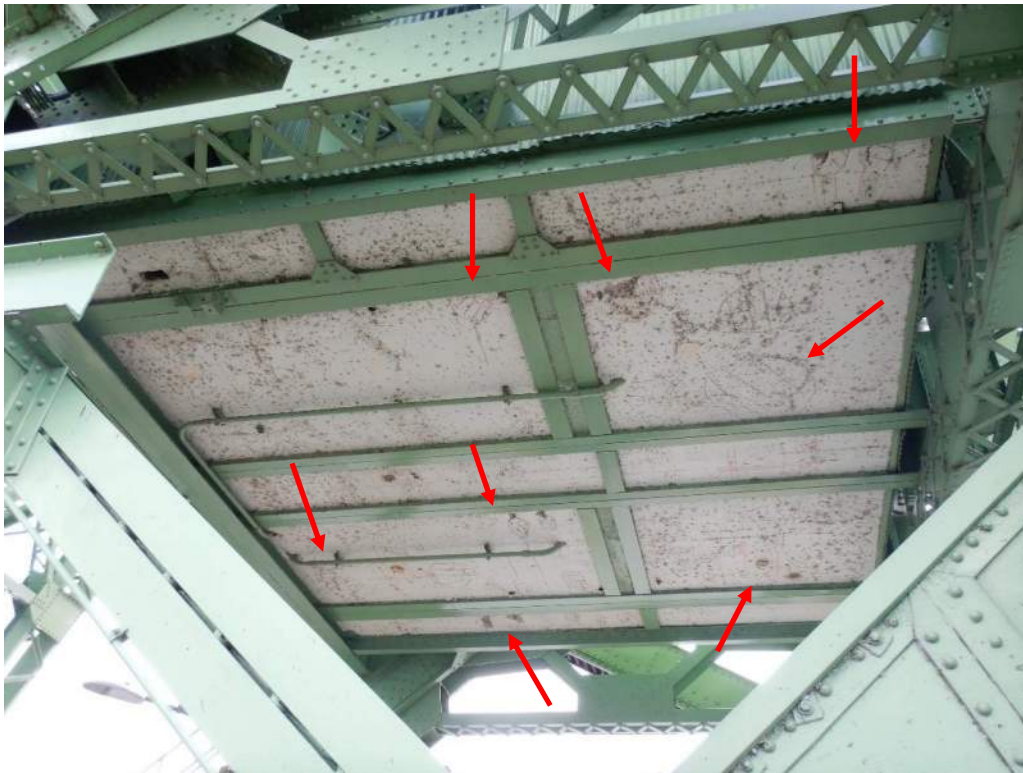
Photo S-96: The mechanical room soffit exhibits several spalls and delaminated areas (some areas indicated). Scaling of the delaminated areas is recommended as they are located over the roadway.
