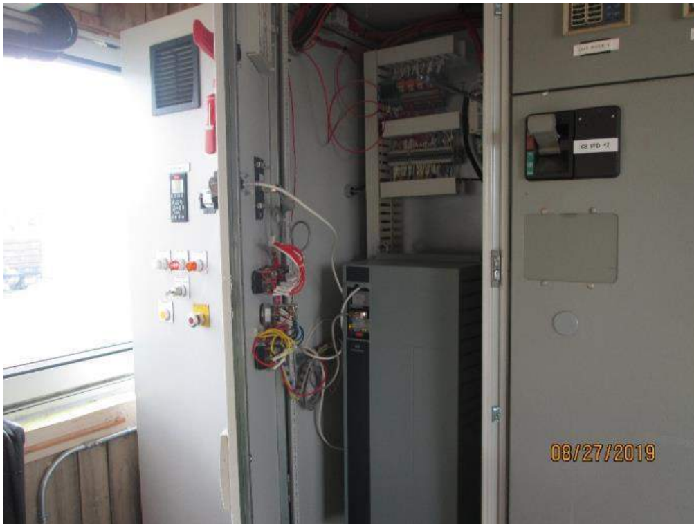
Photo E-7: Span VFD Drive Cabinet. The span variable frequency drives are newly installed and replace the original drive motor controllers for the span drive. The new VFD drives are located in their respective drive enclosures and provide excellent and variable speed and torque control for the operating bridge.
