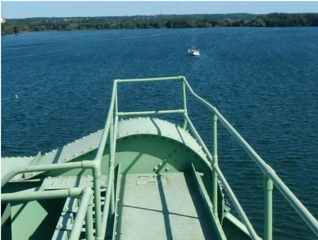
Photo S-120: The east handrail is bent above node 22N.
