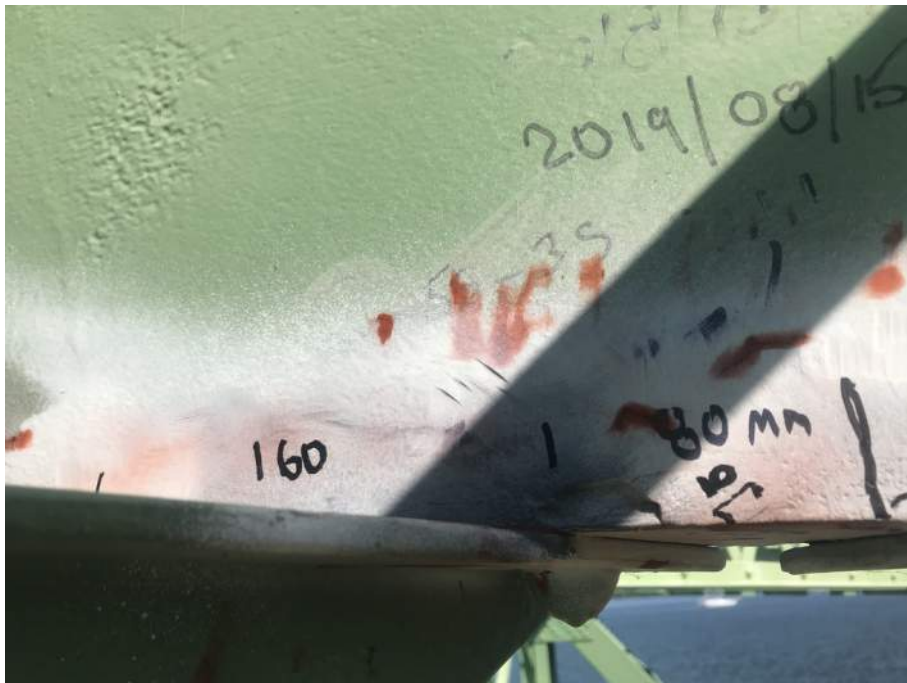
Figure 4: 3mm Crack Branching off of the Bottom
