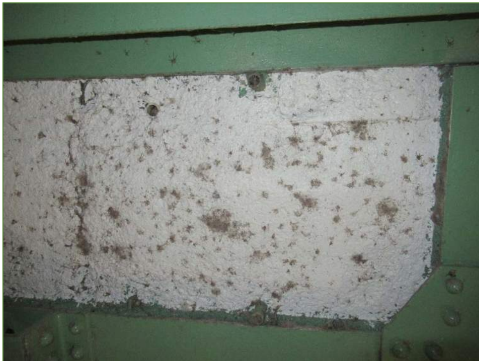
Photo P10 Machinery Room Slab Soffit Deterioration (medium scaling)
