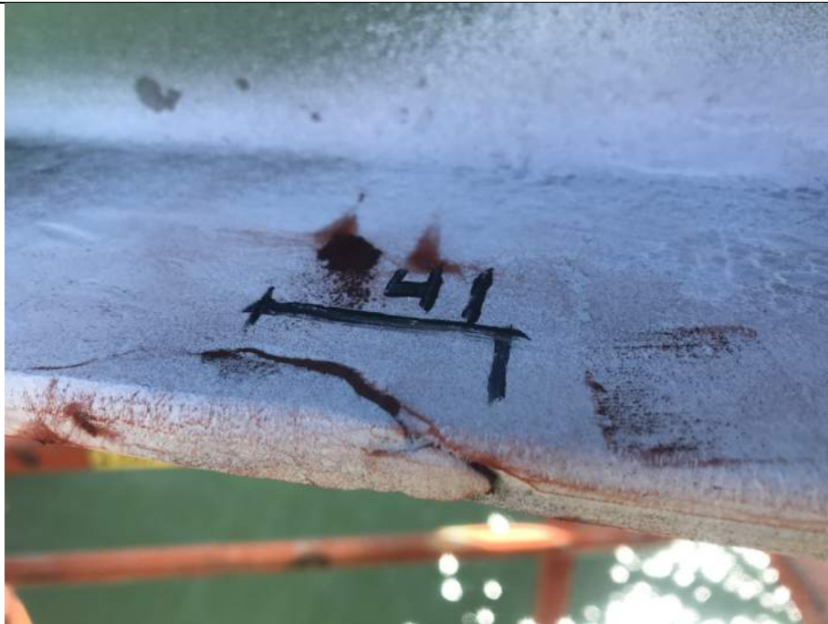
Figure 5: 41mm Crack Detected
