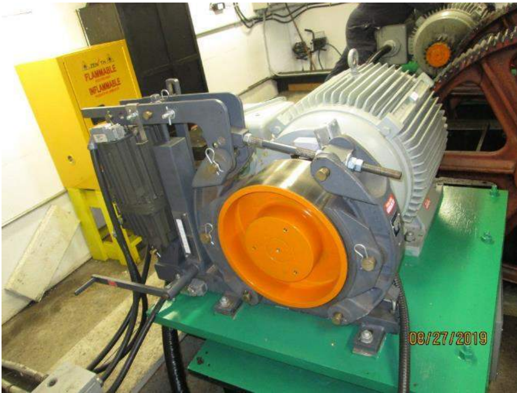
Photo E-11: Typical Motor Brake. The motor brakes are in as-new physical and operational condition and are provided with set, released, and hand released limit switches as per code.
