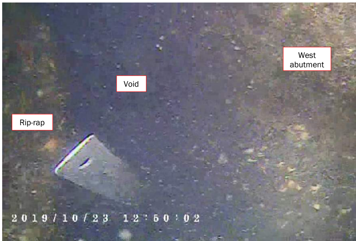
Photo S-85: Triangular void with an area of 1000mm by 800mm and depth of 300mm at the sheet pile/rip-rap interface at the south side of the west abutment of the Bascule Bridge.
