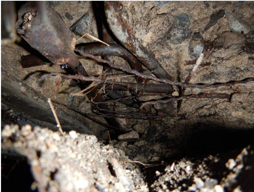
Photo S-68: Exposed, corroded rebar in the soffit of the counterweight at the southeast (photo taken after removal of the bottom east angle).
