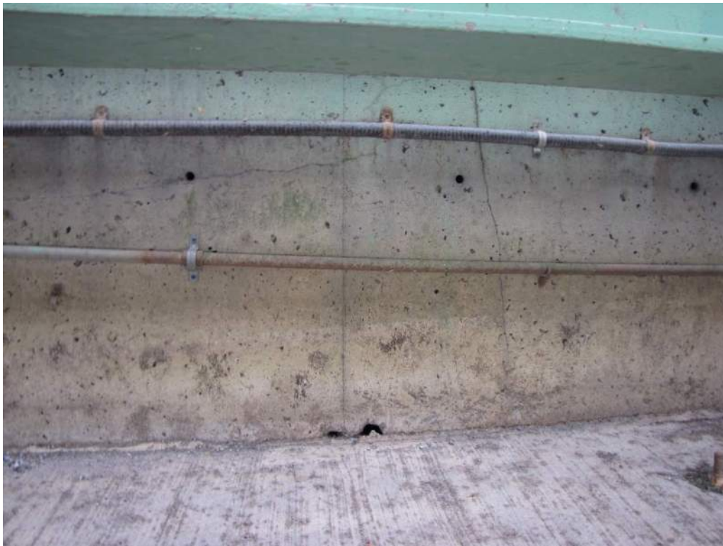
Photo S-104: Wide diagonal and vertical crack in the east ballast wall. Also note the 2 holes at the bottom of the wall, each with an area of 100 mm 2 .
