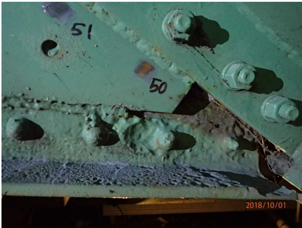
Photo S-48: Very severe section loss in the rivet heads and angle at the base of the exterior face of the south plate of the north trunnion (photo from 2018 CDI).
