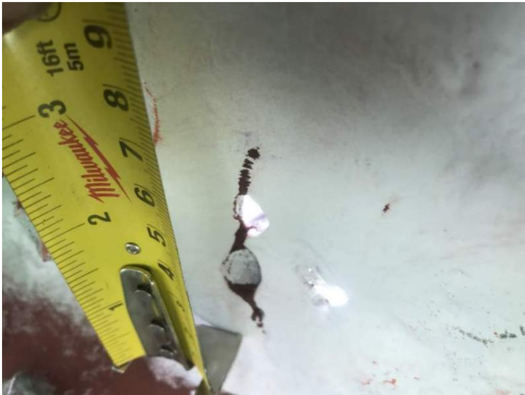
Photo S-38: Fatigue crack propagating from three perforations with a total length of 70mm in the south channel of tower truss member 18S-19S.
