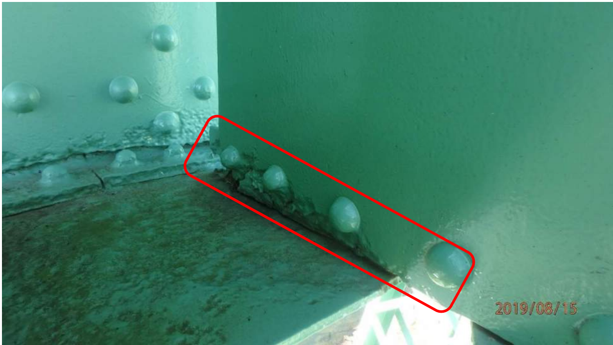
Photo S-92: Bottom west angle of counterweight truss lateral strut member 23N-23S has active corrosion and perforations at last 3 rivets at node 23S.
