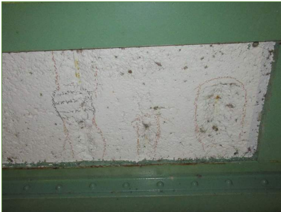
Photo P4 Machinery Room Slab Soffit Deterioration (delaminations)
