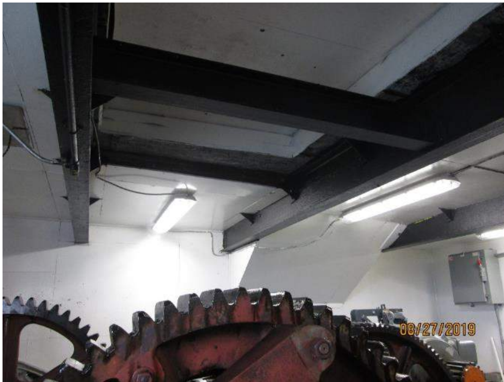
Photo E-37: Machinery Space Lighting. The machinery space is provided with T5 light fixtures. These fixtures are in excellent operational condition and provide adequate lighting levels for maintenance and troubleshooting.
