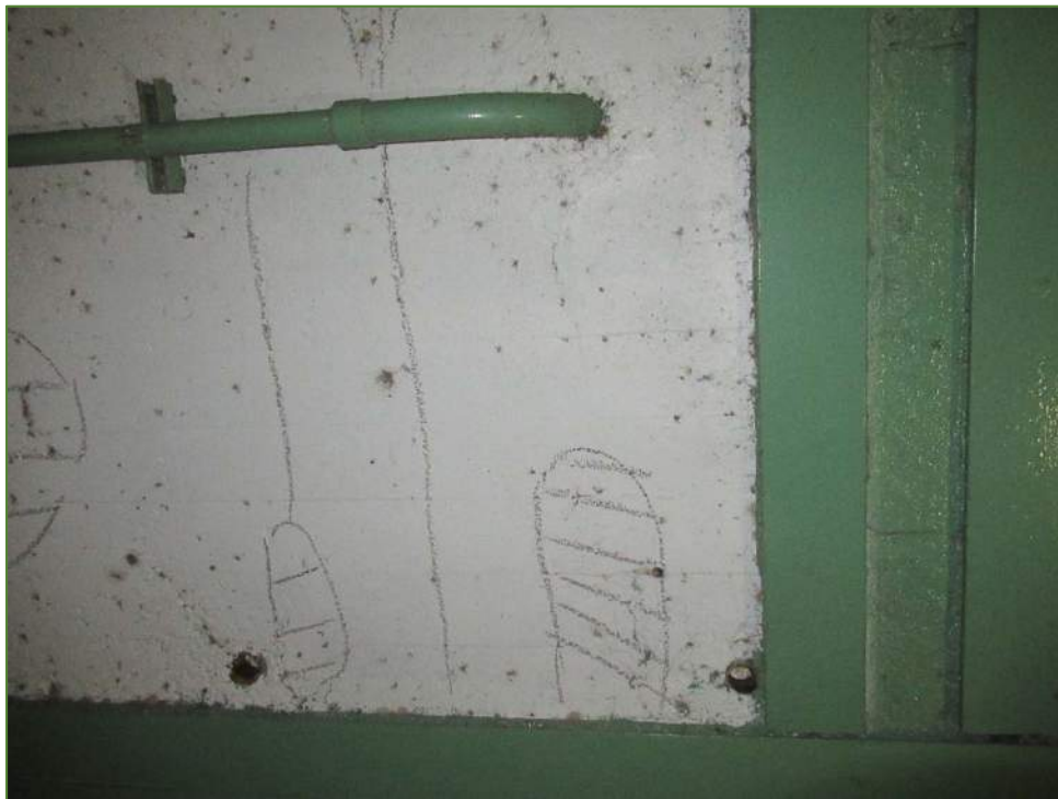
Photo P8 Machinery Room Slab Soffit Deterioration (cracks, delamination and honeycombing)
