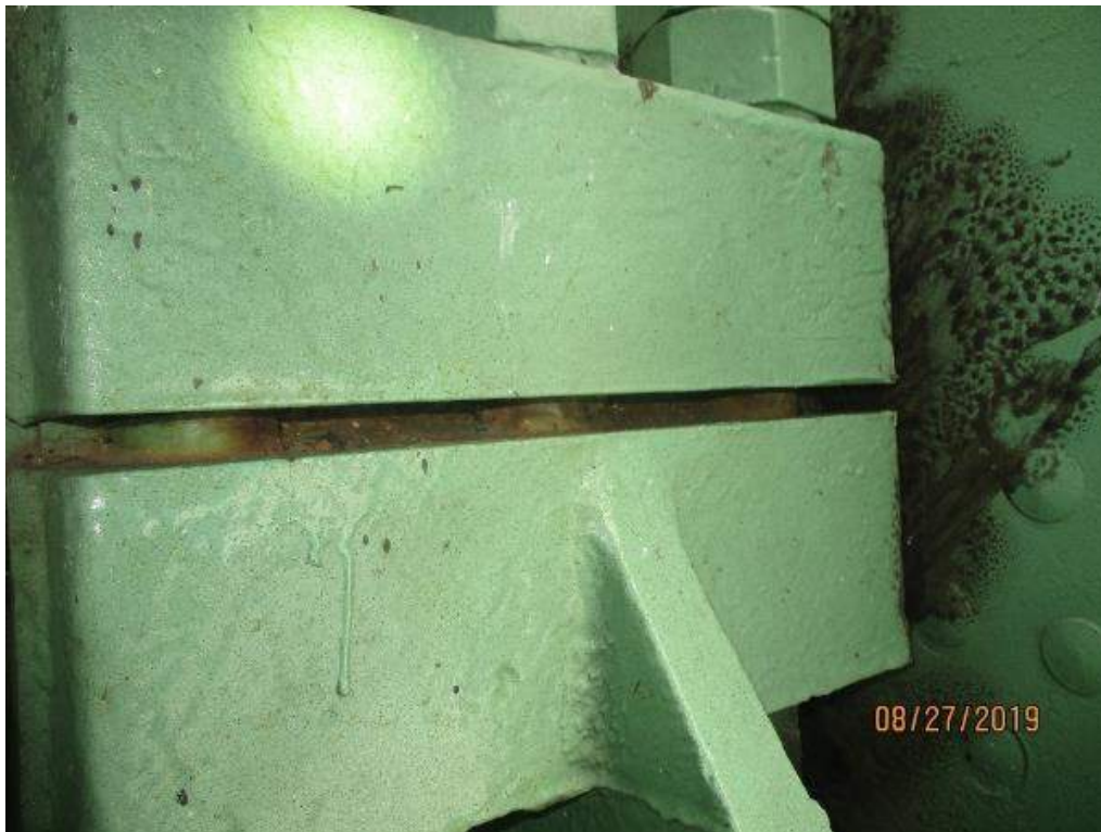
Photo M-1: Span Drive Machinery B1-N Bearing. There is light paint deterioration and corrosion between the bearing cap and base at the upper split line. The B1-S Bearing is similar.
