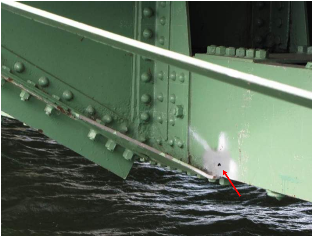
Photo S-18: Severe pitting, section loss, and peeling coating in the sidewalk floor beam connection and in bottom chord member OS-2S at node 2S. A perforation in the web of member OS-2S is also present.
