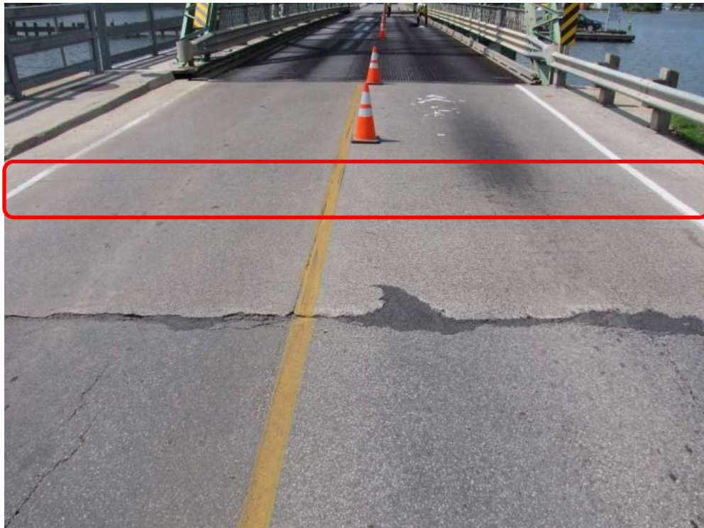
Photo S-109: There are two wide cracks that extend across the full width of the east approach slab. Also note the worn painted combination traffic/bicycle lane symbol.
