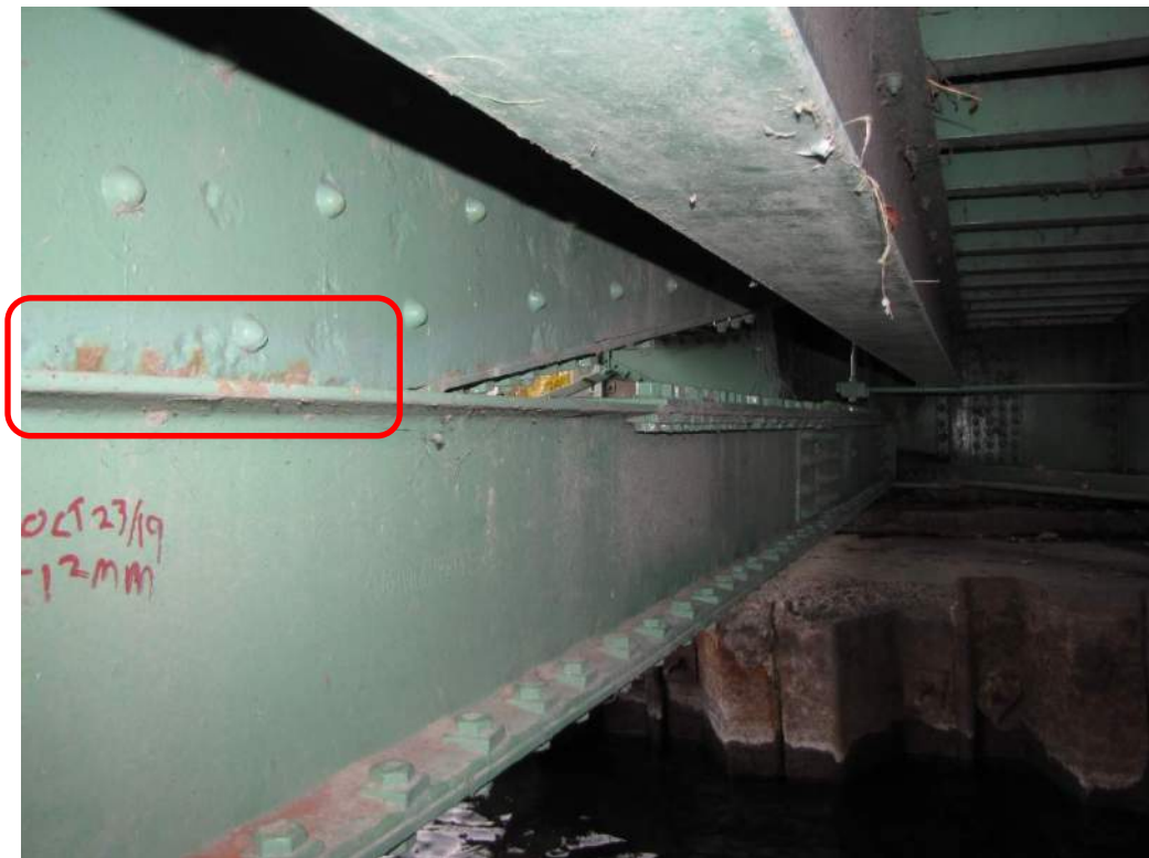
Photo S-17: Severe pitting and rust jacking between member 14N-15N and 14N-16N.
