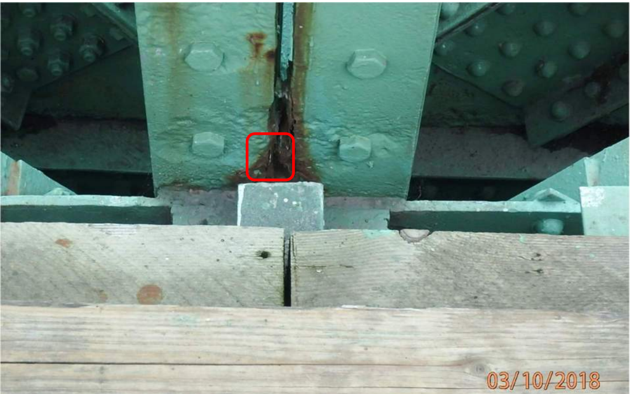
Photo S-27: Very severe pitting with a small perforation in the south angles of vertical member 9N-10N above node 10 (photo from 2018 CDI).
