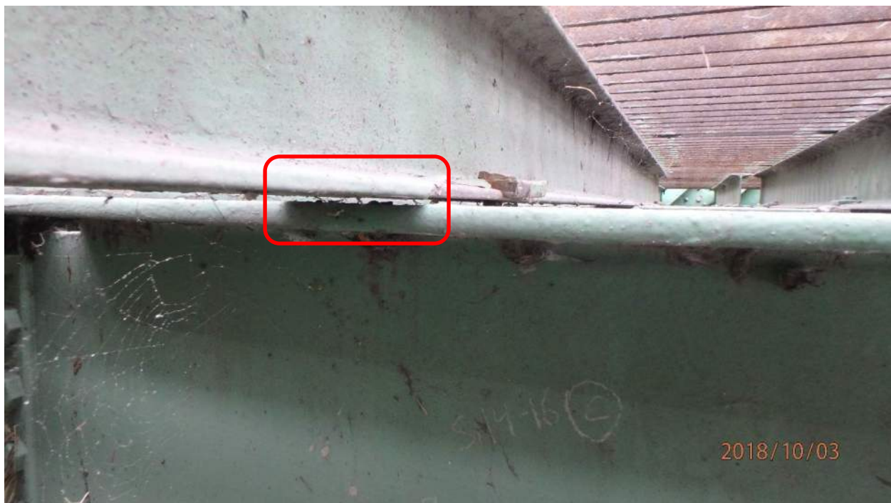
Photo S-63: Multiple sills in bay 14-16 are not bearing on the stringers below (photo from 2018 CDI).
