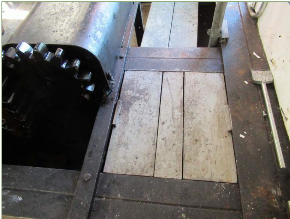
Photo P16 Machinery Room Slab (topside) note light corrosion on steel components
