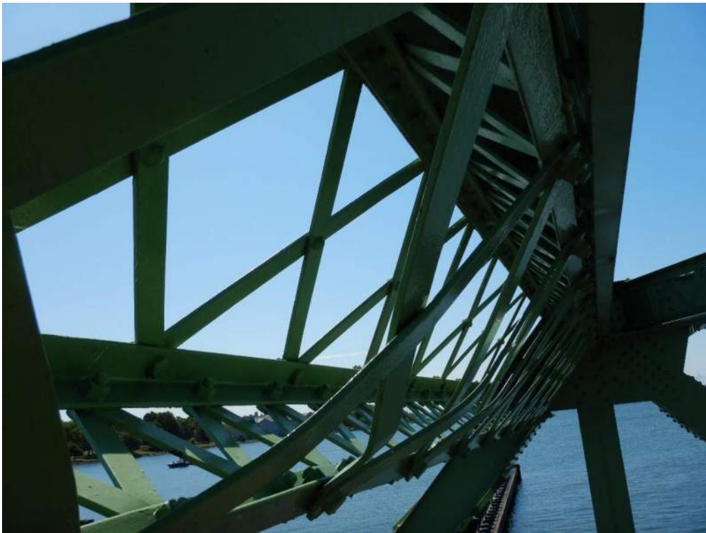
Photo S-86: Six lattices in portal truss member 1S-1N are bent, likely due to vehicular impact of the bottom angle.
