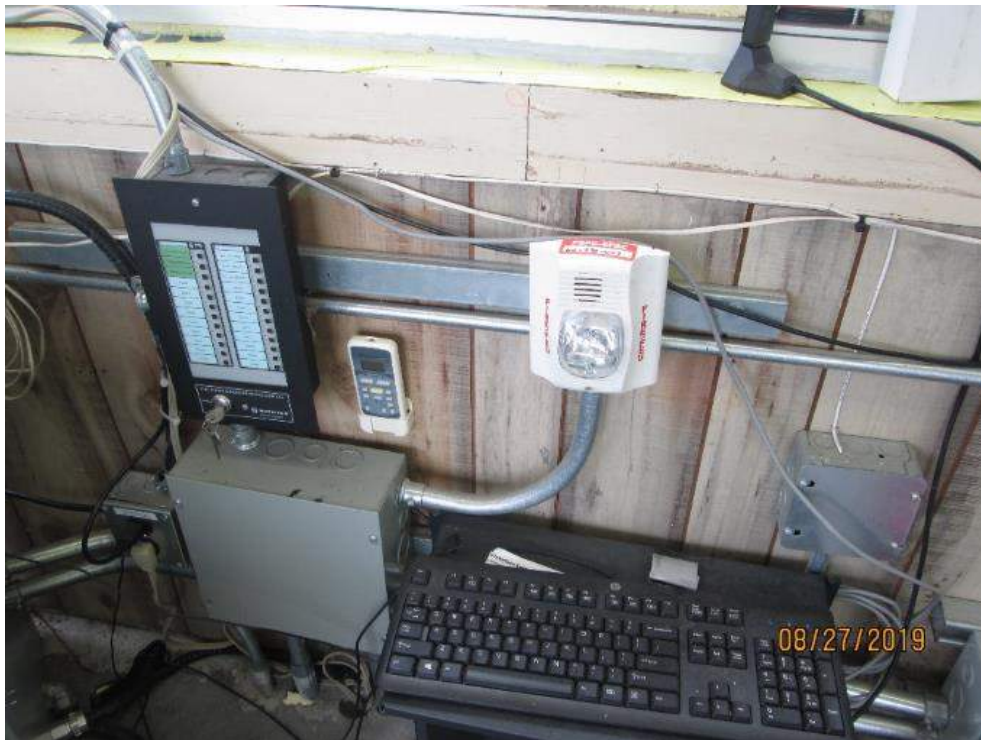
Photo E-35: Fire Alarm System. The bridge is equipped with a fire alarm system. Fire detection devices are provided in the bridge maintenance building, the bridge control house and machinery space. The main fire alarm control panel is located in the bridge maintenance facility with a remote annunciator located in the bridge operators control house. All fire alarm equipment was in good serviceable condition at the time of the inspection.
