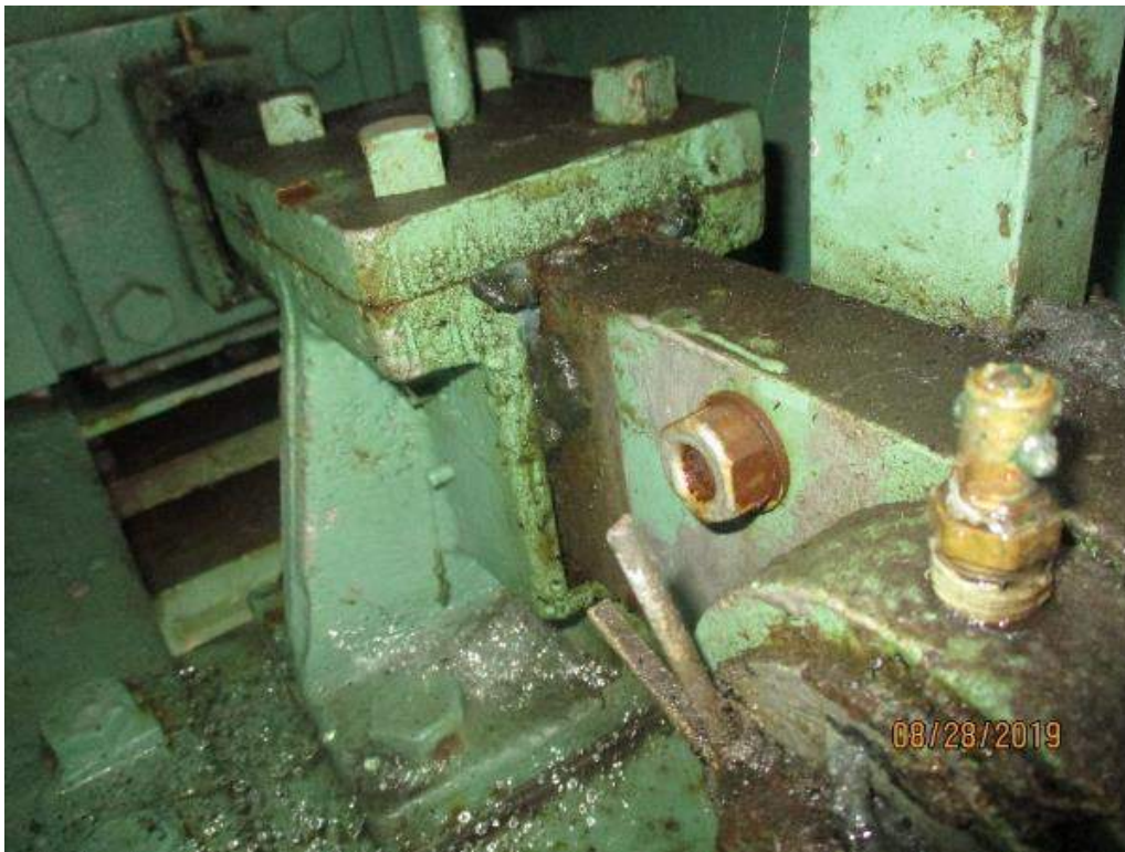
Photo M-23: South Span Lock Crank Shaft CR2. The mounting bolts and nuts for the rotary cam position crank CR2 located on the lock bar are not fully painted and exhibit light corrosion. North Span Lock Crank Shaft CR2 is similar.
