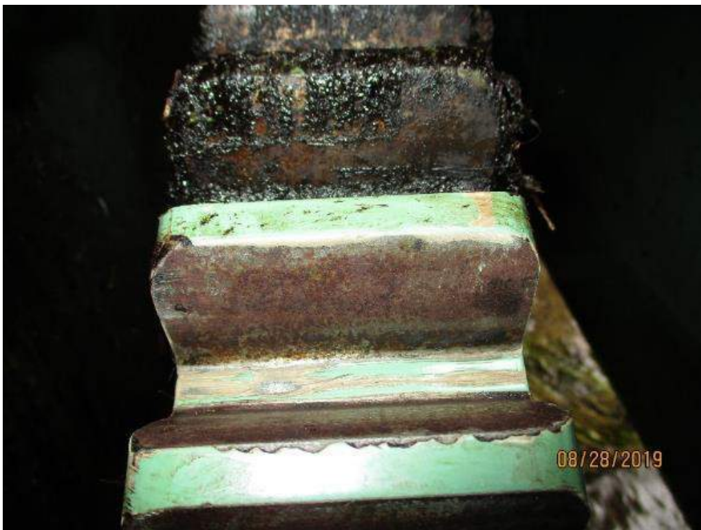
Photo M-20: Span Lock Gear T. The faces of the pinion teeth are corroded. This is likely from previous lack of lubrication, as the gears were well lubricated at the time of the inspection. The teeth of pinion W, gear V, and gear T are similar.
