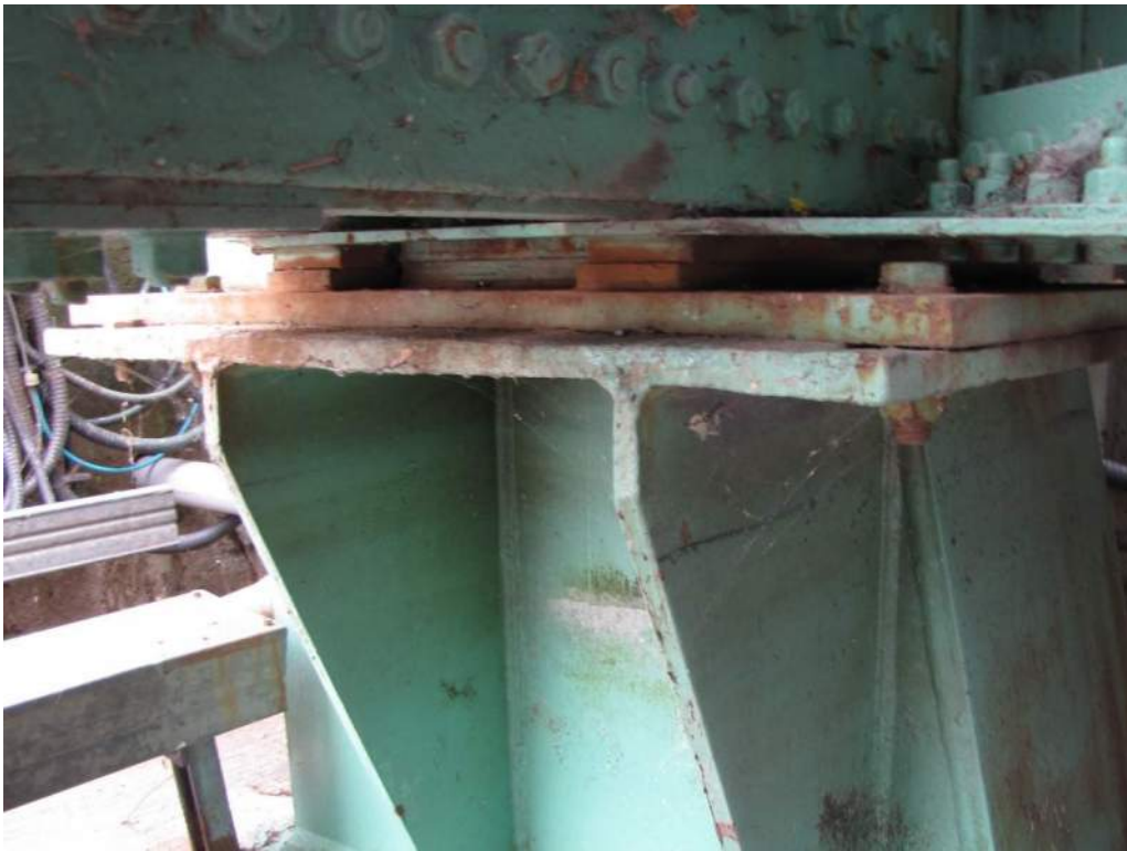
Photo S-108: The leaf span is not fully seated on the north live load support and only seats fully when vehicles are on the east end of the deck. Note the light corrosion occurring on the bearing plate.
