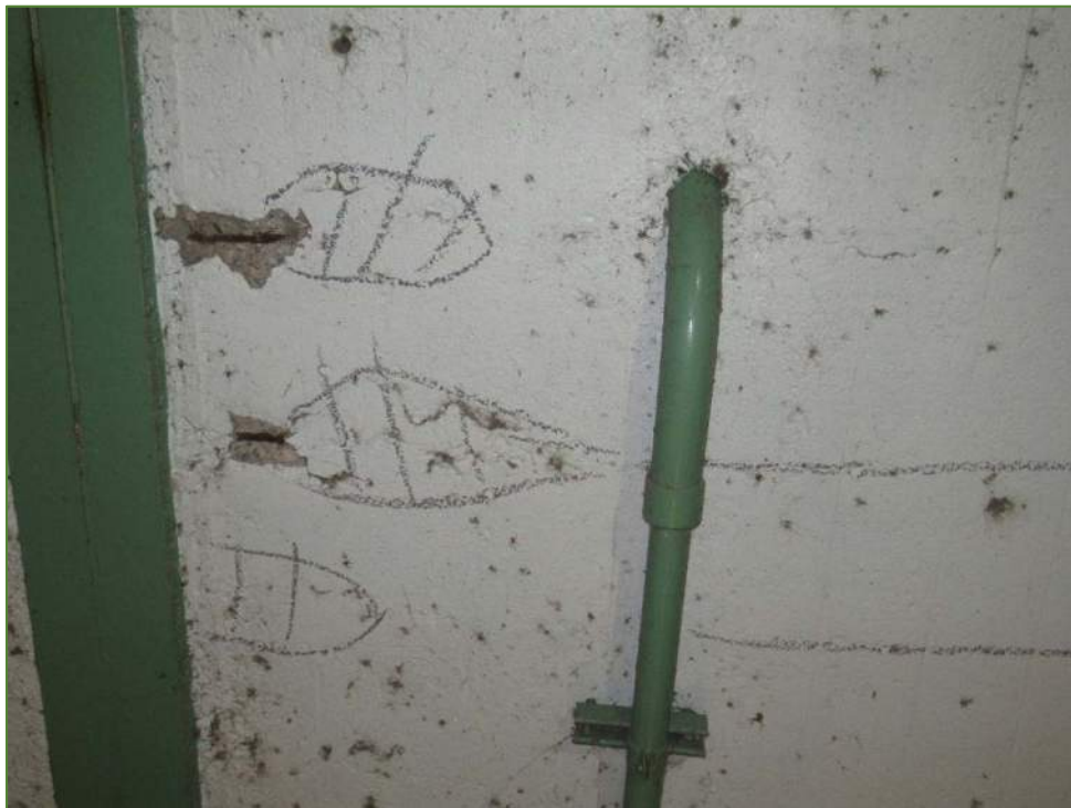
Photo P6 Machinery Room Slab Soffit Deterioration (cracks, spalls and delaminations) note exposed corroded rebar
