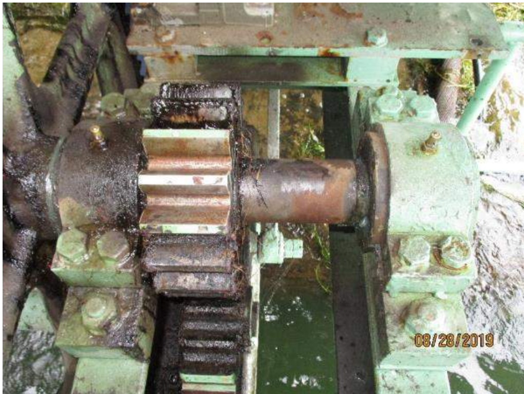
Photo M-19: Span Lock Shaft. The span lock drive shaft between bearings B3 and B4 is not painted. Note the corrosion.
