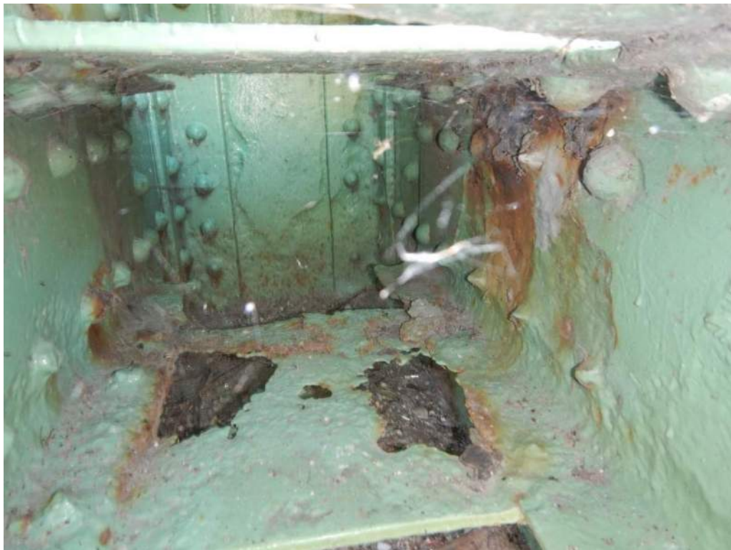
Photo S-35: Tower truss horizontal member 18N-19N has severe section loss of interior angles and rivet heads plus a perforated lower batten plate at node 19N.
