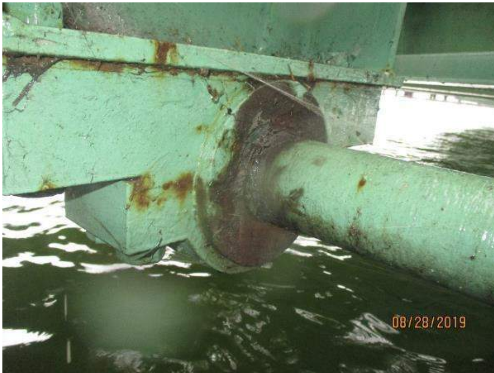
Photo M-21: Span Lock Cross Shaft Bearing B1-S. The housing for the bearing exhibits paint deterioration and light corrosion. All of the span lock cross shaft bearings are similar.
