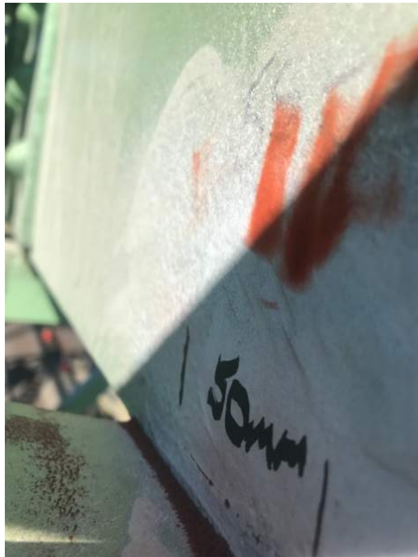
Figure 2: Crack Extended 50mm on Other Side
