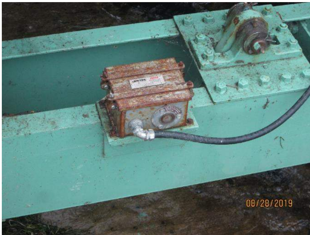
Photo E-17: North Side Span Lock Rotary Cam Switch. The span lock is provided with a second RCLS to monitor the position of the north lock bar. The RCLS enclosure exhibit moderate signs of corrosion.
