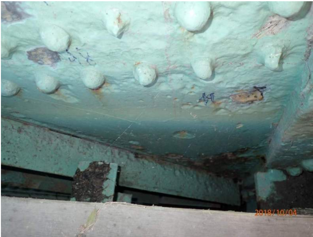
Photo S-52: The north (roadway) side of the south trunnion has widespread pitting in the collar plate (not shown), connecting plate, and some rivet heads (photo from 2018 CDI).
