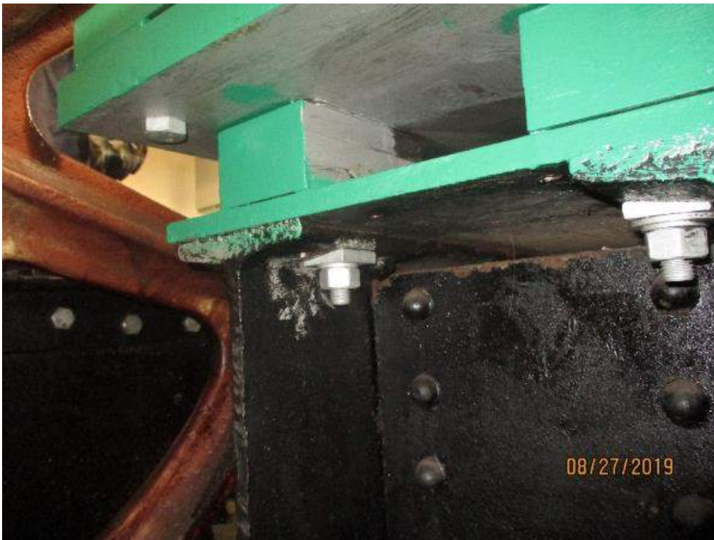
Photo M-3: Span Drive Machinery North Motor. The underside of the motor mounting plate is unpainted. The span drive south motor is similar.
