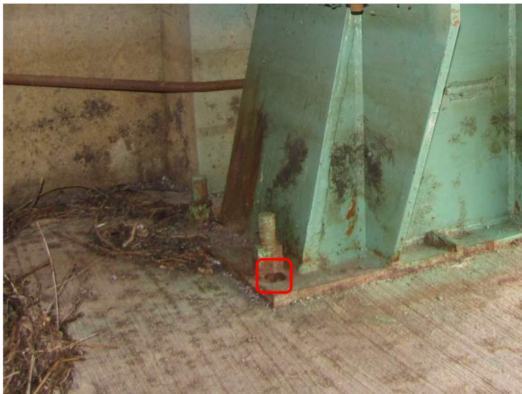
Photo S-107: The northwest anchor bolt of the southeast live load support is bent and exhibits medium to severe corrosion.
