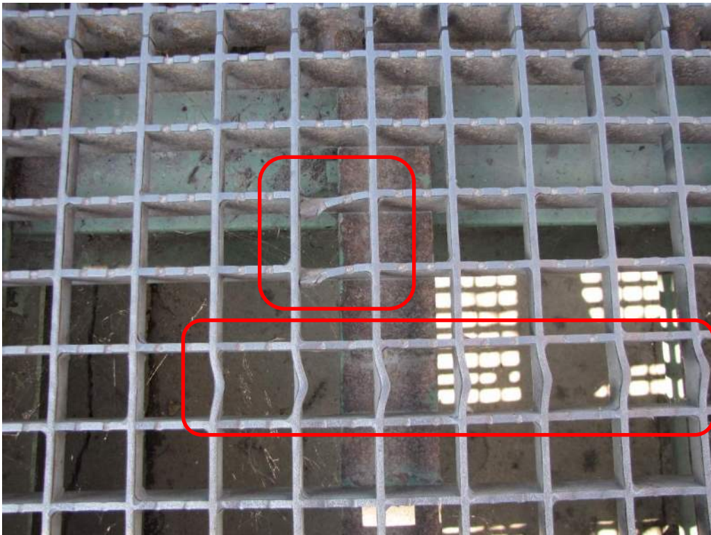
Photo S-76: Cracked bearing (top) and bent cross (bottom) bars in deck grating panel 15-16 B.
