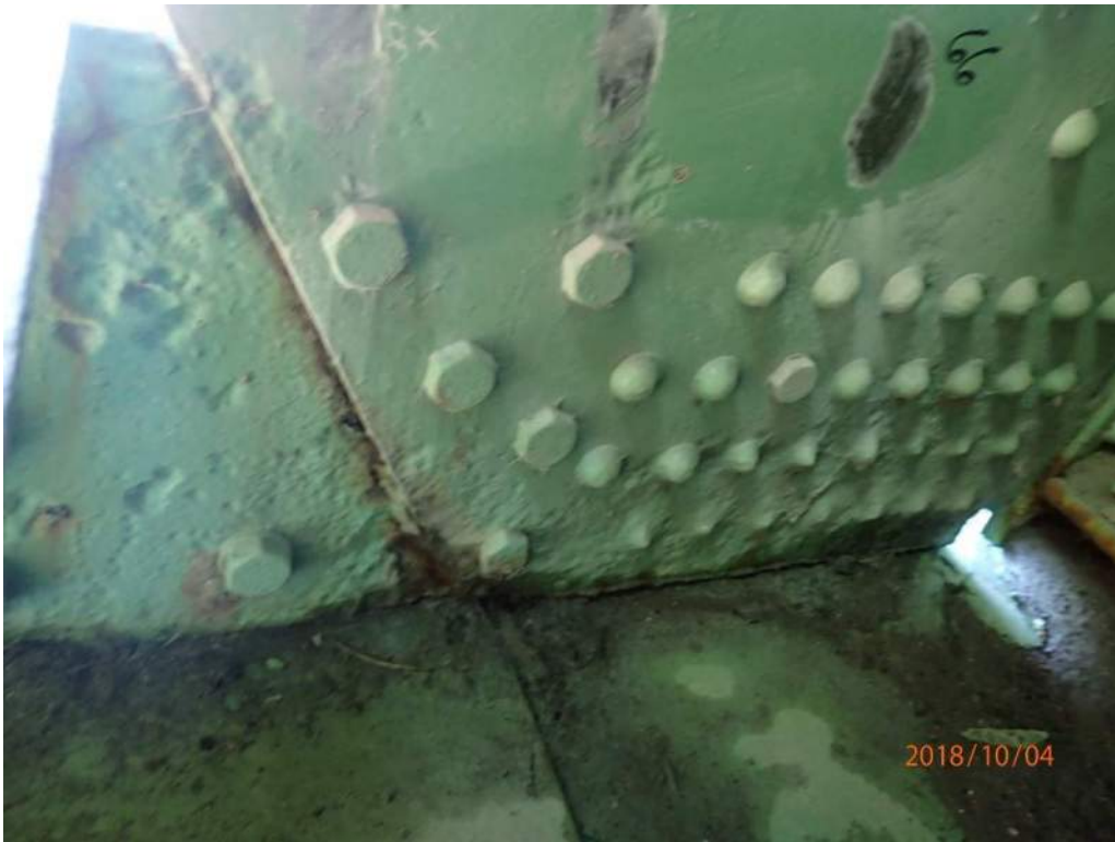
Photo S-50: Severe pitting at the base of the interior face and rivet heads of the south plate of the south trunnion (photo from 2018 CDI).
