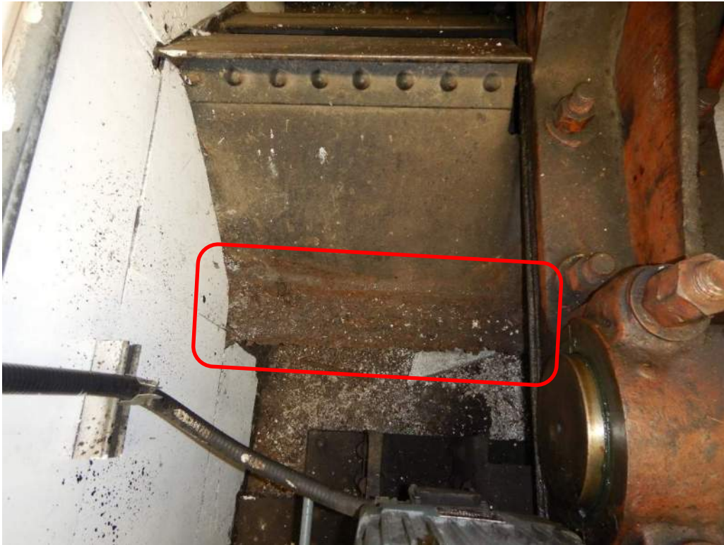
Photo S-44: Severe corrosion on the bottom flange of the northeast transverse strut in the mechanical room.
