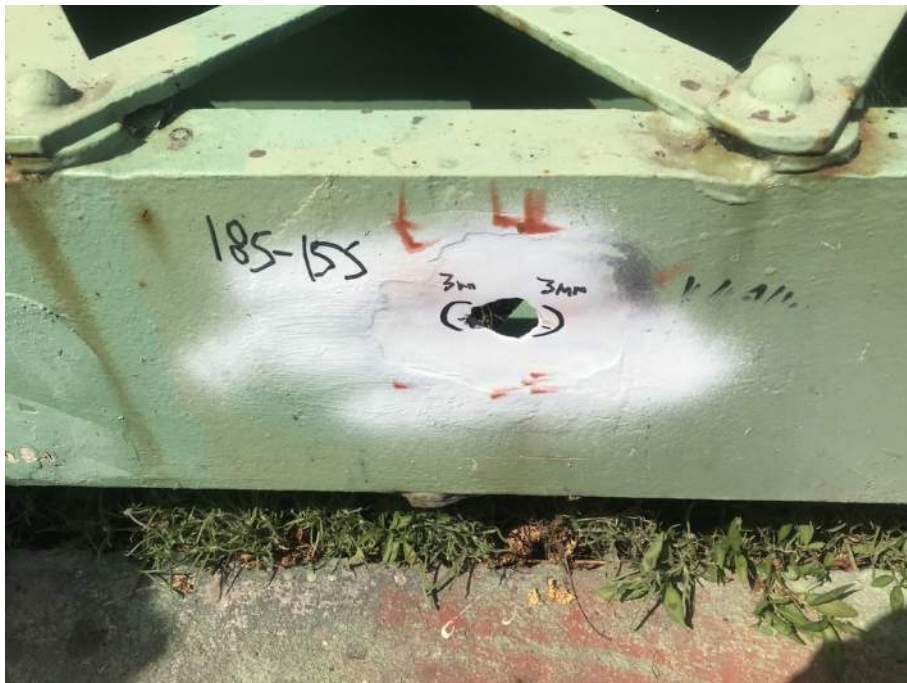
Figure 12: 3mm Cracks Forming on Both Sides
