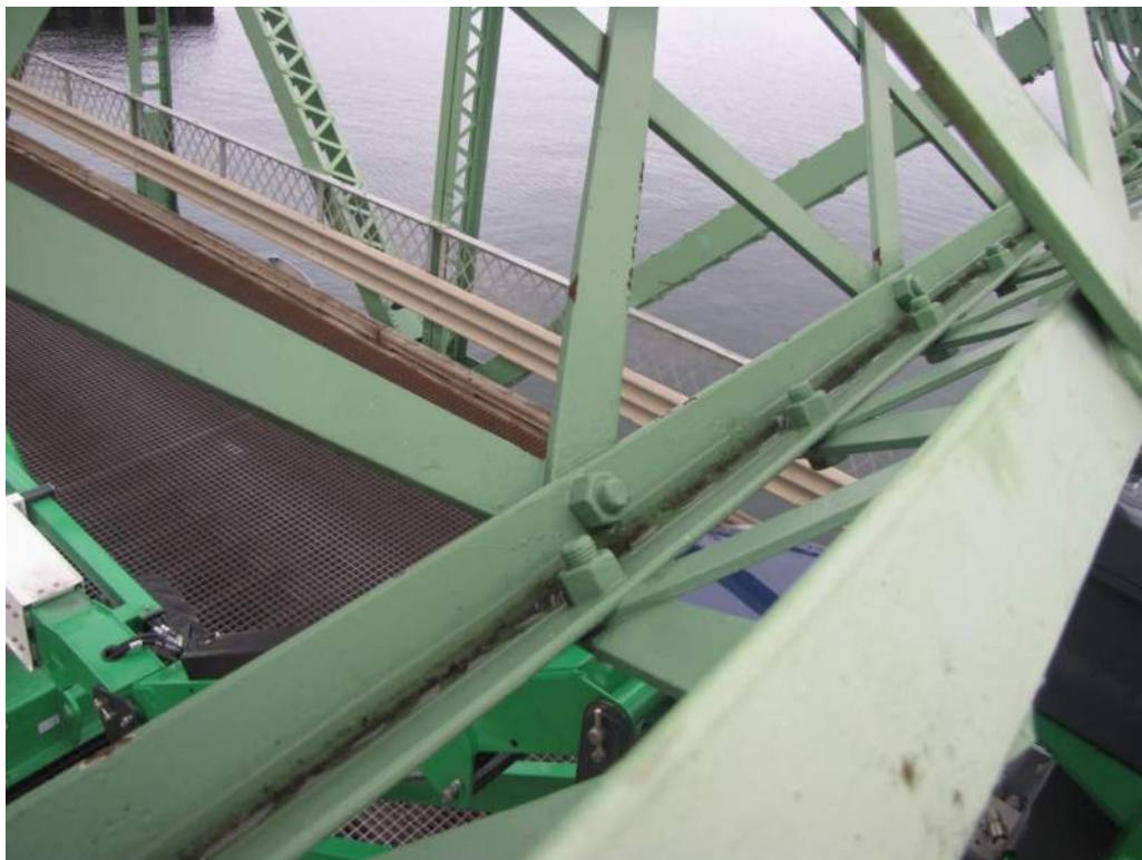
Photo S-87: The lower angle of portal truss member 1S-1N is holding water (photo from 2018 CDI).
