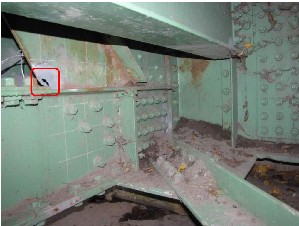
Photo S-49: View of the north side of the south trunnion below deck level. A 3mm crack was found at the indicated perforation.
