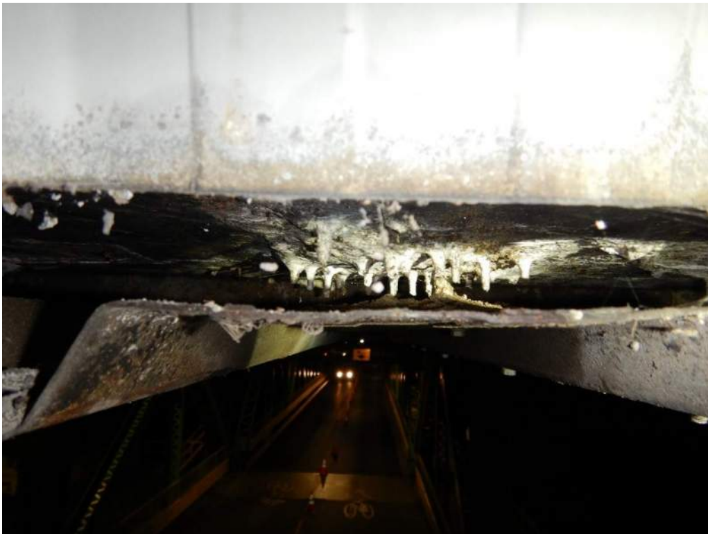
Photo S-67: Efflorescence deposits and staining on the underside of the counterweight concrete (photo taken after removal of the bottom east angle).
