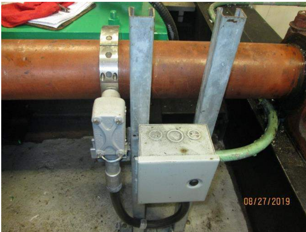
Photo E-22: Speed Switch Sensor. A Hall Effect speed switch was installed as part of a 2012 rehabilitation project to provide span position and motor speed indication on the operator's control desk. The speed switch sensor is in very good condition.
