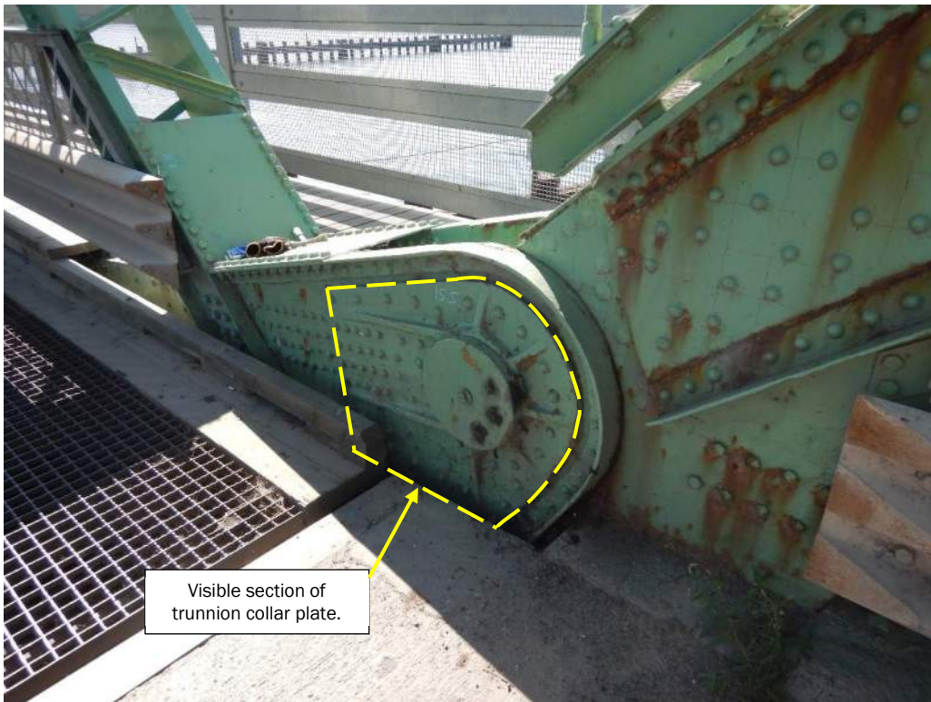
Photo S-83: The north (roadway) side of the south trunnion. Note that there is no railing between the pedestrian sidewalk and roadway.
