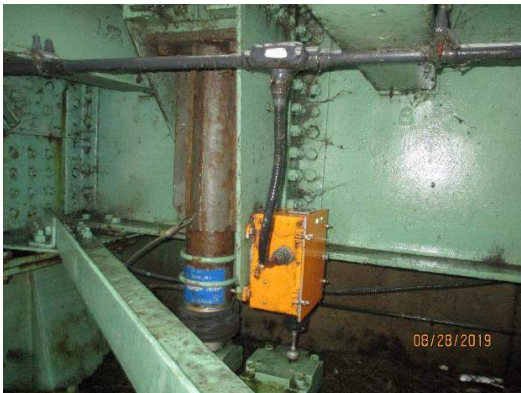
Photo M-28: North Buffer. General View of the buffer, strike plate and seated limit switch. Note the buffer is corroded. The south buffer is similar.
