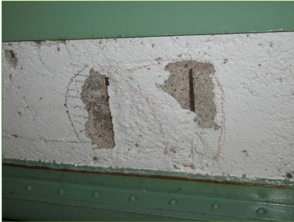
Photo P3 Machinery Room Slab Soffit Deterioration (cracks, spall and delamination) note exposed corroded rebar
