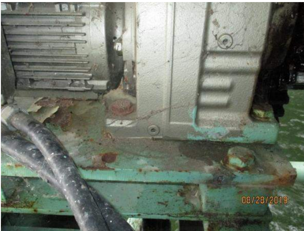
Photo M-16: Span Lock Gearmotor. The mounting bolts and support for the gearmotor are not fully painted. Note the corrosion.
