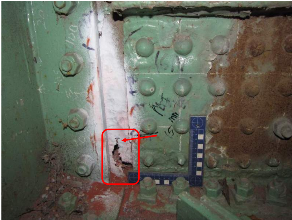
Photo S-45: The interior vertical gusset plate at node 16N exhibits severe section loss and a perforation with a 15mm vertical crack.
