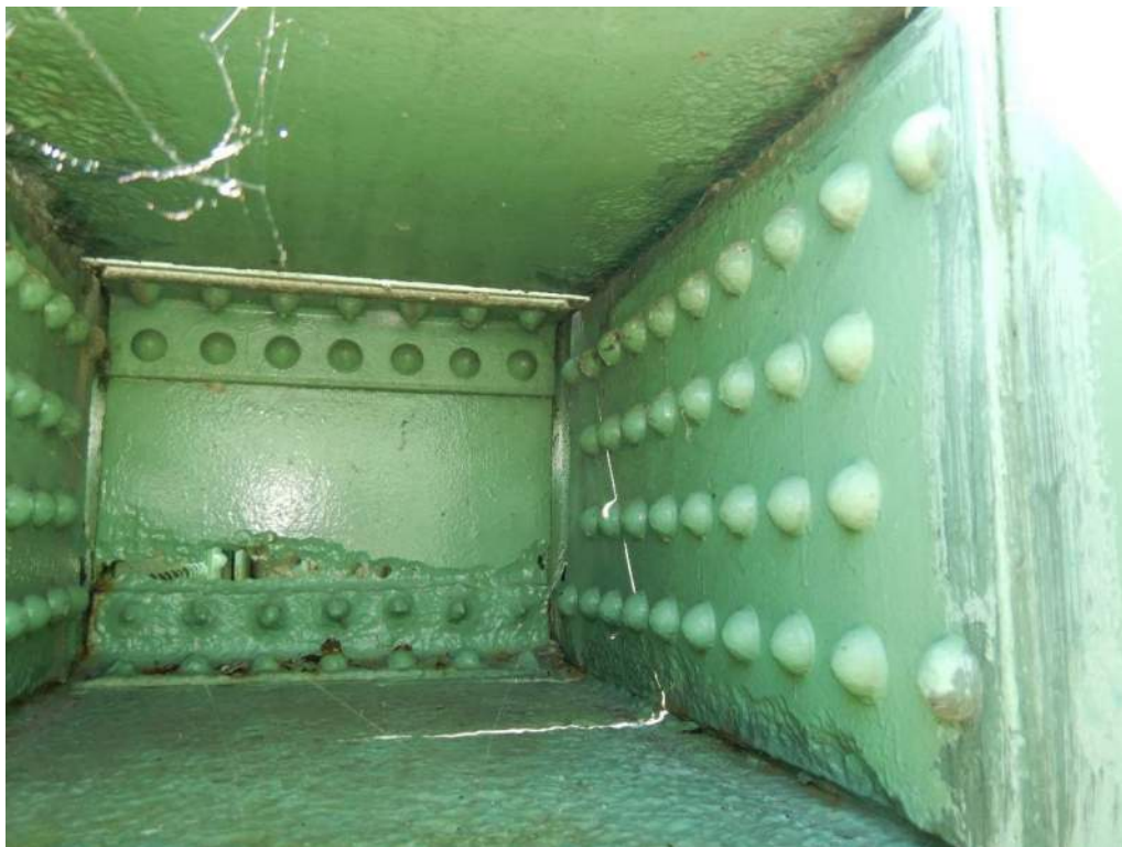
Photo S-15: Perforation and severe pitting of diaphragm inside top chord member 11S-13S near node 13S.
