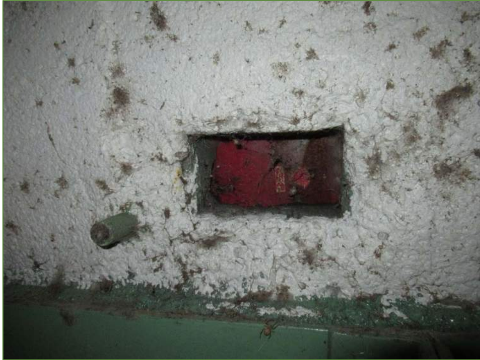
Photo P11 Machinery Room Slab Soffit Deterioration (medium scaling)
