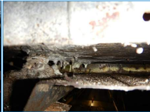
Photo 2 Soffit - Efflorescence, Stalactites, Stalagmites, Typ.
