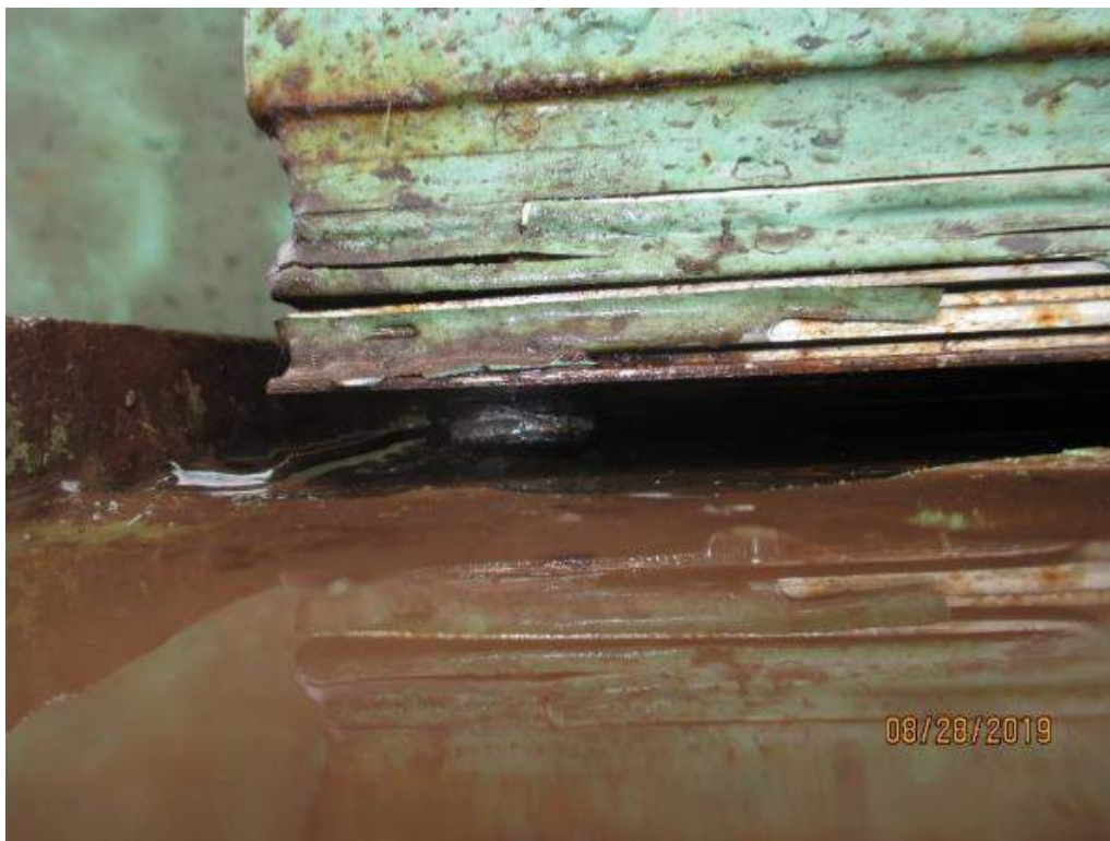
Photo M-26: South Span Lock Receiver. Close-up view of the gap between the support and shims at the northwest corner.
