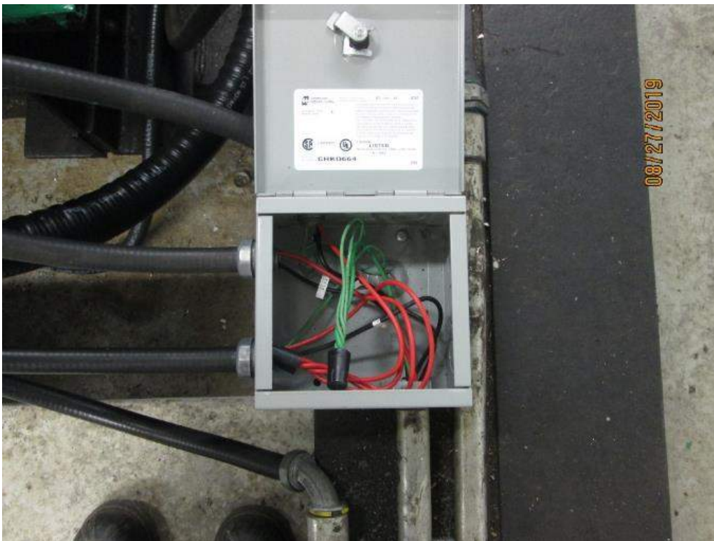
Photo E-12: Junction box near motor brake #1. Note the use of wire-nuts inside the junction box.
