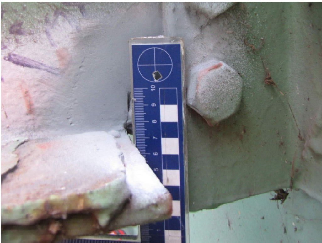
Photo S-57: 15mm notch/crack in the bottom cope of Stringer E (FB0-FB2) at FB0.
