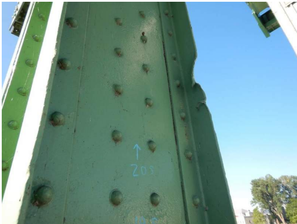
Photo S-39: Impact damage to southeast and southwest flanges above road level on tower truss vertical member 19S-20S.
