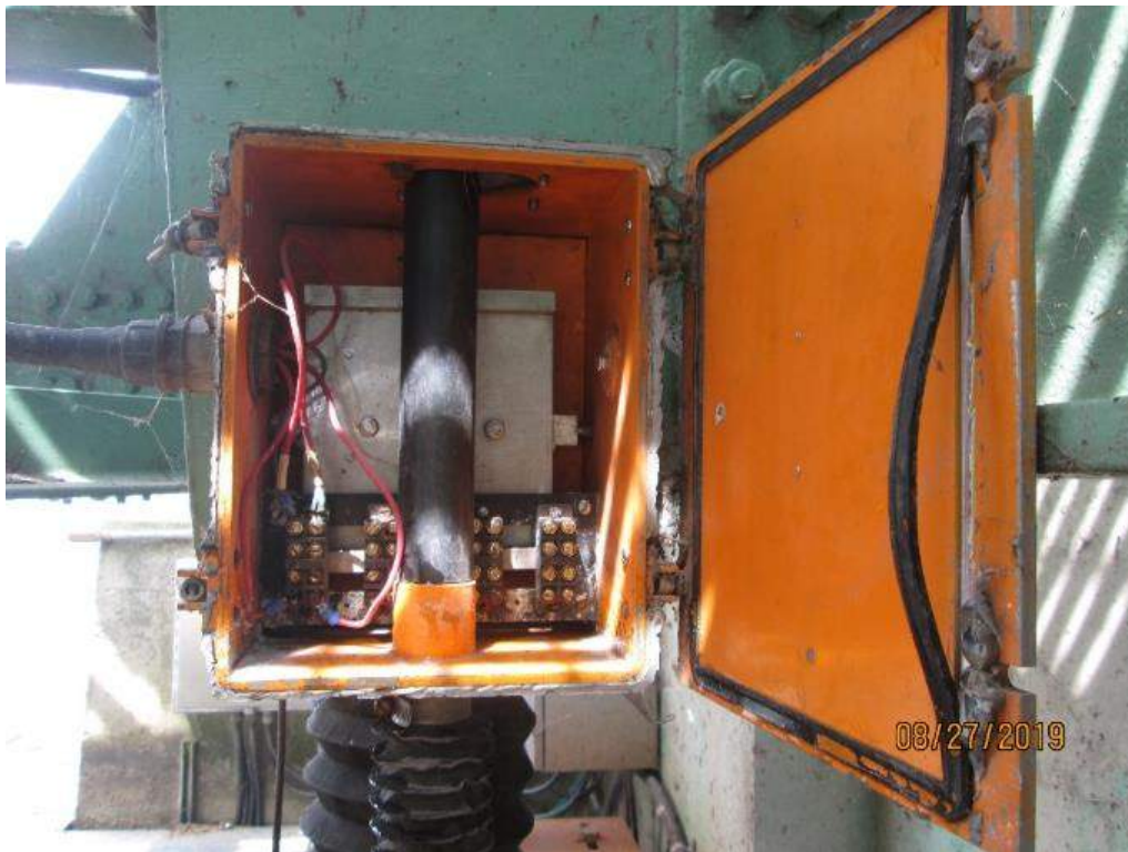
Photo E-21: Span Fully Seated Limit Switch. Two span seated limit switches are provided at the toe end of the span, one at each corner. North seated limit switch exhibits standing water inside the enclosure. Note during high water level, water will get inside the switch enclosure and cause operational issues.
