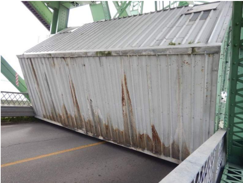
Photo S-65: The panels on the underside of the counterweight have widespread corrosion and wet areas/stains (photo taken when bridge in open position).
