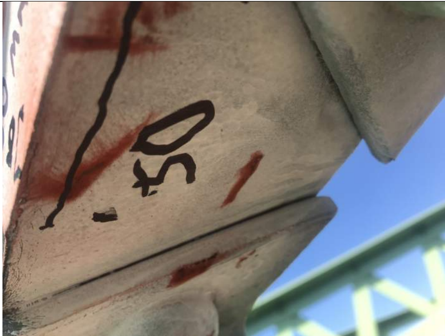
Figure 3: 50mm Crack Located on the Bottom
