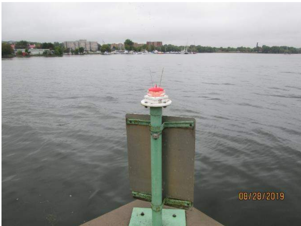
Photo E-30: Typical Fender Light. The bridge is provided with 4 fender light fixtures, one at each corner of the fender. The north fender lights are flash red and the south fender lights are flash green. The fender lights are of LED type and are in good operational condition.
