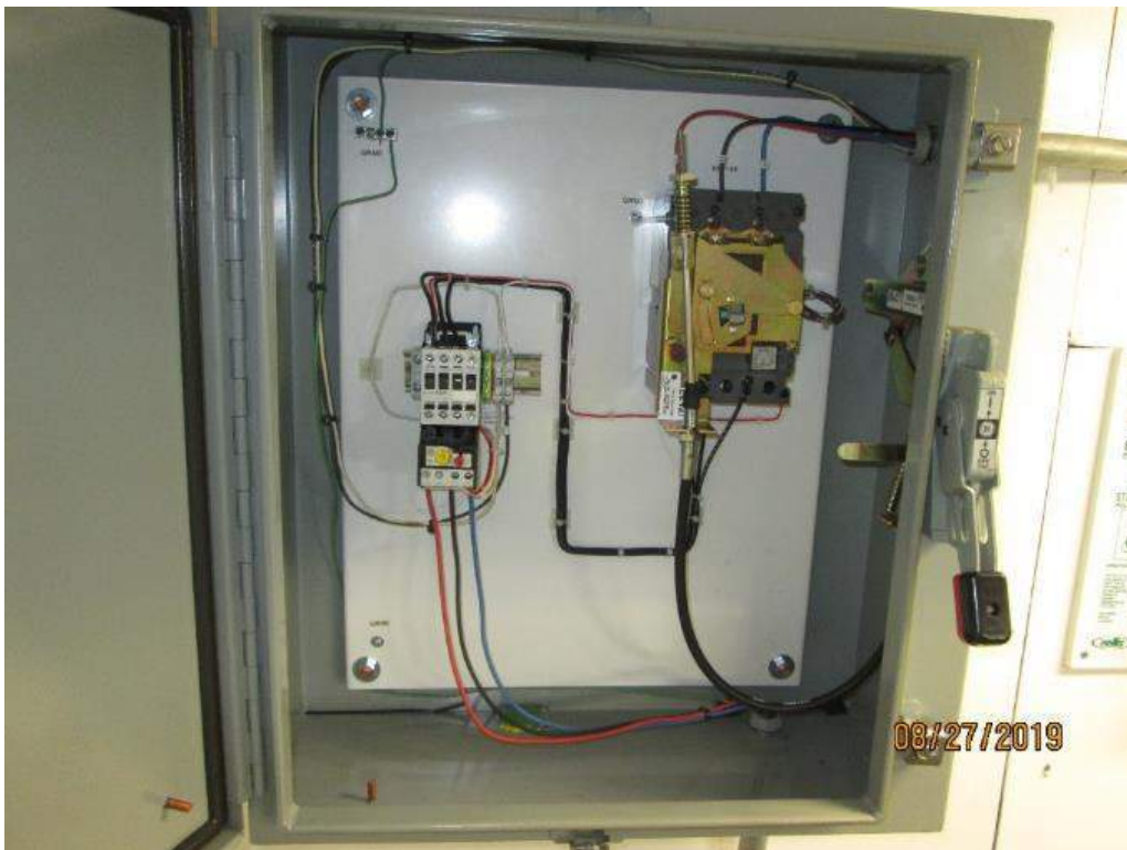
Photo E-14: Motor Brake Disconnect and Starter enclosures. New motor brake starters were recently installed in the bridge machinery space and are in excellent condition. The MCP of the motor brake starter also serves as the local disconnect switch. The wires in the enclosure have not been labelled to aid troubleshooting.
