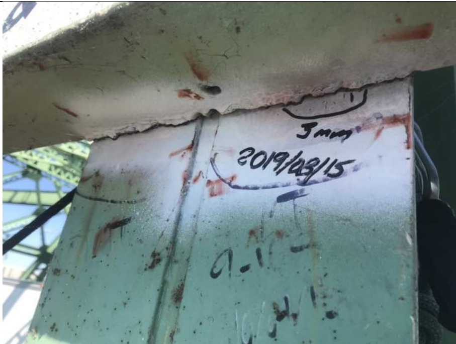
Figure 7: 3mm Crack no Change from Previous Inspection
