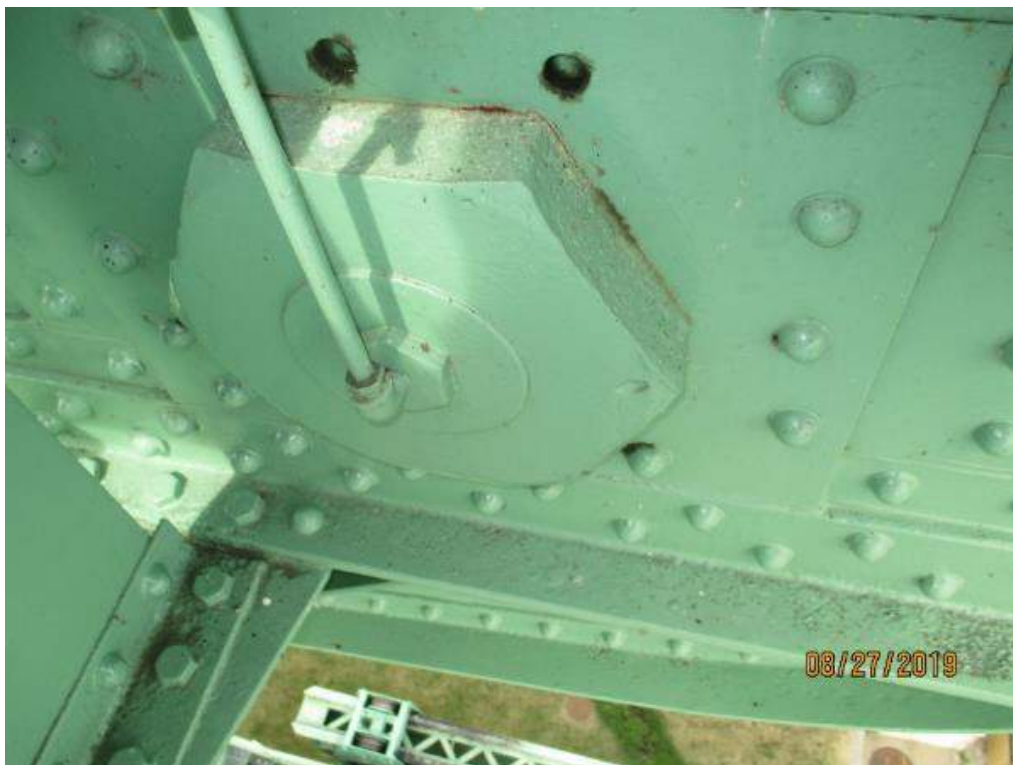
Photo M-14: North First Link Pin. There is cracked paint and fretting between the nut and the structure indicating slight movement.
