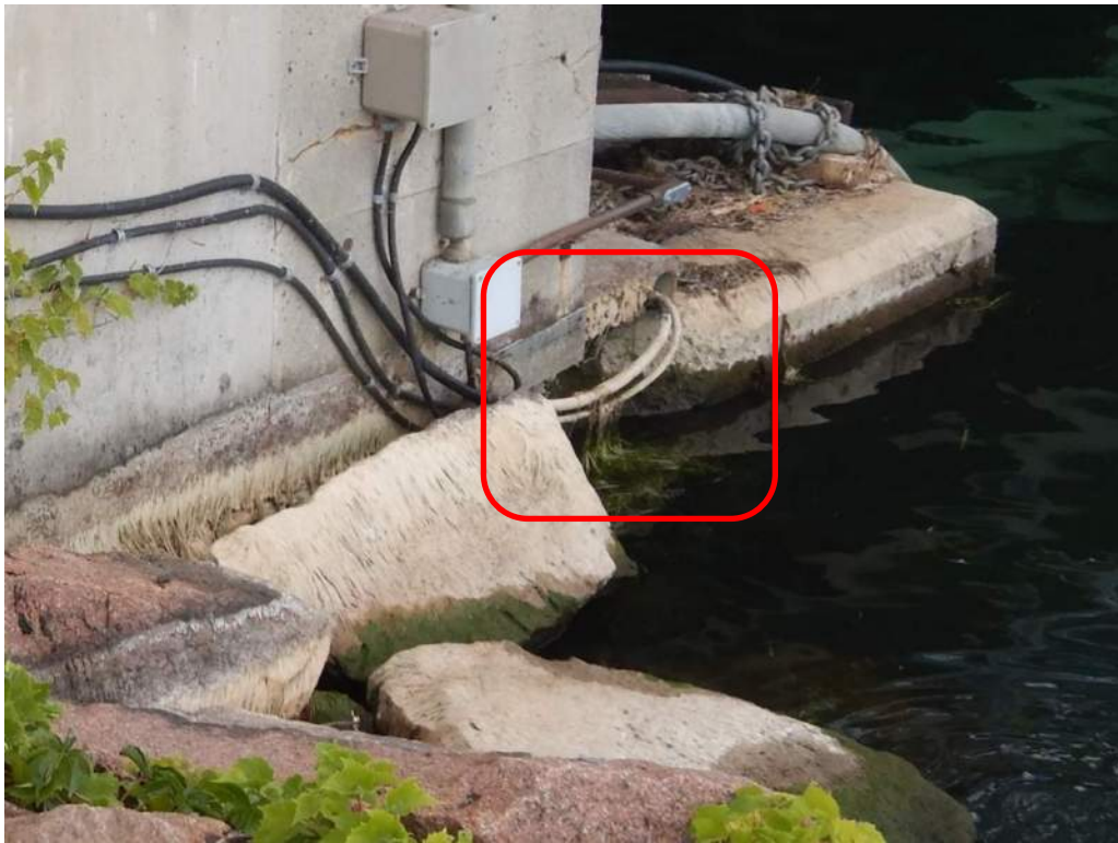
Photo S-106: Very severe spall at the base of the southwest wingwall at the interface with the abutment. Note that about half of the spall is below the water level at the time of the inspection. Also note the vegetation growth occurring below the high-water level.
