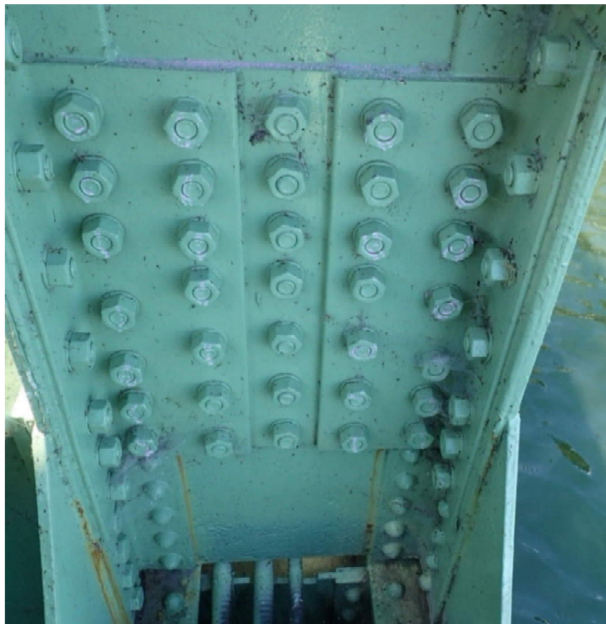
Photo S-29: Bolts used in repaired section on vertical member 13N-14N are too short.
