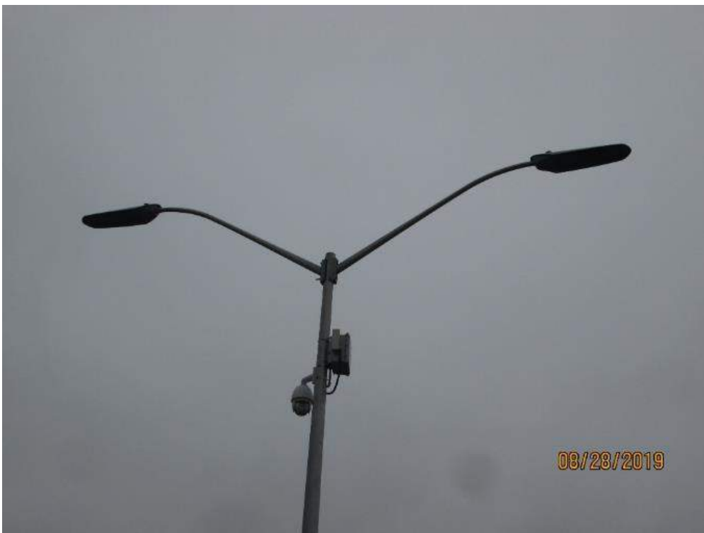
Photo E-38: CCTV System and Roadway Lighting. A CCTV system was installed at the bridge for monitoring of the bridge roadway, waterway and machinery space from the maintenance facility and the operators control house. The CCTV installation is in excellent condition. LED type roadway lighting are provided on the bridge and are photocell controlled.
