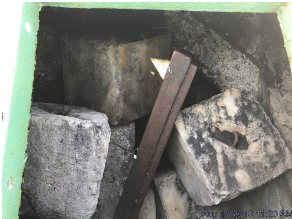
Photo S-69: The concrete in the two upper chambers in the top face of the counterweight exhibits spalls, disintegration, and wet areas (north chamber shown).
