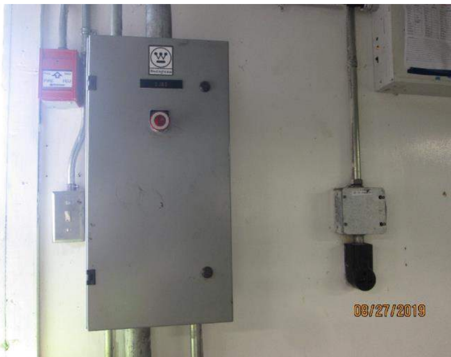
Photo E-20: Machinery Space Local E-Stop. This E-Stop switch is located near the machinery space entrance. It allows maintenance personnel to prevent or stop bridge operation when work is being performed in the machinery space.
