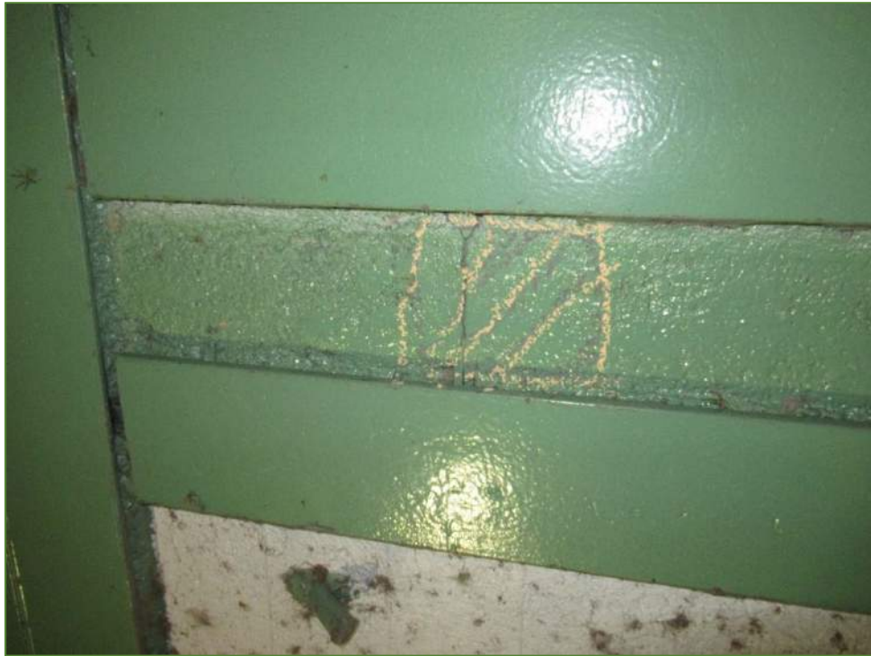
Photo P9 Machinery Room Slab Soffit Deterioration (cracks, delamination and light scaling)
