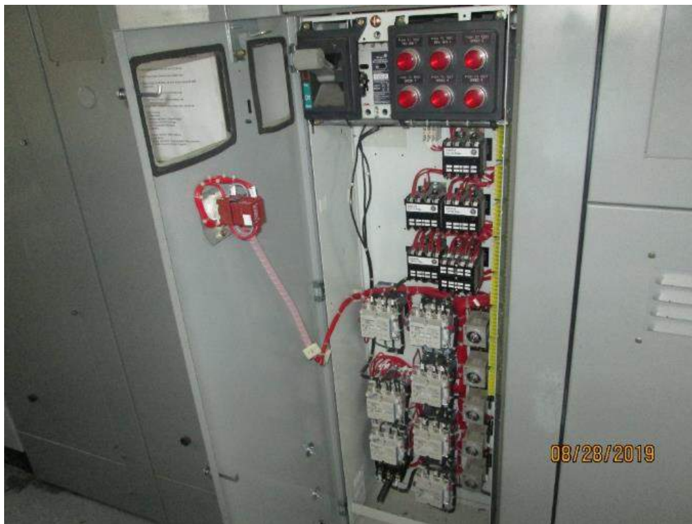
Photo E-15: Span Lock Starter Compartment. Note the span lock was originally designed with 6-speed operating steps. However, at the time of the inspection the span lock was operating at single speed only and the speed stepping contactor and resistor circuit had been disabled.
