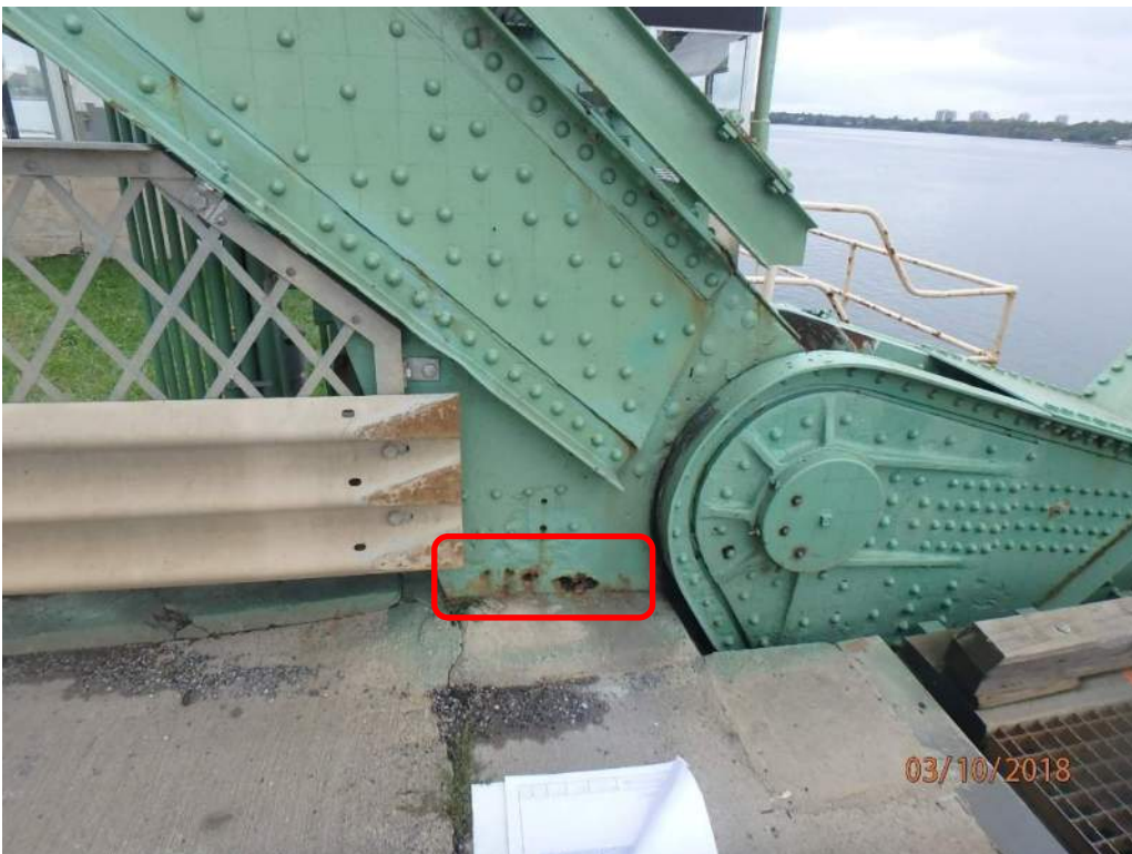
Photo S-55: The vertical gusset plate at node 15N at roadway level exhibits very severe section loss and perforations (photo from 2018 CDI).
