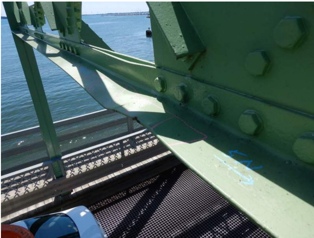
Photo S-88: Severe impact damage to the bottom east angle of through truss sway brace member 5S-5N.
