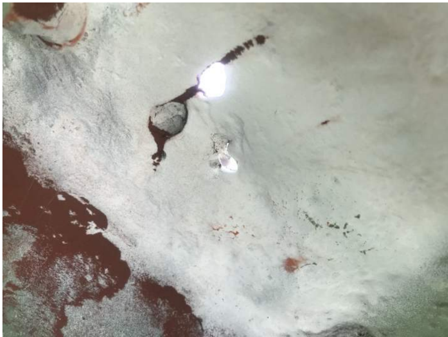
Figure 10: Crack Prorogating from Holes
