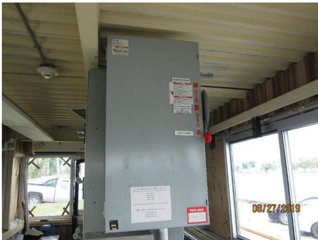
Photo E-4: Manual Transfer Switch (MTS). A manual transfer switch has been mounted on the side of MCC in the operators control house to allow the transfer of power between utility power and the generator power. This MTS is in excellent physical and operational condition.
