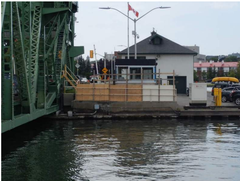
Photo S-101: Temporary timber hoarding in front of the Operator's House east railing.
