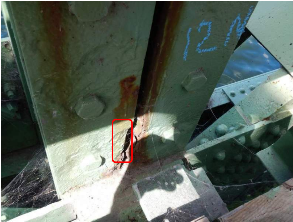
Photo S-28: Perforation in the south angles of vertical member 11N-12N above node 12N.
