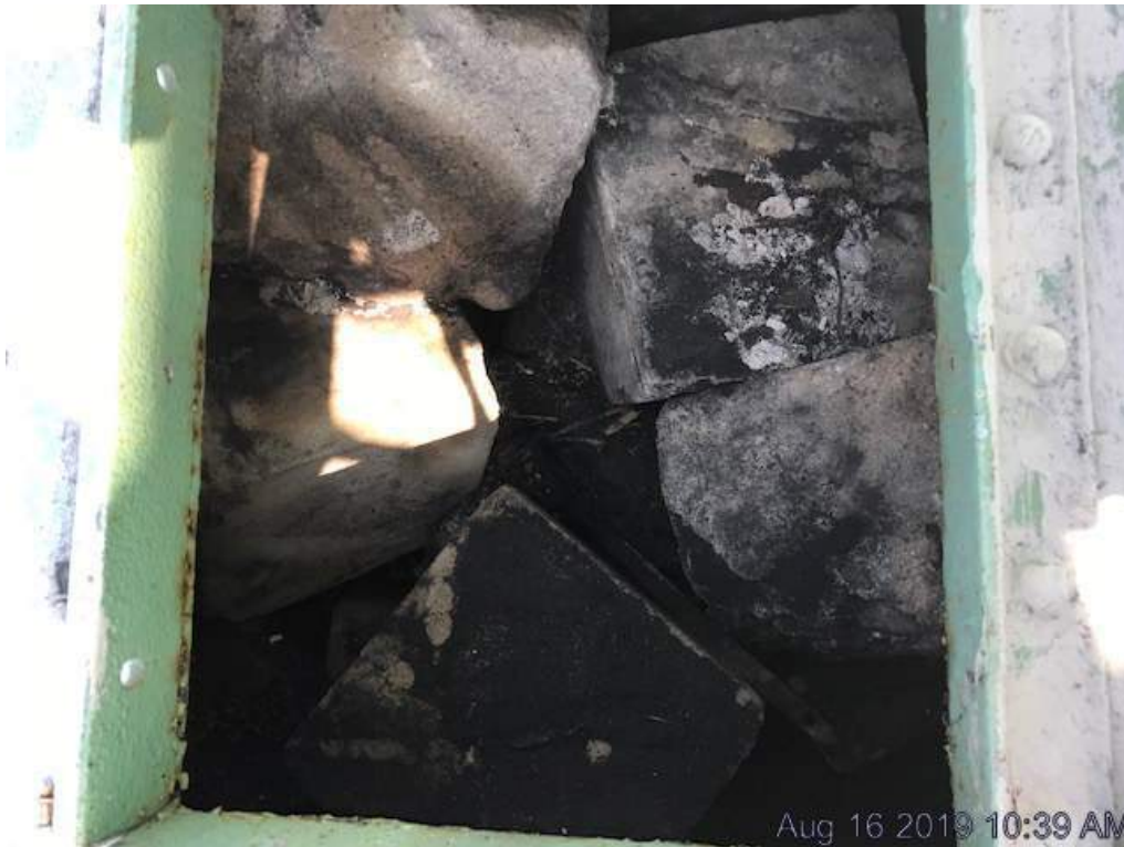
Photo S-70: The concrete in the two upper chambers in the top face of the counterweight exhibits spalls, disintegration, and wet areas (south chamber shown).
