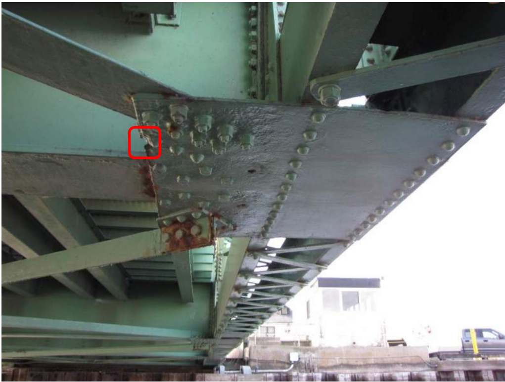
Photo S-54: Section loss and perforation in the bottom horizontal gusset plate at node 10N.
