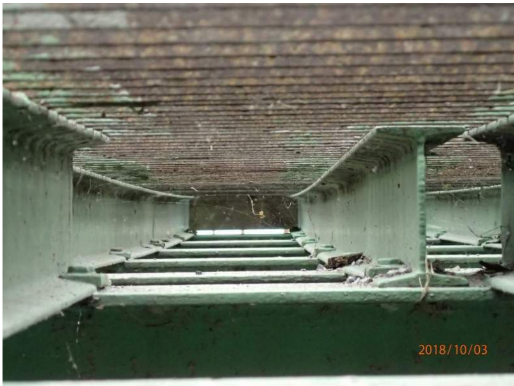
Photo S-62: The sills supporting the deck grating are typically permanently deflected (photo from 2018 CDI).
