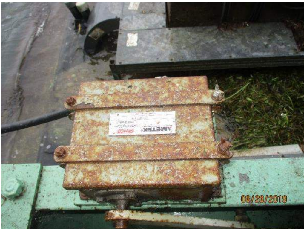
Photo M-24: North Span Lock Rotary Cam Switch. The rotary cam limit switch cover exhibits paint deterioration and light corrosion.
