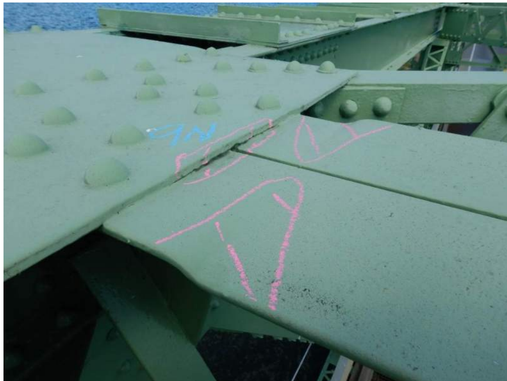
Photo S-89: Deformation of sway bracing member 9S-9N at node 9N.
