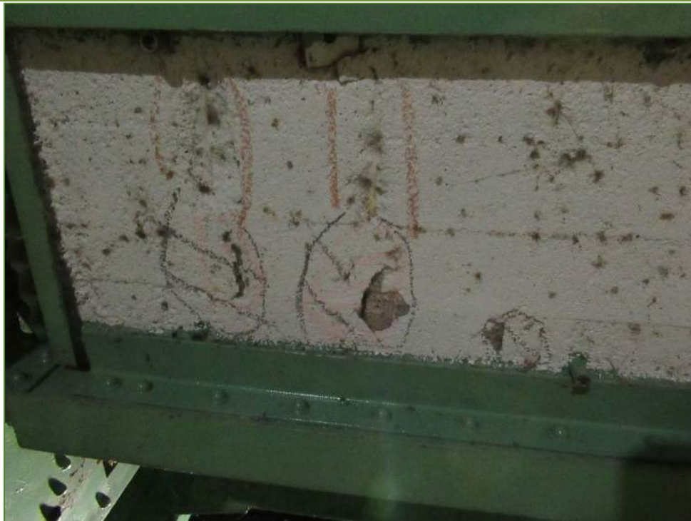
Photo P12 Machinery Room Slab Soffit Deterioration (cracks, spall and delamination)
