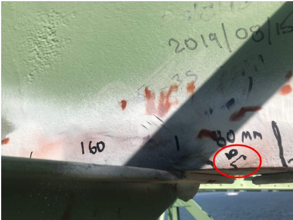
Photo S-14: An 80mm long lamination defect with a 60mm long crack in the south face of top chord member 3S-5S. A diagonal crack 10mm long is propagating from the bottom, where a crack 50mm long parallel to main stress is located (not seen in photo) (photo by Brouco NDT).
