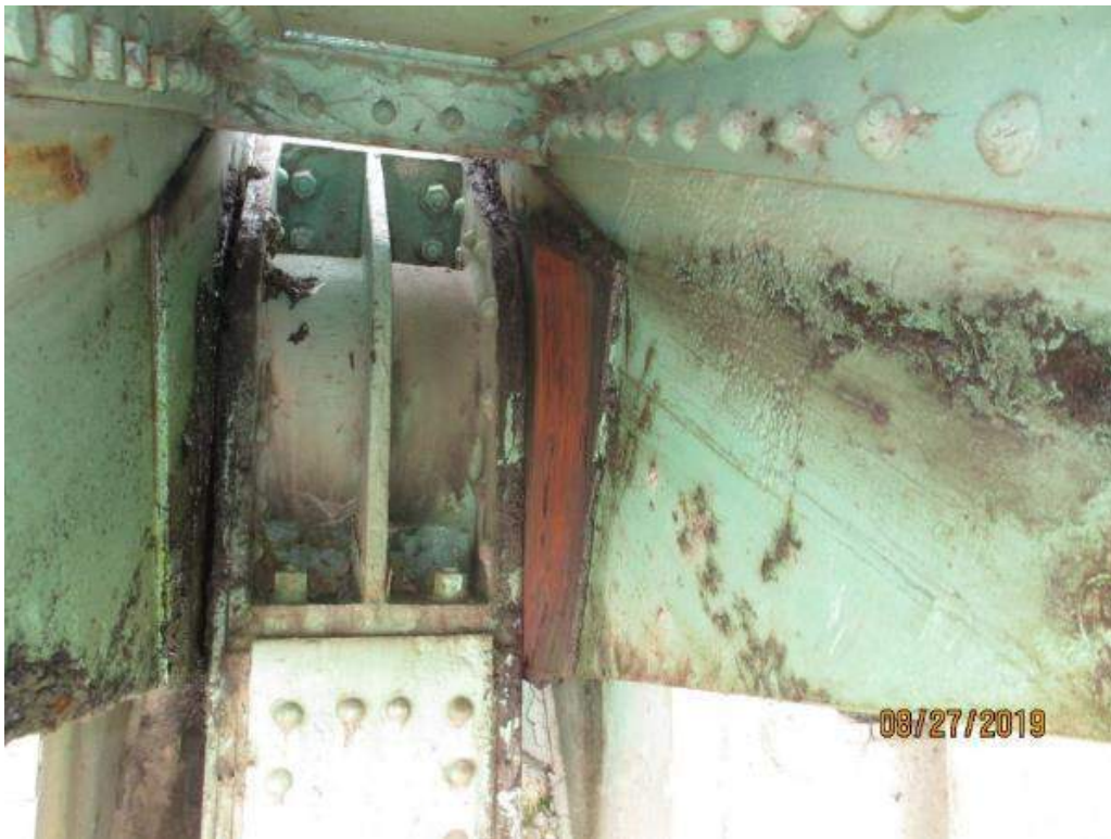
Photo M-11: North Main Trunnion Bearing. There is contact between the moving structure and the fixed structure.
