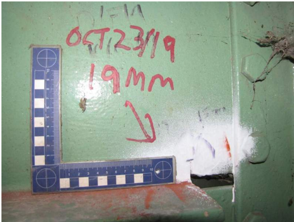
Photo S-60: 19mm notch/crack in the bottom cope of Stringer D (FB14-FB16) at FB14.
