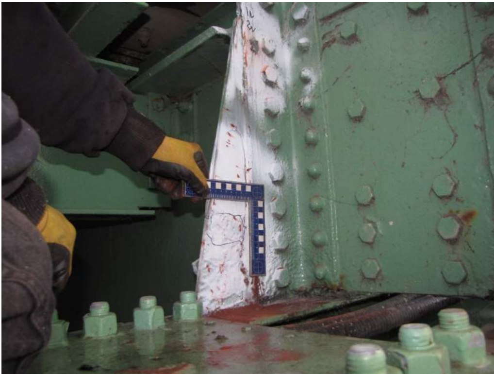
Photo S-53: Full-width crack in southwest vertical gusset plate at 2N (no increase in length from previous inspection).
