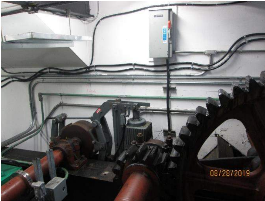
Photo E-13: Manual (Machinery) Brake & Disconnect. A manual brake with a local disconnect switch is provided in the bridge machinery space. Only set and released limit switches have been provided for this brake; the code required brake hand released limit switch has not been provided.
