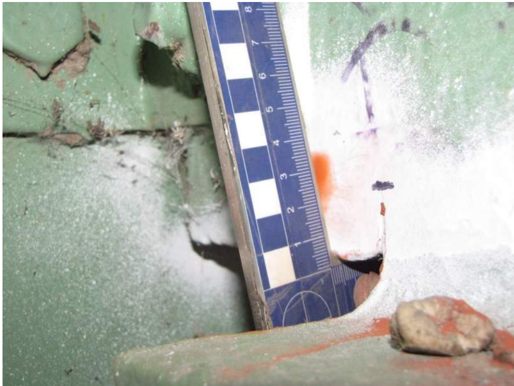
Photo S-59: 25mm notch/crack in the bottom cope of Stringer E (FB10-FB12) at FB10.
