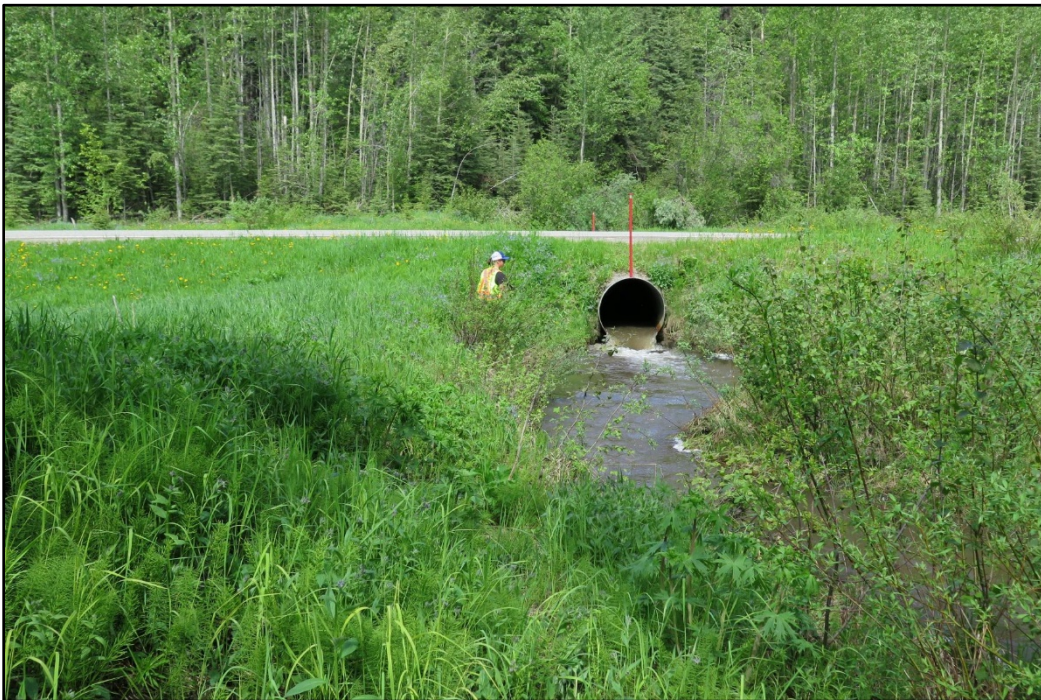
Photo 1: View N of the outlet of a drainage near the W extent of the Project
