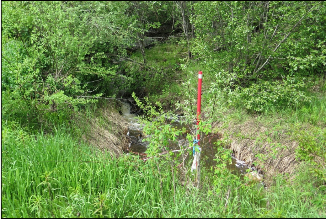
Photo 11: View N of the inlet of a drainage at Tetsa River Lodge
