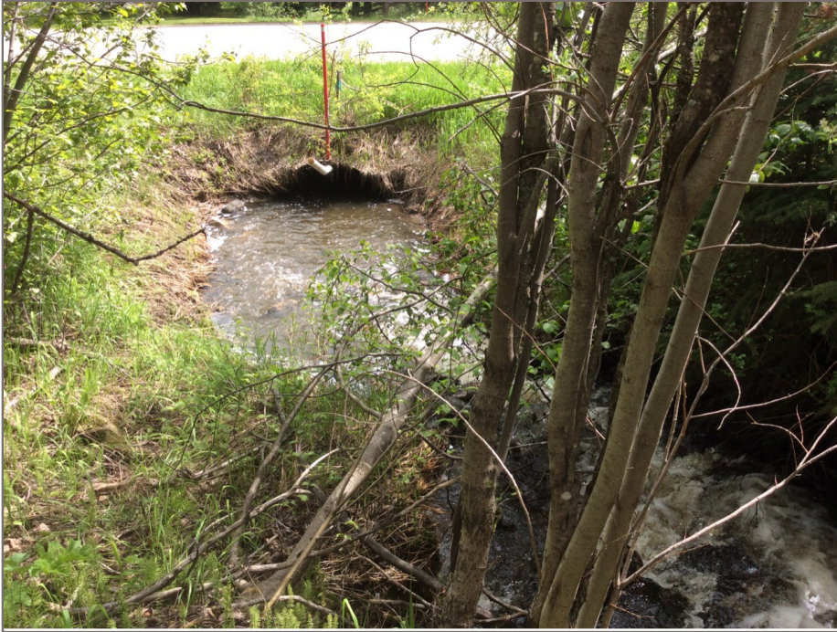
Photo 1: Culvert inlet at KM 568.84. The inlet is located on the north side of the highway.
