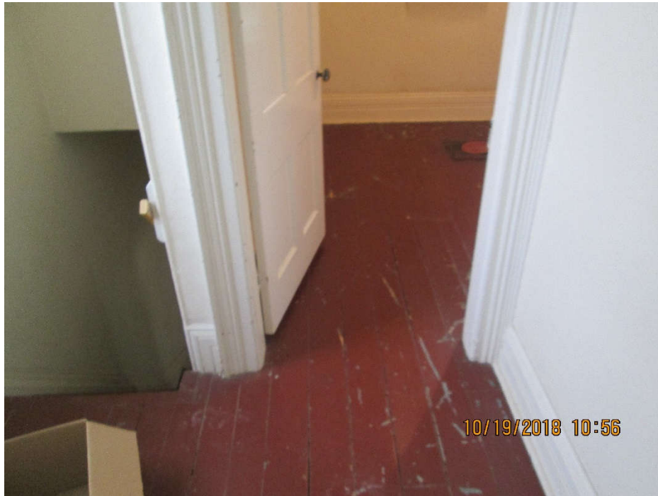
Photo 5: View of the red lead-based paint (Sample 673155-P-08) on the floor of bedroom 4 of the dwelling
