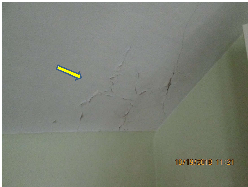
Photo 6: View of white lead-based paint (Sample 673155-P-13) on the ceiling in the bedroom 2 of the dwelling.
