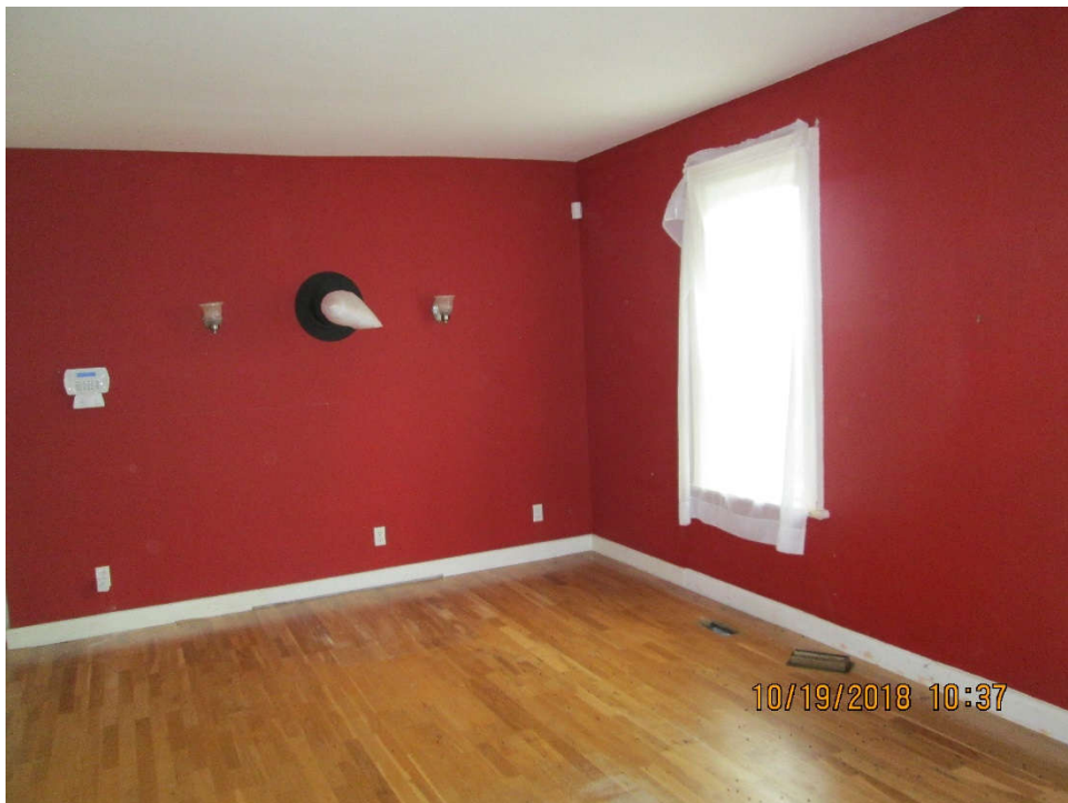
Photo 2: View of the asbestos-containing texture coat (Sample 673155-TC-03-A,B,C and red lead-based paint (Sample 673155-P-06) on walls in the living room and white lead-based paint on the living room window sill (Sample 673155-P-02).
