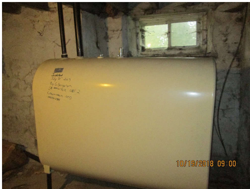
Photo 10: View of the furnace oil AST located in the basement of the dwelling.
