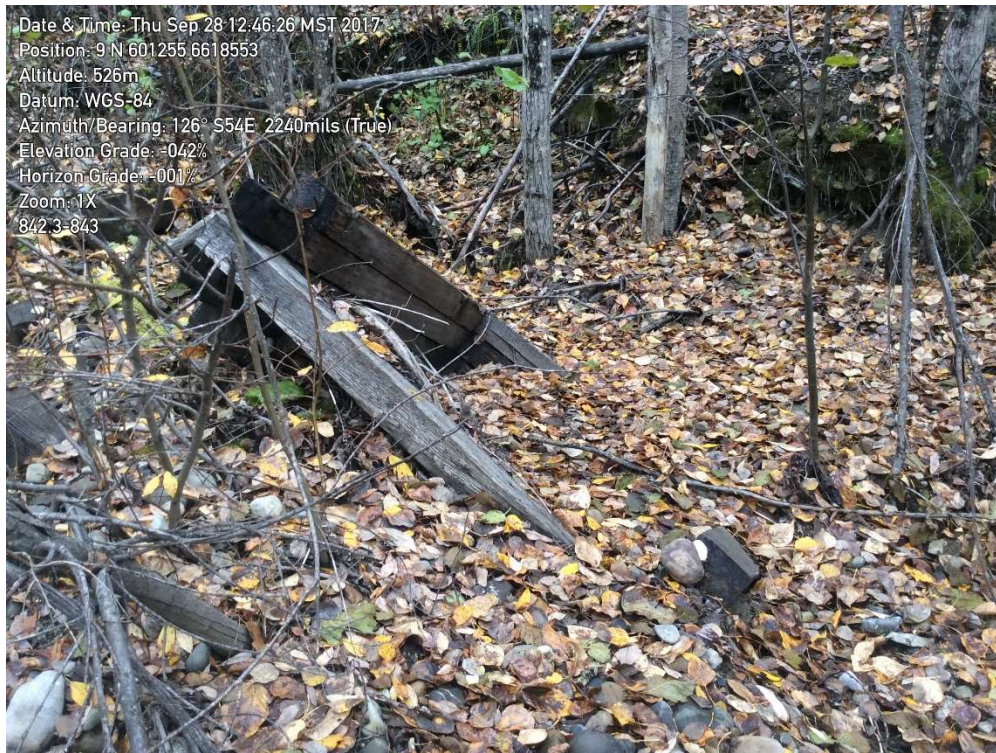
Photo 13: Site 2 (Km 841.95 to 844.40) – Debris downstream of box culvert - Photo 1 of 6
