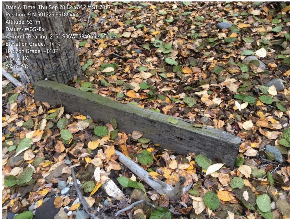
Photo 17: Site 2 (Km 841.95 to 844.40) – Debris downstream of box culvert - Photo 5 of 6
