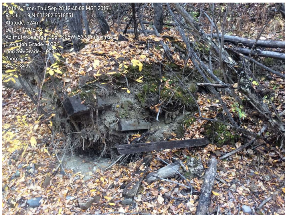
Photo 14: Site 2 (Km 841.95 to 844.40) – Debris downstream of box culvert - Photo 2 of 6
