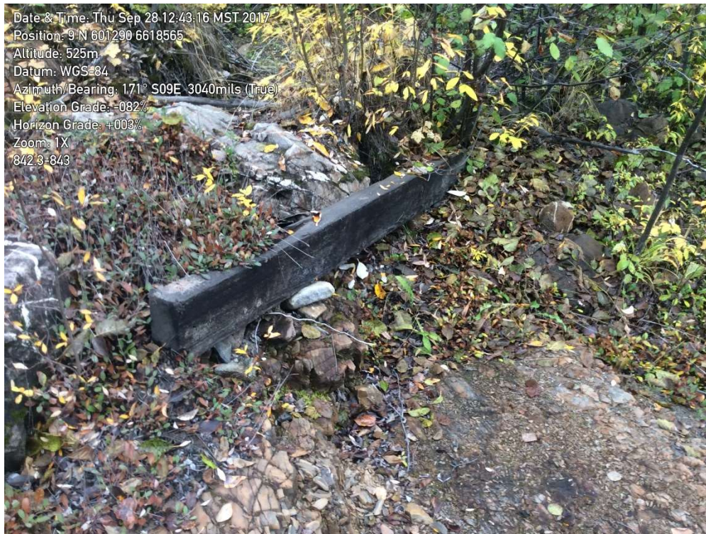
Photo 15: Site 2 (Km 841.95 to 844.40) – Debris downstream of box culvert - Photo 3 of 6
