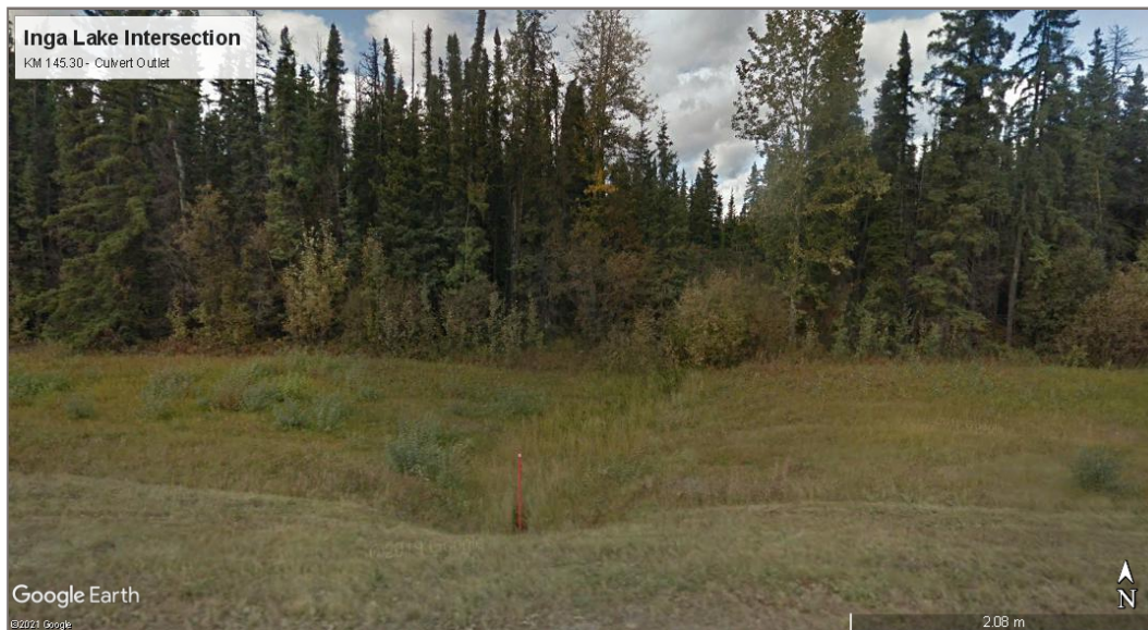
Photo 6: KM 145.30 Culvert outlet / downstream – This culvert is located at the headwaters of a small 1 st order watercourse and will be undergoing a culvert extension (Google Earth 2021).
