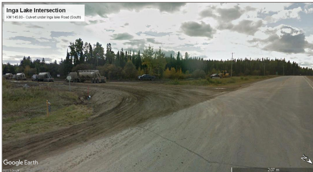
Photo 4: KM 145.80 (south) Culvert – Located under Inga Lake Road south of the Alaska Highway (Google Earth 2021). This culvert conveys the roadside ditch under the side road and is not considered to be a 'stream' under the WSA.
