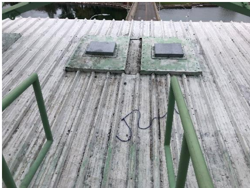
Figure 14: Access Hatches on Top Face
