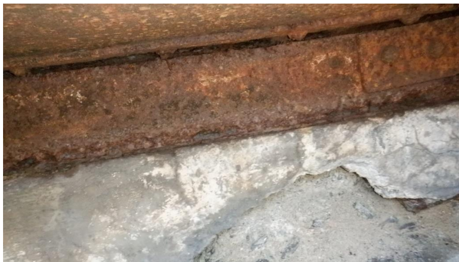
Figure 16: Exposed Structural Steel within Top Face Access Hatches (Member from Girder F Shown)
