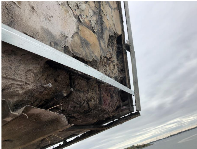
Figure 12: Typical Condition of the Counterweight Bottom Face and Cladding
