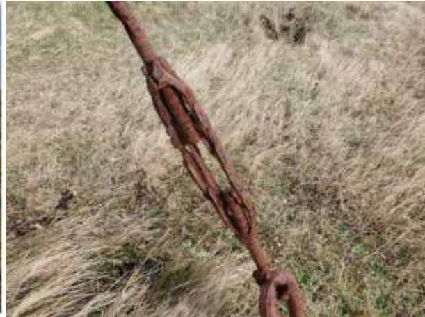
Severely corroded guy rope
