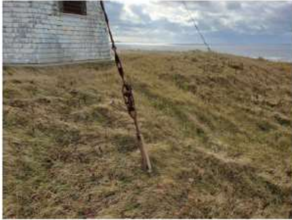
Corroded guy rope
