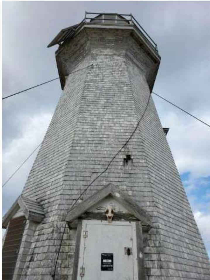
Anchoring of the shrouds on the lighthouse and wooden facing of the lighthouse
