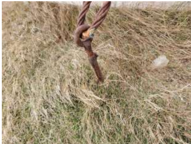
Guy wire not anchored to the ground
