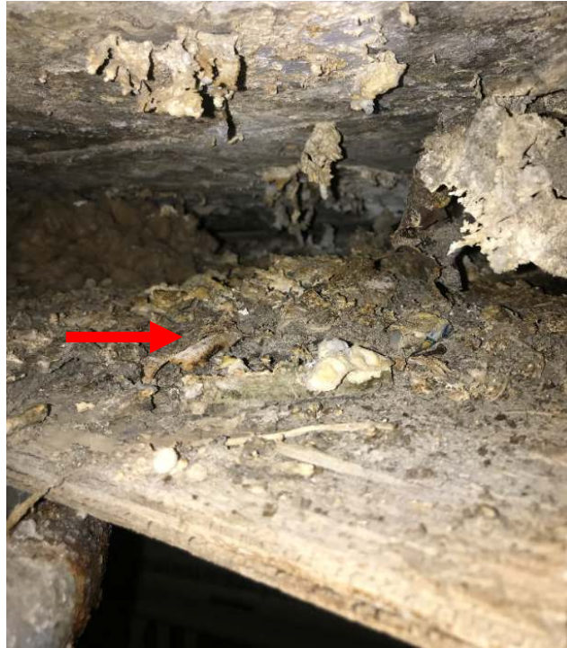
Photo 7. Miscellaneous debris observed on plywood within tunnels under the vents noted in Section 5.1.2 was confirmed non-asbestos containing (DST Sample ID 3603-01A-C to 08A-C).
