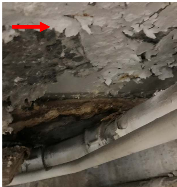
Photo 8. White ceiling paint within the tunnel under Type D Vent V1 was confirmed to contain 918 ppm lead (DST Sample ID 3603-LP01).
