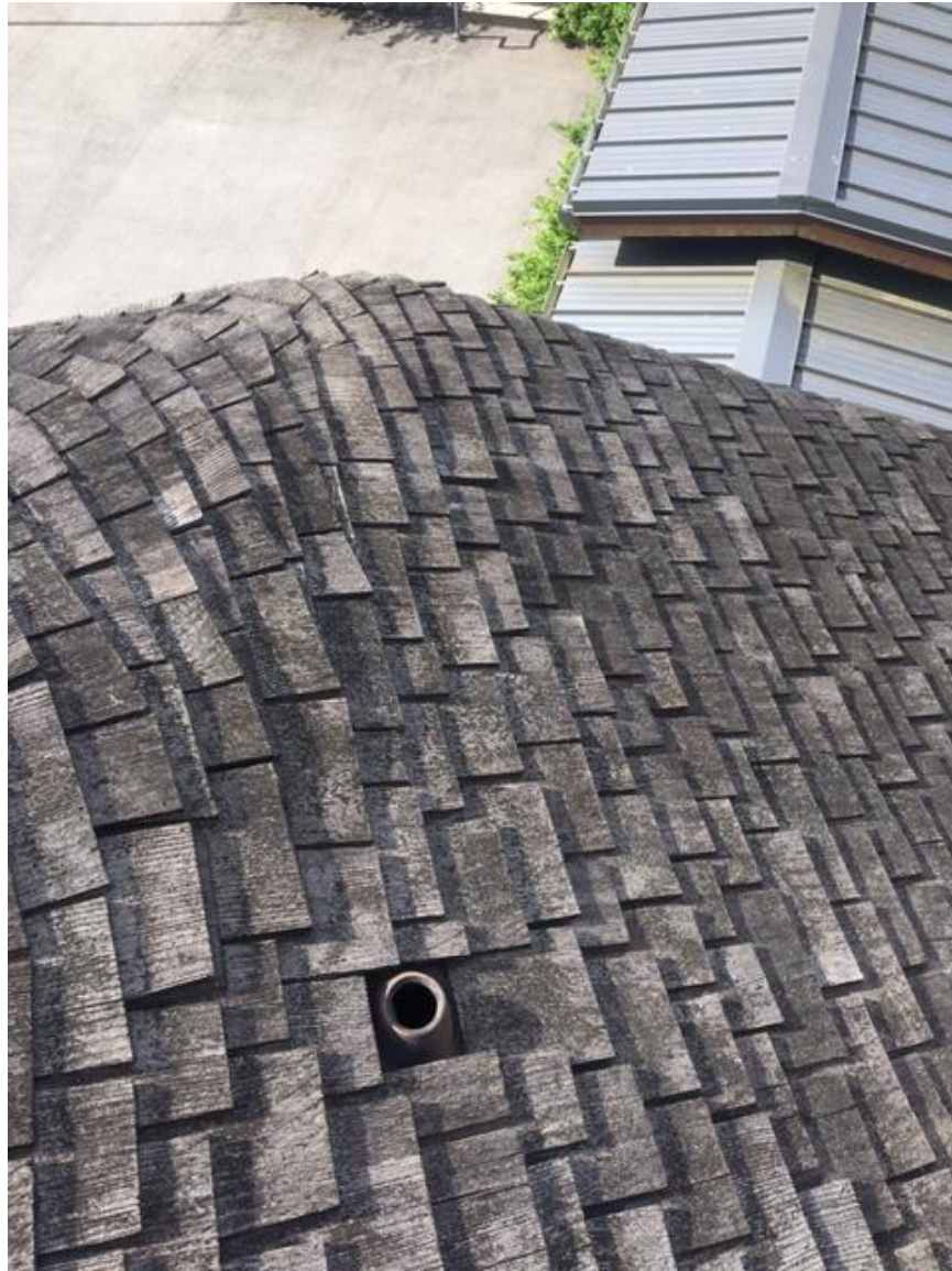
Lodge Building - Lead vent pipe
