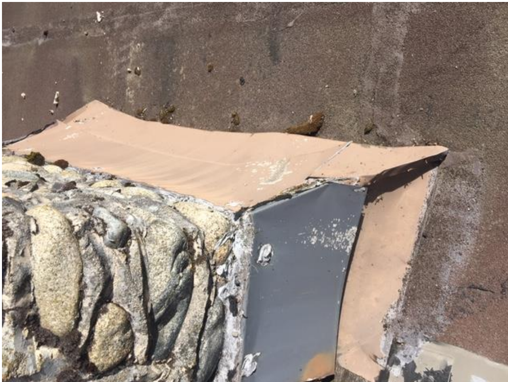
Lodge Building – Grey and black caulking around chimney.
