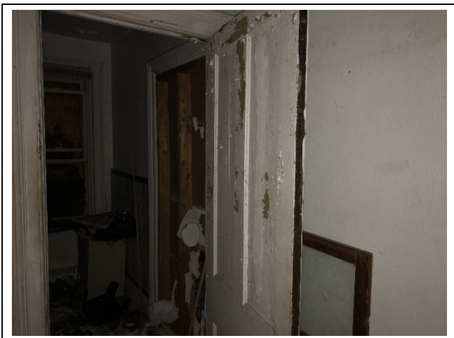
Photo 3: Flaking lead-containing white coloured paint on first floor washroom door.
