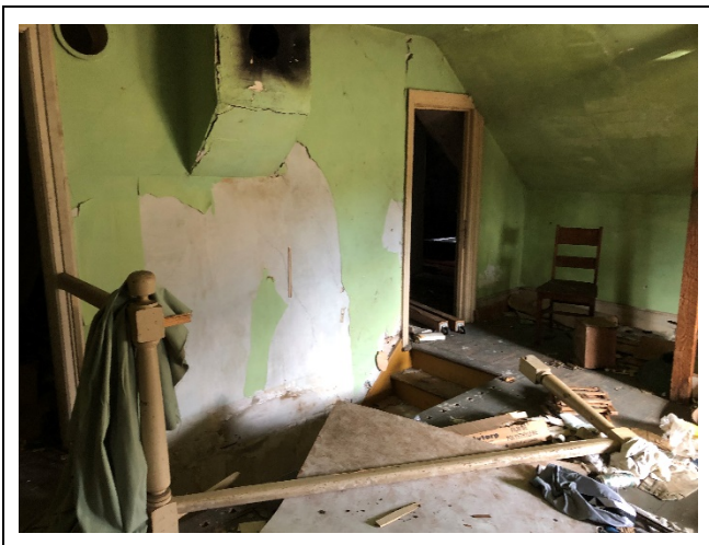
Photo 5: Flaking lead-containing green coloured paint on the walls and ceiling of 2 nd floor bedroom 7.
