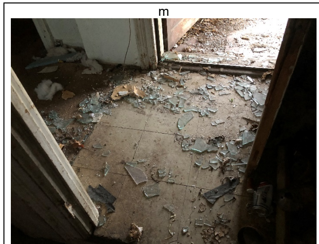
Photo 2: Asbestos-containing vinyl floor tiles – beige in the first floor hallway.
