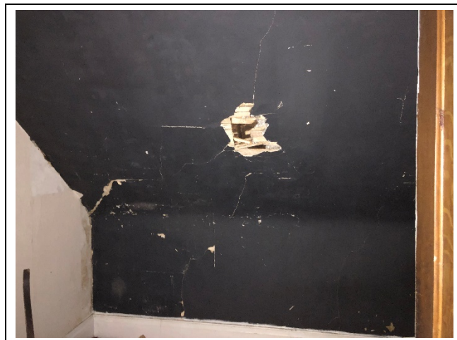
Photo 4: Flaking lead-containing paint on the second floor storage room 2 ceiling.
