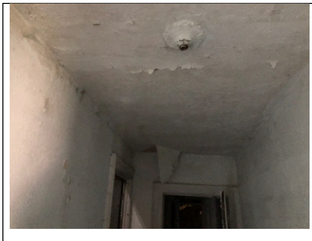
Photo 8: Suspect mould growth on ceiling in second floor hallway.
