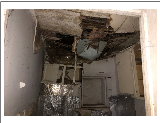
Photo 7: Suspect mould growth and ceiling collapsing in storage room 1 on the first floor.
