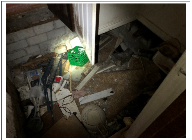
Photo 4: Asbestos-containing paper-backing associated with vinyl sheet flooring – mosaic pattern in first floor washroom 1.
