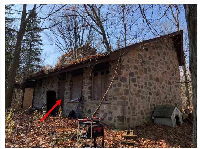
Photo 7: Exterior door caulking – grey on exterior living room door.
