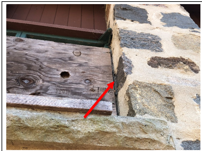
Photo 6: Asbestos-containing exterior window caulking – grey on exterior windows.
