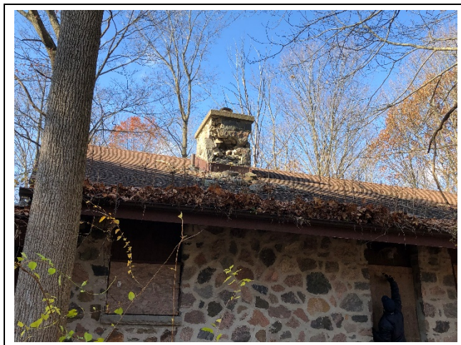
Photo 8: Presumed asbestos-containing roofing material and roof caulking.
