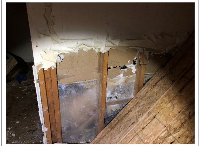
Photo 2: Damaged asbestos-containing drywall joint-fill compound in the first-floor hallway.
