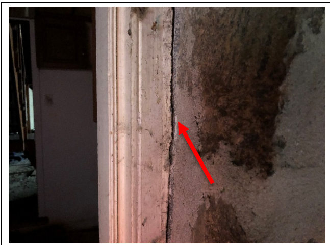
Photo 5: Asbestos-containing interior door caulking in the first-floor foyer.
