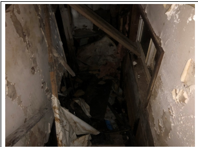
Photo 9: Suspect mould and water staining on walls in stairwell to basement
