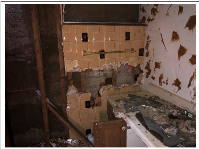
Photo 3: Damaged asbestos-containing drywall joint-fill compound in the first-floor washroom 2.
