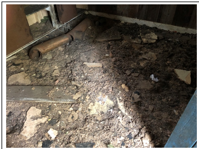
Photo 12: Suspect mould growth on water damaged ceiling tile and insulation debris in the kitchen.
