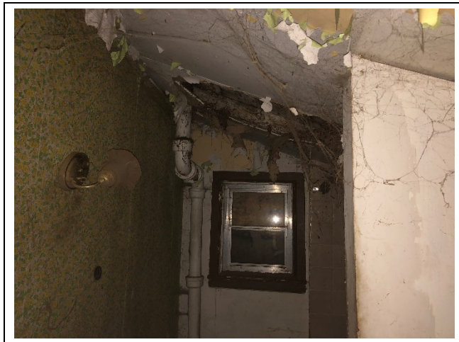
Photo 14: Suspect mould growth on water damaged drywall ceiling in the washroom. The drywall ceiling was observed to have collapsed
