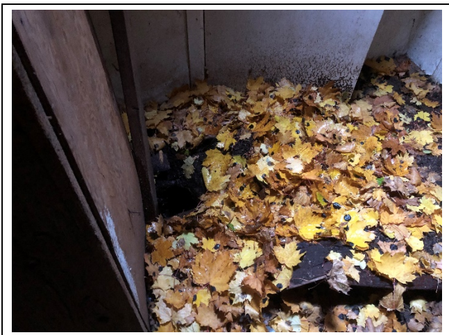
Photo 15: Suspect mould growth on water damaged drywall ceiling debris in the hallway. Leaf litter was observed due to a collapsed roof.
