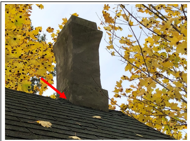
Photo 7: Presumed asbestos-containing roof caulking around chimney.
