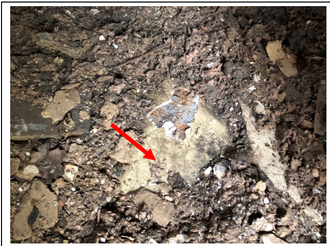
Photo 5: Asbestos-containing paper backing associated with vinyl sheet flooring – yellow in the kitchen. The vinyl sheet flooring is covered by ceiling tile and fibreglass insulation debris.
