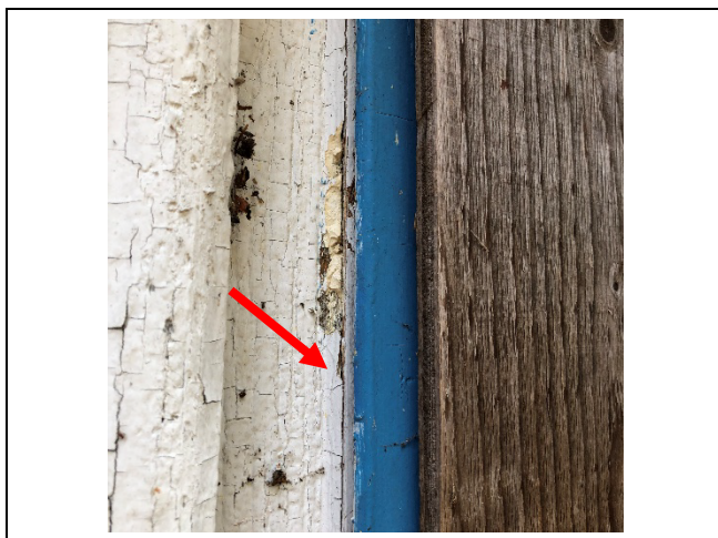
Photo 4: Damaged asbestos-containing exterior door caulking.
