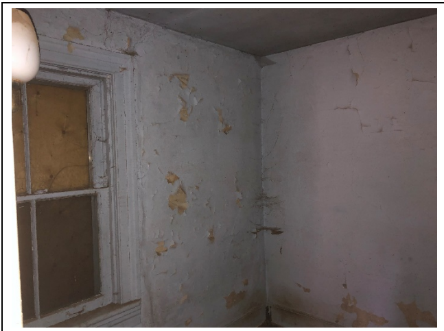
Photo 9: Peeling lead-containing blue coloured paint in Bedroom 2.
