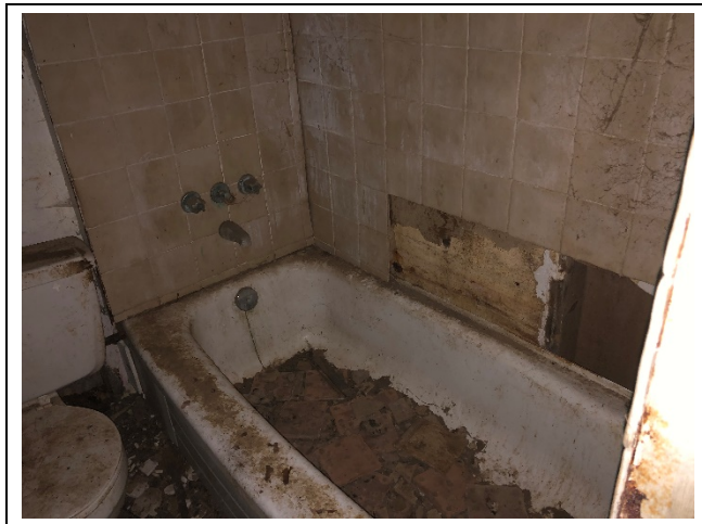
Photo 6: Presumed asbestos-containing ceramic tile grout and mortar/adhesive in the washroom.
