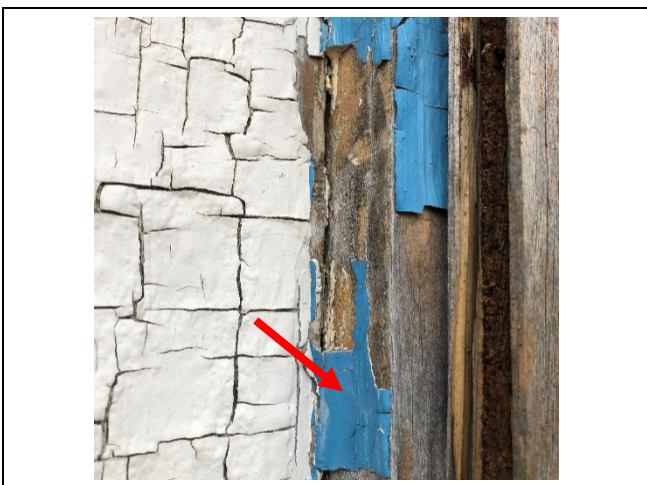
Photo 3: Damaged asbestos-containing exterior window caulking.
