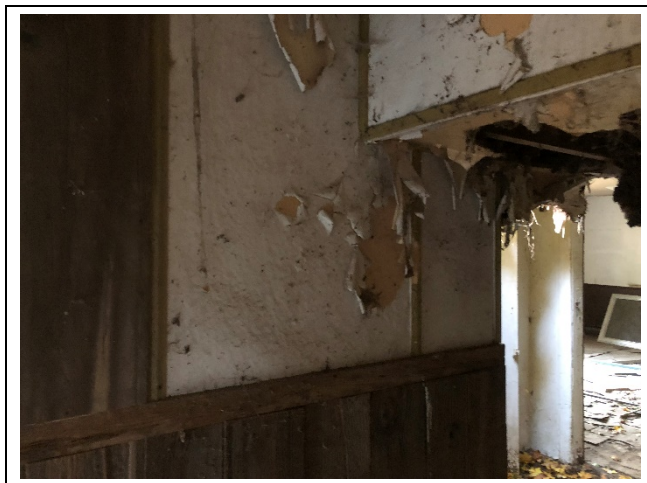
Photo 8: Peeling lead-containing white coloured paint in the kitchen.
