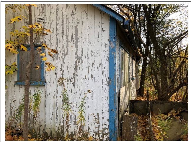
Photo 11: Flaking lead-containing light blue and white coloured paint on exterior walls.
