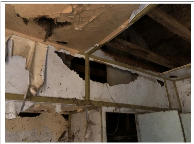
Photo 13: Suspected mould growth on water damaged ceiling tiles and wall panels in the kitchen.
