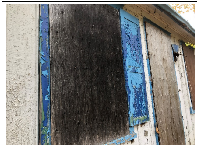
Photo 10: Flaking lead-containing dark blue coloured paint on exterior window shutters and frames.
