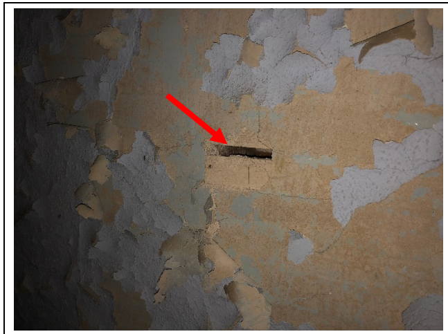
Photo 2: Damaged asbestos-containing wall plaster in bedroom 1.
