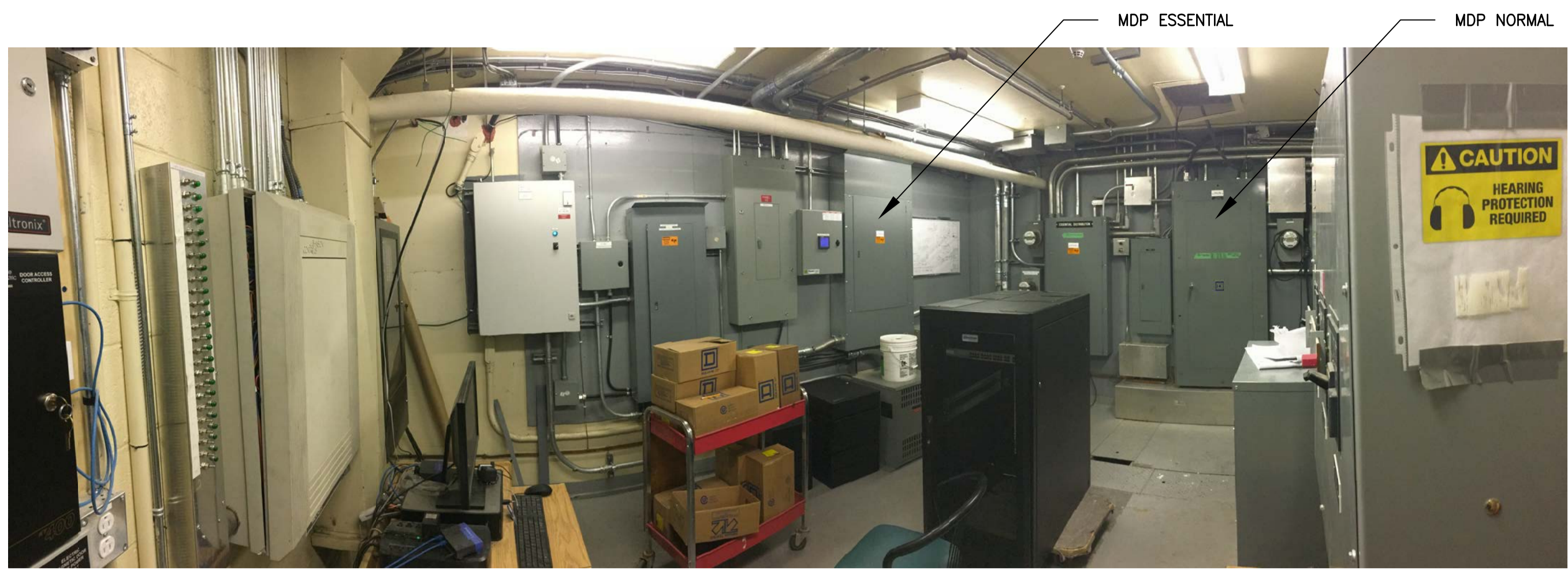
1 ELECTRICAL ROOM E002
