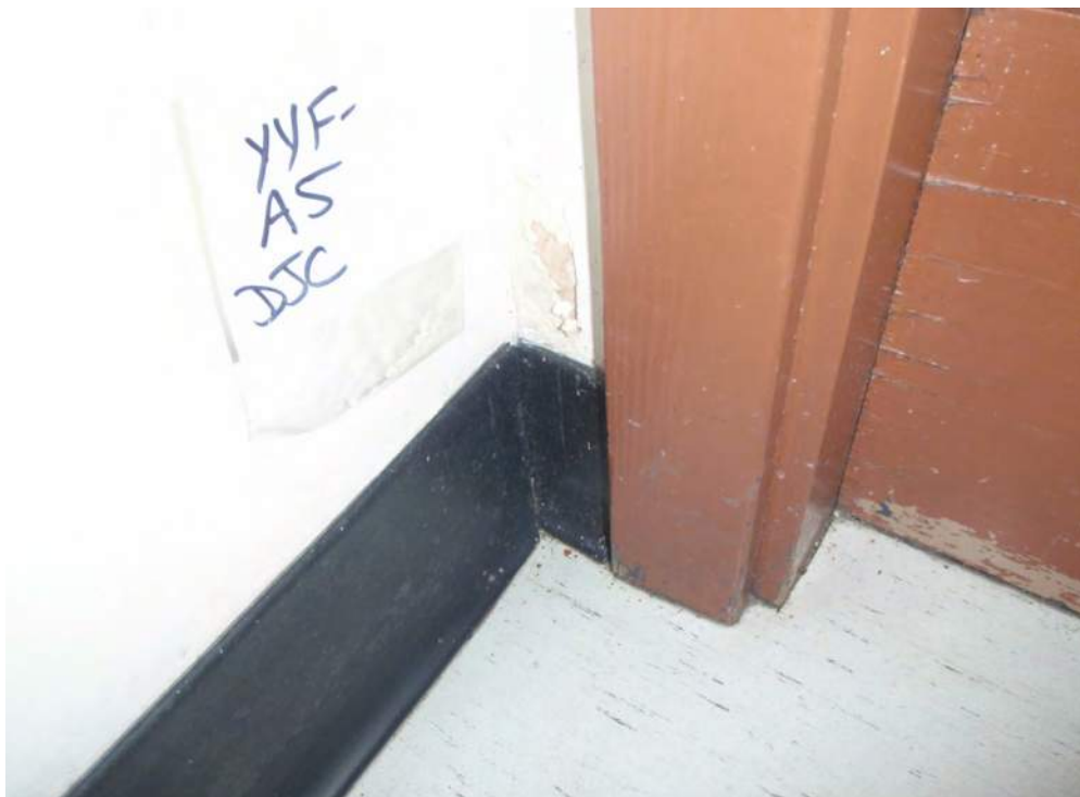
Photograph 30: Asbestos-containing drywall joint compound in Room 125 (Sample A5).
