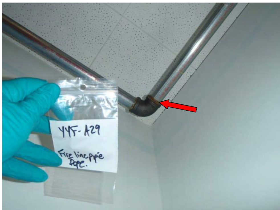
Photograph 36: Asbestos-containing pipe thread sealant on fire line in Room 124 ( Sample A29 ).
