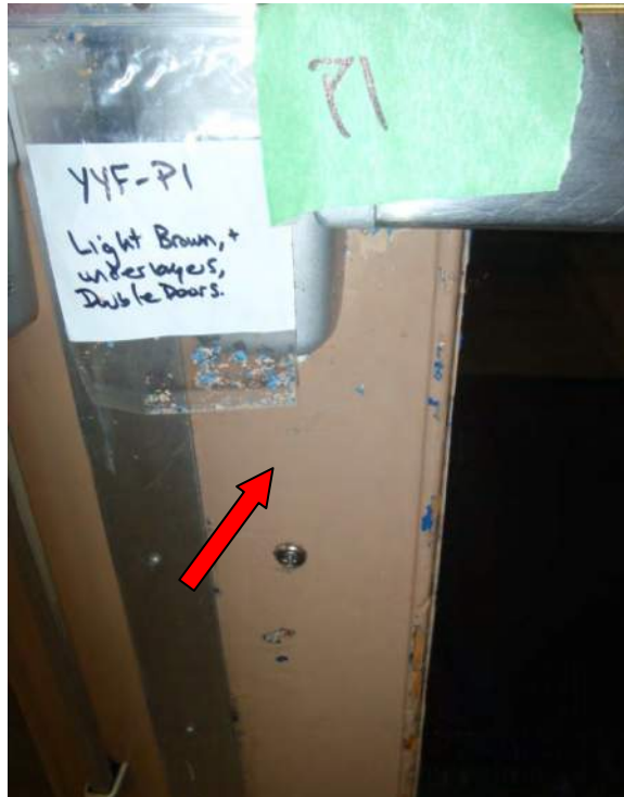
Photograph 59: Lead-based light brown/blue paint on double doors in Room 125 ( Sample P1 ).
