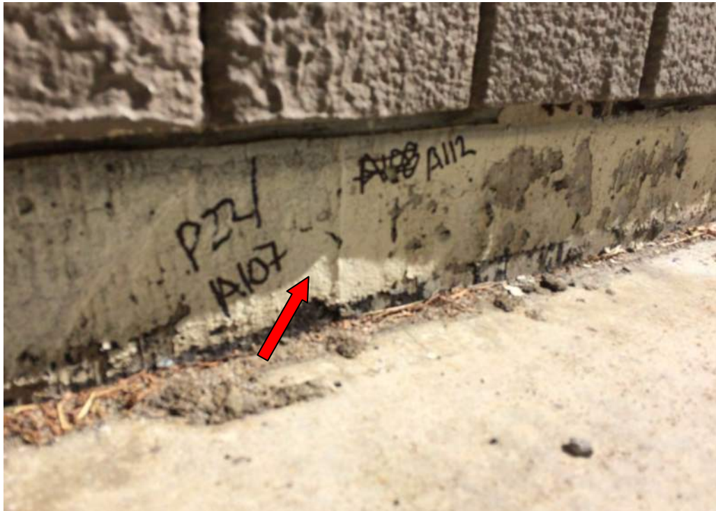
Photograph 73: Lead-based white paint on tar of foundation exterior ( Sample P22 ).
