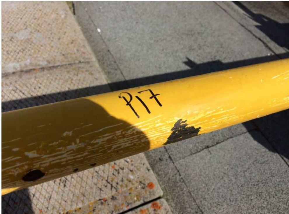
Photograph 69: Lead-based yellow paint on steel pipe on roof ( Sample P17 ).
