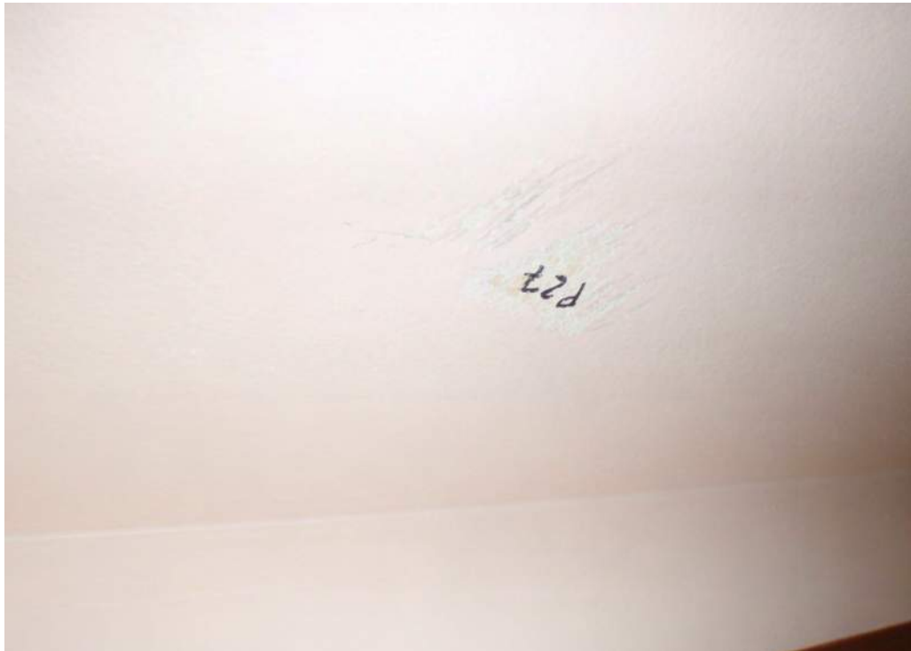
Photograph 77: Lead-based pink wall and ceiling paint in Room 128B ( Sample P27 ).
