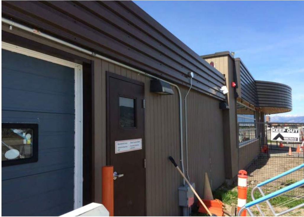
Photograph 5: East side of building (Rooms 105B/107 on left, new hold room on right) – Facing northwest.
