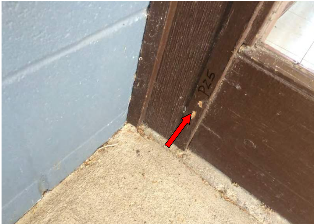
Photograph 75: Lead-based dark brown paint on exterior door frame to Room 125 ( Sample P25 ).
