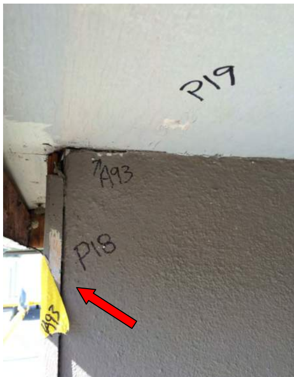
Photograph 70: Lead-based grey paint on wall of raised portion of roof ( Sample P18 ) and lead-based white paint on soffit of raised portion of roof ( Sample P19 ).
