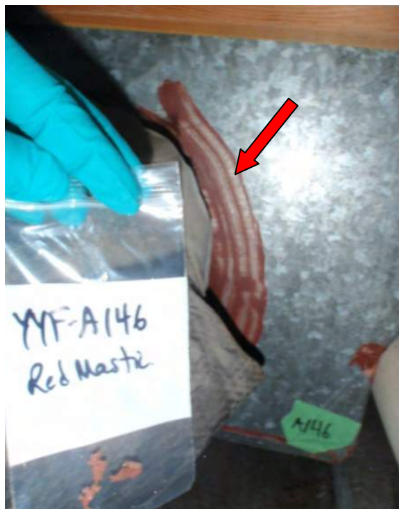
Photograph 50: Asbestos-containing red mastic on HVAC ducting in crawlspace beneath Room 136 ( Sample A146 ).
