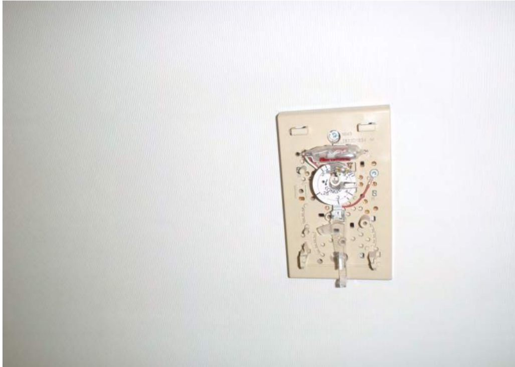
Photograph 25: Typical mercury-containing thermostat (Room 142).
