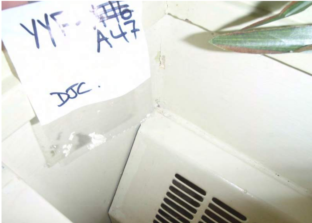
Photograph 43: Asbestos-containing drywall joint compound in Room 120 ( Sample A47 ).
