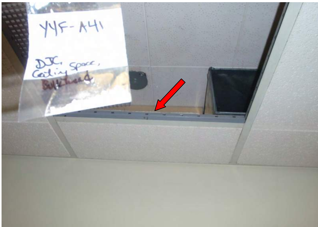
Photograph 40: Asbestos-containing drywall joint compound in ceiling space of Room 120 ( Sample A41 ).
