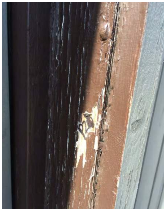
Photograph 72: Lead-based dark brown paint on window trim on east side of raised portion of roof ( Sample P21 ).
