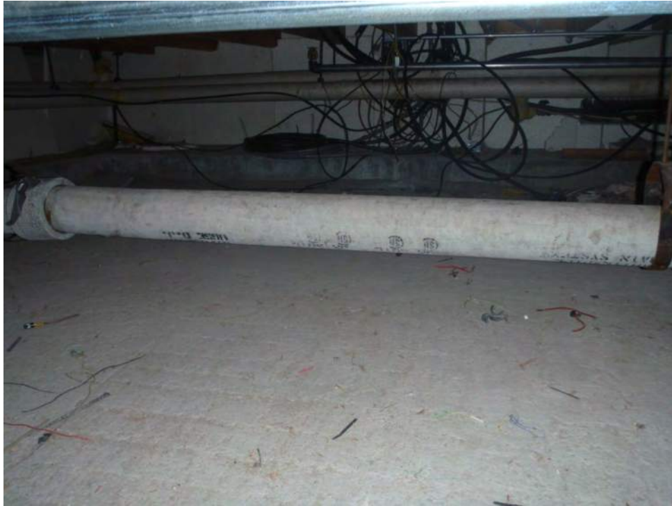
Photograph 17: Room 127 crawlspace with asbestos-containing concrete pipe.
