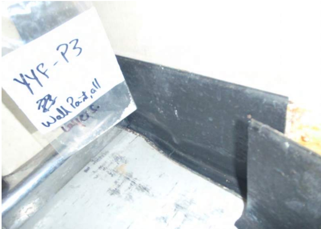
Photograph 61: Lead-based white paint on walls in Room 125 ( Sample P3 ).
