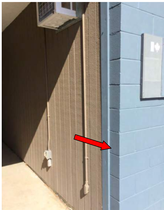
Photograph 74: Lead-based blue paint on exterior of building ( Sample P24 ).
