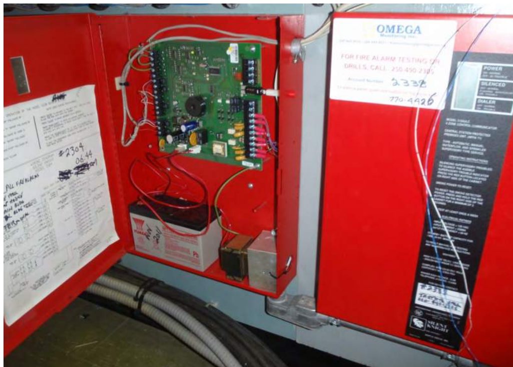
Photograph 22: Typical lead-acid battery in fire control box (Room 127).
