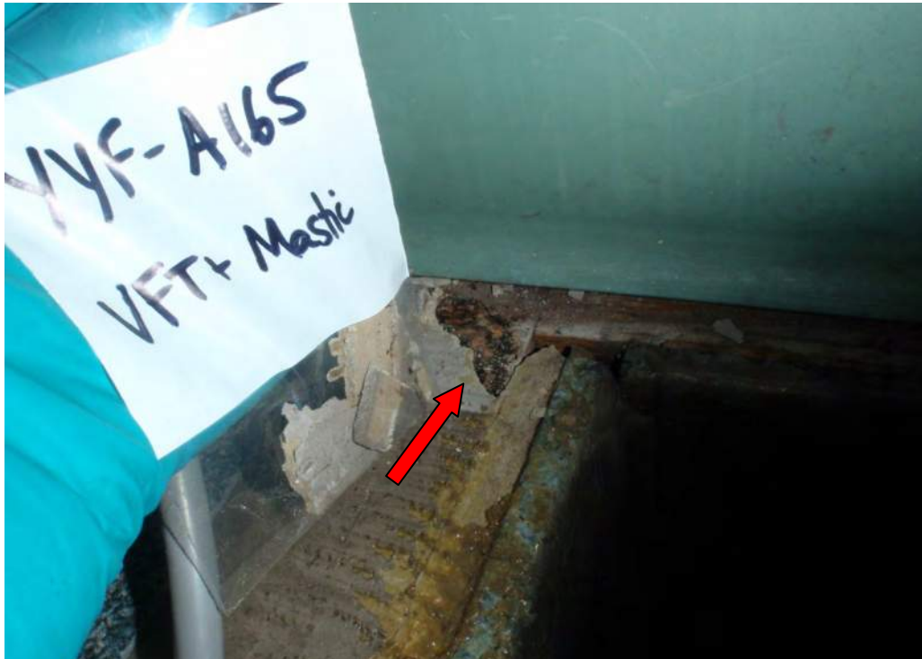
Photograph 51: Asbestos-containing off-white vinyl floor tile in Room 117 ( Sample A165 ).
