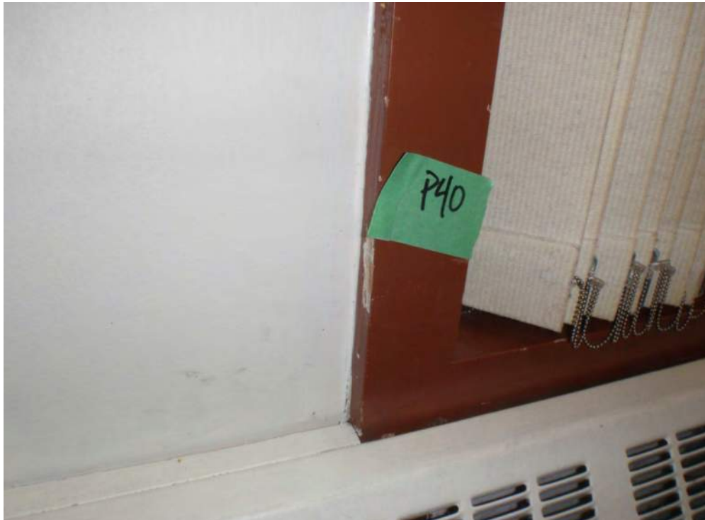
Photograph 83: Lead-based red paint on window trim along the west wall of Room 106B ( Sample P40 ).
