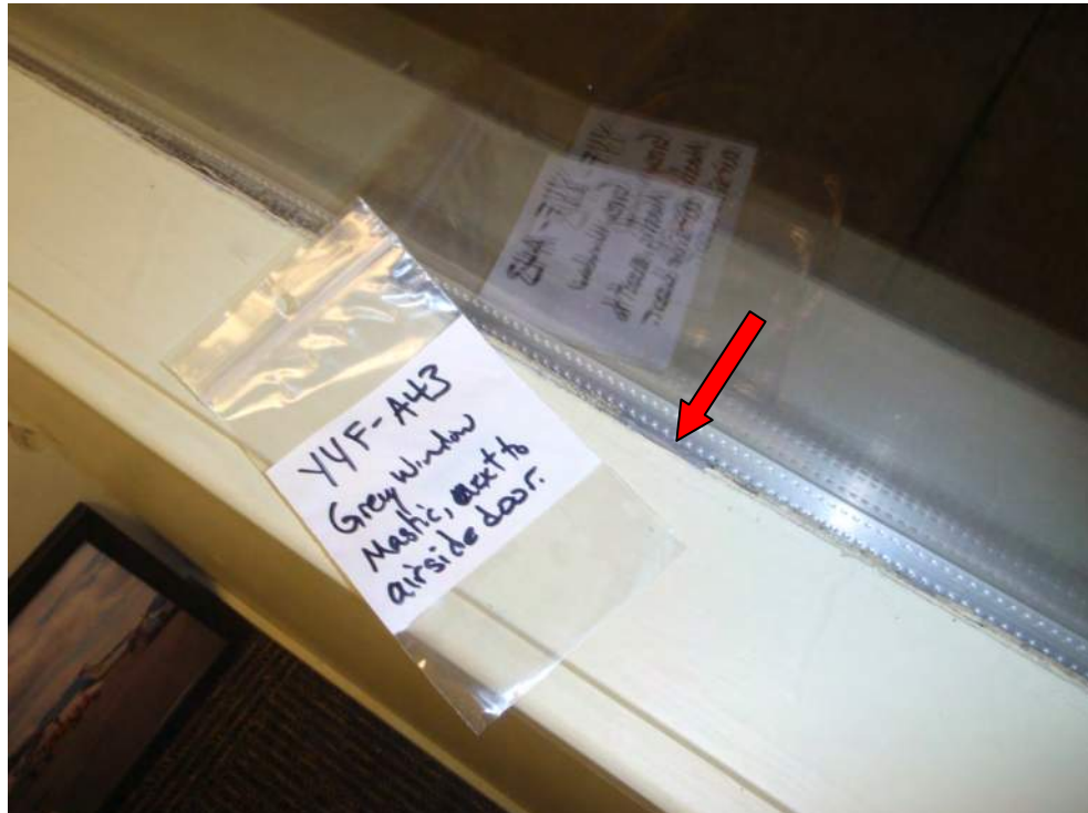
Photograph 41: Asbestos-containing grey window putty in Room 120 (Sample A43).
