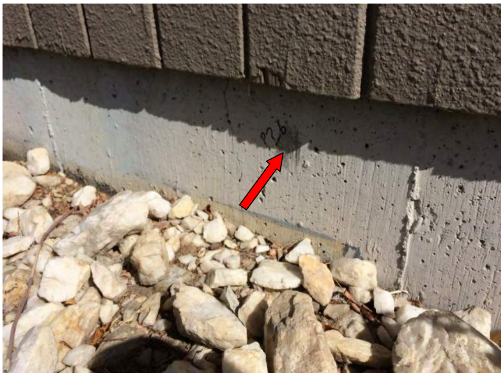
Photograph 76: Lead-based exterior light grey / white paint on concrete foundation ( Sample P26 ).
