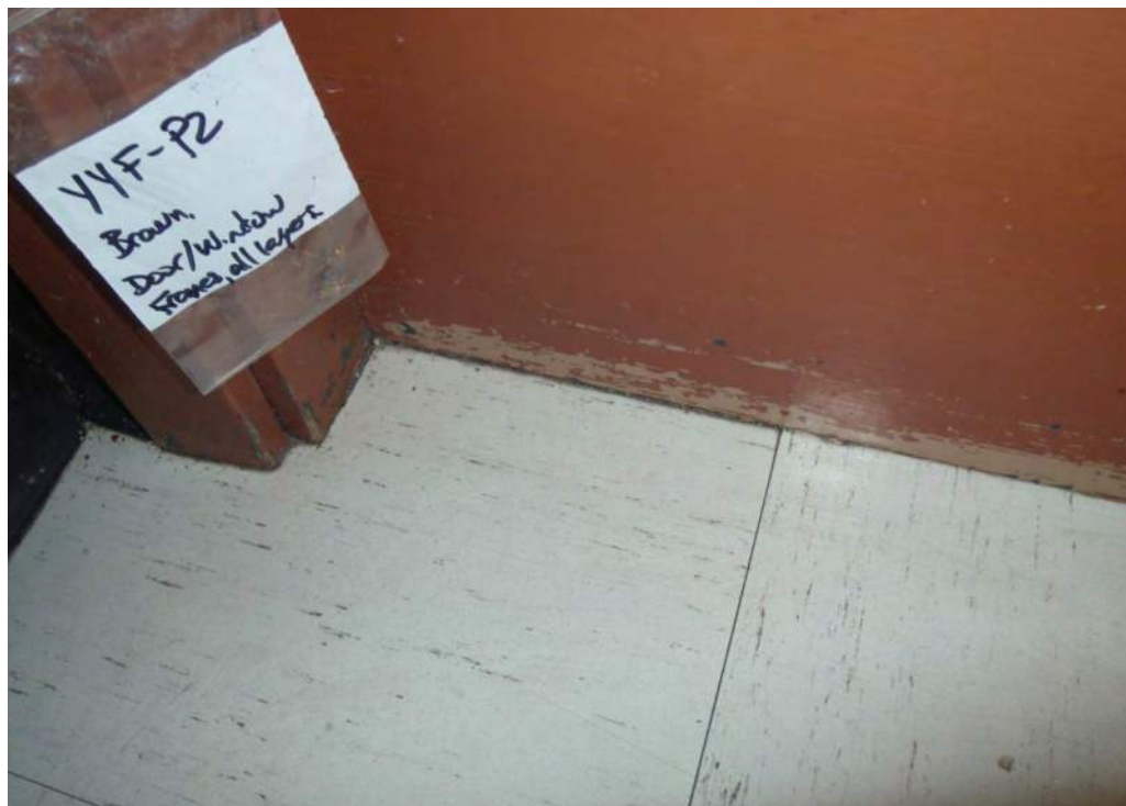
Photograph 60: Lead-based brown paint on door and window frames in Room 125 ( Sample P2 ).
