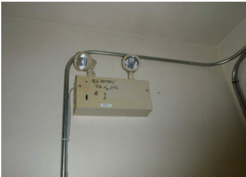
Photograph 24: Typical emergency light with potentially lead-containing battery (Room 127).
