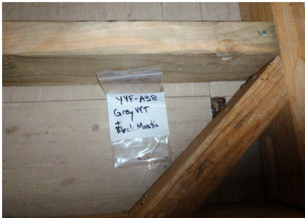
Photograph 38: Asbestos-containing grey vinyl floor tile ( Sample A38 ).
