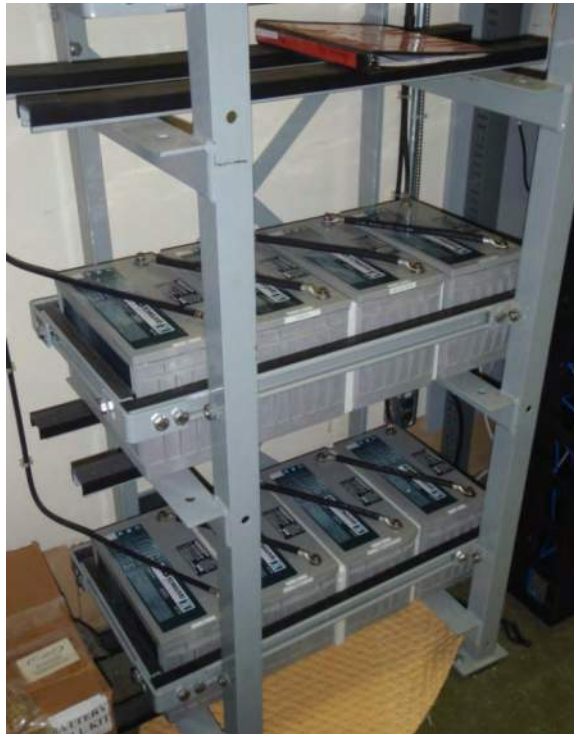
Photograph 23: Room 127 lead-containing batteries.
