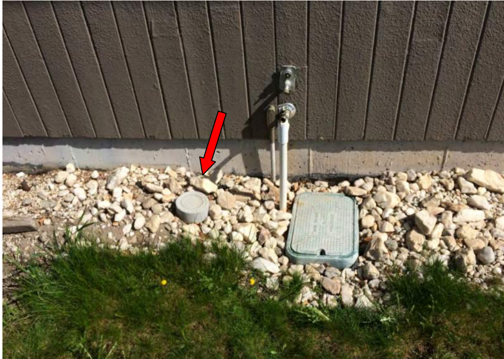
Photograph 19: Asbestos-containing concrete pipe (capped) on west side of building.
