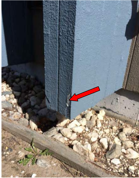
Photograph 47: Asbestos-containing exterior wall texture on west side of building ( Sample A114 and Sample A116 ).
