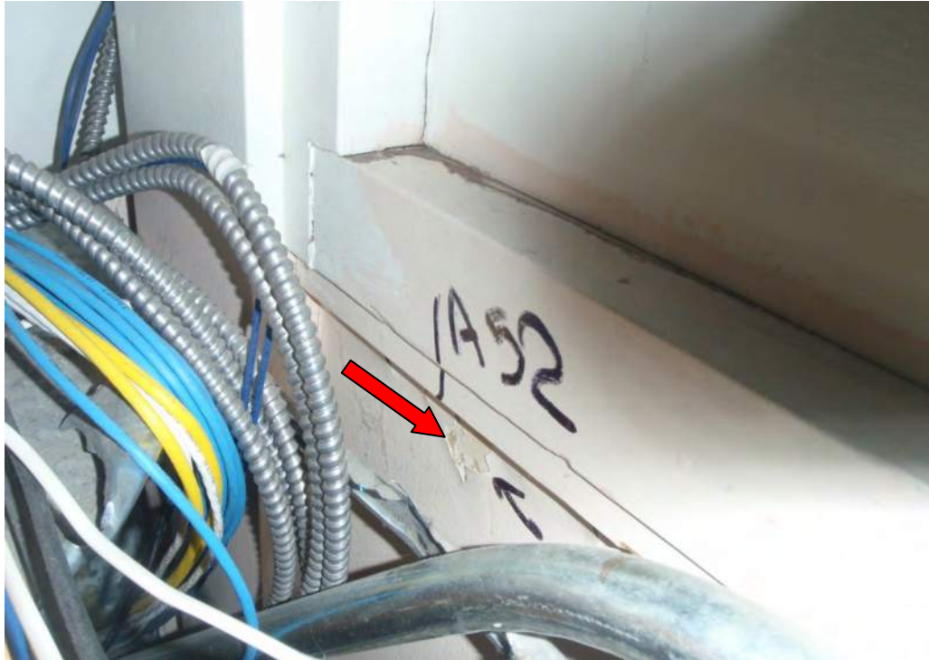
Photograph 45: Asbestos-containing drywall joint compound in Room 106A above Room 143 ( Sample A52 ).
