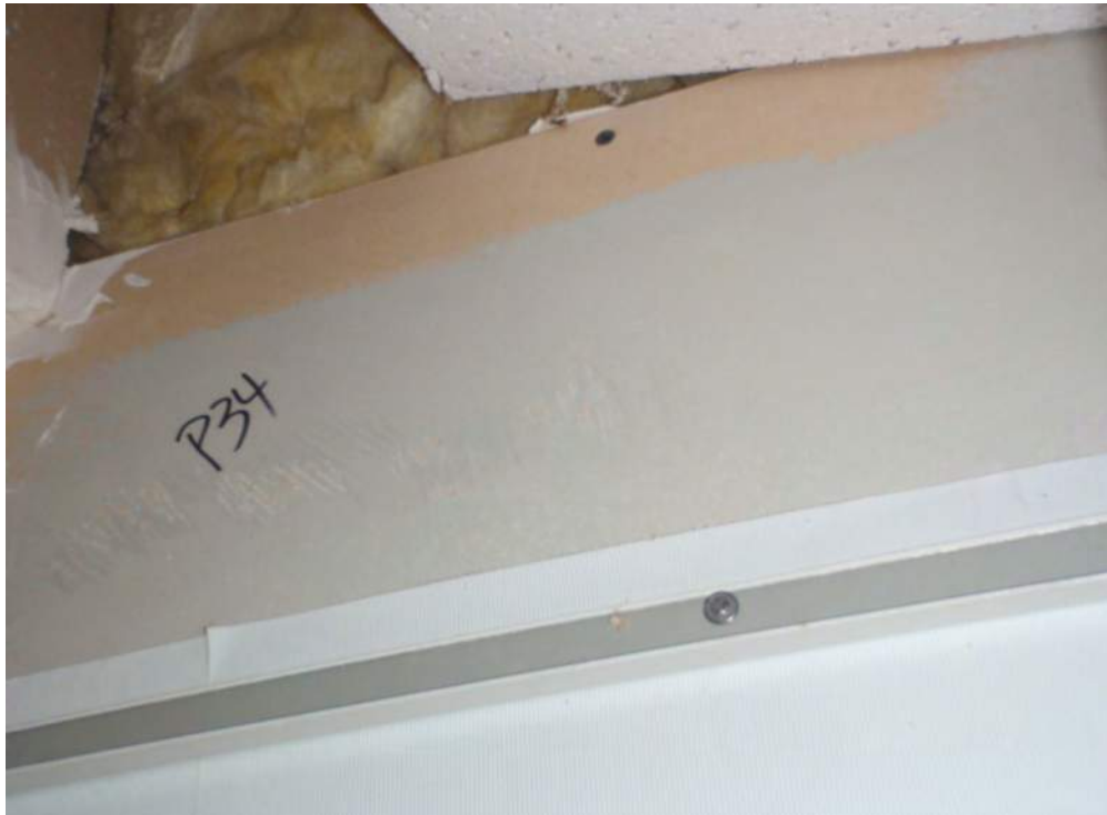
Photograph 81: Lead-based grey primer paint on wall in ceiling space of Room 142 ( Sample P34 ).
