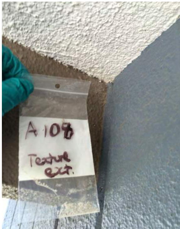
Photograph 46: Asbestos-containing exterior ceiling texture on south end of building ( Sample A108 ).
