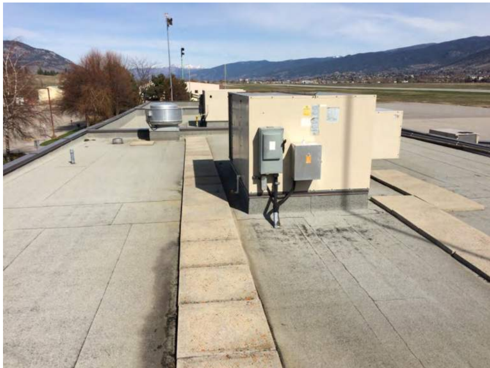
Photograph 26: Typical rooftop air conditioning unit.
