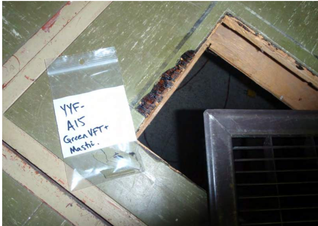
Photograph 31: Asbestos-containing green vinyl floor tiles ( Sample A15 ).
