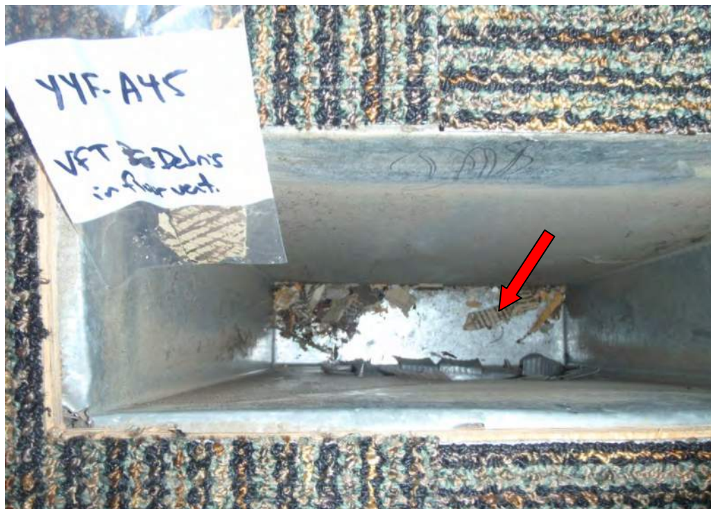
Photograph 42: Asbestos-containing grey vinyl floor tile debris located in the floor vent in Room 120 (Sample A45).
