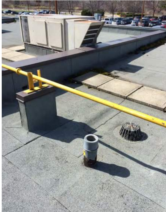
Photograph 27: Typical potential lead-containing roof vent pipe.
