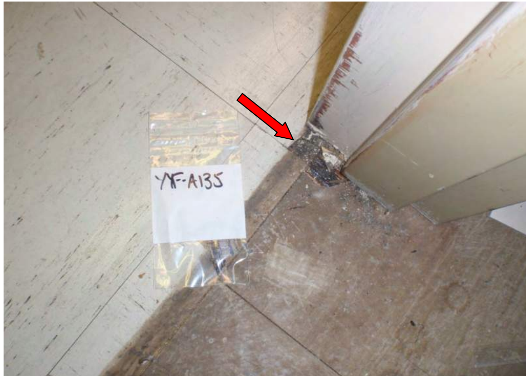
Photograph 49: Asbestos-containing off-white vinyl floor tile in Room 117 ( Sample A135 ).
