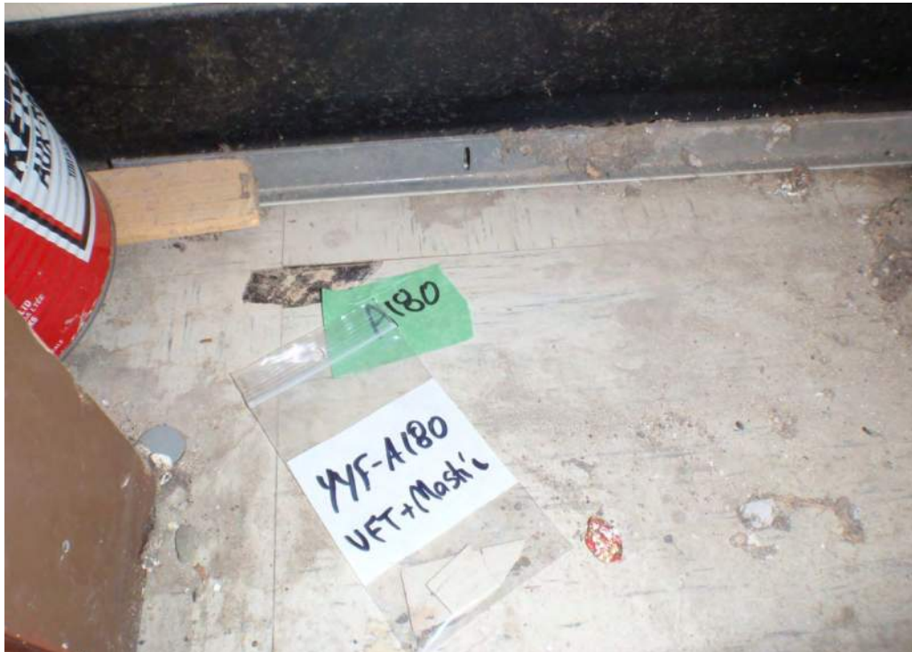
Photograph 55: Asbestos-containing grey vinyl floor tile located inside wall compartment in Room 106B (Sample A180).
