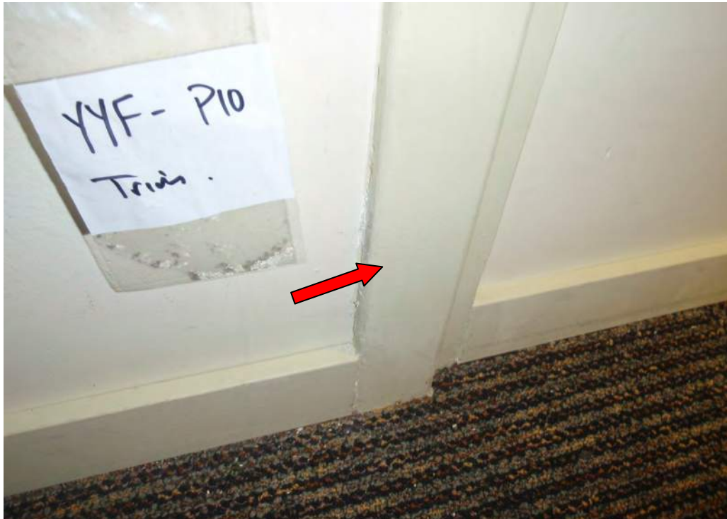
Photograph 65: Lead-based beige wall trim in Room 120 ( Sample P10 ).
