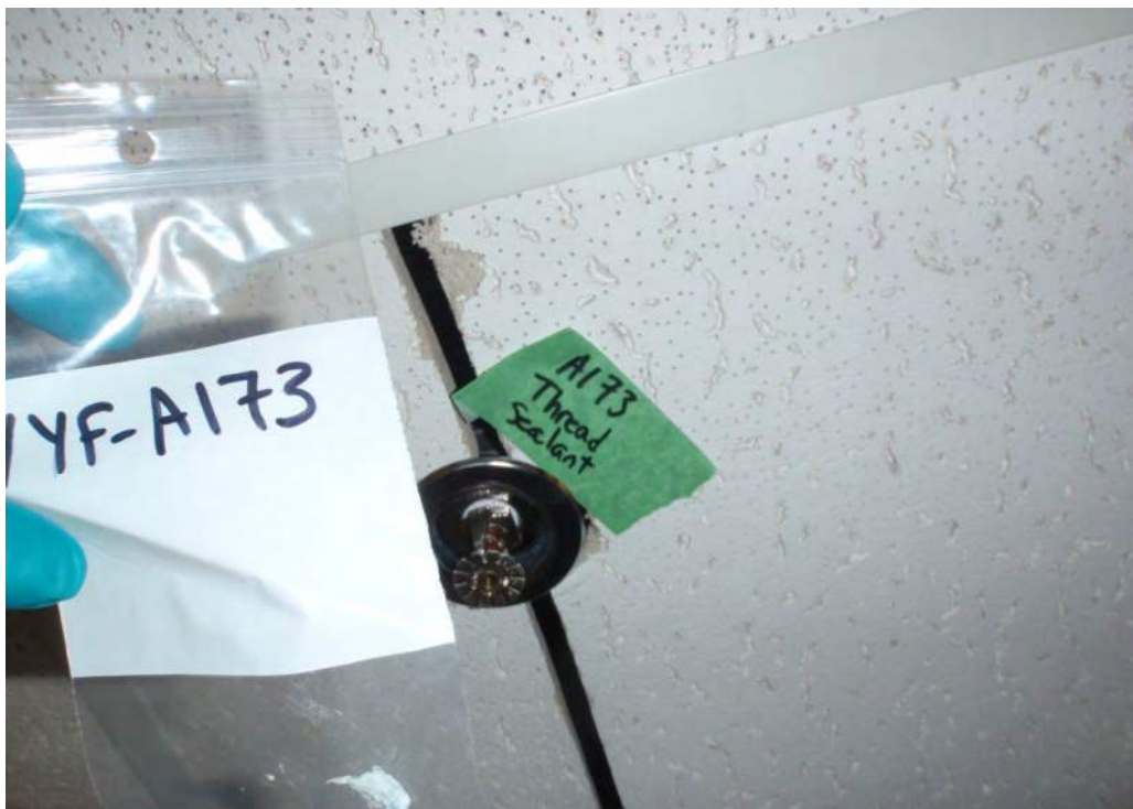
Photograph 54: Asbestos-containing pipe thread sealant on fire line in Room 143 ( Sample A173 ).
