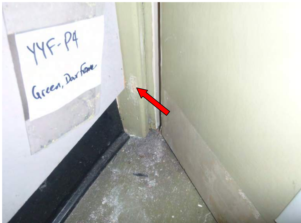
Photograph 62: Lead-based green paint on door frame in Room 127 ( Sample P4 ).
