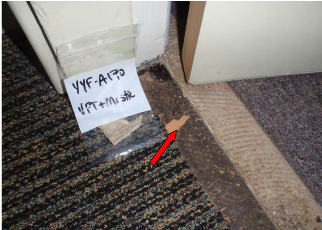
Photograph 53: Asbestos-containing tan vinyl floor tile in Room 119 ( Sample A170 ).
