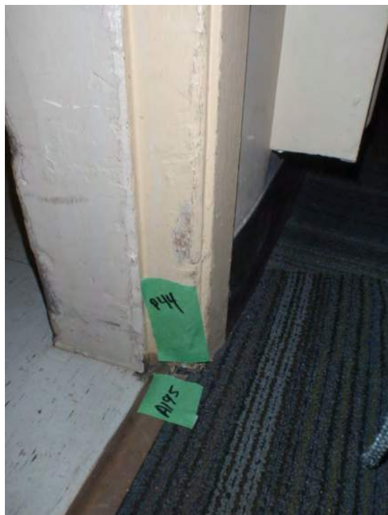
Photograph 86: Lead-based yellow paint on door frame of Room 112 ( Sample P44 ).
