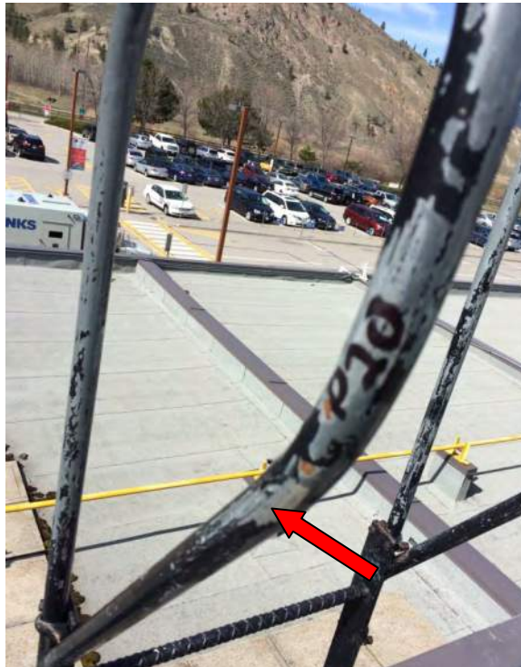
Photograph 71: Lead-based black paint on ladder to raised portion of roof ( Sample P20 ).
