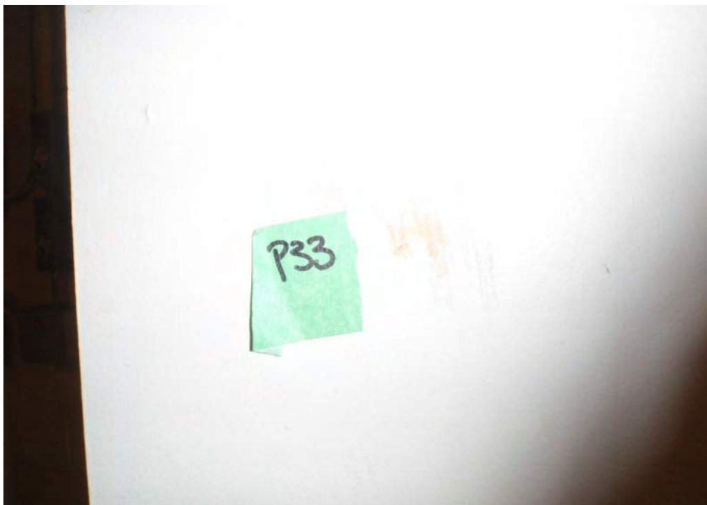
Photograph 80: Lead-based beige paint on walls of Room 137 ( Sample P33 ).
