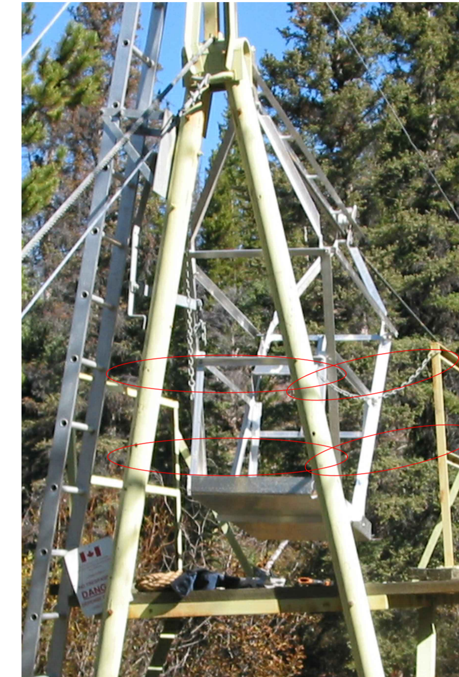
PHOTO 6: HOME SIDE A-FRAME SAFETY BAR - INSTALL A-FRAME SAFETY BAR BETWEEN A-FRAME LEGS AND SIDE GUARDRAIL
