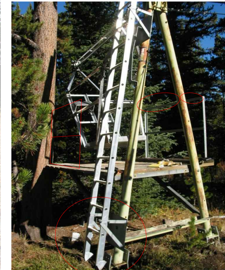
PHOTO 3: HOME SIDE LADDER - INSTALL PLATFORM RAILING ON SIDE INDICATED, SAFETY RAIL BETWEEN A-FRAME LEGS AND BETWEEN A-FRAME AND GUARDRAIL. RE-INSTALL LADDER SO THAT BOTTOM RUNG IS WITHIN 14" OFF THE GROUND
