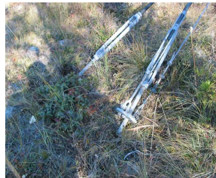
PHOTO 4: HOME SIDE ANCHOR CABLE TERMINATION AND TURNBUCKLE
