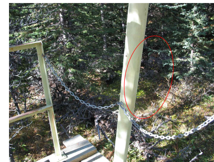
PHOTO 9: FAR SIDE A-FRAME LEG - INSTALL SAFETY RAIL BETWEEN A-FRAME LEGS AND BETWEEN SIDE RAIL AND A-FRAME LEG
