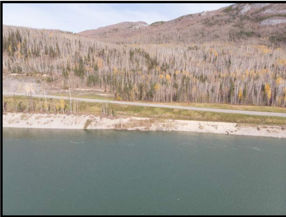
Photograph 3: Central part of slope failure of Liard River bank
