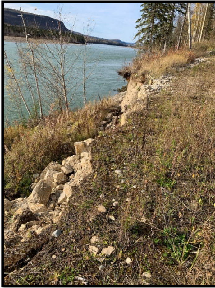
Photograph 9: Looking north along the northern extent of the bank failure
