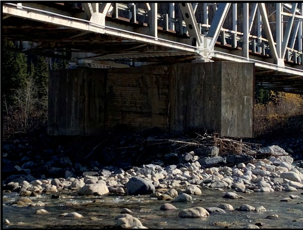
Photograph 4: Central pier that will require erosion repairs.
