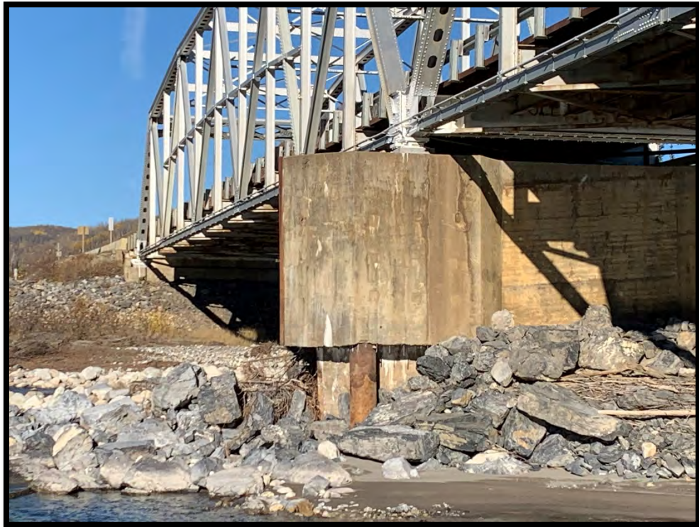
Photograph 1: Exposed pier on Racing River bridge.
