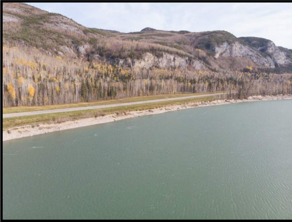
Photograph 2: Southern part of slope failure of Liard River bank
