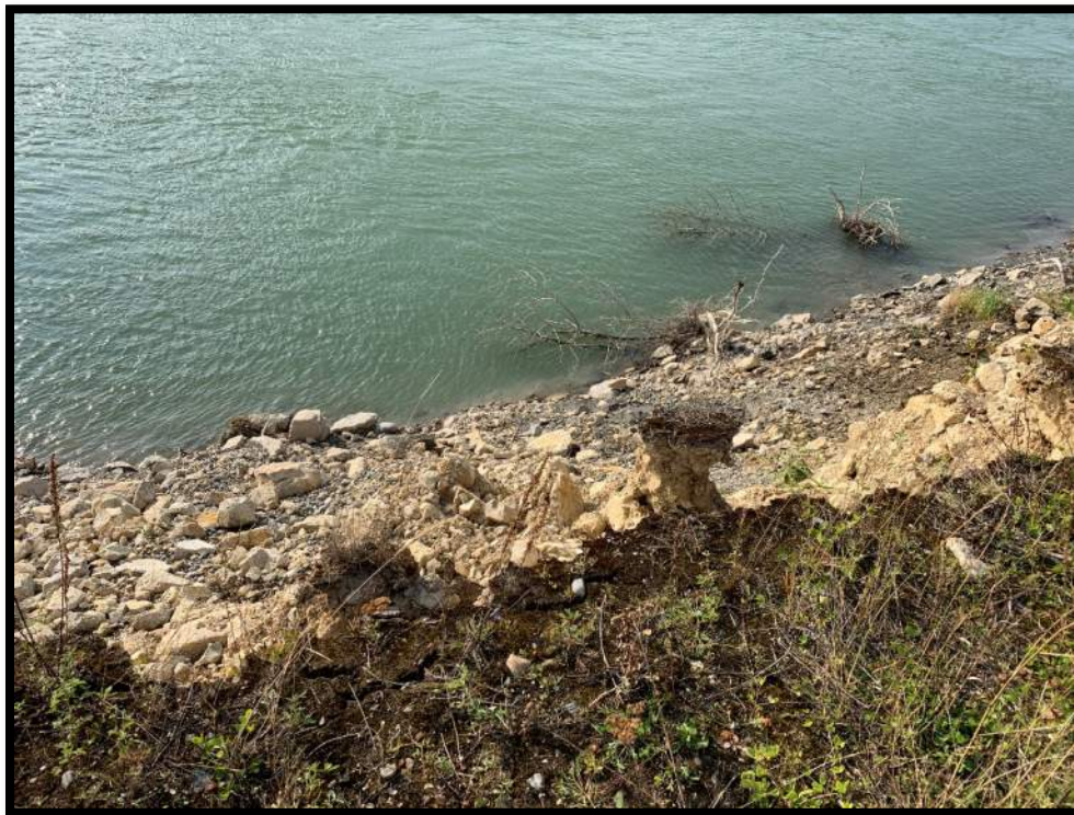
Photograph 8: Looking downslope to Liard River from the top of the failing bank
