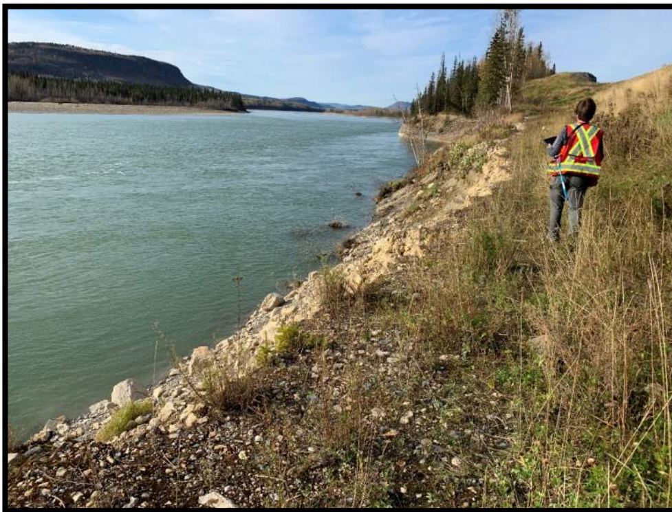
Photograph 5: Looking north along top of bank of Liard River in bank failure area
