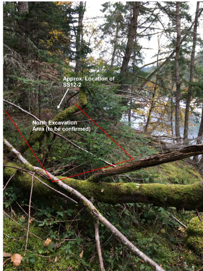
Photograph 15: North excavation area, looking north (excavation extent to be confirmed by contractor prior to start of work).
