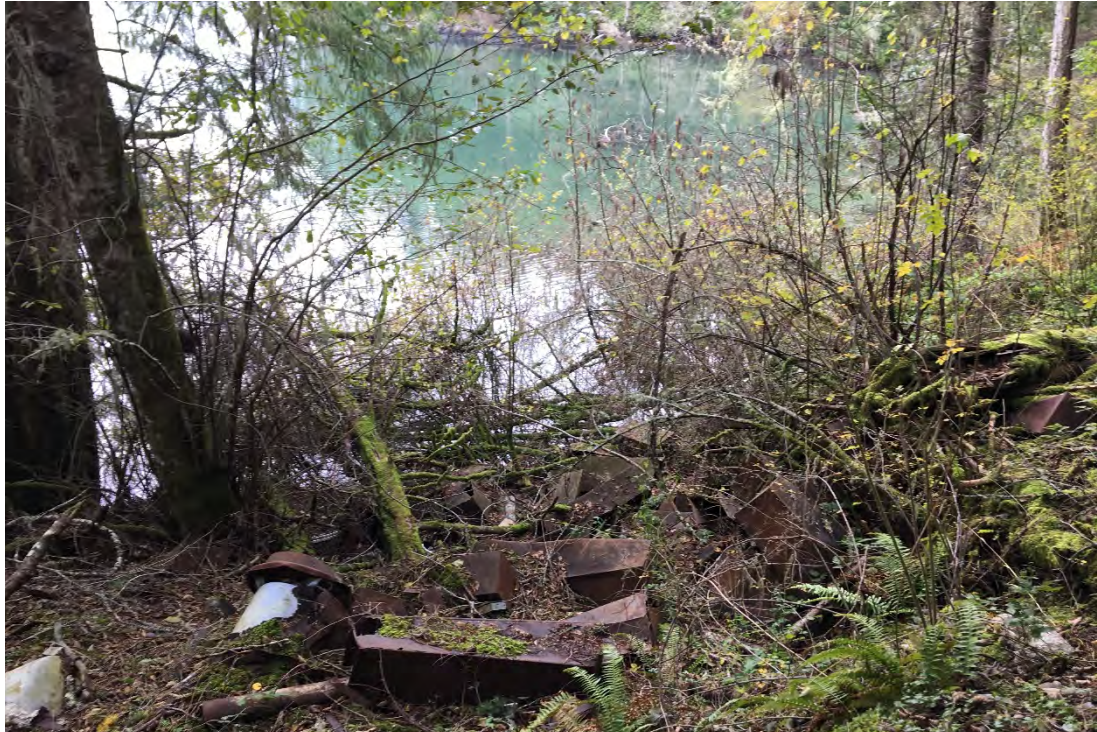
Photograph 7: East edge of southern excavation showing non-contaminated debris (excavation extent to be confirmed by contractor prior to start of work).
