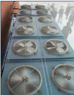
Rooftop cooling unit compressors
