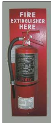
Portable fire extinguisher
