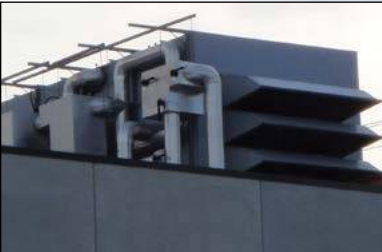
Large rooftop air conditioner
