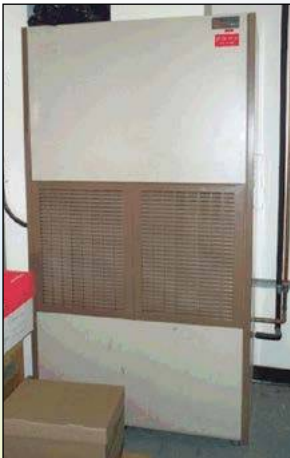
Air conditioning evaporator
