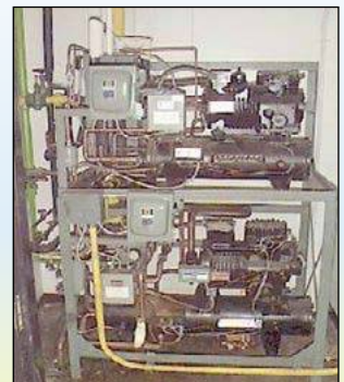
Walk-in refrigerator compressors
