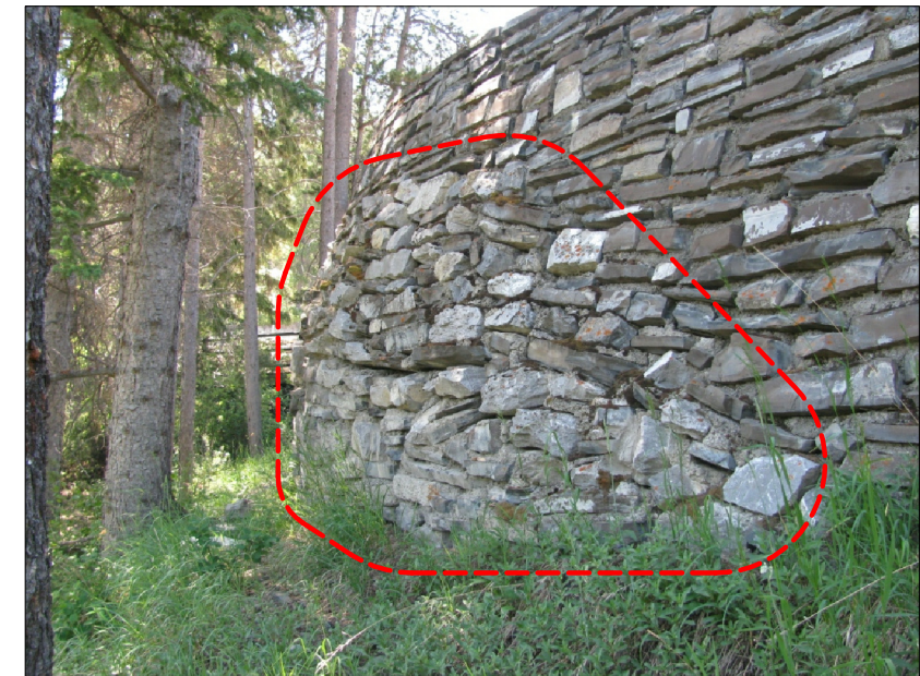
DET. 6/S2 - PORTION OF CURVILINEAR LEG OF STONE RET. WALL. DASHED LINE SHOWS 'BULGE' IN STONE RET. WALL, INDICATIVE OF OVERLOAD.
