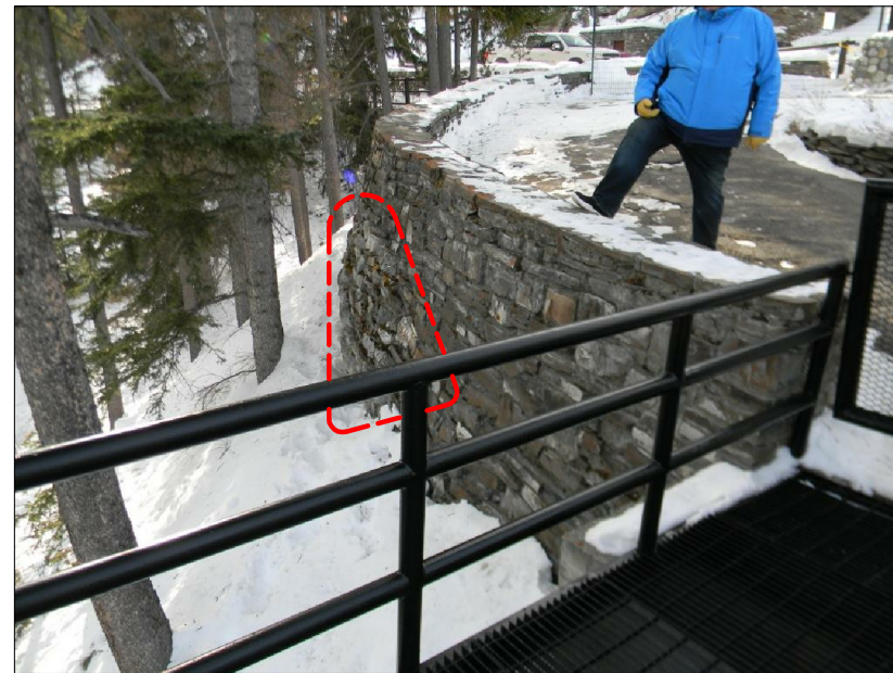
DET. 5/S2 - NORTHERN '3RD' OF CURVILINEAR LEG OF STONE RET. WALL (LOOKING SOUTHWEST). DASHED LINE SHOWS 'BULGE' IN STONE RET. WALL, INDICATIVE OF OVERLOAD.
