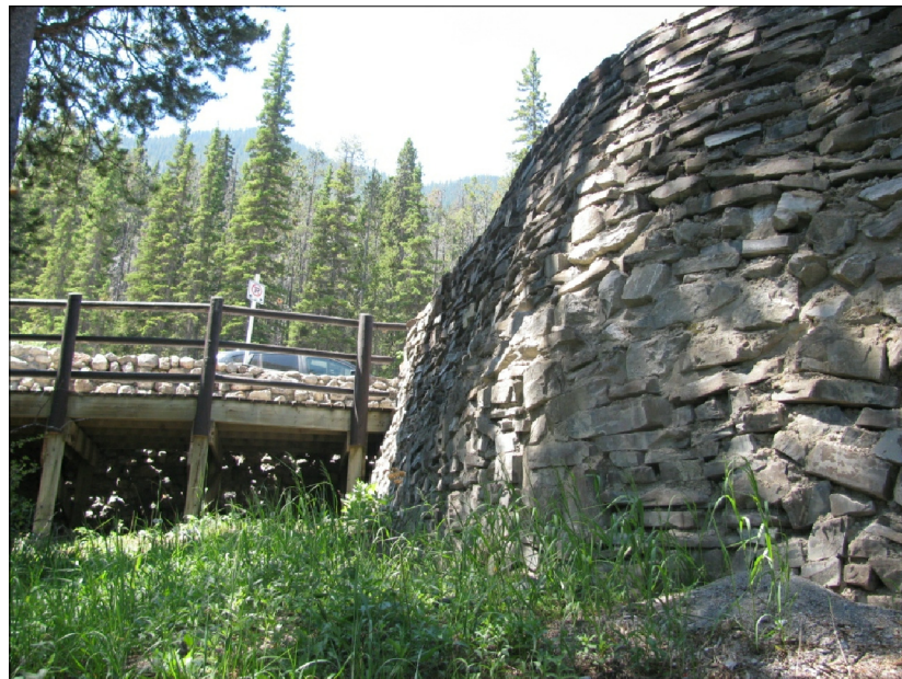
DET. 4/S2 - WESTERN '3RD' OF CURVILINEAR LEG OF STONE RET. WALL (LOOKING WEST).
