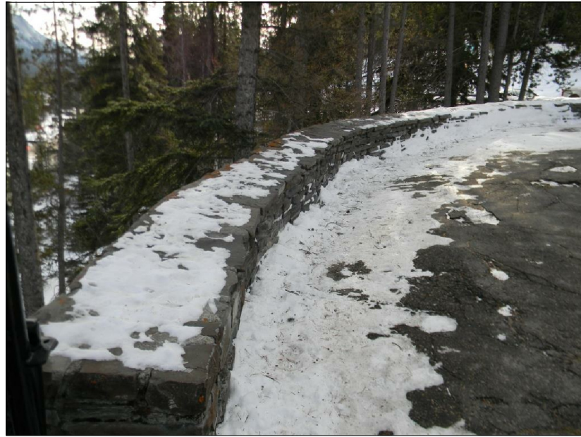
DET. 1/S2 - UPPER LEVEL OF CURVILINEAR LEG OF STONE RET. WALL (LOOKING SOUTH).
