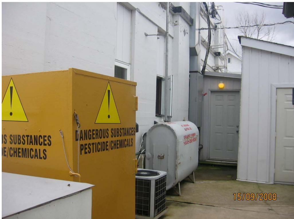
Photograph 6: View of 935-L fuel oil AST.
