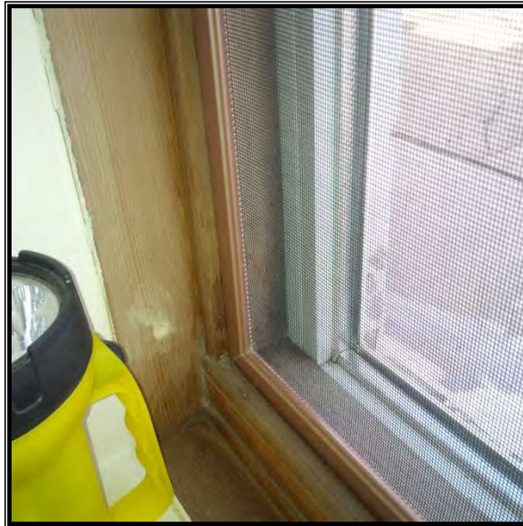
Interior caulking not present at interior window frames, Cabin #1, Galley House
