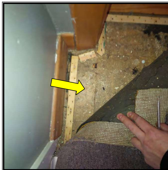
Photo 6 Non-asbestos vinyl sheet flooring present below carpet (samples 0003A-C), Entranceway, Office House
