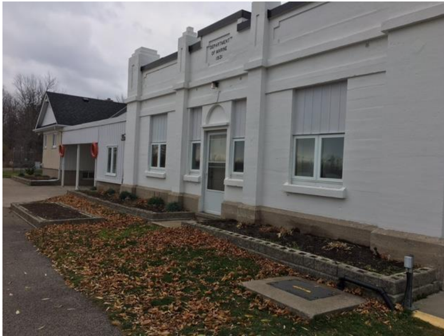
Photo 3: View of the exterior of the Galley House and Office House, where asbestos containing caulking on the main floor windows and basement windows were observed. All caulking was observed to be in good condition at the time of the assessment.
