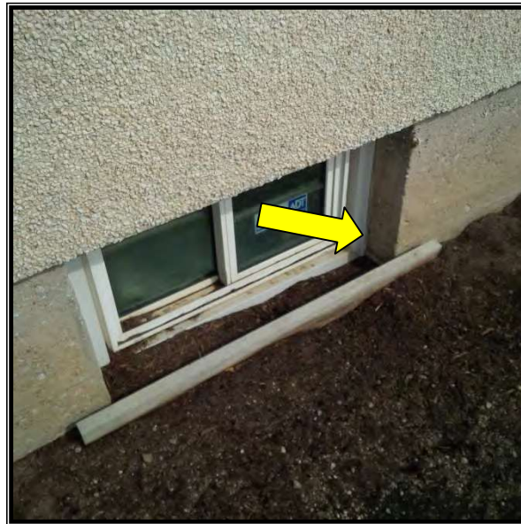
Photo 9 Asbestos-containing grey caulking (sample 0006A), Exterior, Office House
