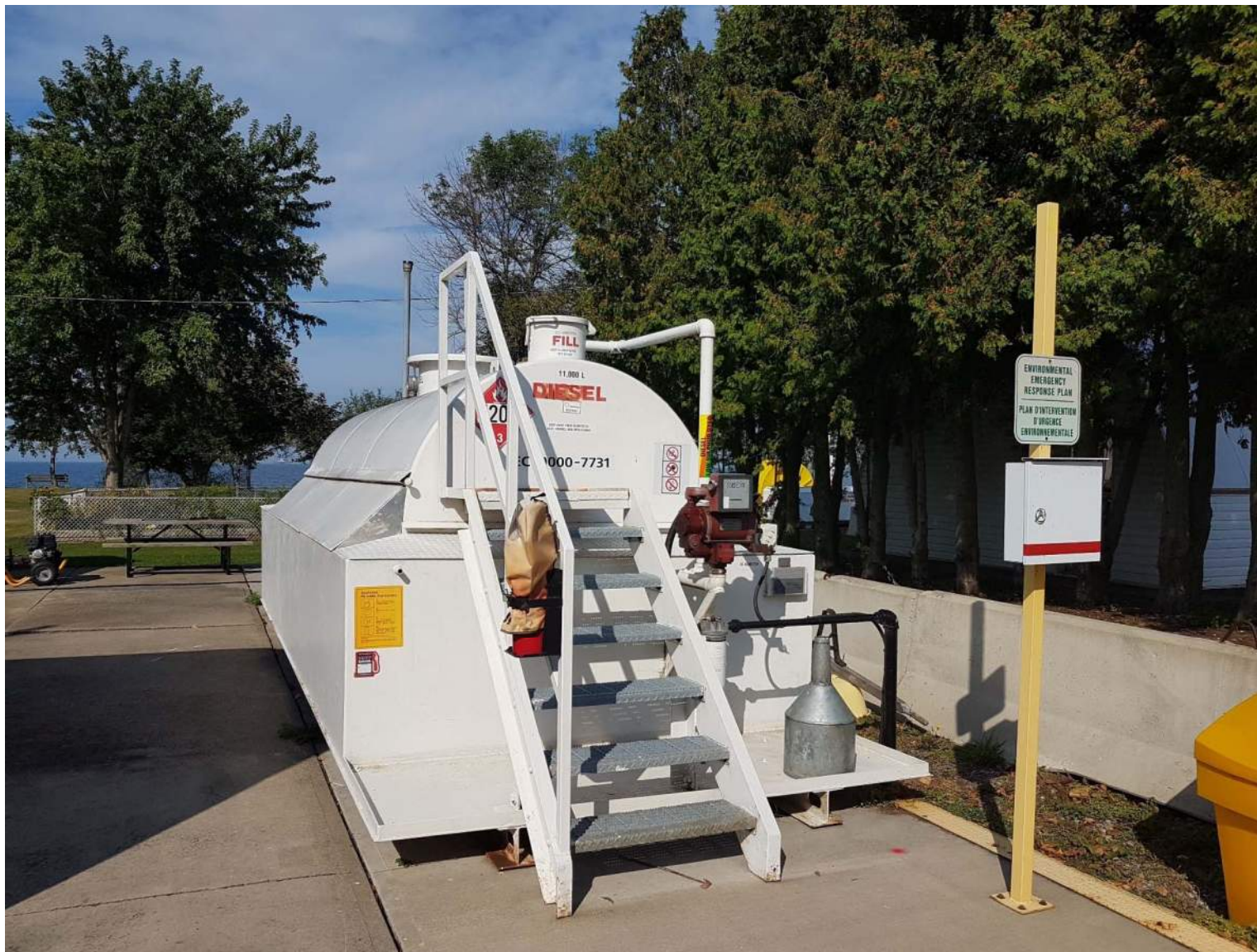
Figure 3-15 Diesel Storage Tank
