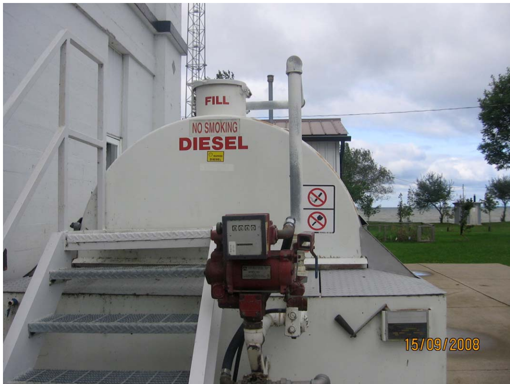
Photograph 9: View of 11,000-L diesel AST.
