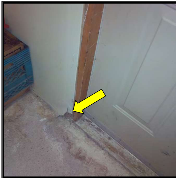
Photo 14 Mould present on water-damaged drywall (sample B-001), Generator Room, Galley House
