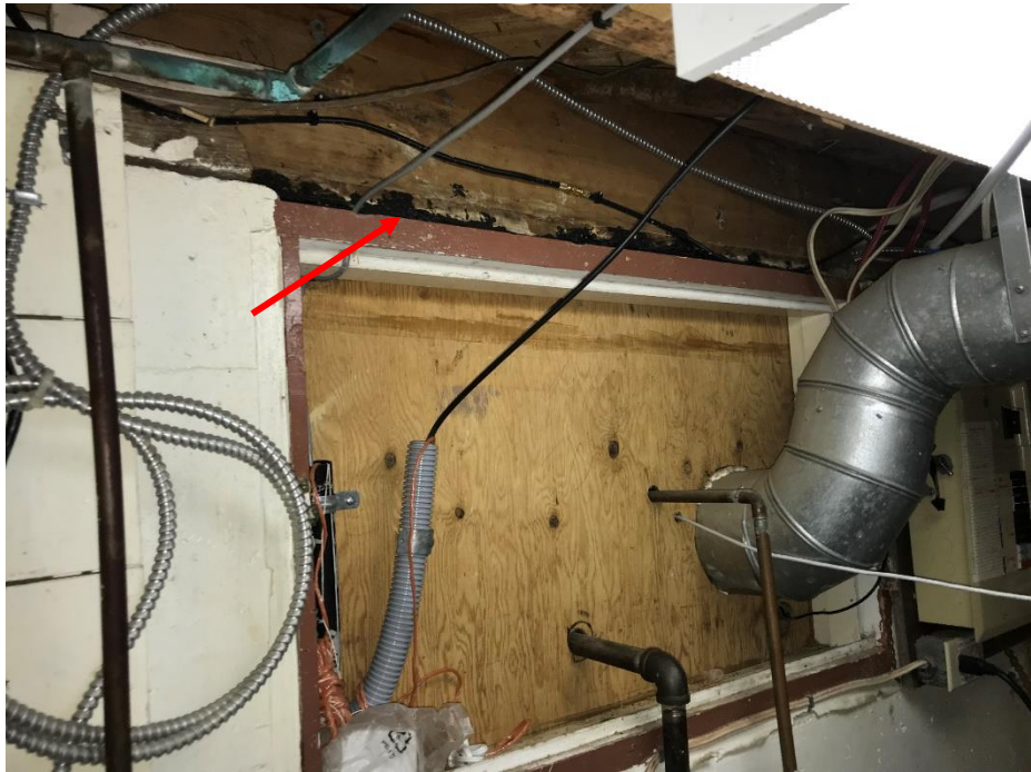
Photo 5: View of Tar on wall in basement boiler room of the Office House.
