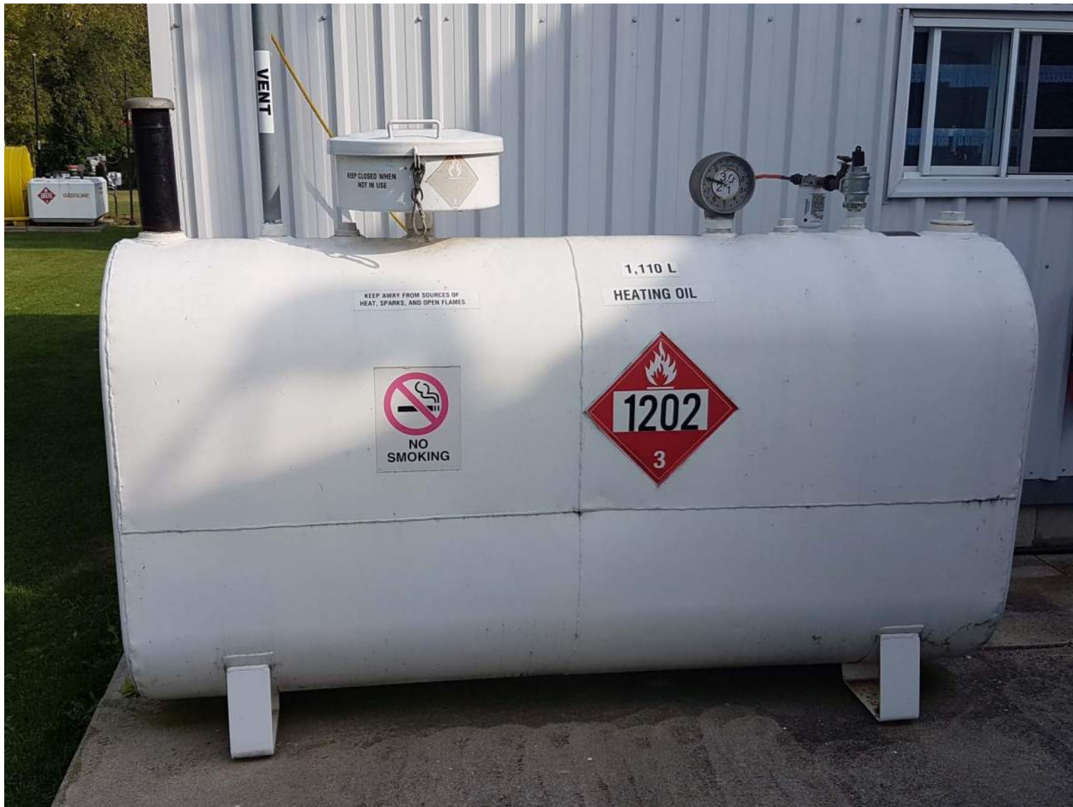
Figure 3-12 Heating Oil Tank
