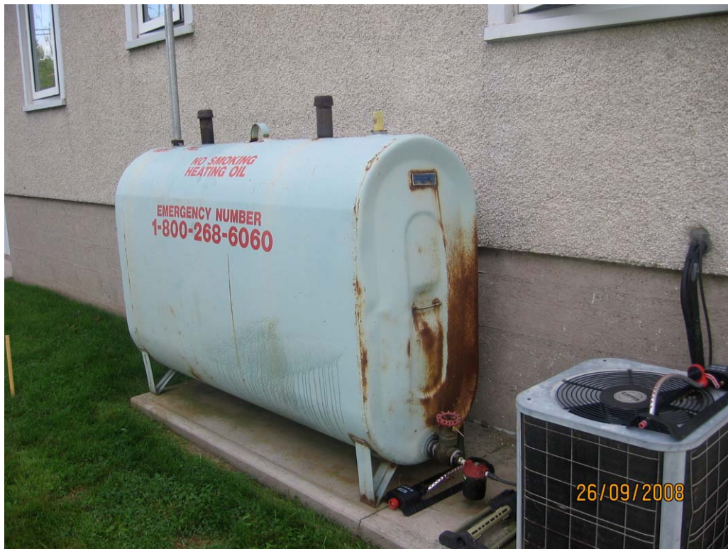
Photograph 21: 1,100-L fuel oil AST.
