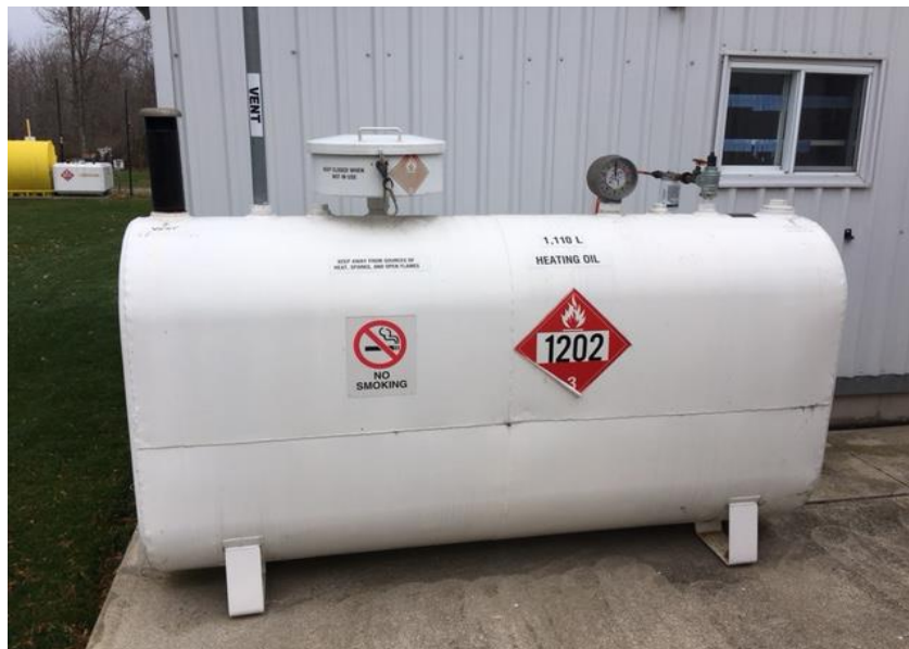
Photo 2: View of an exterior fuel storage tank, observed on the property
