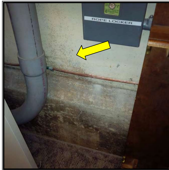
Photo 15 Surface mould present on concrete wall (sample B-002), Breaker Closet, Galley House
