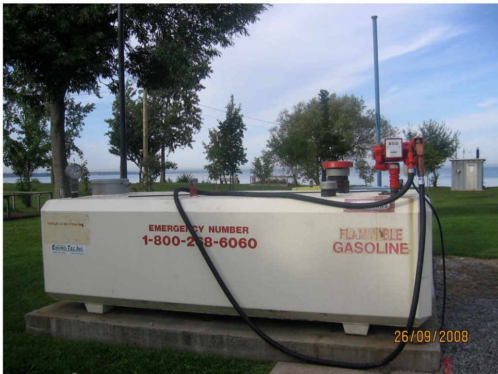
Photograph 20: 1,900L gasoline AST-looking west.
