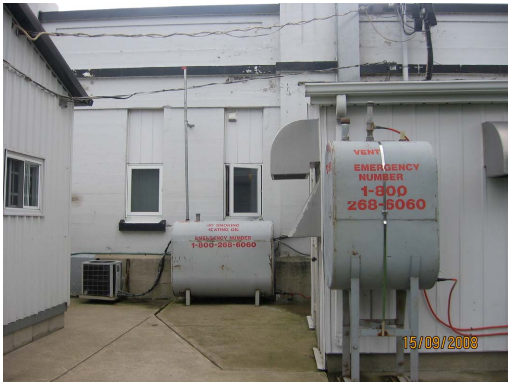
Photograph 7: View of 935-L fuel oil AST and 910-L diesel AST.
