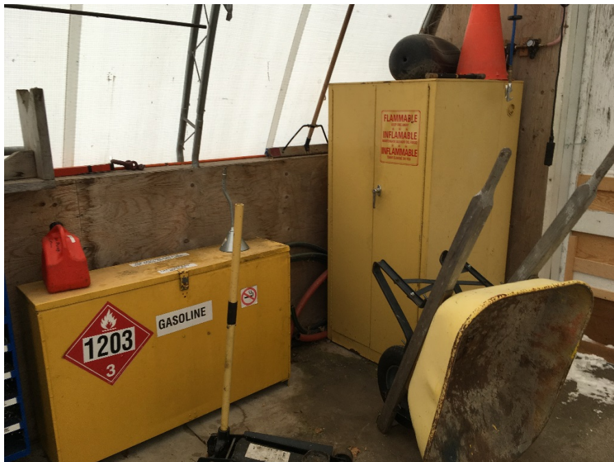
Photograph 10: Hazardous good storage cabinets located within storage shed #1.
