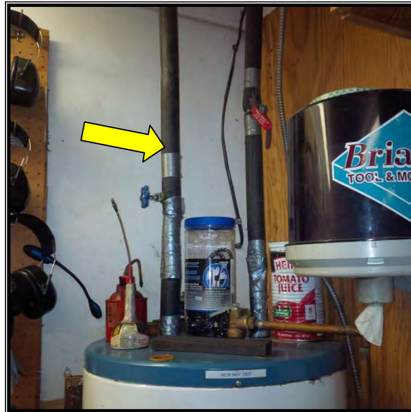
Photo 1 Non-asbestos foam insulation on domestic hot water piping, Connecting Garage
