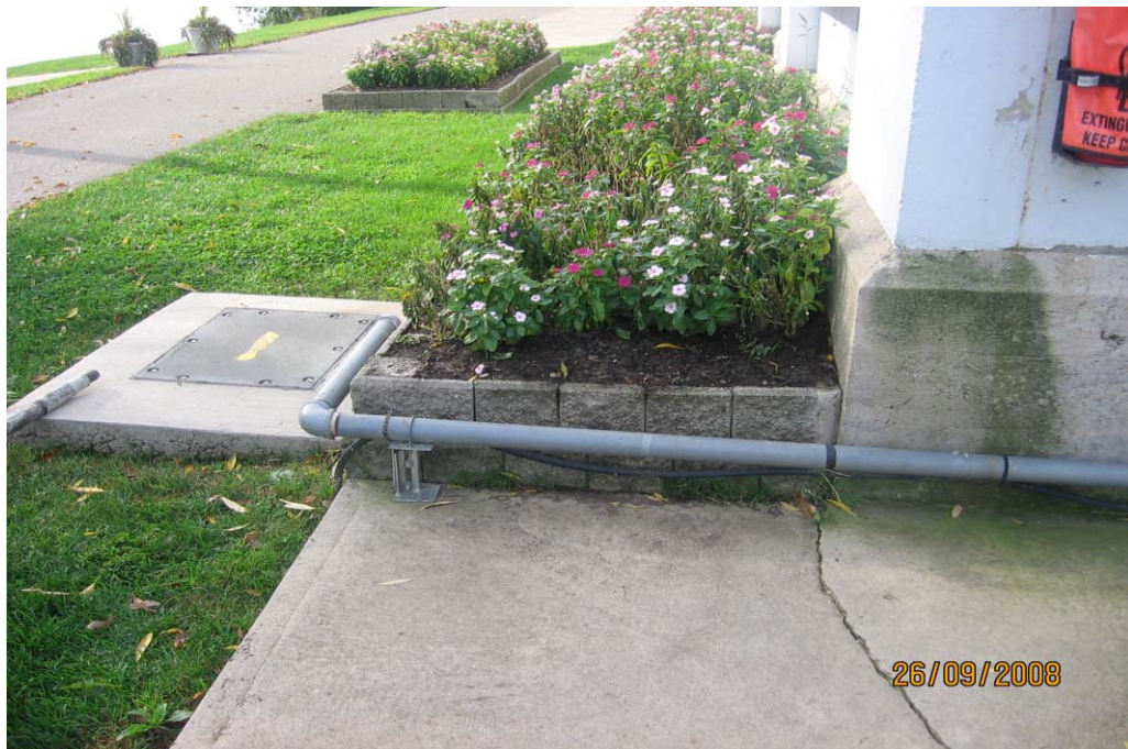
Photograph 22: Piping from 11,000-L diesel AST to sump.
