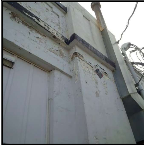
Photo 13 Flaking lead-containing paint on concrete walls (L006 to L009), Exterior, Galley House
