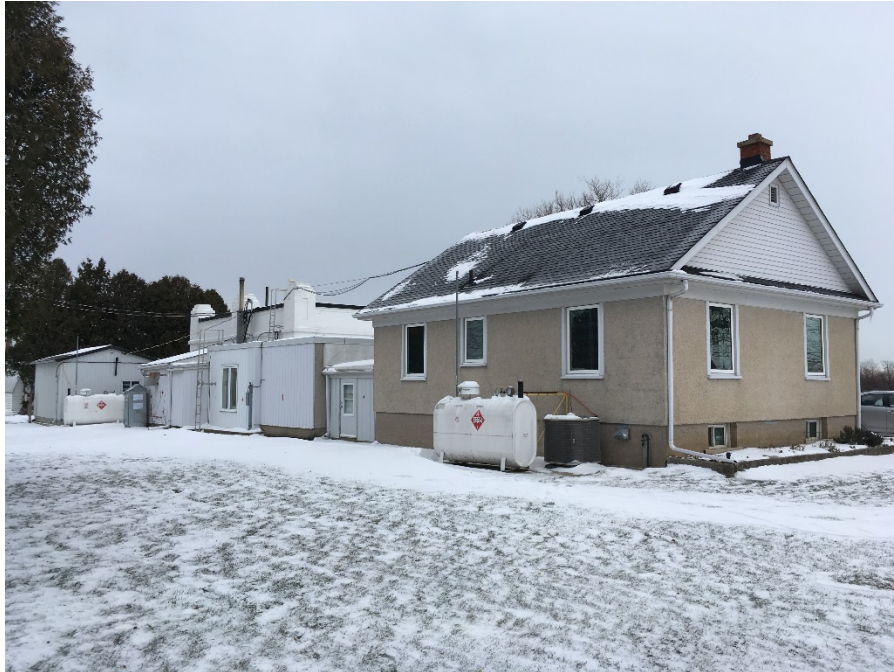
Photograph 5: Fuel oil ASTs (1,100 L each) and pad mounted air conditioning unit located along the western exterior wall of the Main building.
