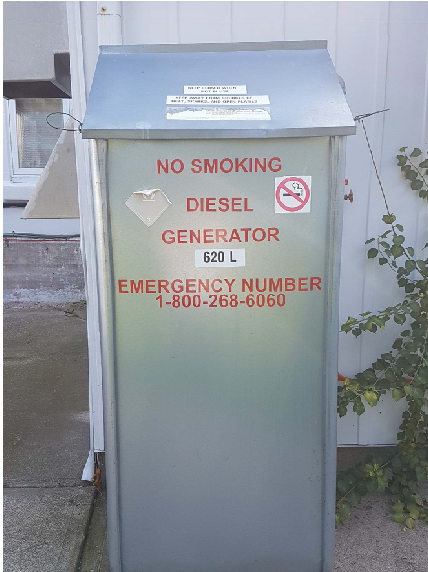
Figure 3-13 Emergency Diesel Generator
