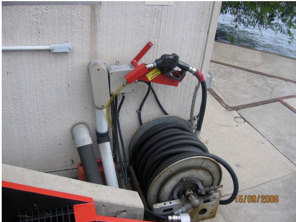
Photograph 3: View of fuel dispenser at Ready building.
