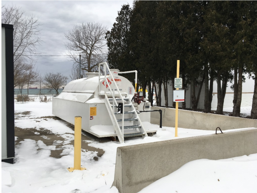
Photograph 7: Diesel AST (11,000 L) located to the north of the Main building.
