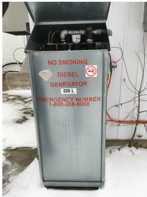
Paragraph 6: Diesel AST (600 L) located along the northwestern exterior wall of the Main building.
