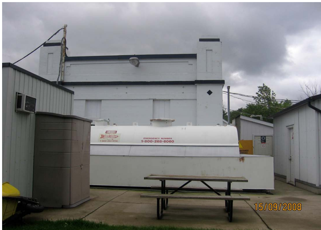
Photograph 8: View of 11,000-L diesel AST.
