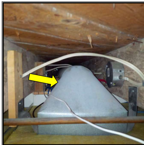
Photo 2 Uninsulated ductwork, Basement of Office House
