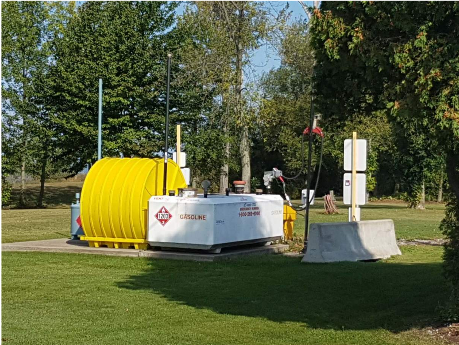
Figure 3-14 Gasoline and Waste Oil Storage Tanks
