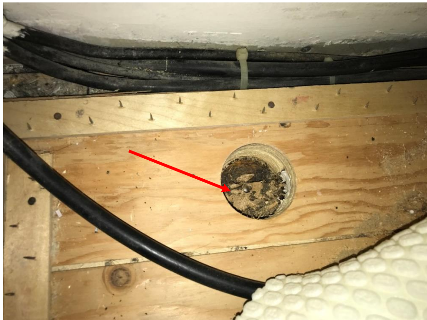
Photo 4: View of black mastic applied to plywood subfloor in living room of Galley House. This mastic is assumed present beneath plywood sheeting throughout all areas of the Galley House, unless proven otherwise.
