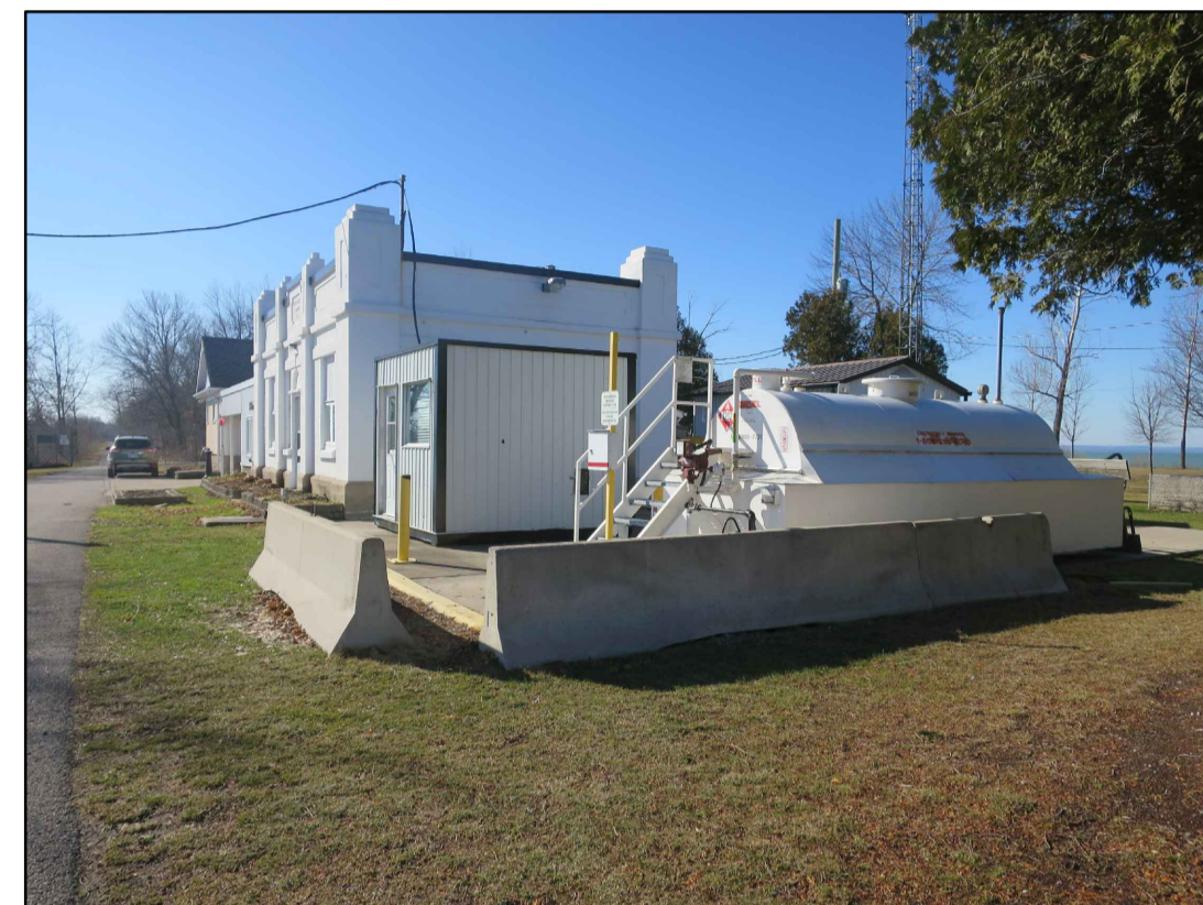
FIG. 5 - EX. DIESEL TANKS TO REMAIN. PROTECT IN PLACE AND MAINTAIN ACCESS THROUGHOUT CONSTRUCTION.
