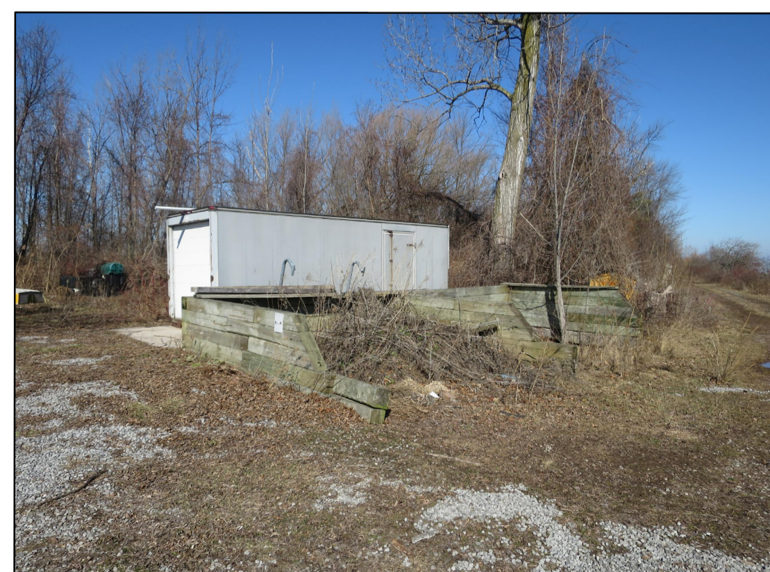
FIG. 11 - EX. STORAGE CONTAINER TO BE REMOVED FROM SITE AND EX. OPEN WOOD GARDEN STRUCTURE TO BE DEMOLISHED.
