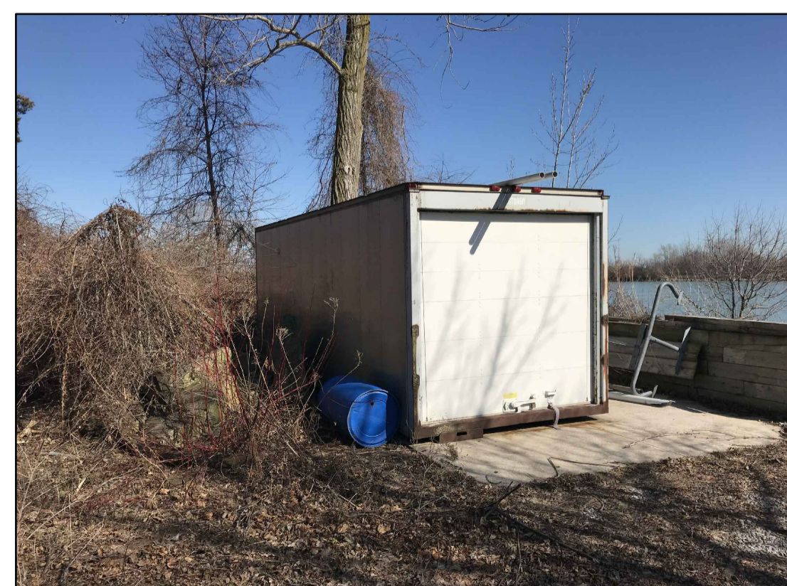
FIG. 12 - EX. STORAGE CONTAINER TO BE REMOVED FROM SITE AND EXISTING CONCRETE SLAB TO BE DEMOLISHED
