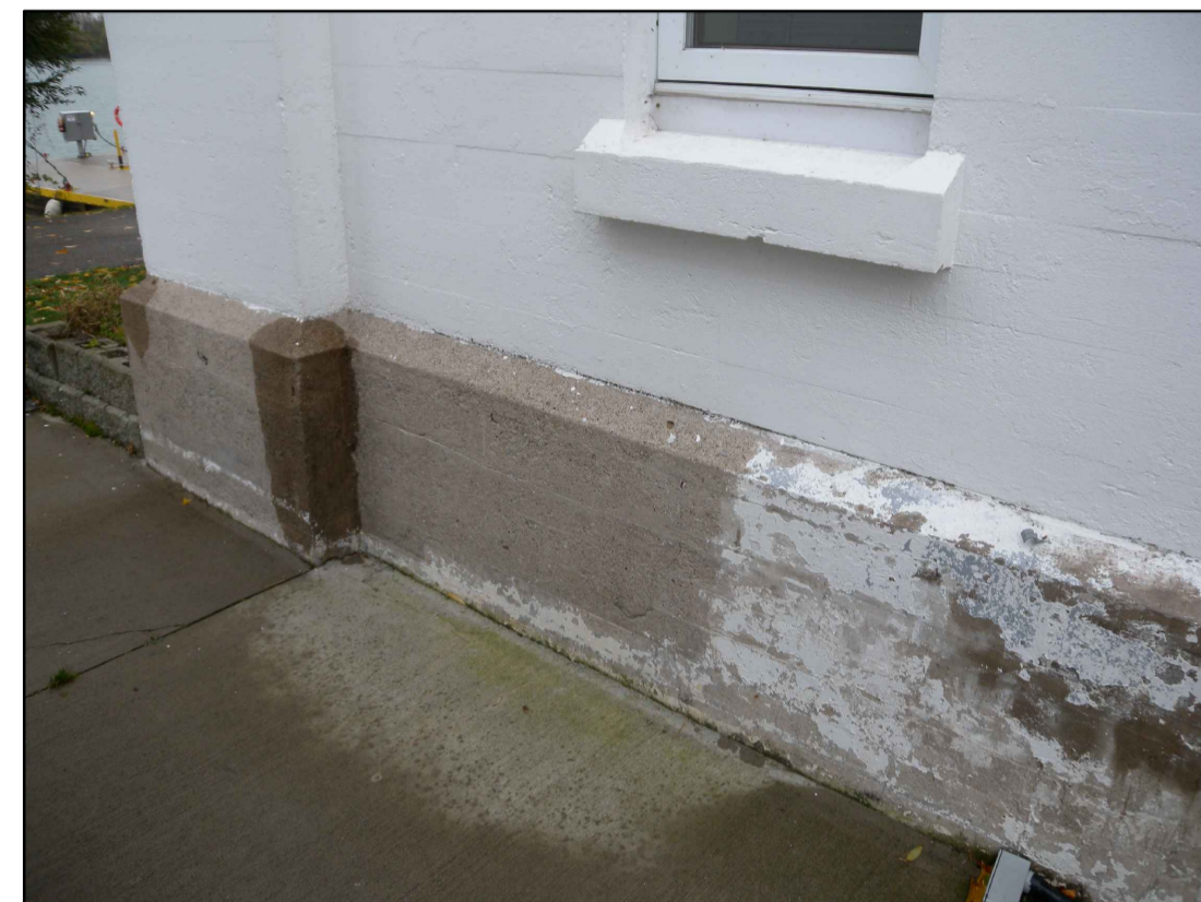
FIG. 6 - EX. PLINTH CONCRETE TO BE REPAIRED (TYPICAL)
