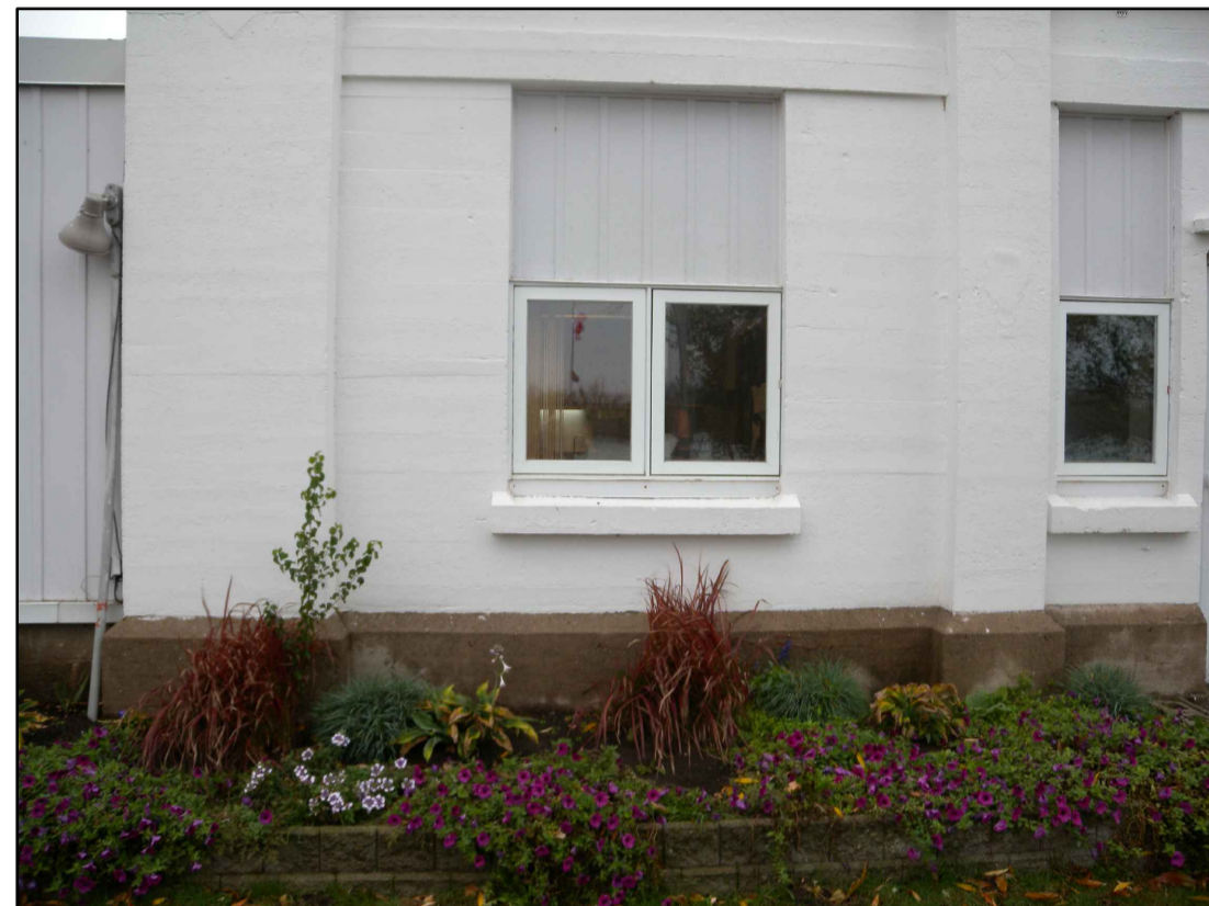
FIG. 5 - TYPICAL EXISTING WINDOW AND PANEL TO BE REMOVED AND NEW WINDOW TO BE INSTALLED IN EXISTING OPENING
