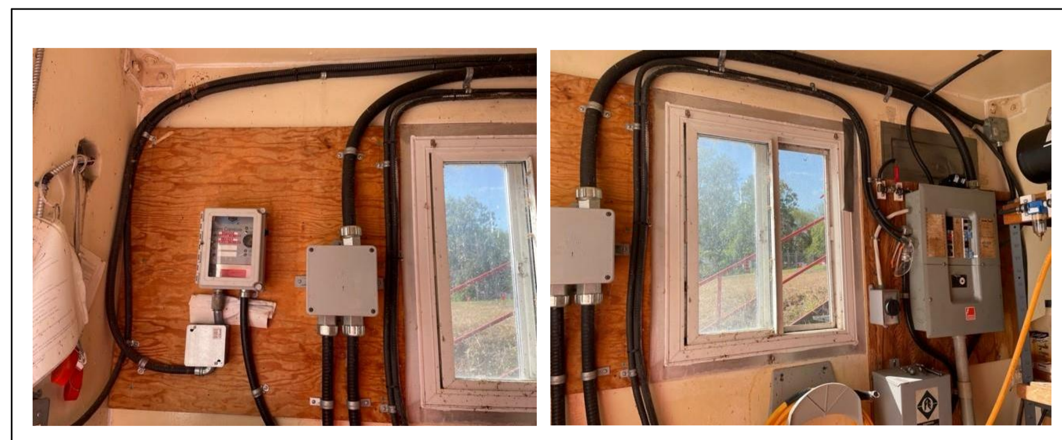
6 EXISTING POWER DISTRIBUTION IN READY ROOM HUT REMAIN AS CONNECTED E901 N.T.S.
