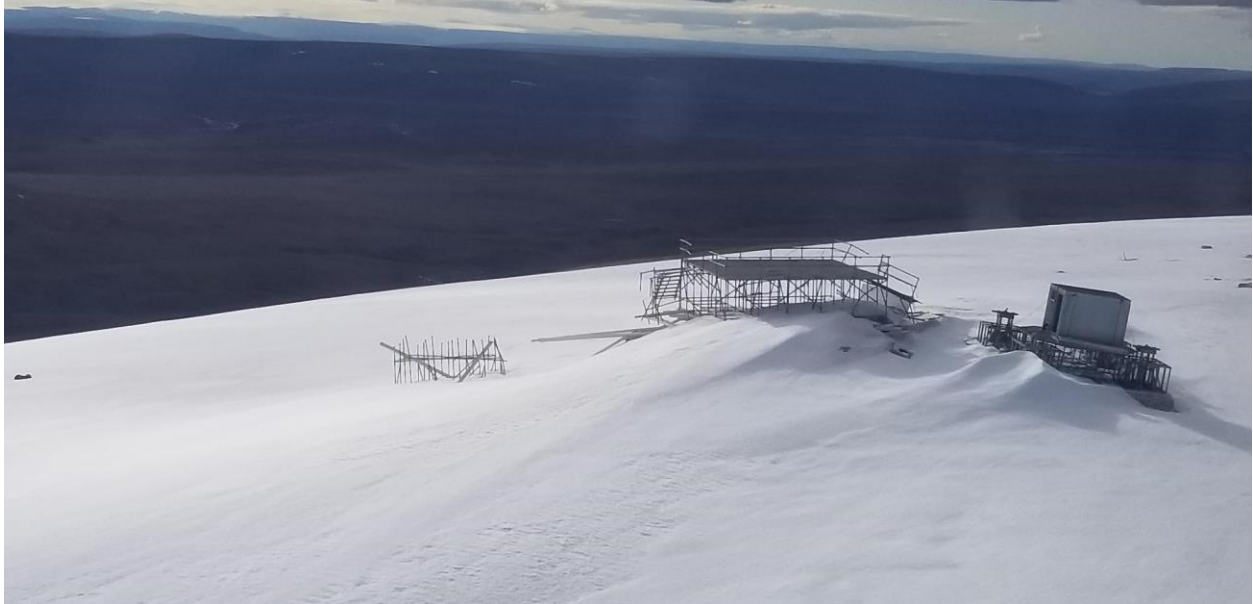
Figure #62A: 4 August, 2021 - Mount Arthur Platform Failure into 3 Separate Sections
