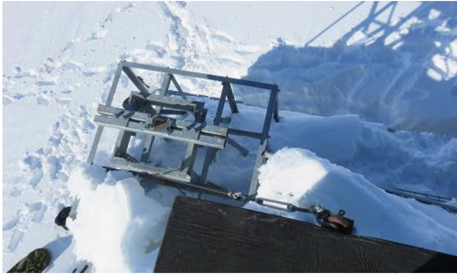
Figure #74: Antenna tower ballast boxes
