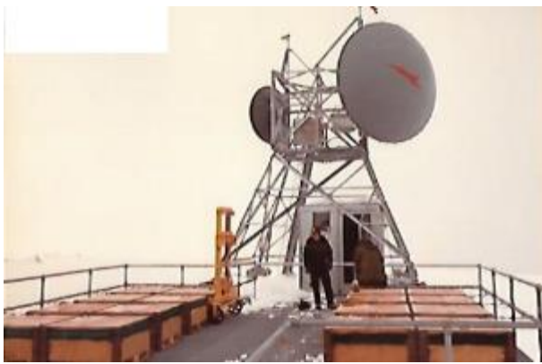
Figure #7: Mount Arthur microwave repeater site (July 1982)
