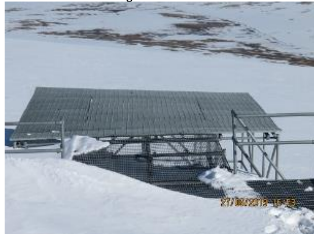
Figure #27: Close up view of deformed loading pad
