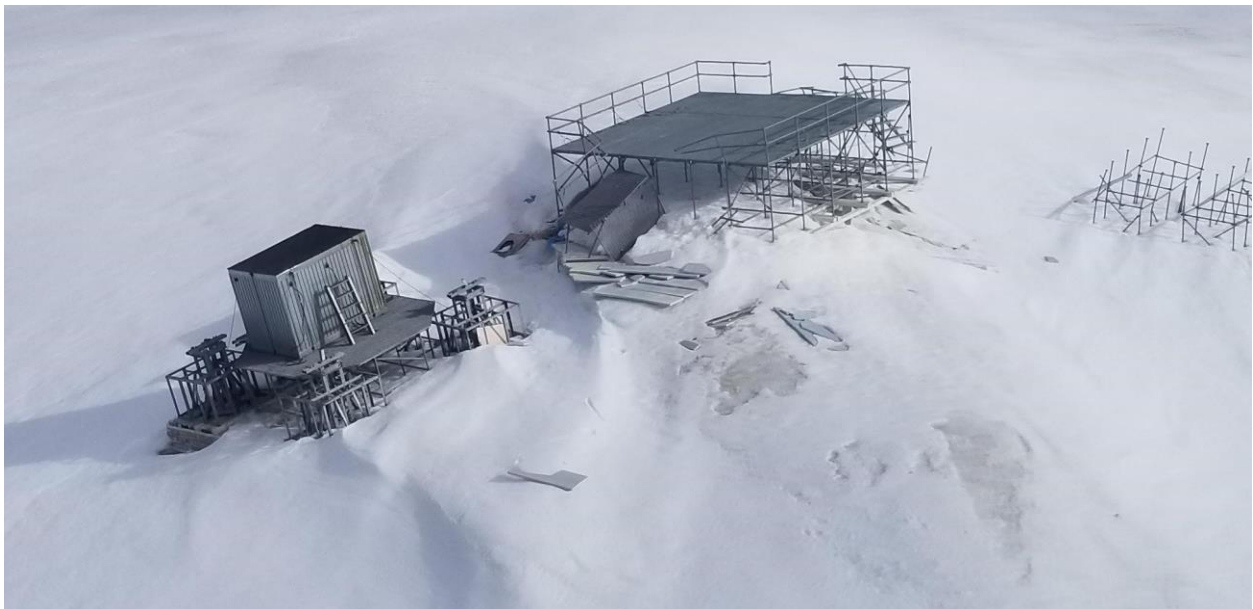
Figure #62B: 4 August, 2021 - Mount Arthur Platform Failure into 3 Separate Sections
