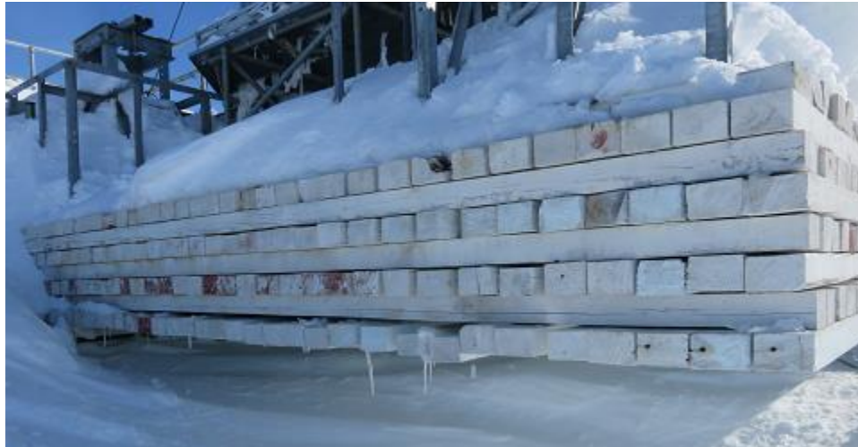
Figure #68: Layers of timber supporting platform Seven (7) layers under full platform plus one additional layer under tower ballast boxes
