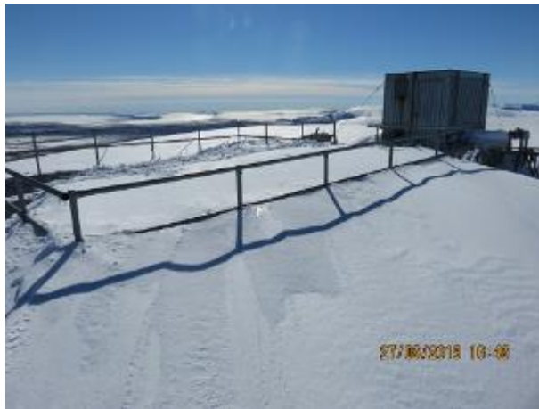
Figure #18: View of existing platform looking South. North-East section of platform buried in snow
