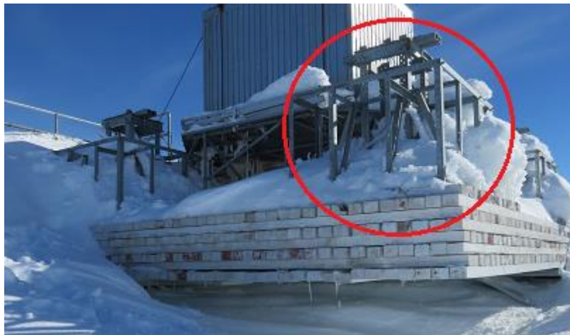
Figure #73: Antenna tower ballast boxes
