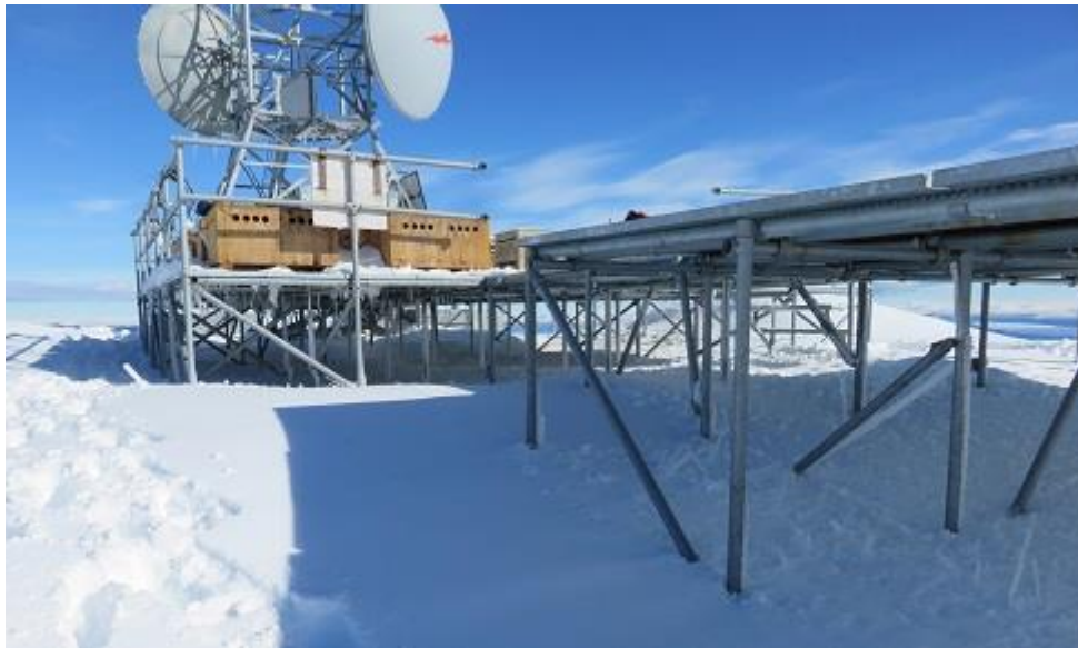
Figure #69: Steel lattice platform (Yankee Repeater Site)
