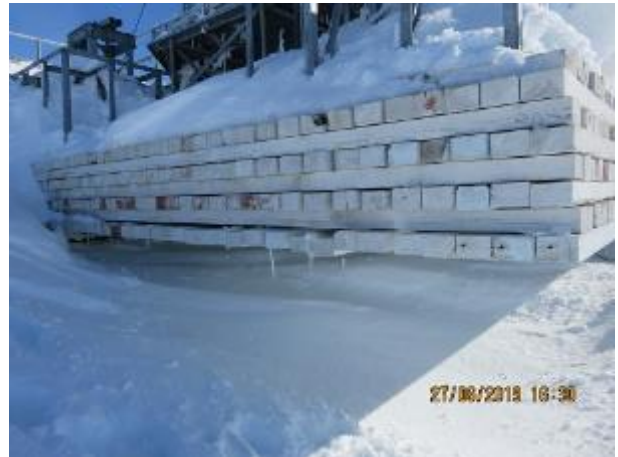
Figure #37: Closer view of wood framework separation
