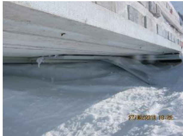
Figure #39: View of two (2) layers of Styrofoam insulation (total 4") which was originally placed under the lumber structure foundation to prevent heat transfer to the ice surface. A significant amount of Styrofoam has disappeared and is assumed to be buried on the mountain.
