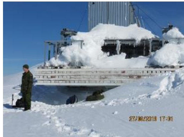
Figure #21: View of platform looking East – Wood beams (4"x6"x24') are not supported by previously existing ice layer. Melting ice has created a cavern under the platform.
