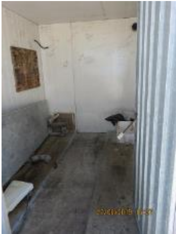
Figure #24: Inside abandoned equipment shelter
