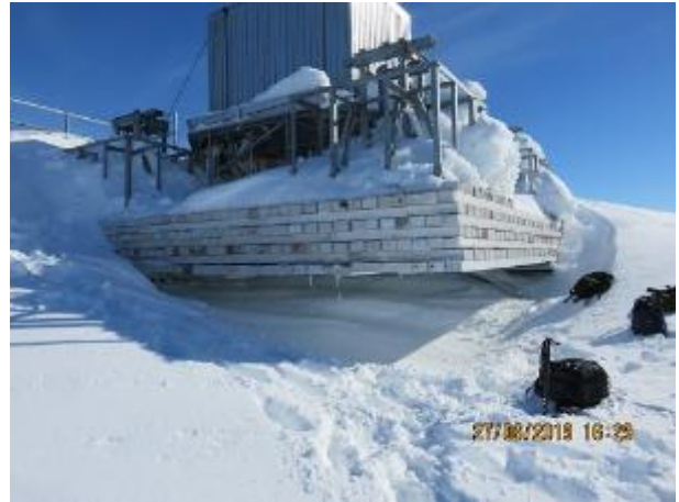
Figure #35: Bottom layer of wood framework is separating
