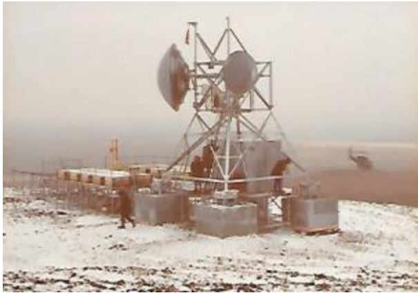
Figure #5: Typical microwave repeater site (July 1982)
