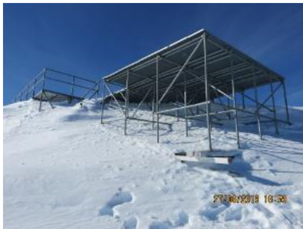
Figure #28: View of foundation failure at South-East section of loading pad
