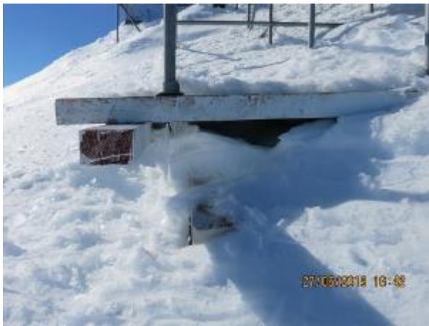
Figure #32: Close-up of foundation failure – Top layer of wood beams has separated from the remaining wood framework. Ice has melted under the wood framework causing settlement creating forces which separated the wood framework.
