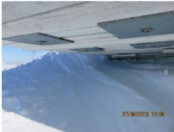
Figure #38: North-West corner of platform is fastened together with 1" dia. threaded steel rods, 18"x18"x3/4" steel plates and 2 1/2" x 2 1/2" x 1/2" steel washers (all galvanized). Four (4) rods are located at the corner section at 3 feet center to center. The fastening rods have prevented the cantilevered section of the platform from collapsing completely so far.
