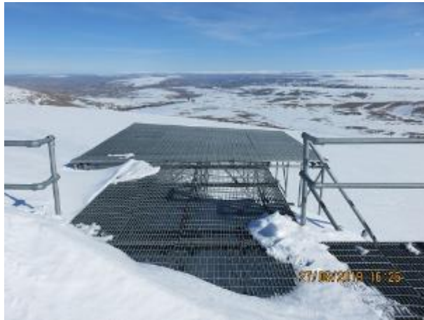
Figure #26: Closer view of loading pad – Significant platform twisting movement and settlement is clearly visible towards the South
