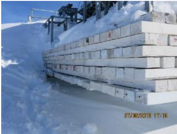
Figure #36: Closer view of wood framework separation
