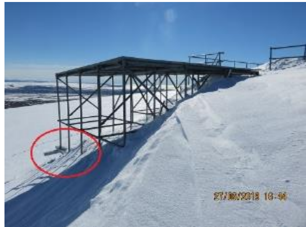
Figure #31: View looking South towards the foundation failure at South-East section of loading pad
