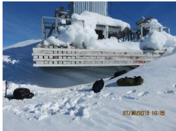
Figure #33: North-West corner of platform located directly under the equipment shelter. Lumber structure is now cantilevered (approx. 20 feet – 6 m) over section where ice has melted. Red circle identifies potential lumber failure point.
