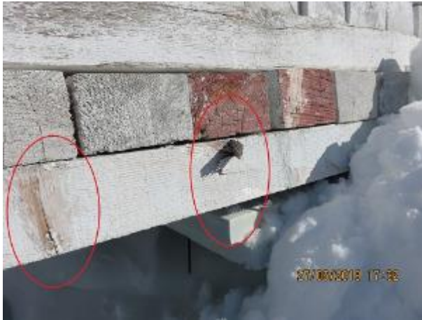
Figure #34: Visible signs of early lumber failure (failure lines are visible)
