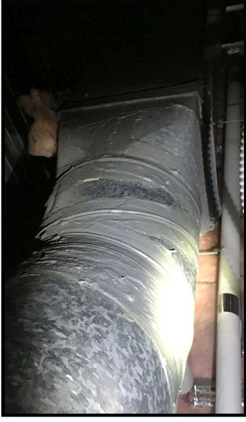
Locker Room Ceiling Plenum Ducting Grey Mastic
