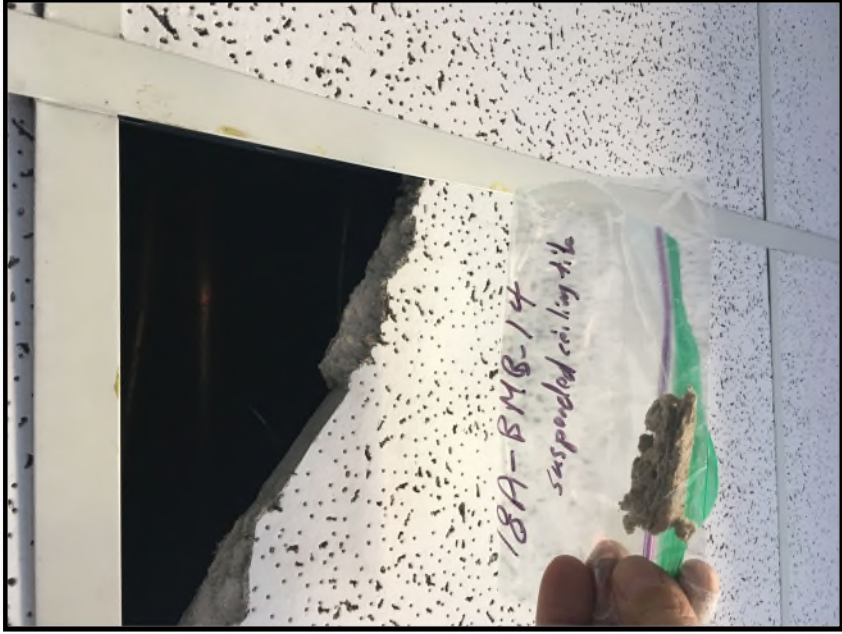
Corridor Ceiling, Suspended Ceiling Tile Sample 18A-BMB-14 was 'None Detected' for asbestos.
