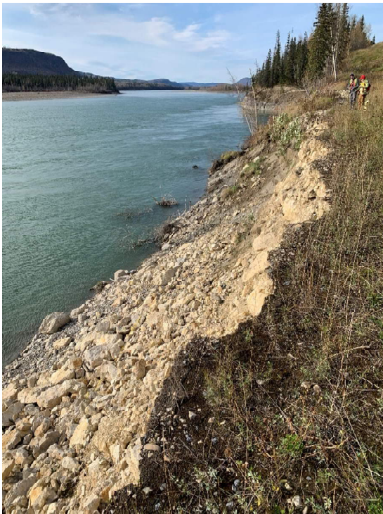
P08 - Eroded slope
