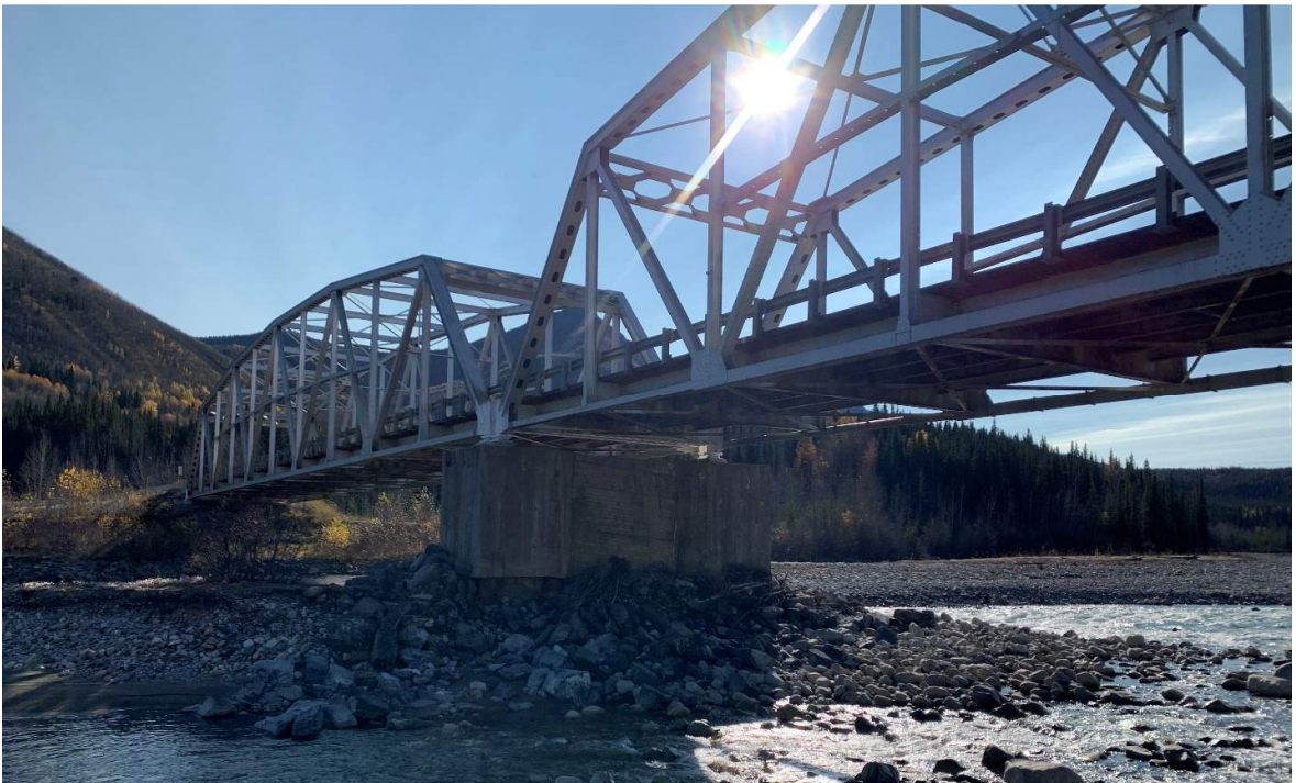
P12 - Side view of existing pier, looking upstream (looking towards Fort Nelson)
