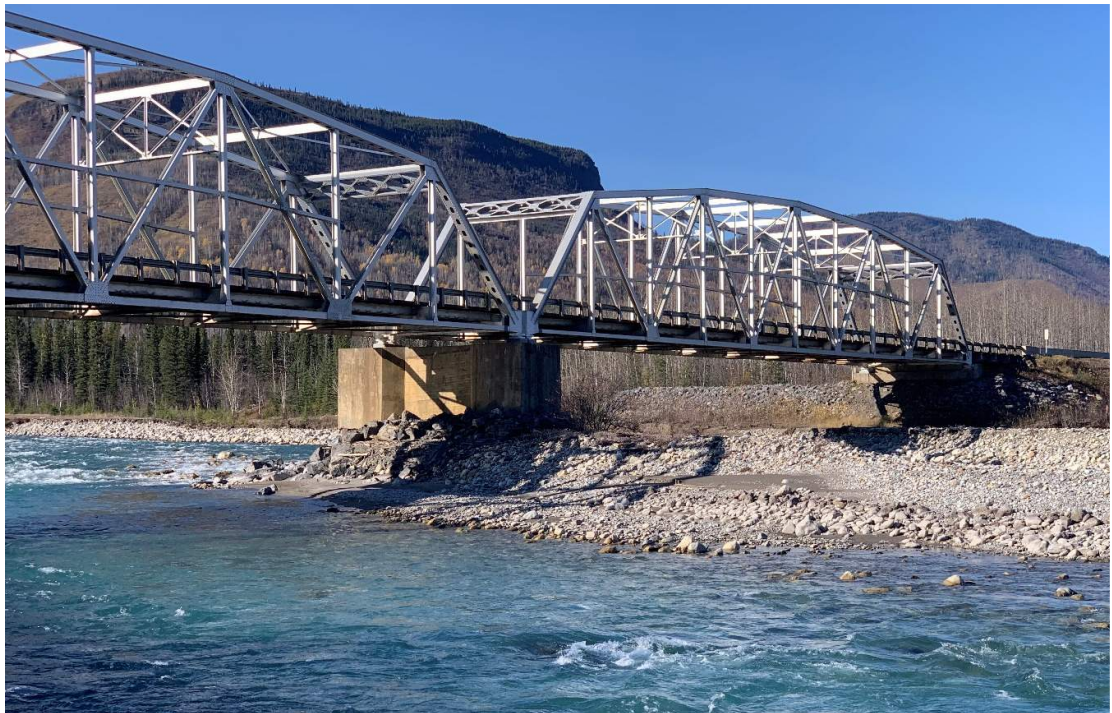
P08 - Side view of existing pier, looking upstream (looking towards Watson Lake)
