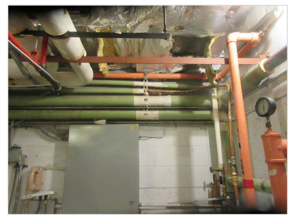
09: SOUTH WEST CORNER OF MECHANICAL ROOM
