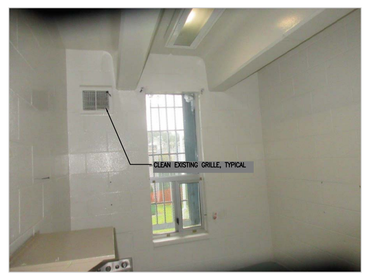
06: TYPICAL CELL CONDITION, TOWARDS WINDOW
