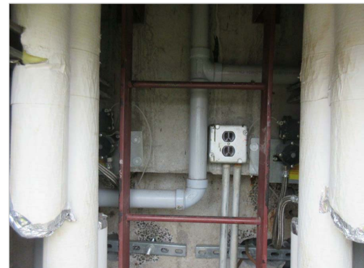
10: TYPICAL VIEW OF EXTERIOR CHASE, BEHIND LOWER ACCESS PANEL
