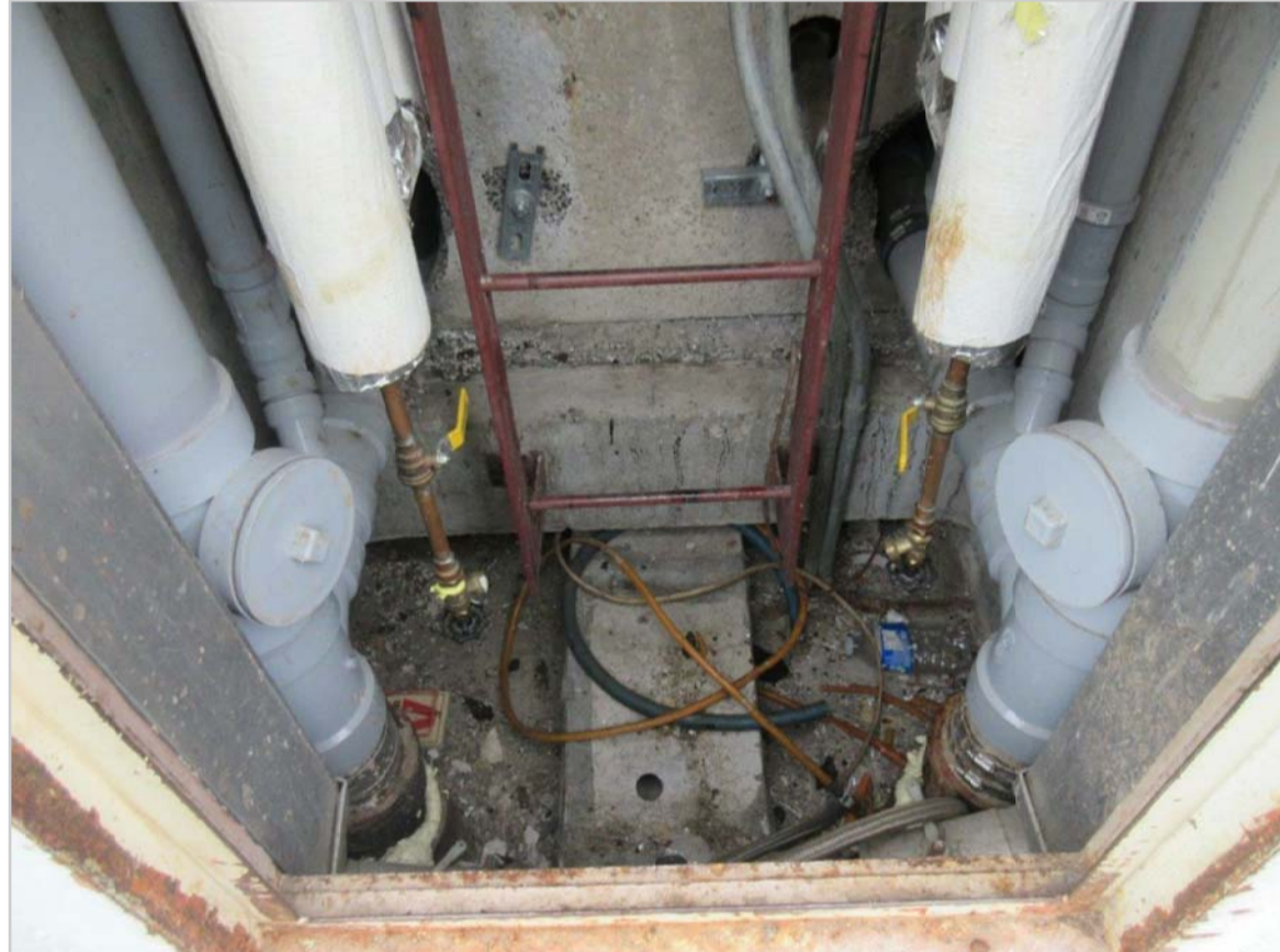
07: TYPICAL CONDITION OF EXTERIOR CHASE BASE, WITHOUT RAIN WATER LEADER
