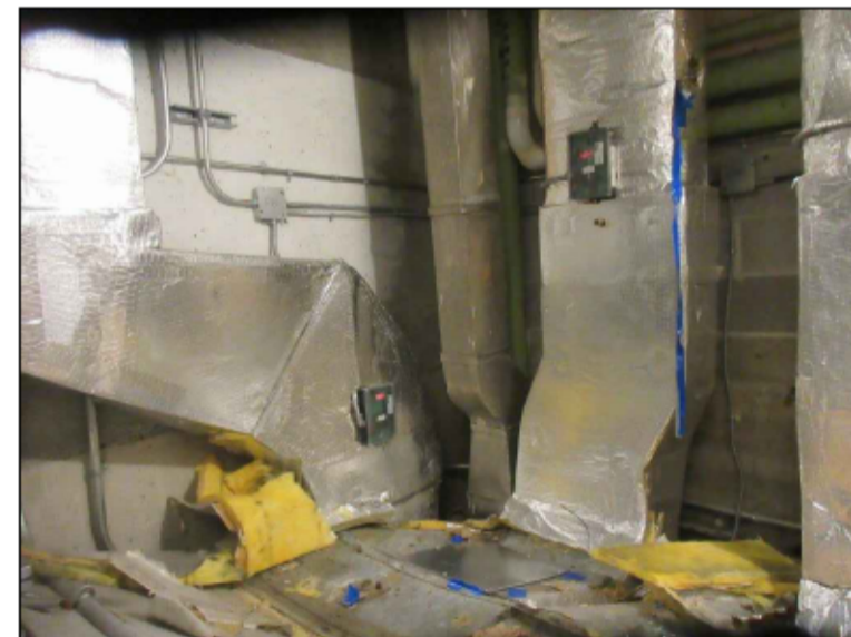
#17 - LU5 - BASEMENT AHU
