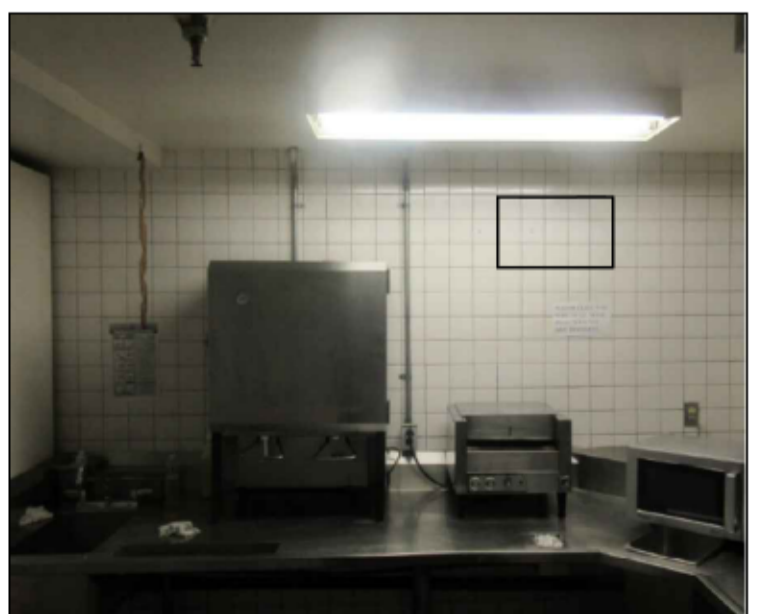
#21 - LU5 - KITCHEN WALL INSIDE - EXHAUST FAN LOCATION
