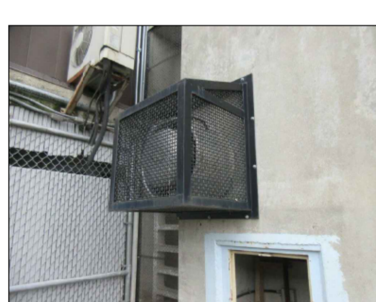
#22 - LU5 - EXAMPLE OF EXHAUST FAN ENCLOSURE
