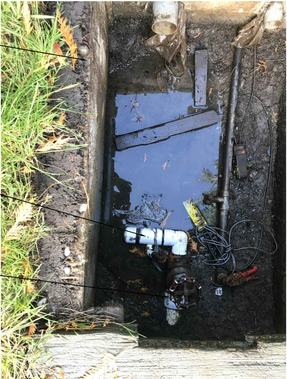
PHOTO: POINT OF CONNECTION
