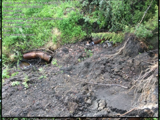
Culvert 21+830: Debris around the culvert (top) and Outlet (bottom)
