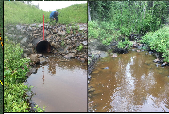
Culvert Ex-4 (SE): 41" Diameter / Pool at mouth / Downstream side / Silt, boulder, cobble, gravel substrate
