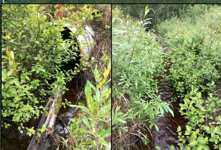
Culvert Ex-10 (NW): 48" Diameter / Perched 12" / Upstream side / Boulder and gravel substrate
