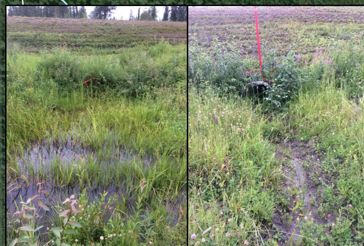
Culvert Ex-3: The culvert drains a wetland area upstream with no defined channel
