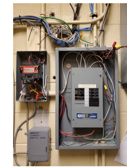
5 PANEL 'C' EXTERIOR LIGHTING CONTACTOR AND TIME CLOCK E2.1 NOT TO SCALE
