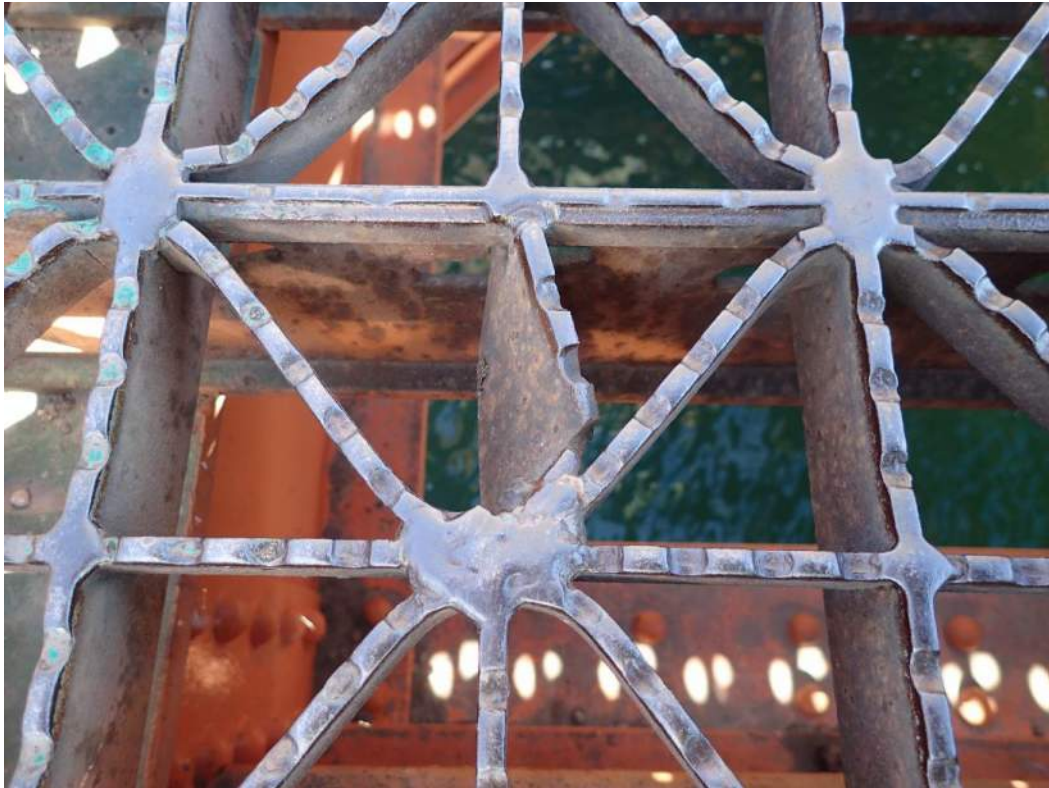
Photo 11: Typical warped grating members
