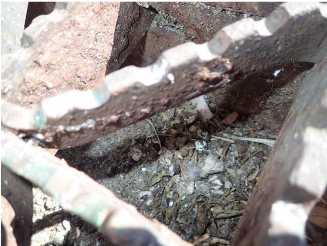
Photo 26: Debris – typical - mostly at end panels (A, C, D, F)
