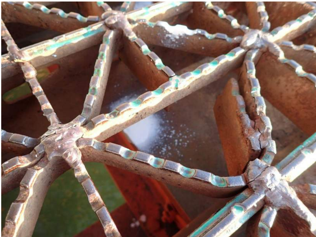
Photo 12: Typical broken grating members
