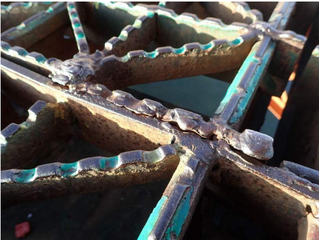
Photo 22: Previous Welding Repairs – typical example of failure between panels
