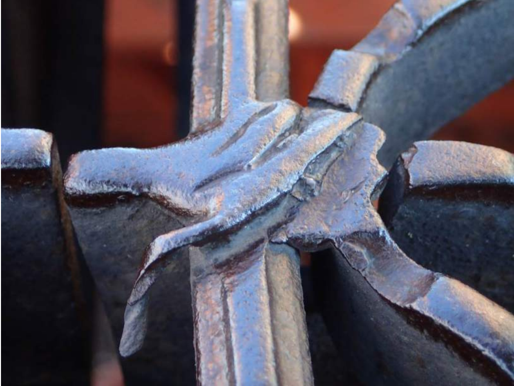
Photo 21: Previous Welding Repairs – typical example of failure at Repaired Button Weld
