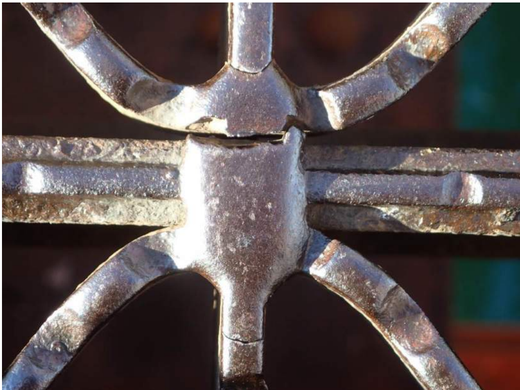
Photo 18: LGF detail – BW crack, full depth, complete connection failure
