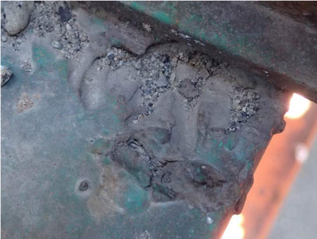
Photo 9: M-beam to stringer fillet weld deterioration and damage to stringer's flange
