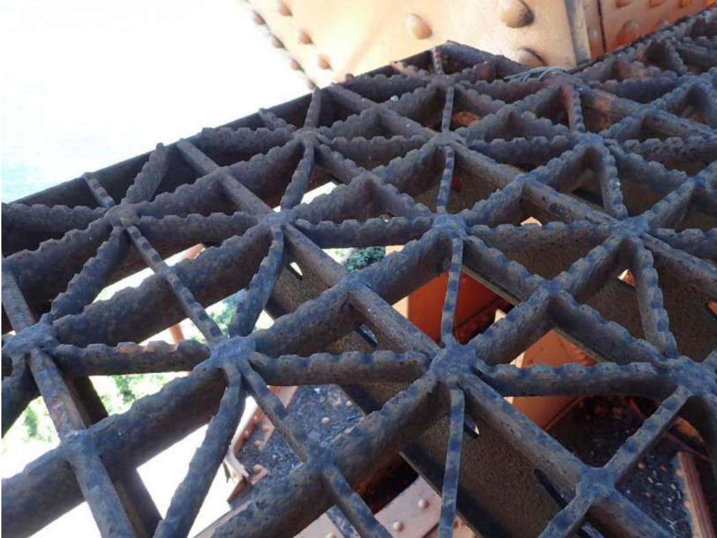
Photo 23: Surface rust on panels – mostly outside of traffic load zone
