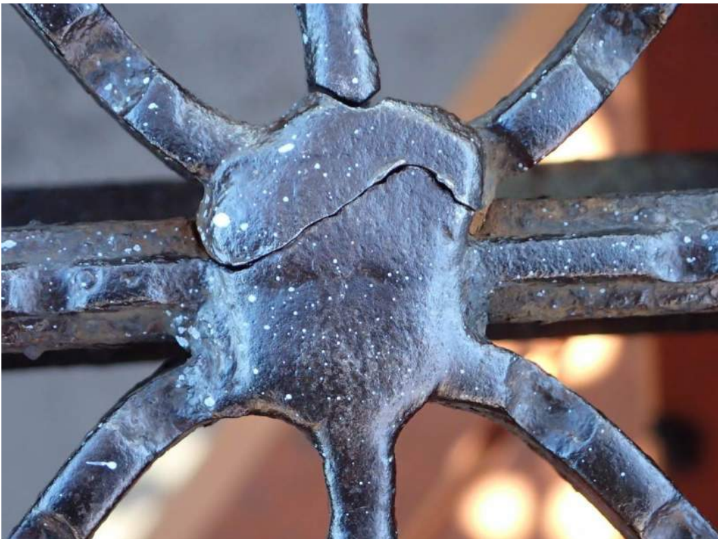
Photo 8: BW crack – typical example
