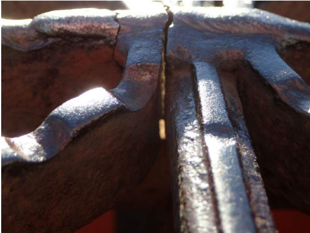
Photo 19: LGF detail – BW crack, full depth, complete connection failure
