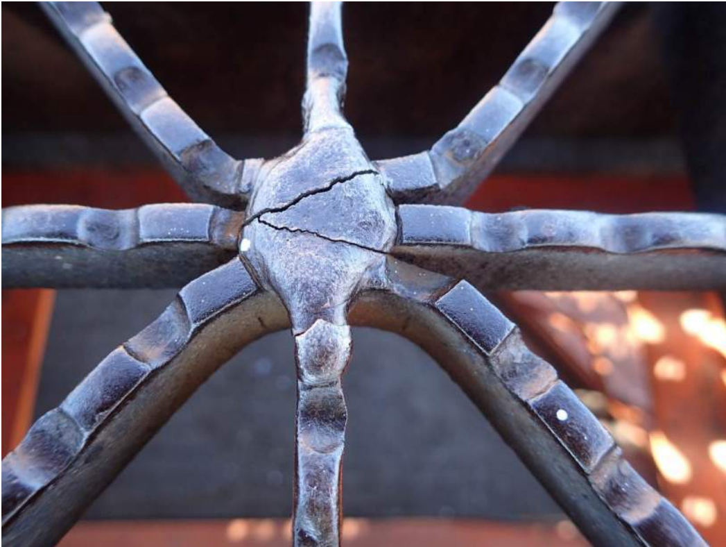
Photo7: Button Weld crack – typical example
