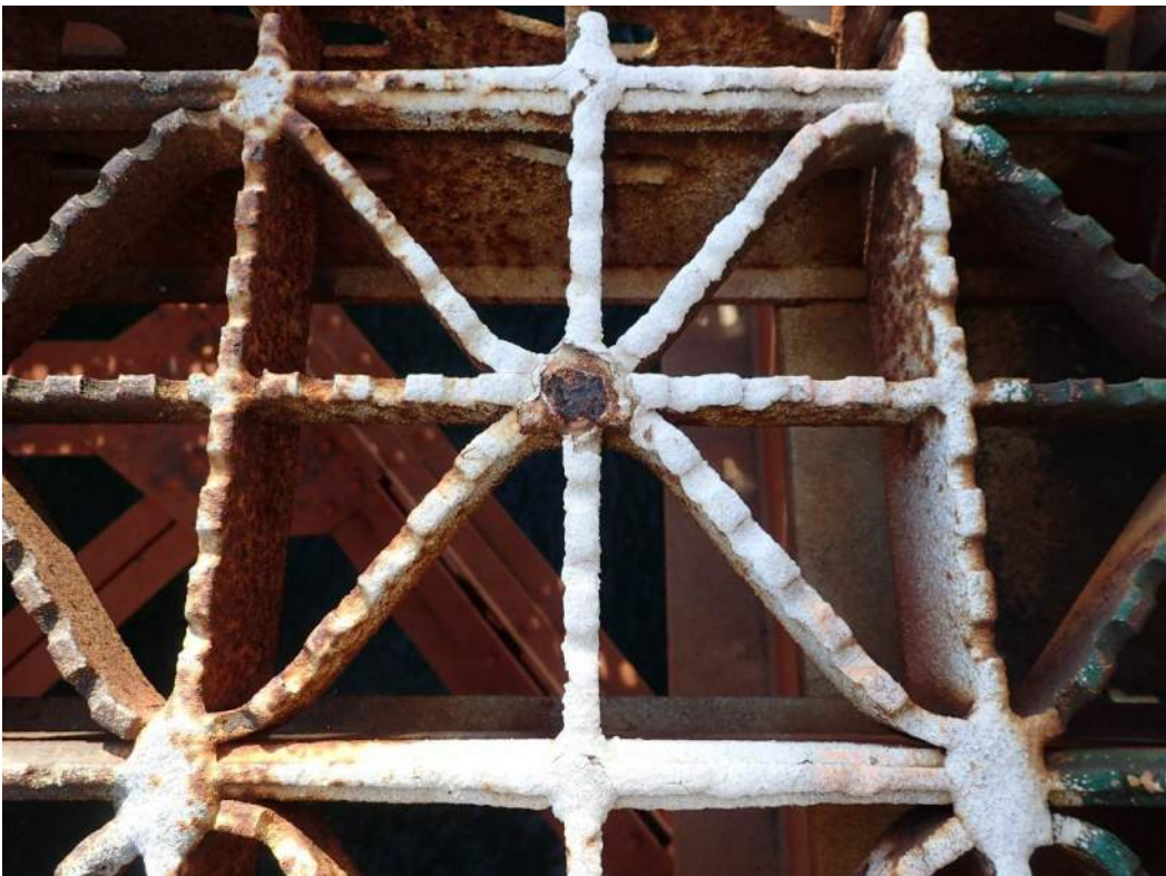
Photo 24: Surface rust on panels – paint facilitates corrosion of Button Welds
