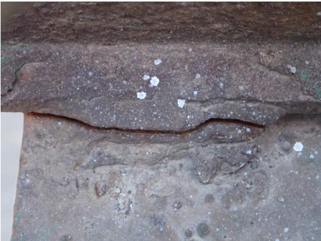
Photo 10: M-beam to stringer fillet weld – typical crack, full length and depth
