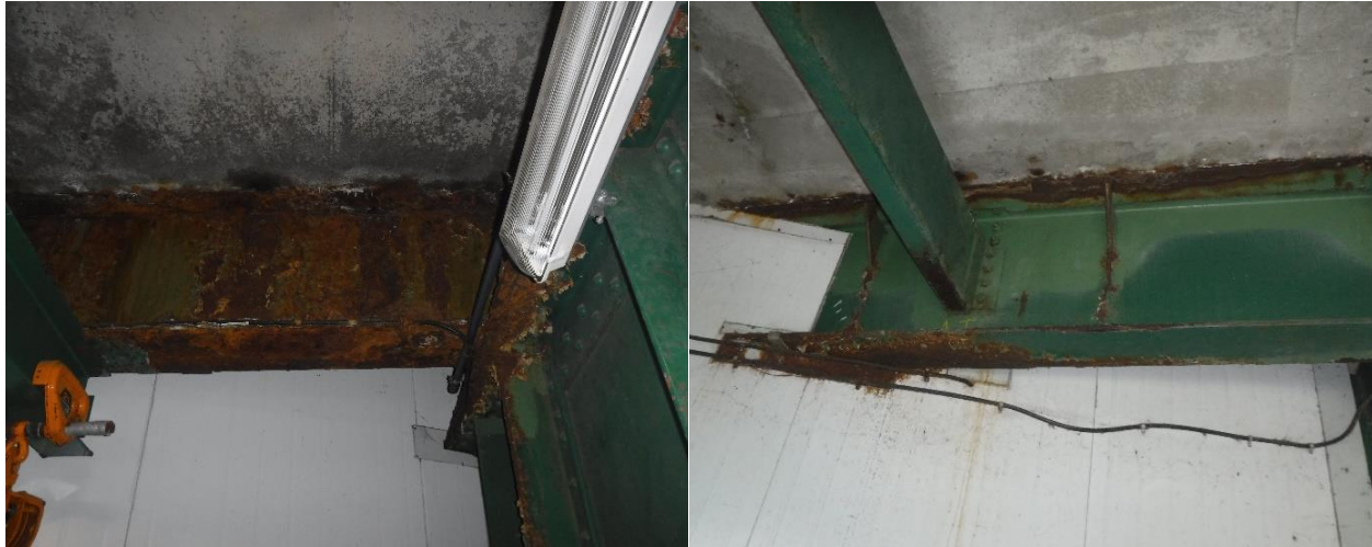
Inside the Span Lock Room
