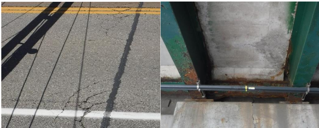
Typical Paved over Joint
