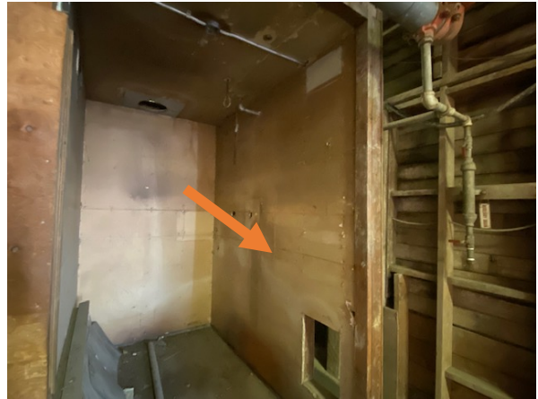
Asbestos cement board behind drywall
