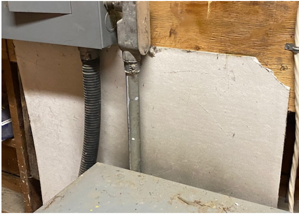
Asbestos fiber board behind panel in electrical room
