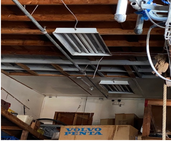
Tube lighting in storage rooms
