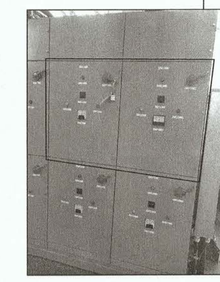
PARTIAL VIEW OF EXISTING MCC
