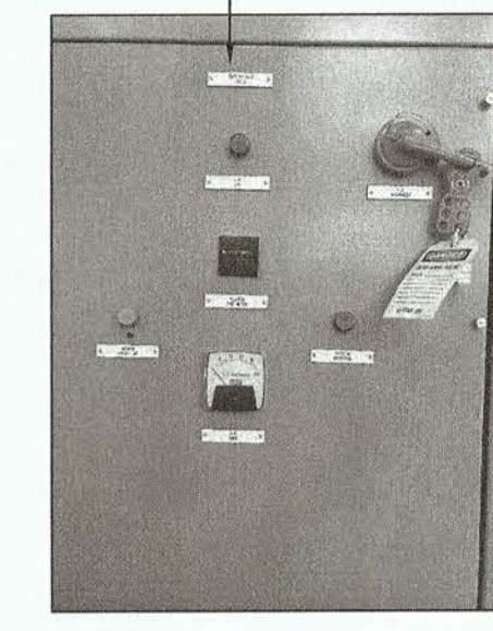
EXISTING DISCONNECT FOR CAPSTAN NO. 2
