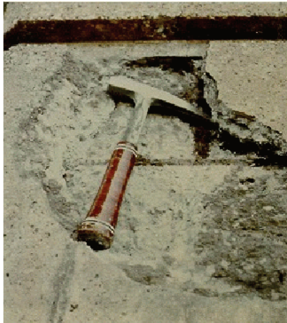
Figure 2.2.6(b) Severe Localized Spalling
