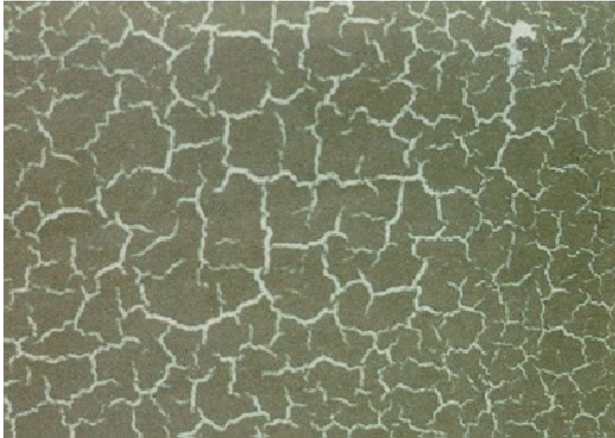
Figure 2.8.1(c) Alligatoring (typical mud crack pattern)
