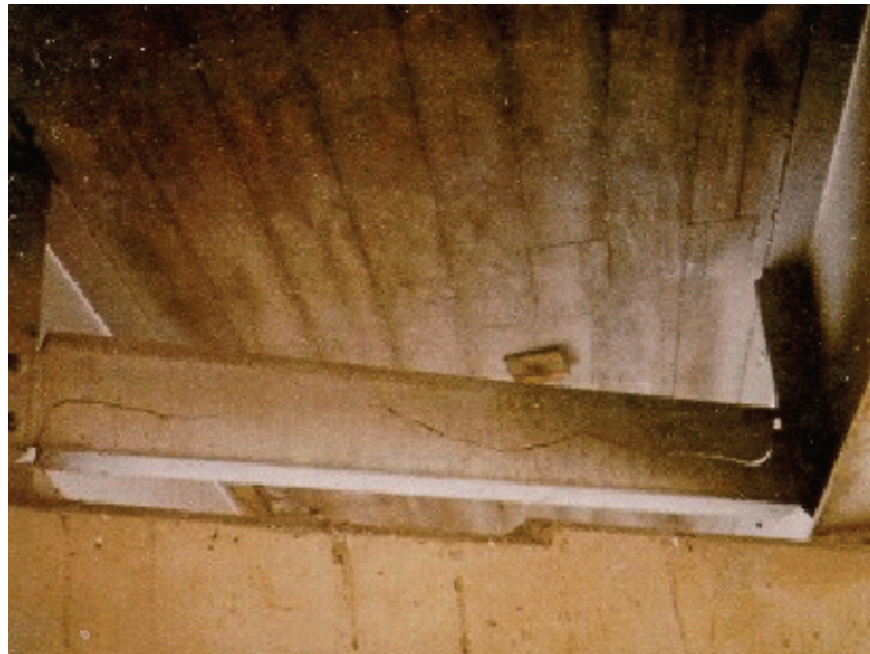
Figure 2.3.3(a) Very Wide Cracks in a Diaphragm
