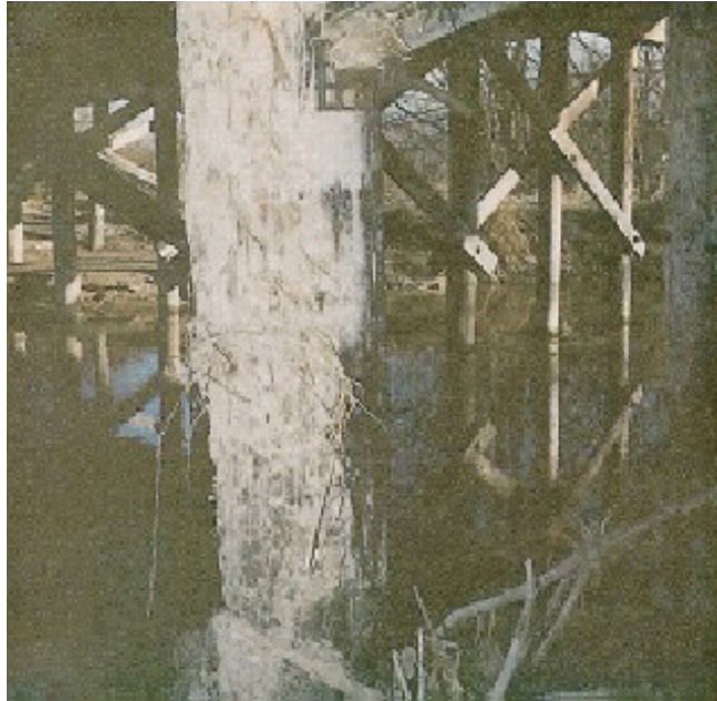
Figure 2.4.4(b) Very Severe Abrasion on a Wood Pile Due to Ice
