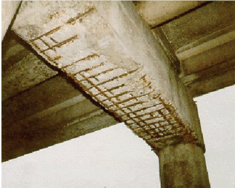
Figure 2.2.6(a) Very Severe Spalling in a Concrete Pier Cap due to Corrosion of Reinforcement
