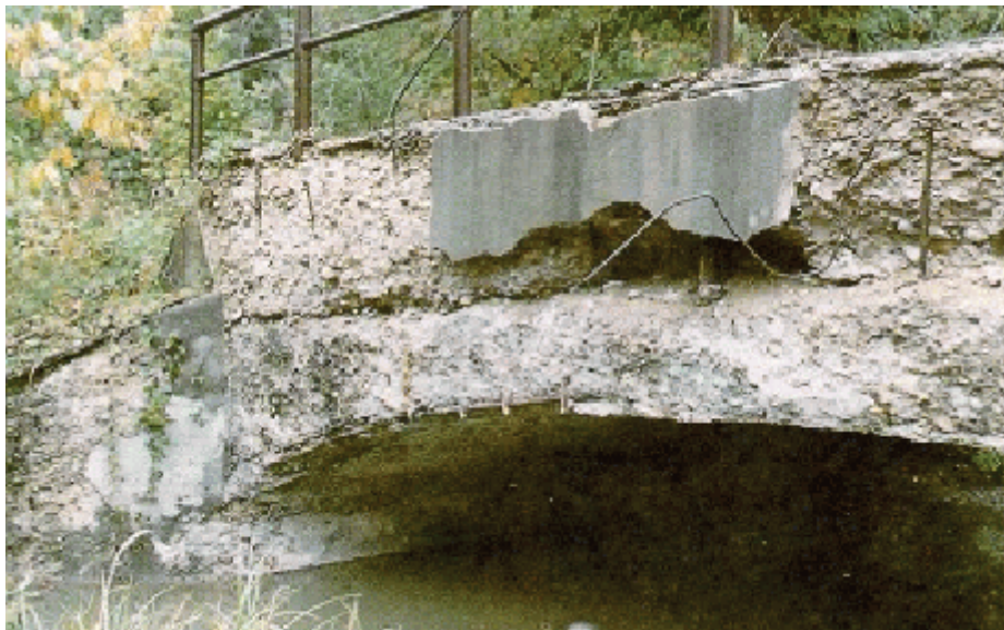
Figure 2.2.2 Very Severe Disintegration of the Outer Surface of Concrete
