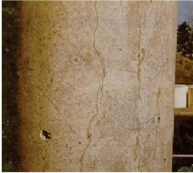
Figure 2.2.7(e) Medium cracks due to Corrosion of Reinforcement
