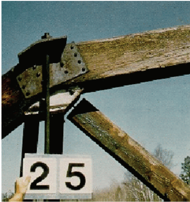
Figure 2.4.7 Loose Connection in Wood (25 mm gap measured)
