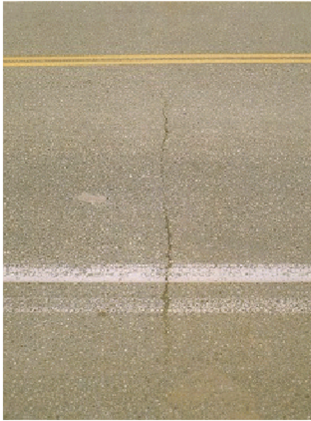
Figure 2.7.1(b) Medium Transverse Crack
