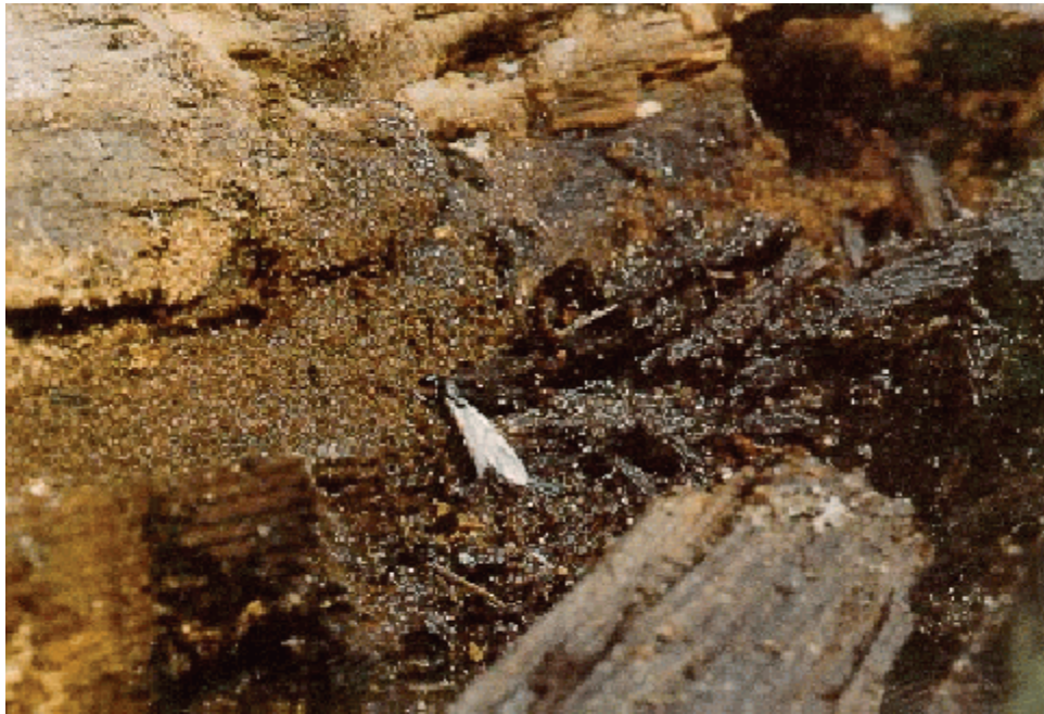
Figure 2.4.3(b) Very Severe Insect Damage in Wood
