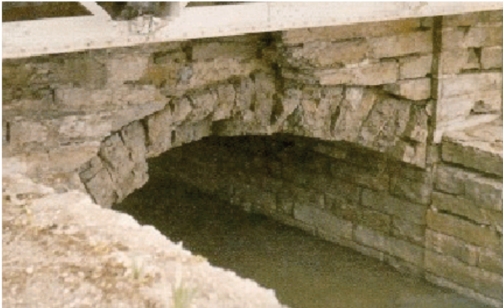
Figure 2.5.3 Very Severe Loss of Mortar and Stone in a Masonry Arch
