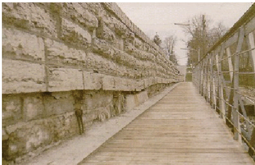
Figure 2.5.2 Very Severe Splitting, Spalling and Deterioration in Masonry
