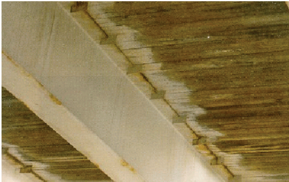
Figure 2.4.6(b) Light Chemical Damage on Underside of a Wood Deck
