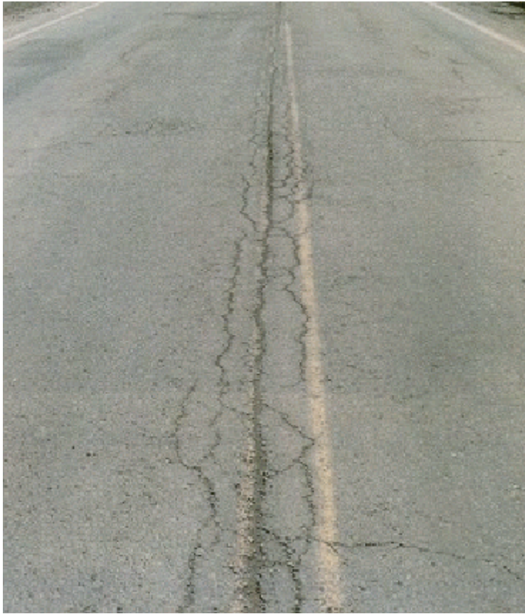
Figure 2.7.1(a) Medium Longitudinal Crack
