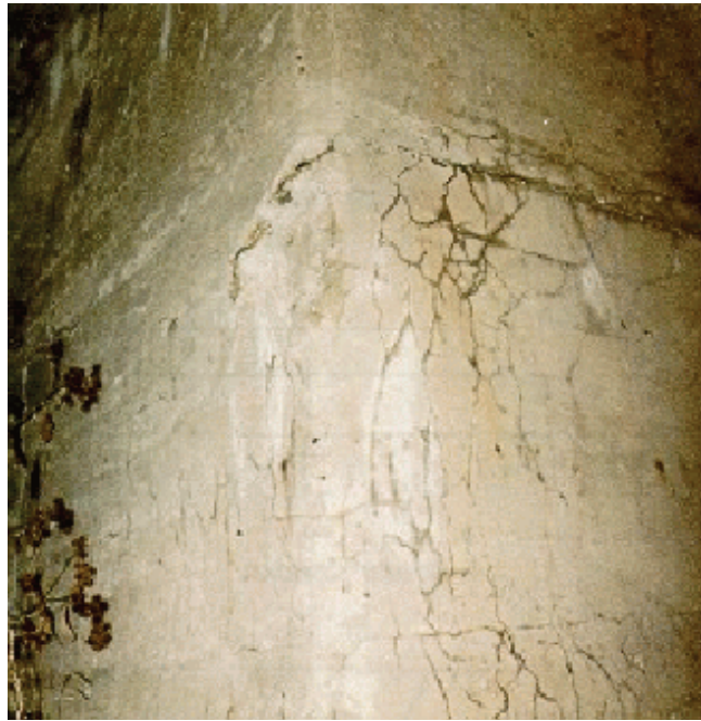
Figure 2.2.7(c) Medium Pattern Cracks in an Abutment
