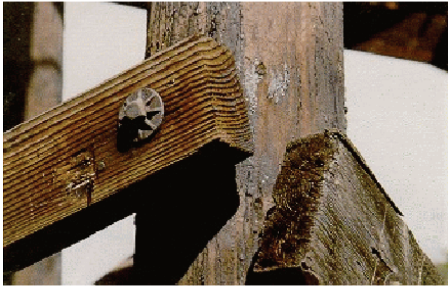
Figure 2.4.1(a) Light Weathering in Wood Members
