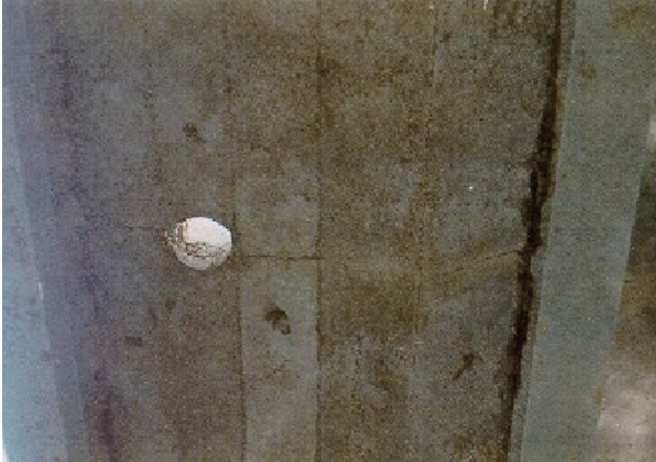
Figure A7.1.2(m) Deck Drain (Hole in Deck)
