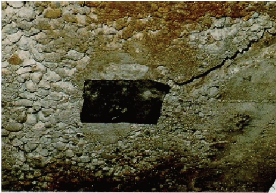
Figure 2.2.9 Severe Honeycombing on the Underside of a Deck Slab
