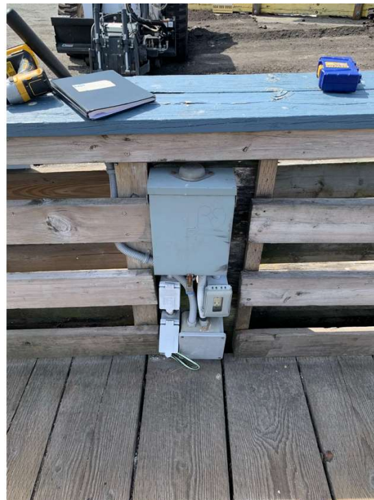
Potential Utility and Handrail Interference with Stringer Replacement
