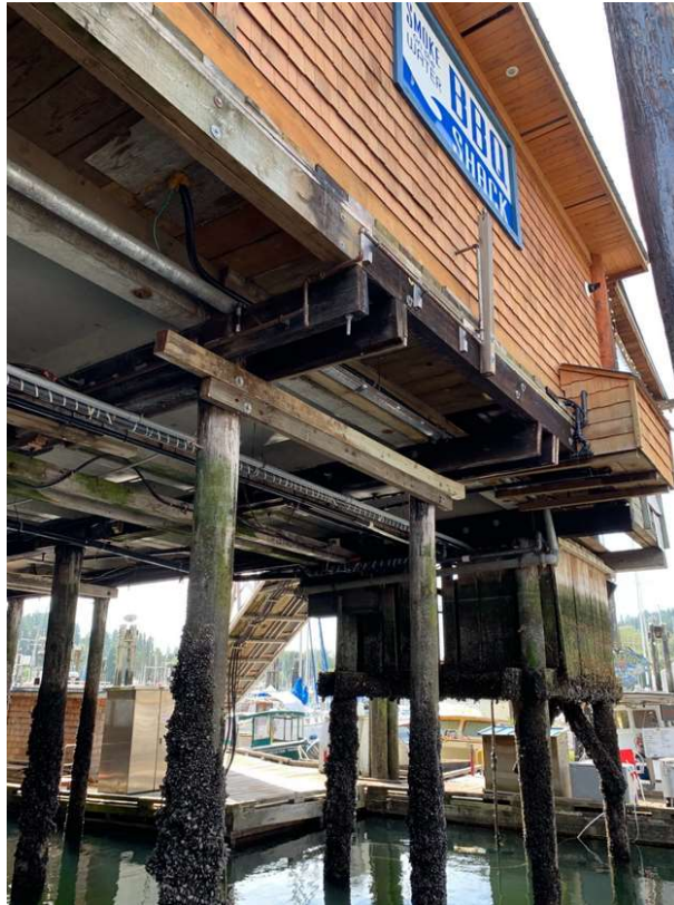
Utilities Interference for Cap Replacements (run under caps and secured to panels)
