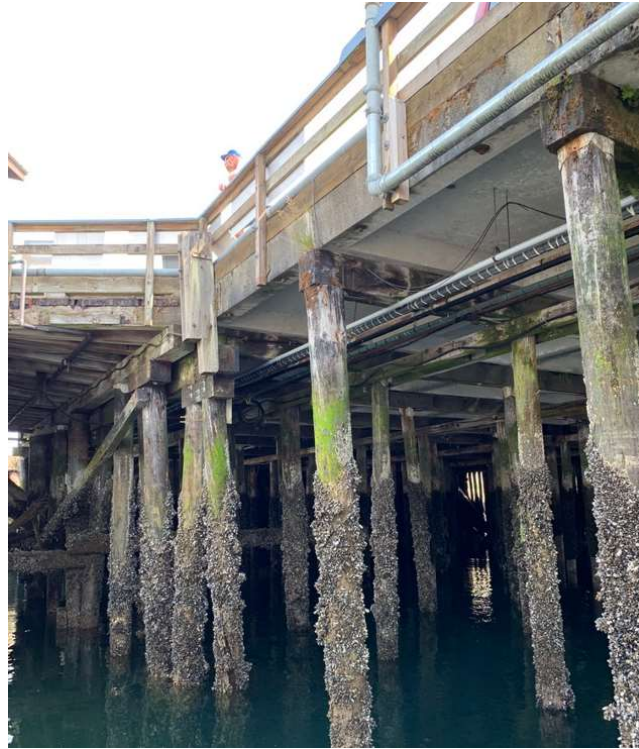
Utilities Interference for Cap Replacements (run under caps and secured to panels)
