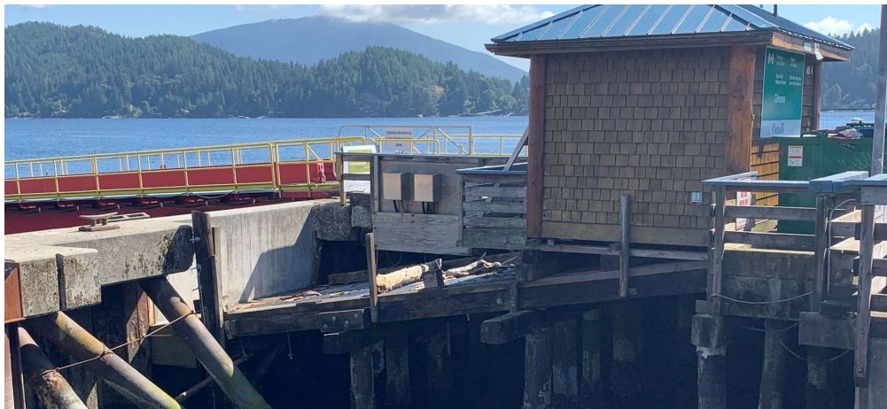
Handrail Interference (Note: shed, sloped timber structure and junction boxes to be removed by others)
