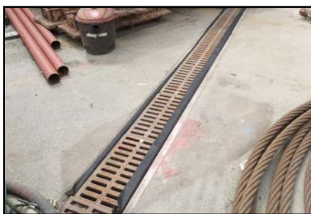
Prevent deleterious substances entering marine environment by placing filter cloth in the trench drains.
