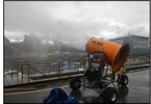
Dust suppression unit in operation.
