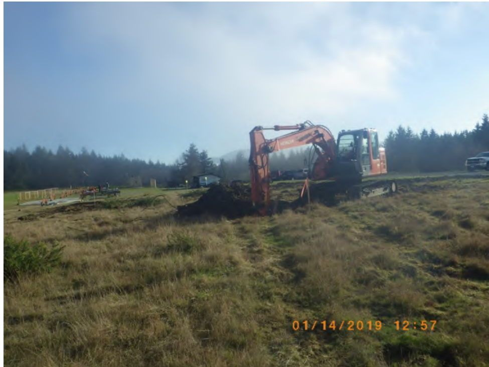
Photograph 3: Looking east at TP19-49. The PDQ hut and playing field are visible further east.
