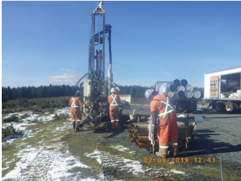
Photograph 5: Looking west during drilling of BH19-08D. The gravel parking lot is visible on the right.
