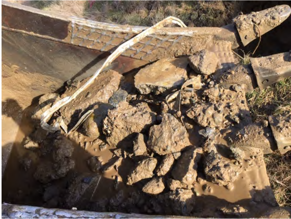
Photograph 5: View of concrete debris.
