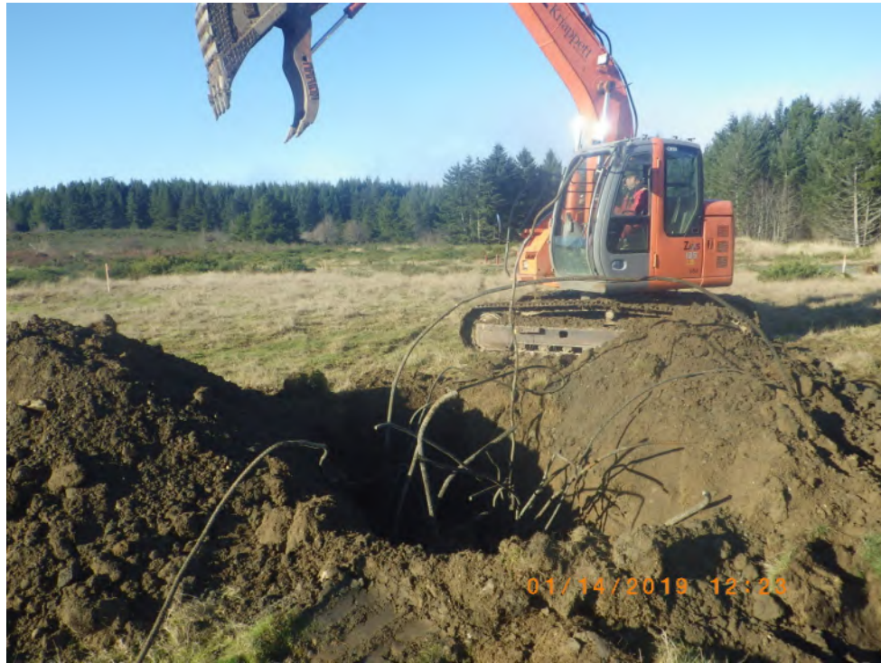
Photograph 1: Looking northwest at TP19-50. Rebar encountered in the debris unit is visible in the test hole.
