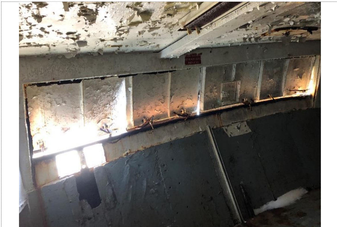
14. Aft fantail area – doors not properly closed
