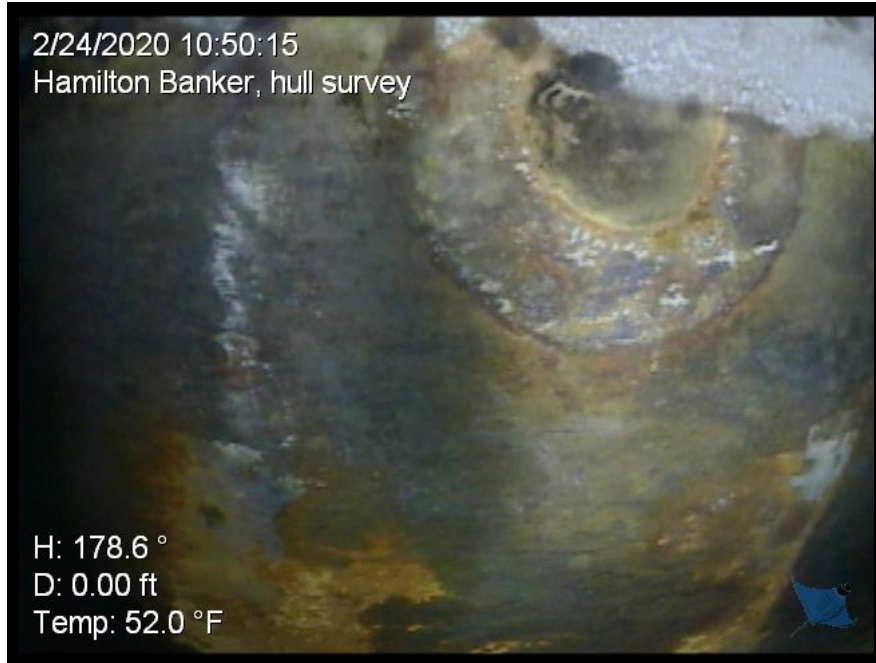
Figure 5 - Starboard side hull penetration.
