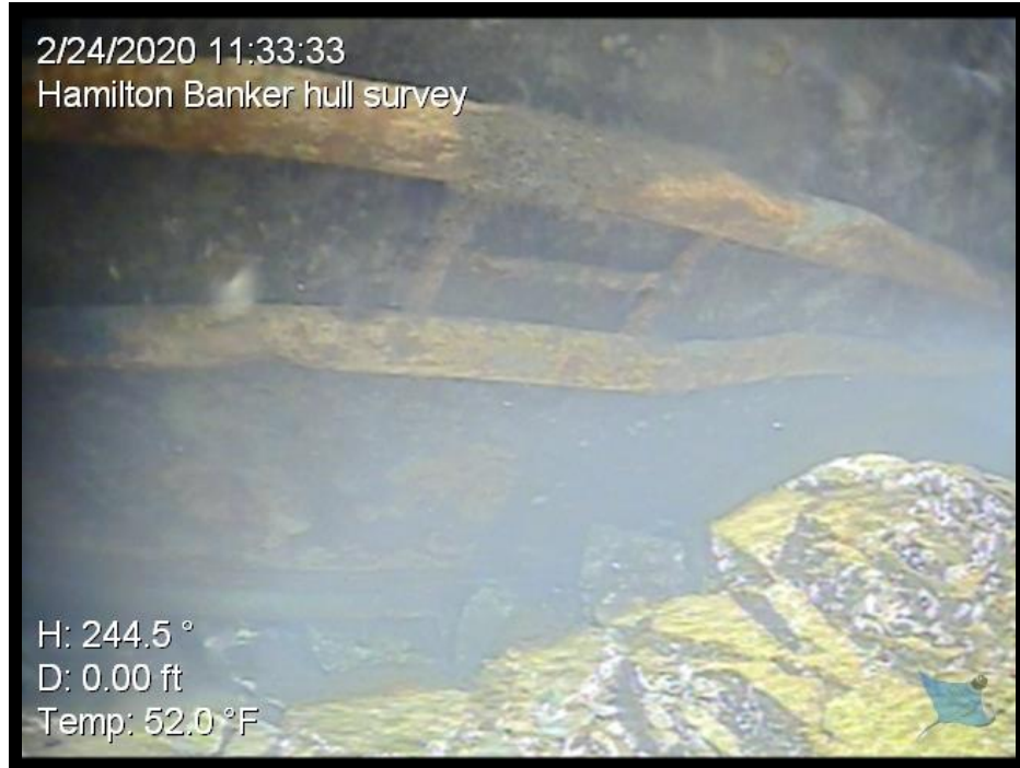
Figure 11 - Missing bilge keel area on port side.
