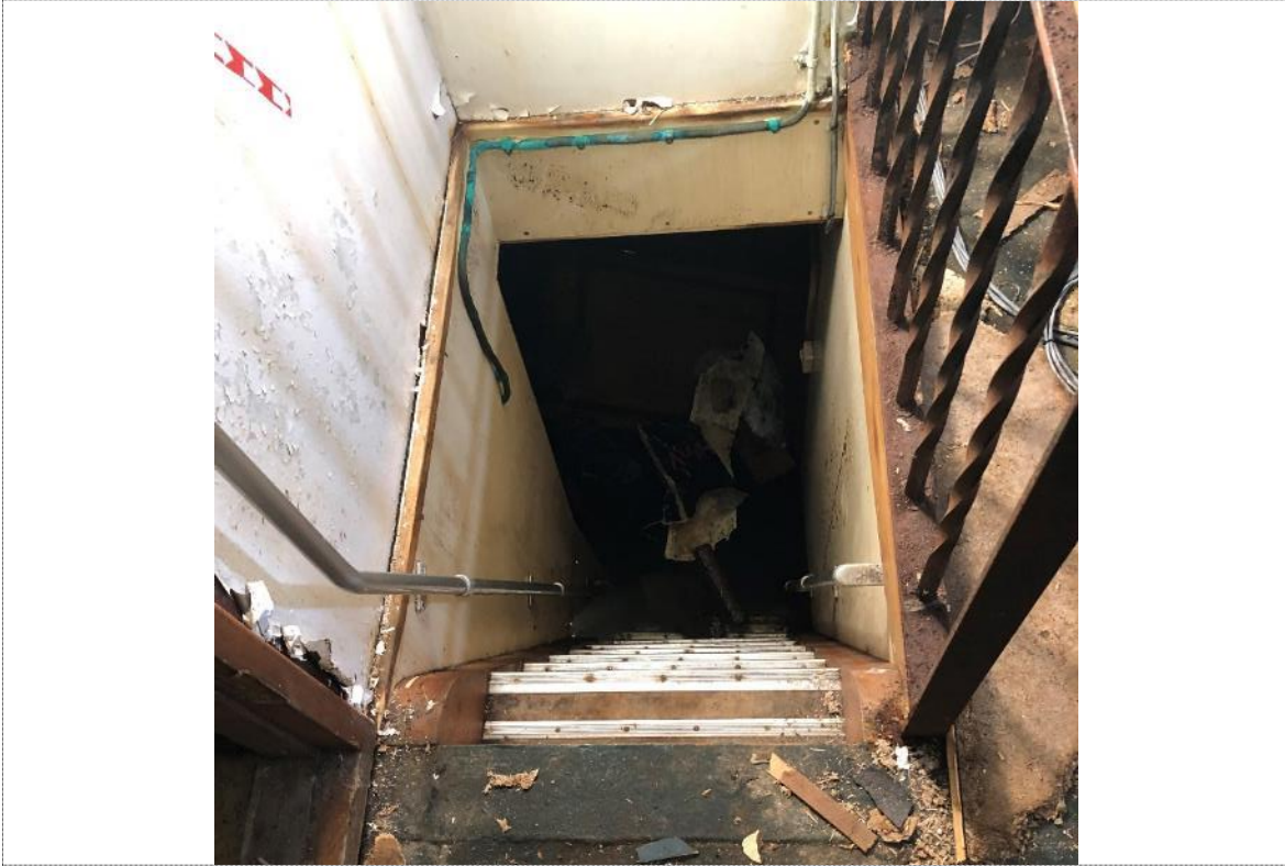
11. Access to bunk room – flooded with floating debris
