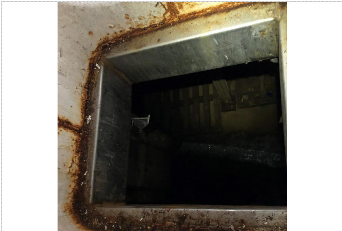
20. Processing deck – view of cargo space through hatch - flooded
