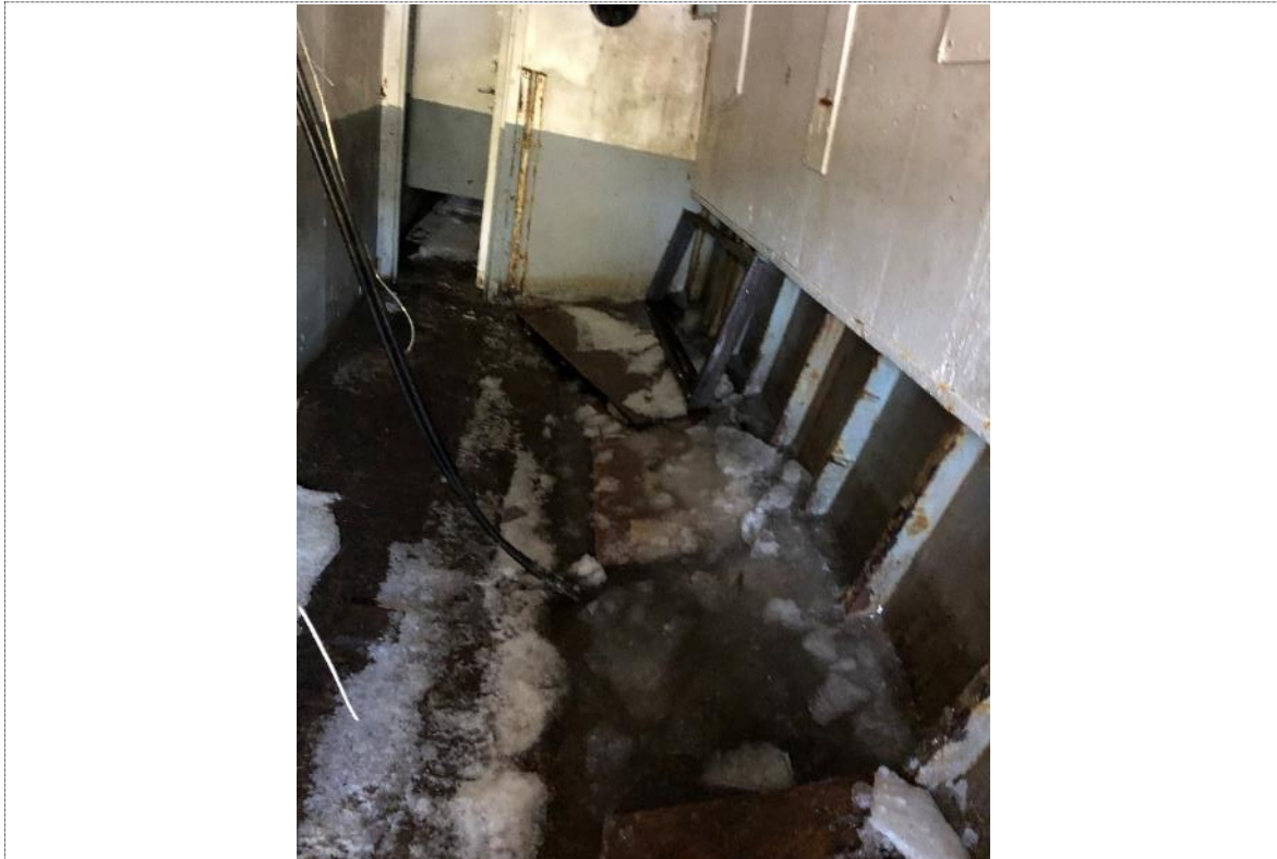
13. Starboard access to fantail area – flood water against sidewall
