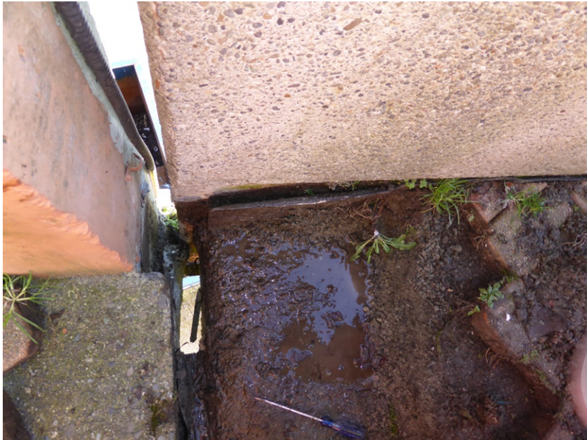
Photo 4: Test #4 located at the joint between the cantilever slab and the exterior stairs.
