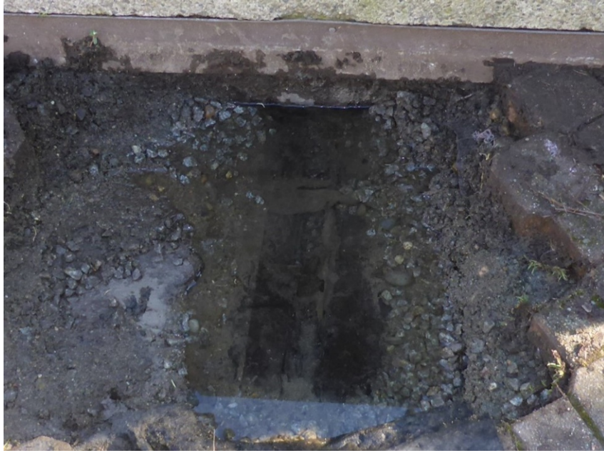
Photo 3: Test #3 at an expansion joint in the cantilever slab. 40 mm deep water ponding
