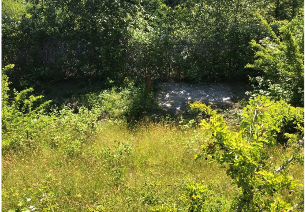
Photograph 5: Excavation 1b, facing east down the slope with fenceline beyond the monitoring well.
