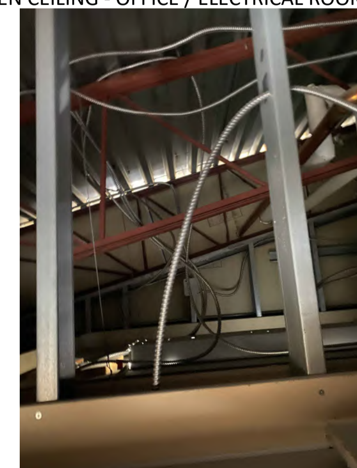
A18 PLAN - ENTRE-PLAFOND - SALLE DE PAUSE / COULOIR PLAN - BETWEEN CEILING - BREAK ROOM / CORRIDOR
